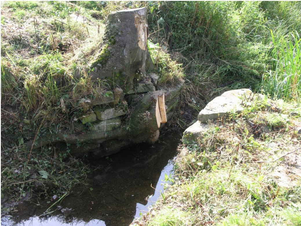
Plate2: General view of eastern side of sluice showing root damage.
