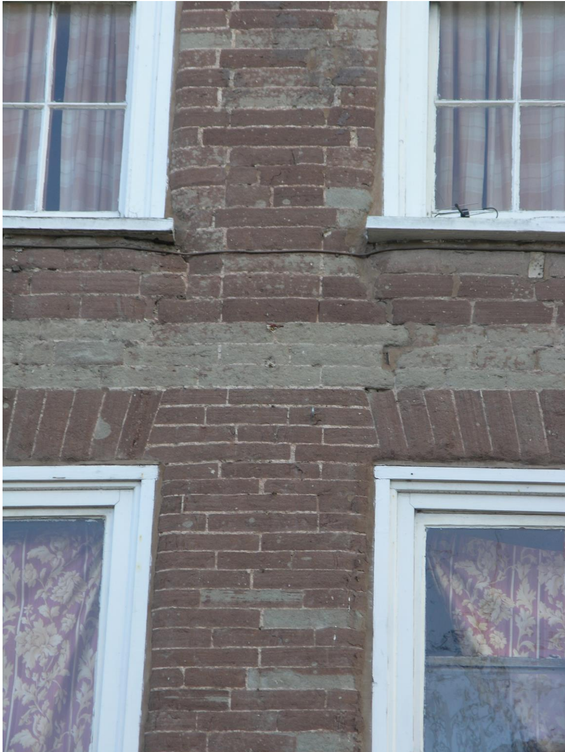
Fig.10 36 Broad Street: detail of the sandstone blocks (with polychrome band) cut to brick-like dimensions
