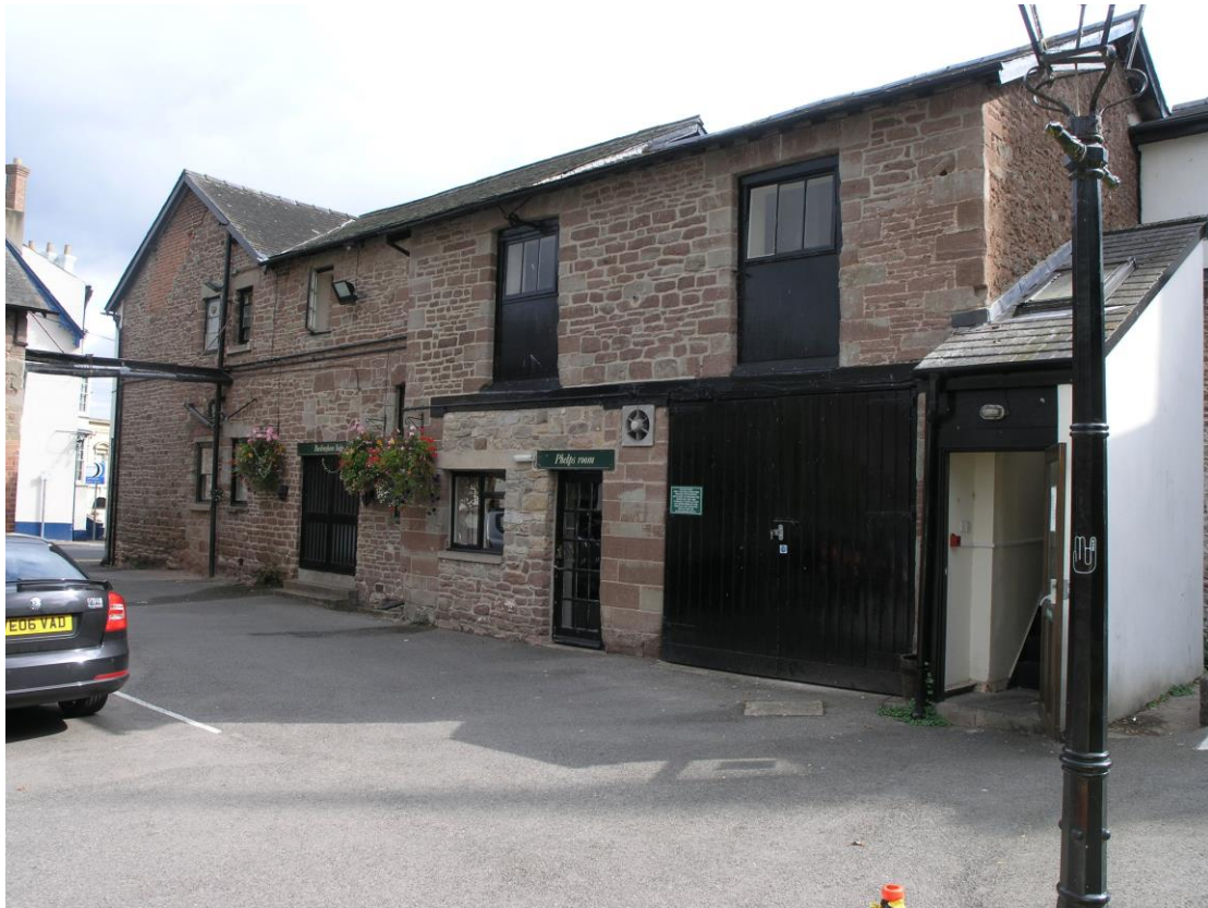
Fig.15 The Royal Hotel, south-east range with blocked features in its rear (courtyard) elevation
