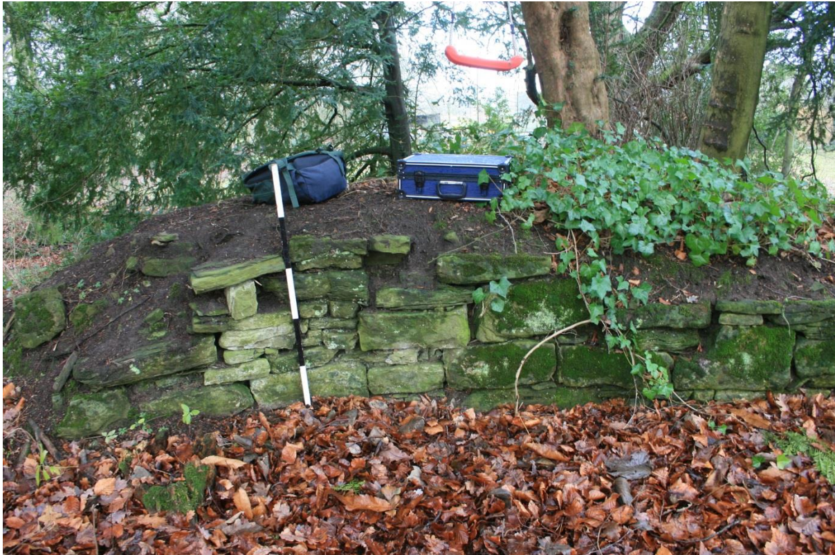
7. The north-east angle of the inner bailey curtain wall showing probably original coursed masonry; the one-metre scale marks the angle
