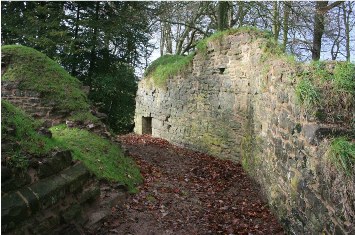
3. The north side of the keep with battered base and plinth, looking west
