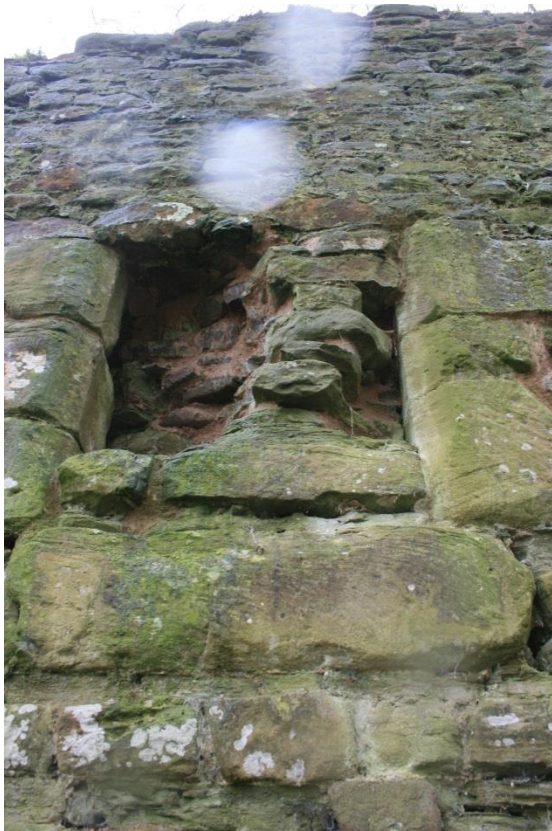
14. Detail of the exterior face of the blocked door in the curtain wall
