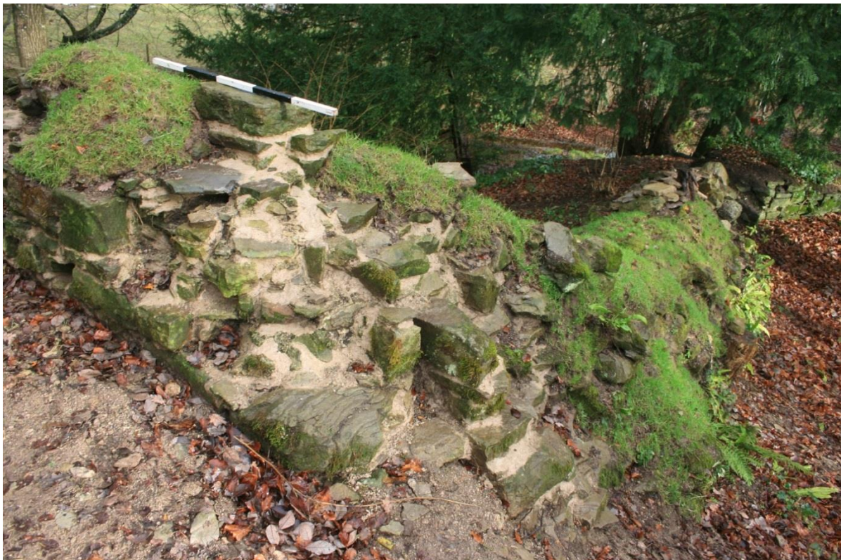
8. Thickening-up of the inside face of the curtain wall at its turn north around the keep
