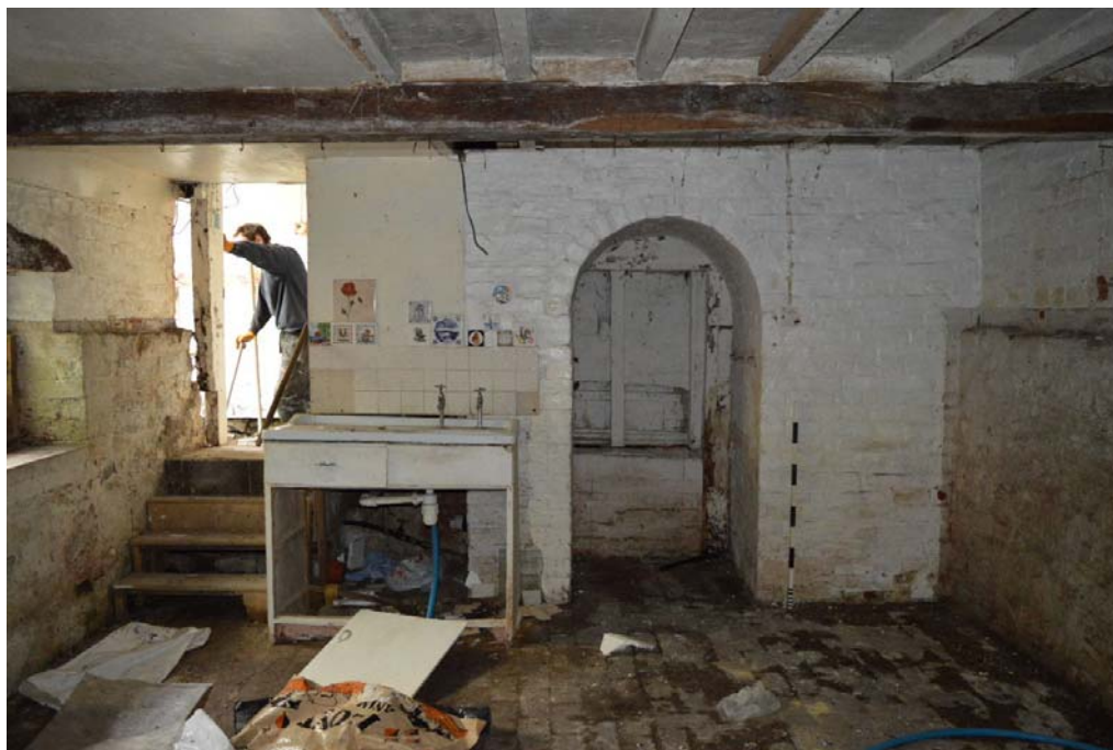
Fig. 10 The blocked original doorway from the cellar, viewed from the north-west. Photo CPAT 3888-0013
