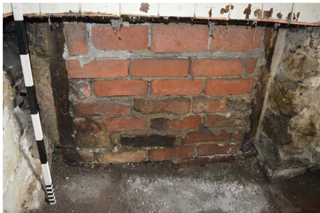
Fig. 9 The blocked original doorway to the 19 th -century school room in the cellar, viewed from the south-east. Photo CPAT 3888-0007
