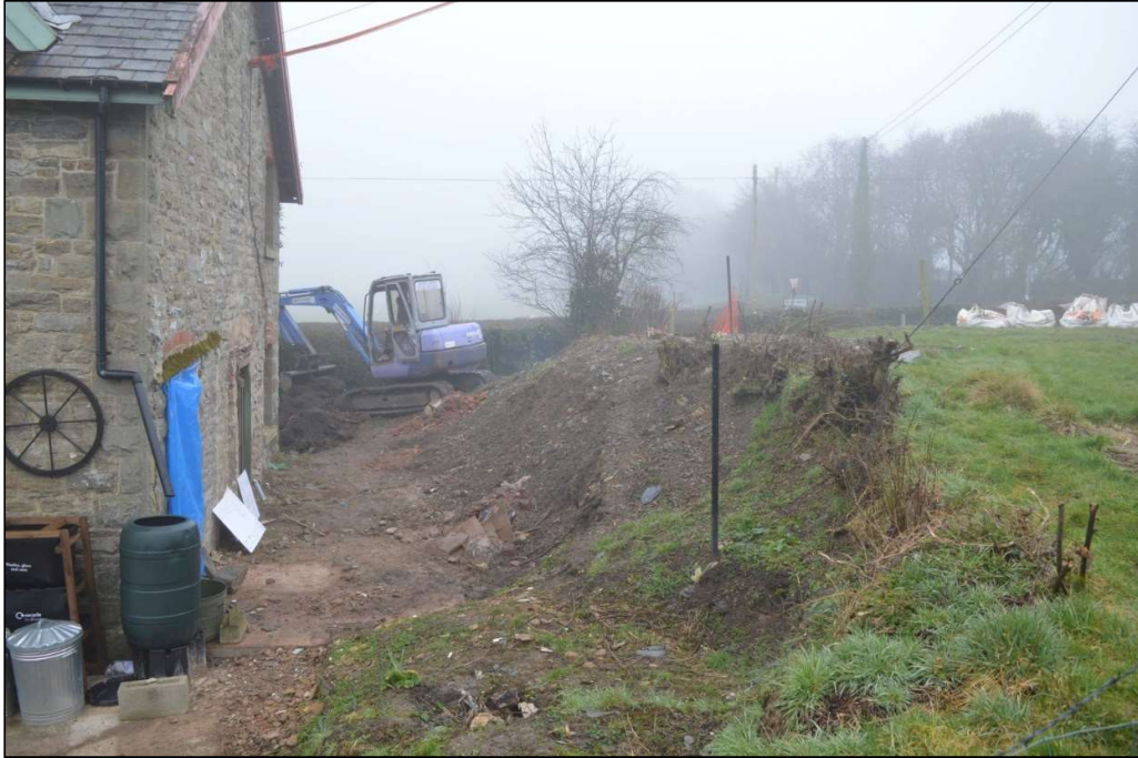
Fig. 6: The area of the extension prior to machining, from the east. CPAT 4898-0001
