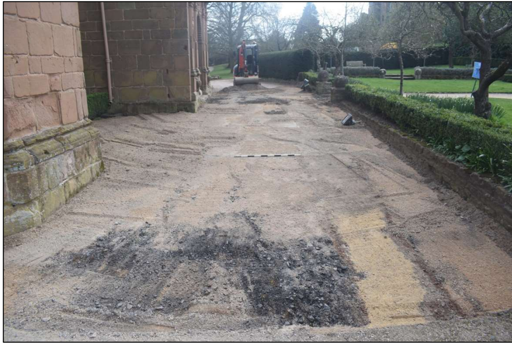
Fig. 4 Groundworks to the west of Leicester's Gatehouse viewed from the north Photo CPAT 4915-023
