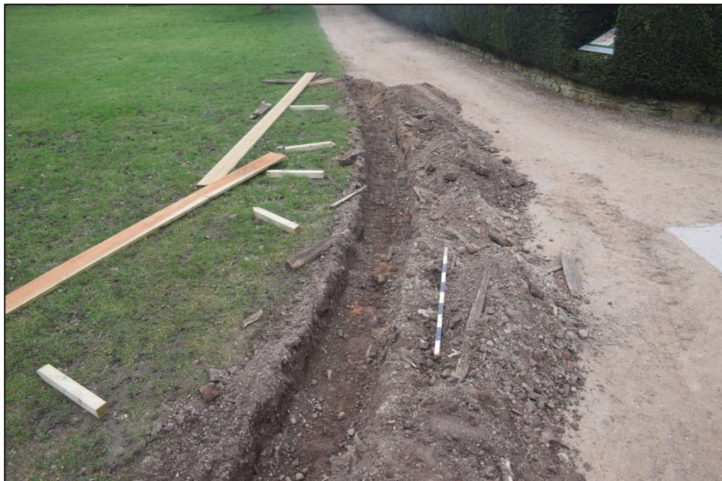
Fig. 3 Trench excavated for edging boards between Leicester's Gatehouse and the gardens, viewed from the east. Photo CPAT 4915-009
