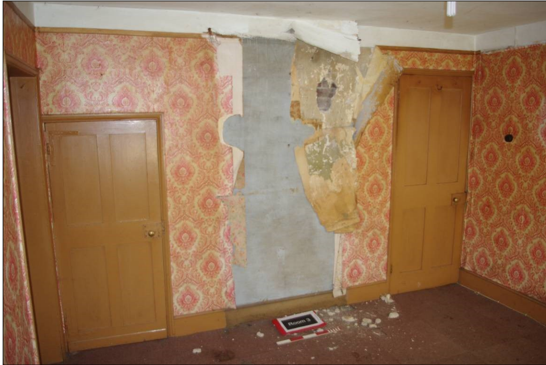
Figure 8. North wall of Room 3. Left hand door to under-stairs cupboard, right door to Room 2, hallway.
