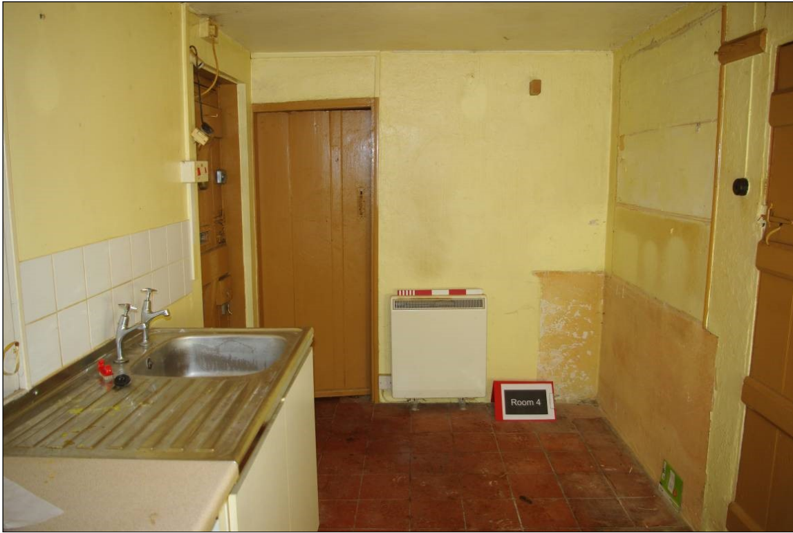
Figure 13. North wall of Room 4, with door to exterior on left, door to Room 5 in centre, door to Room 3 on right. Note traces of where dresser stood to right.
