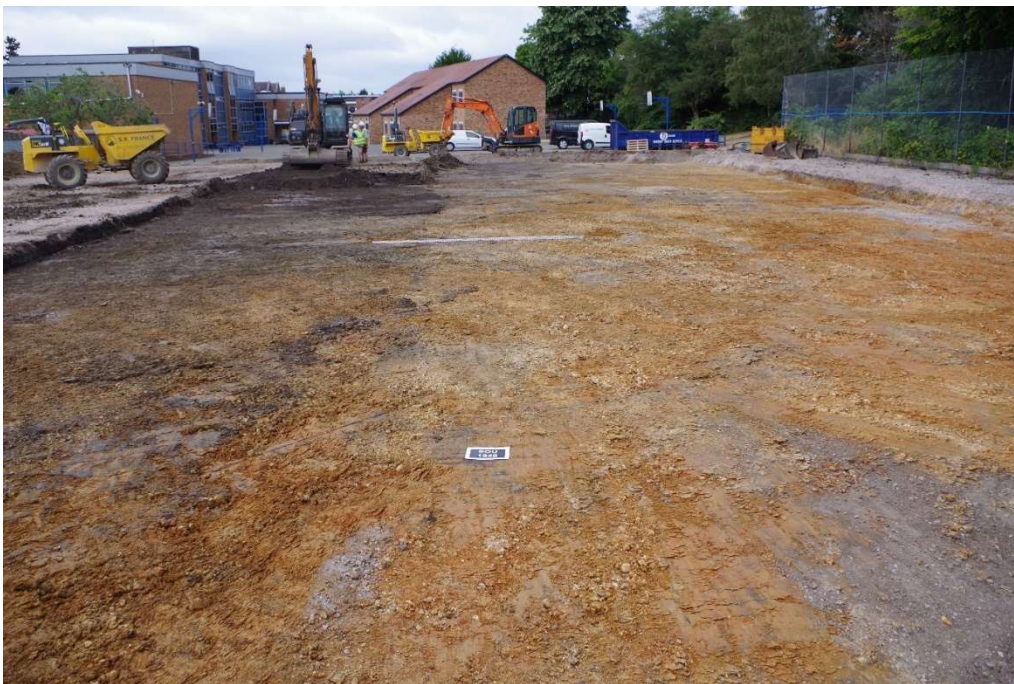
Figure 6. View looking west across the site during early stages of the level reduction. The centre and right of the photo shows the lower part of the River Terrace 6 to 7 gravel (context 3) thinning out to the south (left), where the top of the Wittering Formation (context 2) is being exposed by removal of the topsoil.
