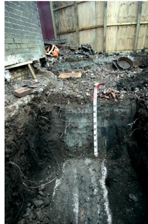
Trench for earlier concrete foundation (note no sign that the foundation had previously been built on)
