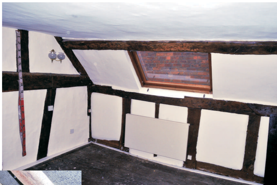
Front bedroom - view facing west - note notching of wall plate for former dormer window
