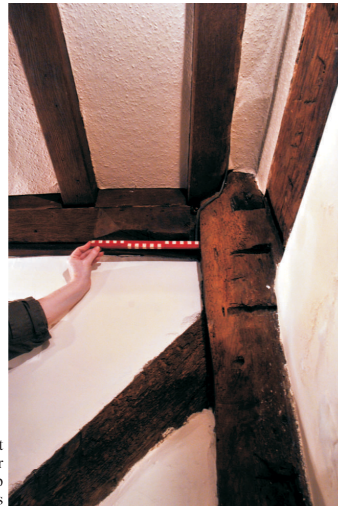
Detail of eastern storey post of Truss 2 - note the two redundant mortices representing a mid rail (lower mortice) and probable tension brace (above) - these prove that there was originally no doorway opening between Bay 1 and 2 at ground floor - two pairs of peg holes at mid rail level disprove any original link to Building 2 at this point
