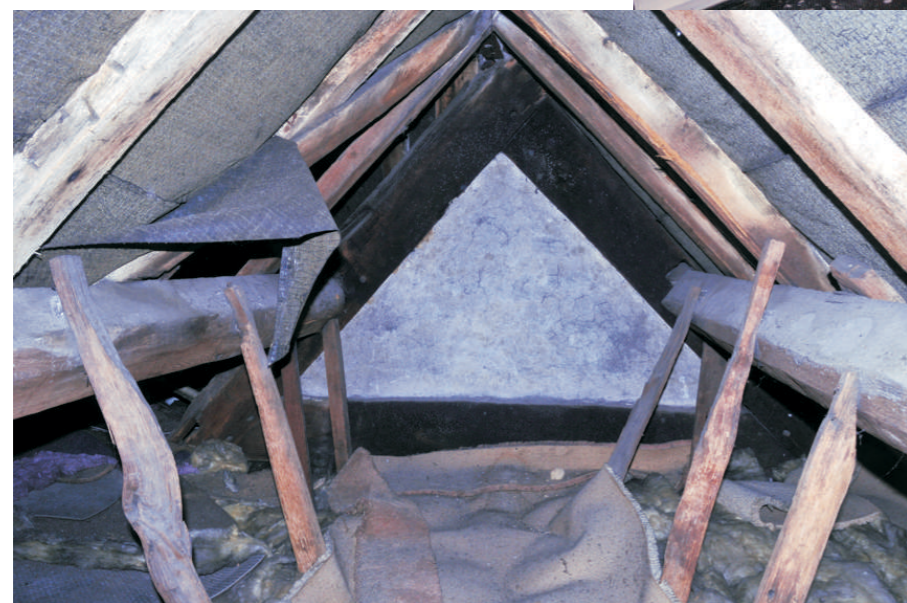
Roof space facing south - note sooting of truss but clean purlins. Note also redundant mortice possibly for wind-brace beneath LH purlin. Brick infill of Truss 2 apex is plastered and colourwashed indicating that it was formerly exposed.
