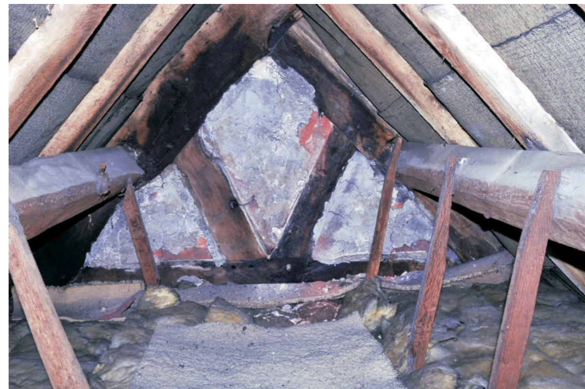
Roof space facing north, note extensive sooting of truss which does not extend to purlins - interior of Truss 3 infill panels are plastered. Timber hangers for ceiling are nailed to purlins
