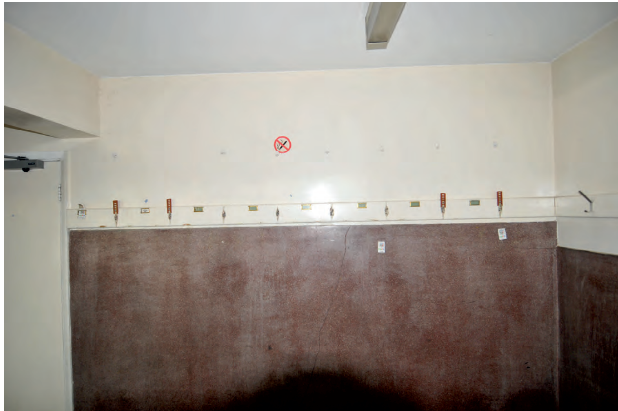
Equipment room off garage
