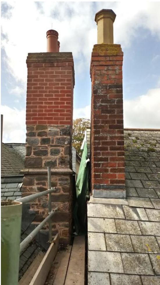
Fig. 48 Chimney of south gable, note brick repair of upper nine courses, with chimney of The Walronds to the south (photo ref: 0064).
