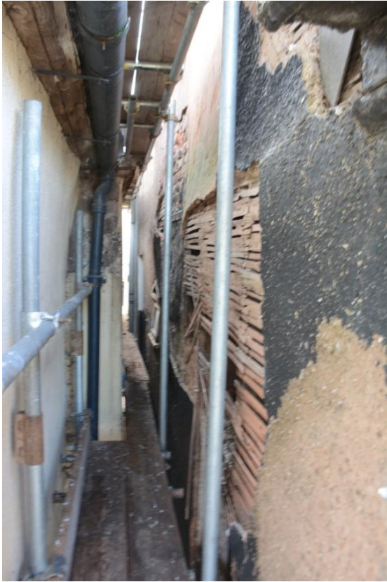
Fig. 34 South elevation, oblique view looking west along the wall in the narrow gap between Veryards (left) and The Walronds (right), showing condition before stripping in September 2017 (photo ref: 6868).
