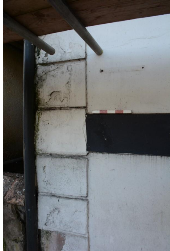
Fig. 23 Southern quoin, detail of rusticated quoins and plat band, looking south west (photo ref: 6908).
