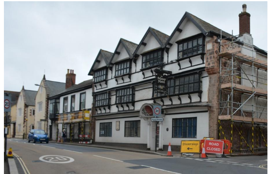
Fig. 19 The same view in November 2015, with works coming to an end on the Manor House and an inspection scaffold erected on No. 4 (photo ref: 8239).
