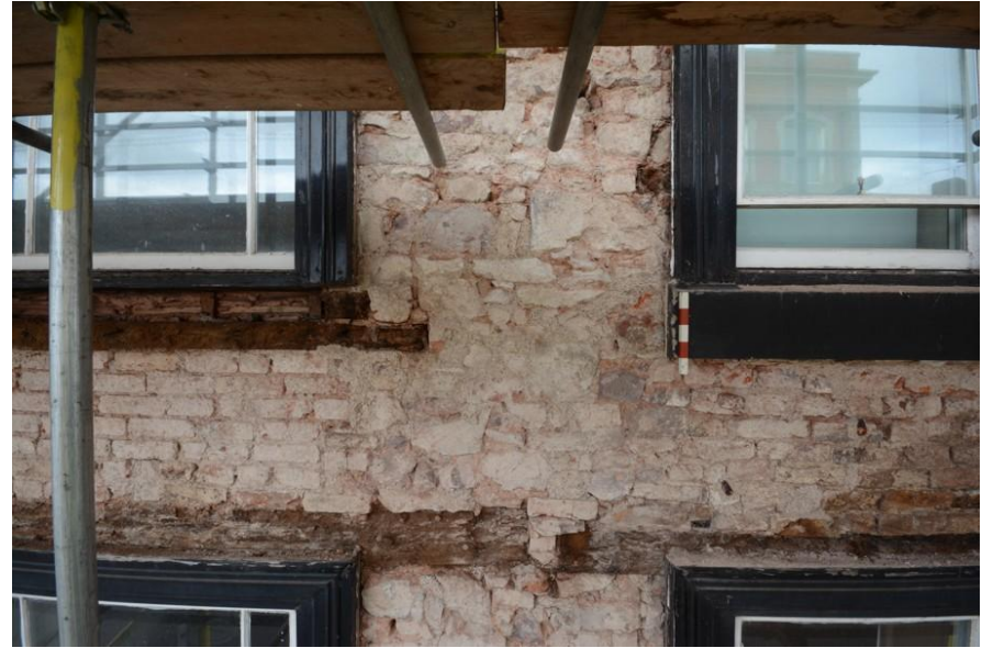
Fig. 27 Southern and central first-floor windows, showing brick aprons beneath and original lintels to ground-floor windows below (photo ref: 7028).
