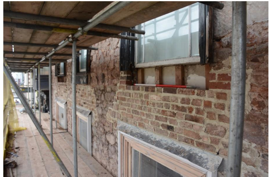
Fig. 29 Oblique view along first floor at window sill level, showing repairs in progress after inserted of new concrete lintels (photo ref: 7522).
