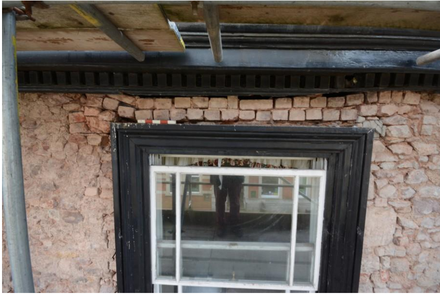
Fig. 26 Northern first floor window, showing improvised 1980s brick repair of decayed lintel (photo ref: 6997).
