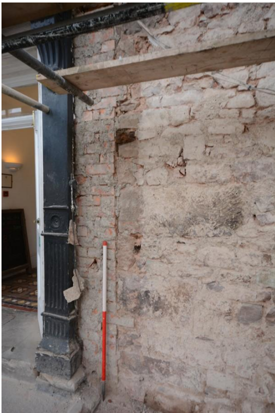
Fig. 32 Masonry quoin, ground floor stage, showing also brick north pier of late 19th century doorway (photo ref: 7055).
