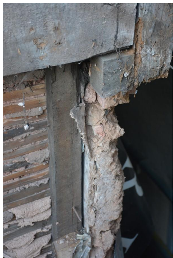
Fig. 41 Rear elevation, detail of cob filled partition of south wall, seen here in section in the west, looking south east, note plaster on inside face (photo ref: 7486).
