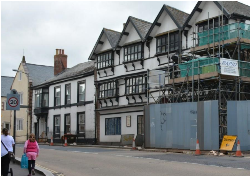
Fig. 18 Nos 2 and 4 Fore Street in August 2015, with works in progress on the Manor House Hotel, showing Veryards pre-works (photo ref: 2115).
