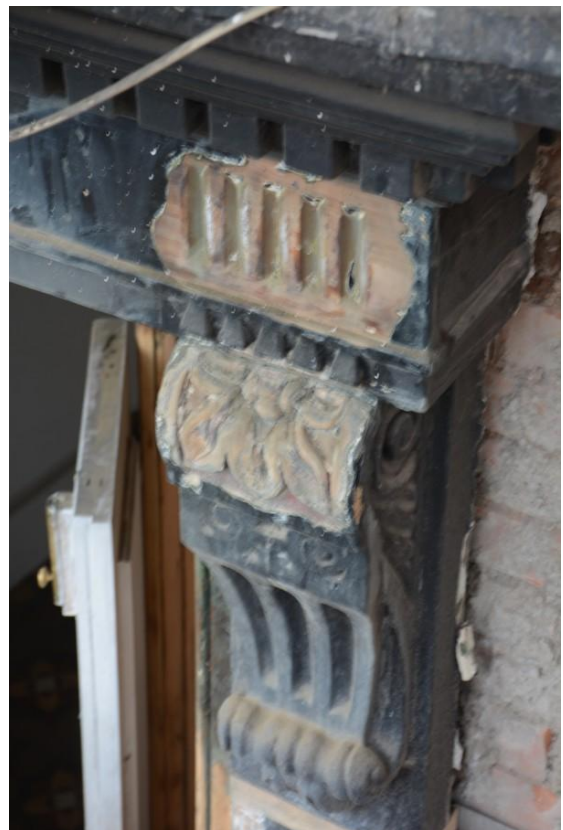
Fig. 25 Detail of console bracket of late 19th century doorway to the side passage, partially stripped, showing the clarity of detail beneath layers of paint (photo ref: 7528).
