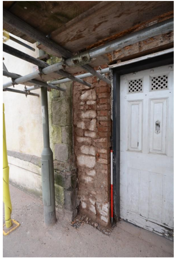
Fig. 33 Masonry pier on the south side of the original side entrance, abutting the quoin of The Walronds, looking south west (photo ref: 7051).
