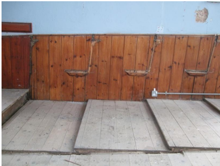
Plate 5 Wroot Wesleyan Chapel: west wall panelling and stepped platforms with fixing points for the missing pews.
