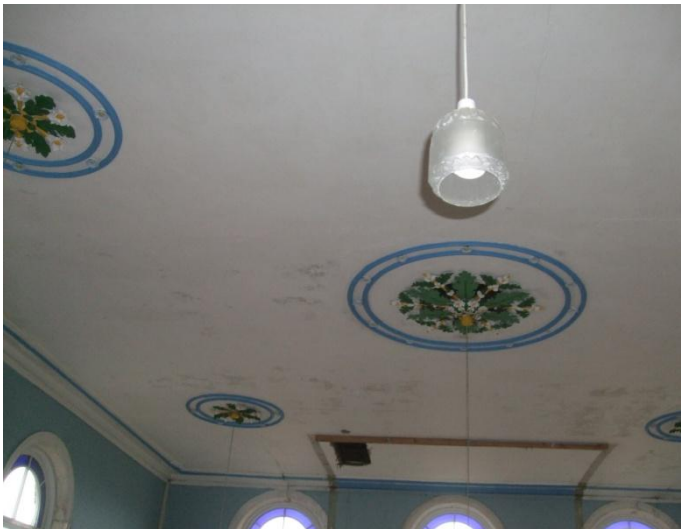
Plate 10 Wroot Wesleyan Chapel: the ceiling, with central and smaller roses, and the entrance lobby scar, viewed from the south.
