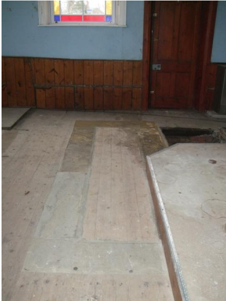
Plate 7 Wroot Wesleyan Chapel: stone surround for a heating grille.
