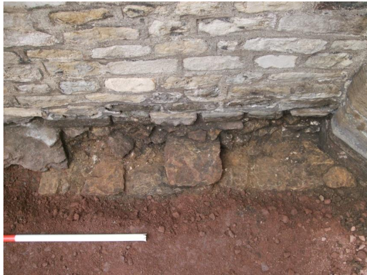
Plate 12 (Archive image PCGC 384) Eastern Gateway: west side, east elevation with the footing courses of the wall blocking the arch. Photograph: Caroline Atkins
