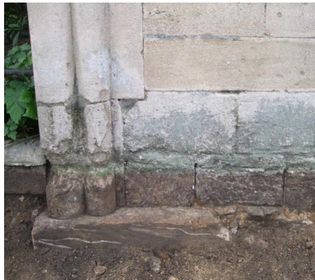
Plate 21 (Archive image PCGC 142) Bishop's Gate: east side, north elevation, showing the offset course exposed by the groundworks. Photograph: Caroline Atkins
