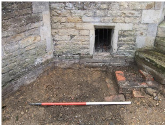
Plate 26 (Archive image PCGC 153) No. 27: north elevation, east of the front door, showing the location of the coal-hole. Photograph: Caroline Atkins
