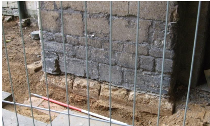
Plate 36 (Archive image PCGC 103) Norman Gate: east gate arch, south side - medieval footings exposed in the reopened service trench. Photograph: Caroline Atkins
