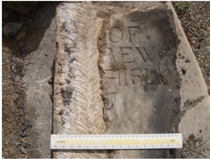
Plate 51 (Archive image PCGC 221) South Portico steps: stone SR 002 Photograph: Caroline Atkins
