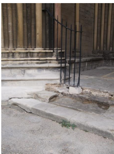
Plate 46 (Archive image PCGC 233) North Portico steps, north end: after stone removal, showing the location of Plate 44.
