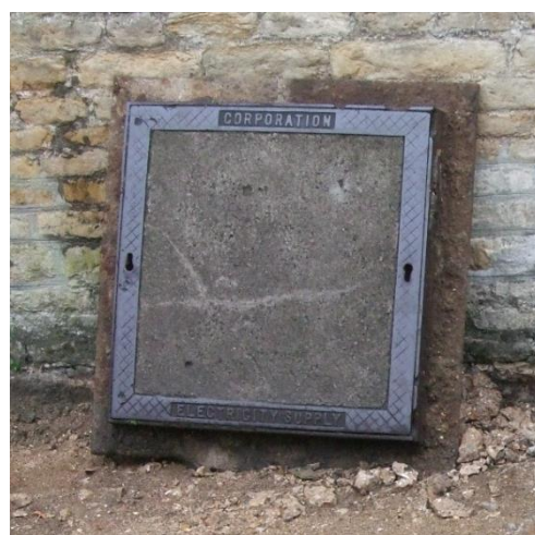
Plate 29 (Archive image PCGC 014) The 'CORPORATION ELECTRICITY SUPPLY' inspection chamber lid. Photograph: Caroline Atkins
