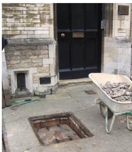
Plate 28 (Archive image PCGC 008) The electricity supply inspection chamber outside No. 27A Photograph: Caroline Atkins
