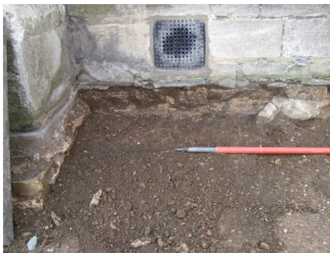
Plate 32 (Archive image PCGC 127) No. 28: potential medieval footings to the west of the buttress. Photograph: Caroline Atkins
