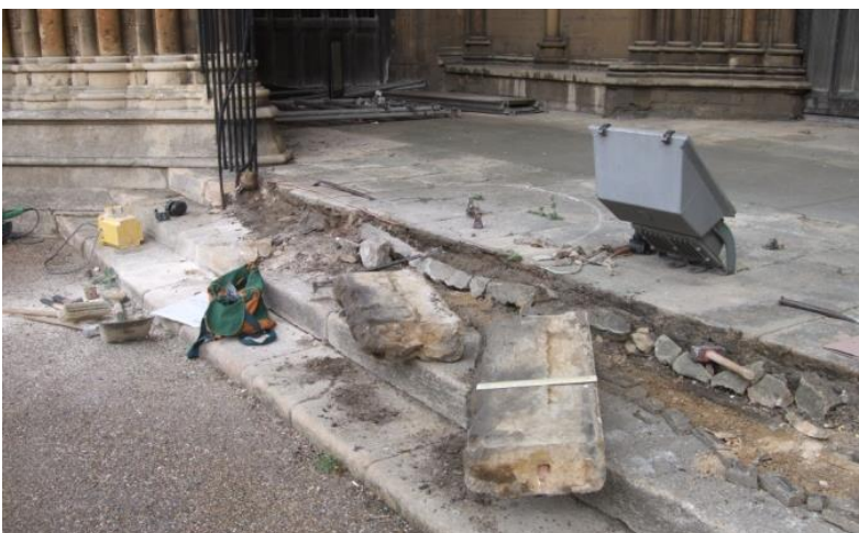
Plate 50 (Archive image PCGC 217) South Portico Steps: reused memorial stones SR 002 and SR 001 as lifted from the top step.
