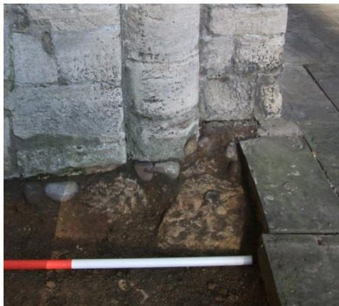
Plate 35 (Archive image PCGC 078) Norman Gate: east elevation, medieval footings exposed by reduction of levels prior to the reopening of the service trench. Photograph: Caroline Atkins
