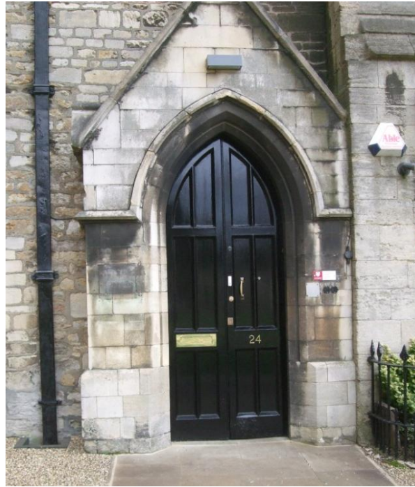
Plate 15 (Archive image: PCS 17 001) Interpretation board G-WF-14: intended location on No. 24 Minster Precincts. Photograph: Caroline Atkins
