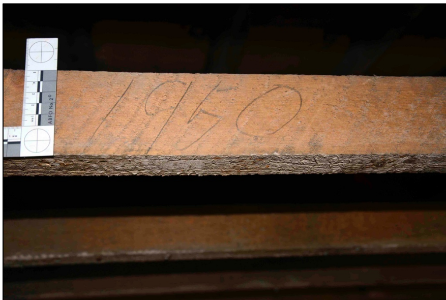
Appendix I.36: Detail of pencil date on lower ceiling joists in Area A - 1950.
