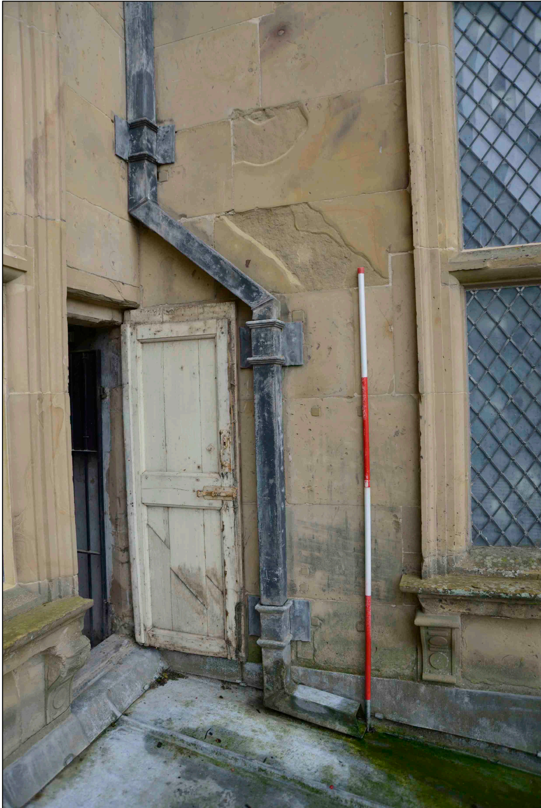
Appendix I.5: View of south-east door onto West Loggia roof prior to repairs in October 2020.
