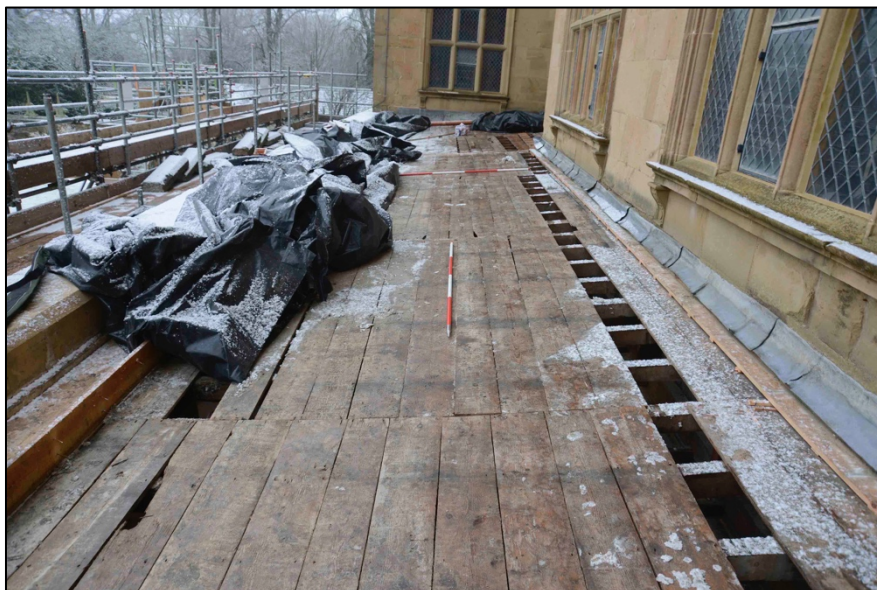
Appendix I.16: View of exposed 'original' boards in central section of roof ( Area B ), looking north.
