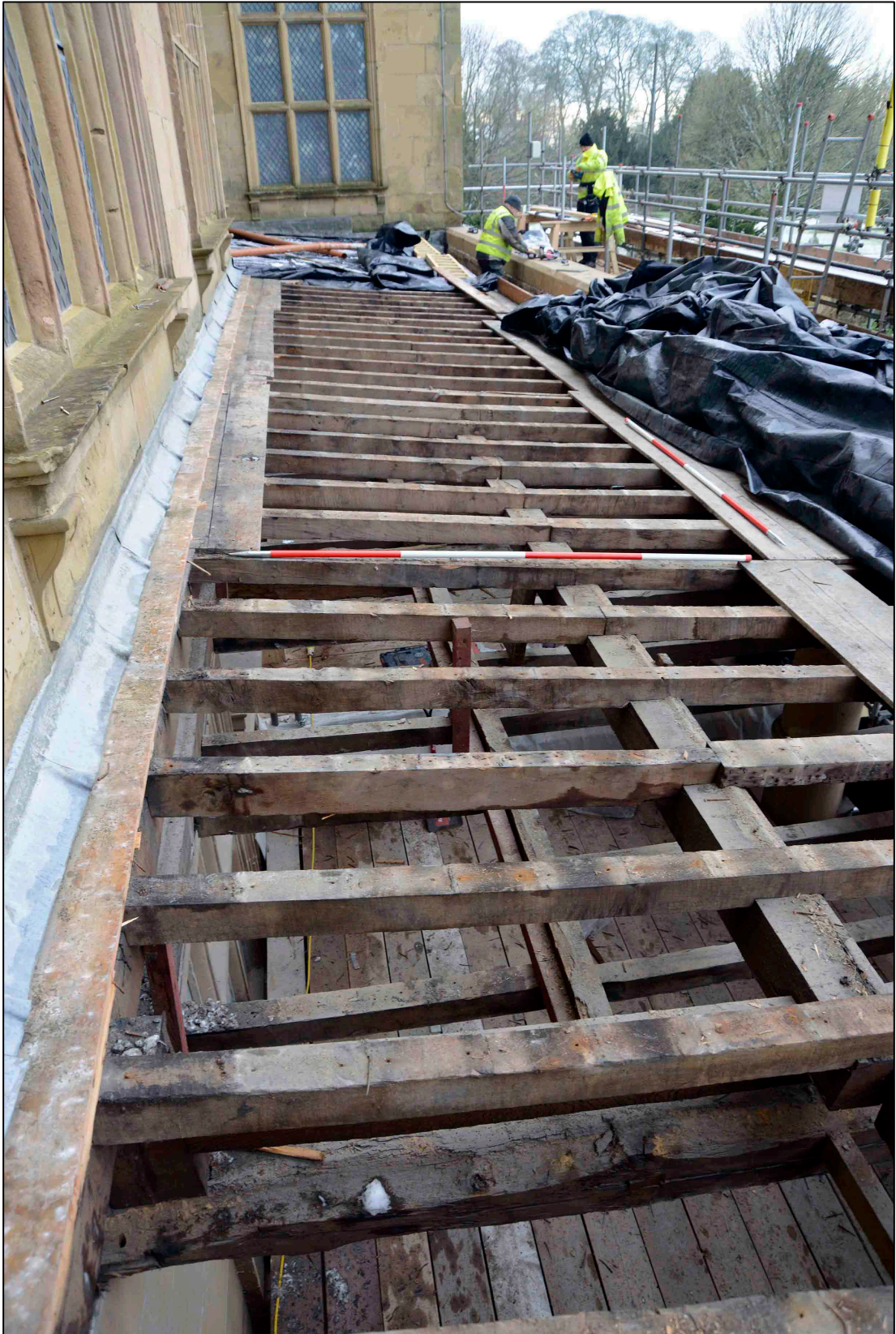
Appendix I.21: Detail of central section of roof (Area B) following removal of boards, looking south.
