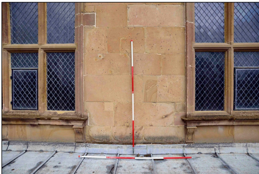
Appendix I.10: Detail of central section of west elevation ( Area B ), looking east.
