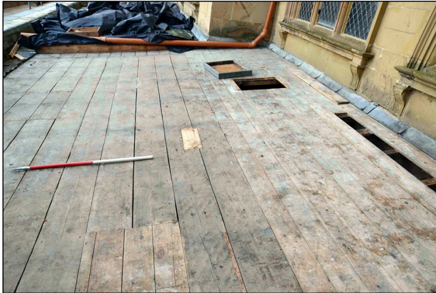
Appendix I.15: Detail of exposed boards in Area A ; note narrow replacements, looking north.
