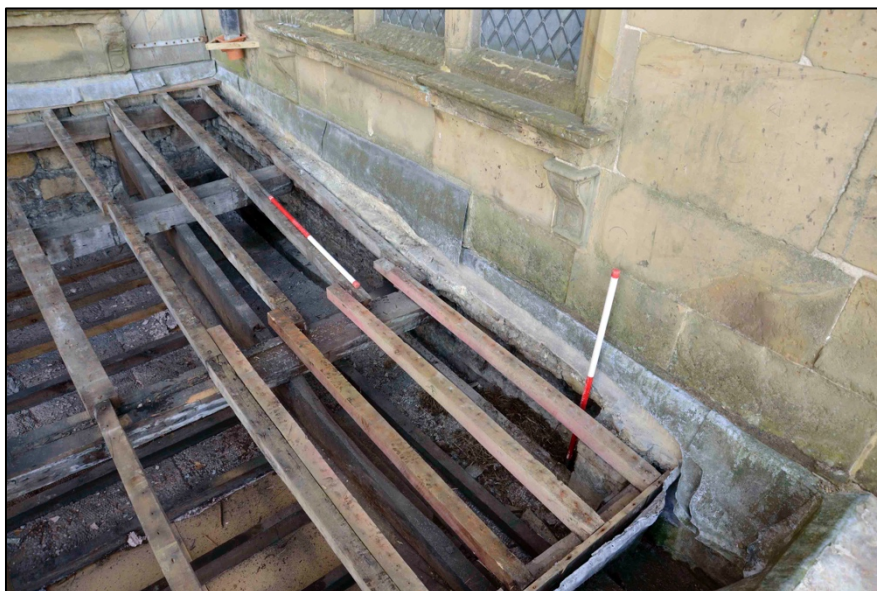
Appendix I.20: Detail of rafters and south wall of Area A ; note stone offset at a different angle to the rafters.
