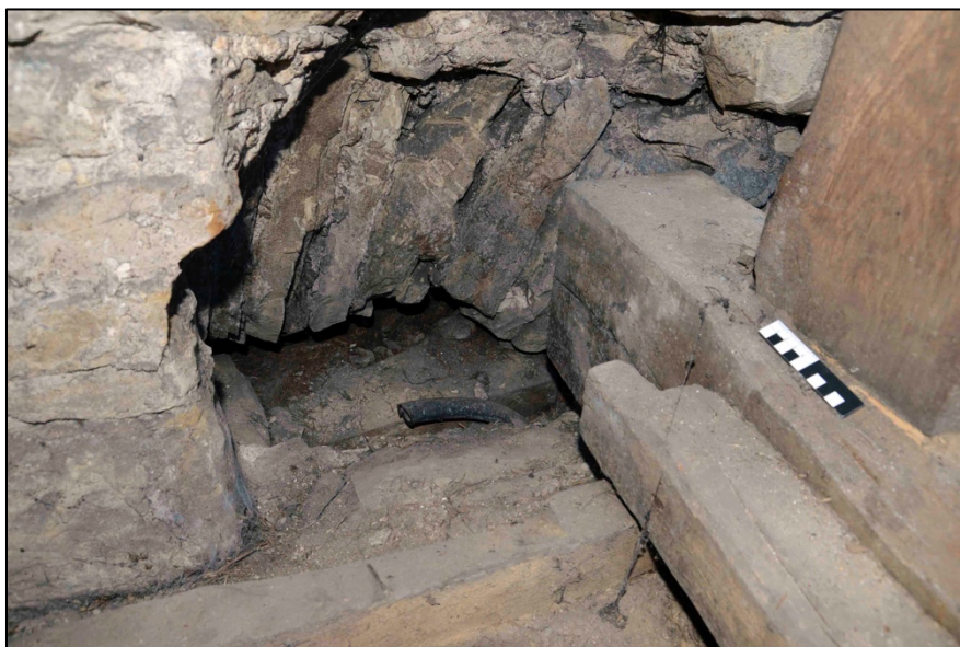
Appendix I.56: Detail of inserted hole within west wall of Area A ; note internal relieving arch of window below and cut back lead pipe.
