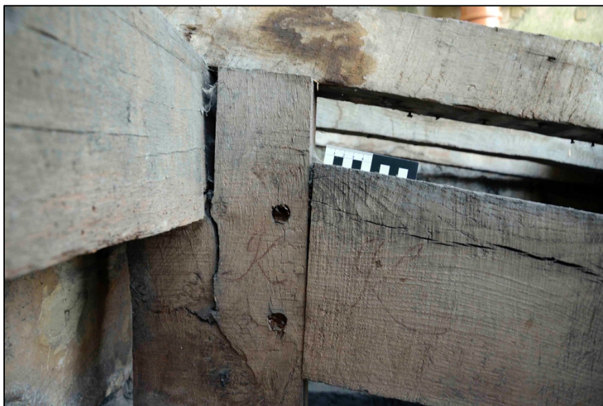
Appendix I.59: Detail of red painted letter 'K' on north face of post and principal joist of T10.
