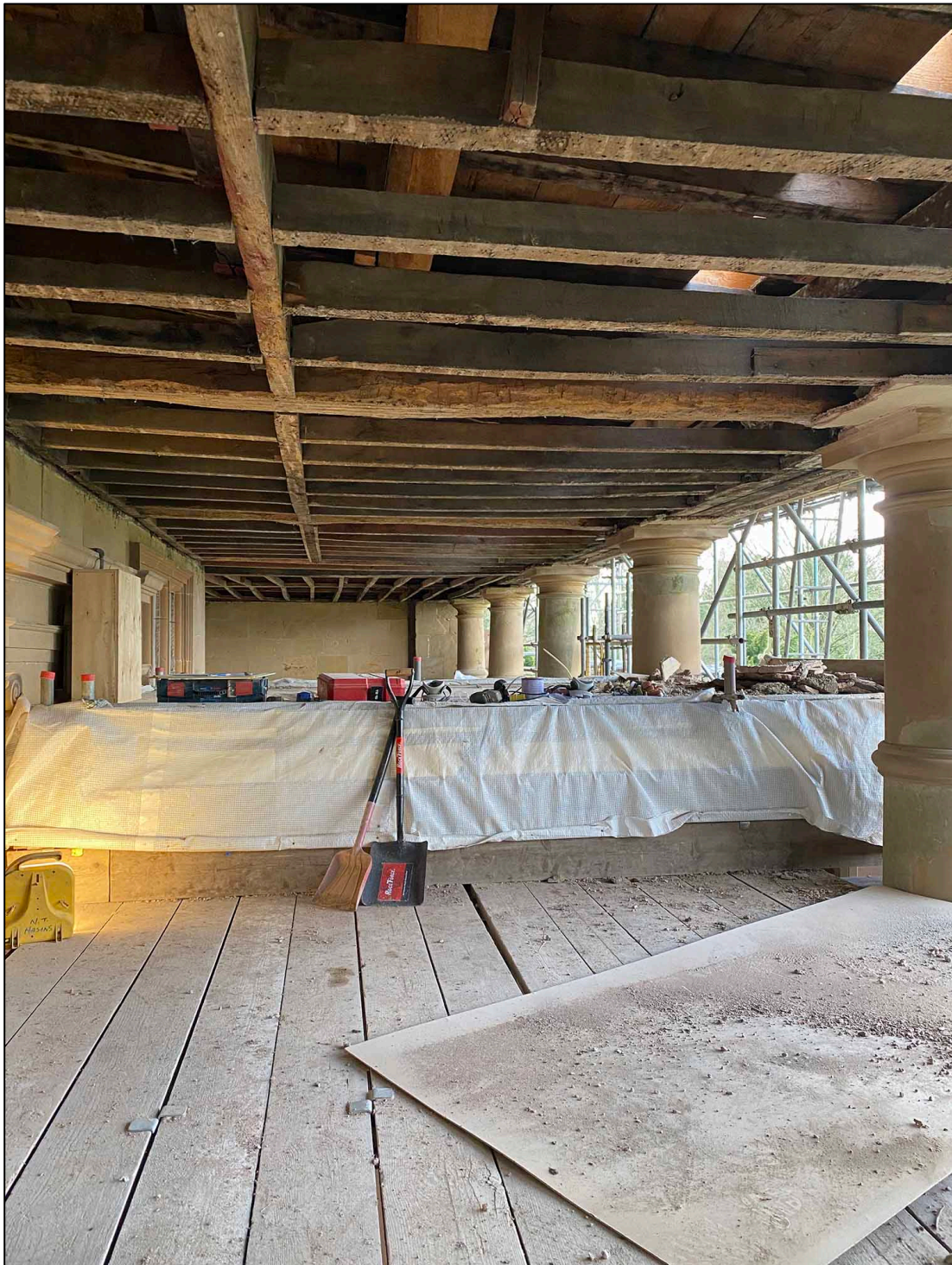
Appendix I.31: General view looking south of lower ceiling joists following removal of plaster
