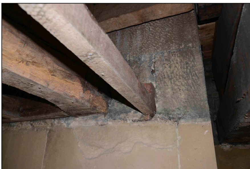
Appendix I.47: Detail of secondary ceiling beam inserted into masonry of Hall at south end of Area B ; note rough tooling above and ashlar below.
