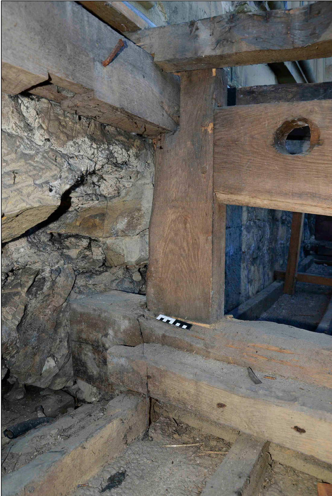
Appendix I.38: Detail of post at east end of T9; note inserted hole in walling.
