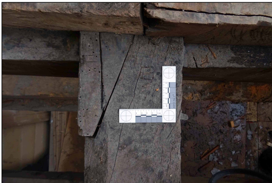
Appendix I.55: Detail of pegged and scarfed upper purlin in Area B ; note chisel cut assembly numerals (VII).
