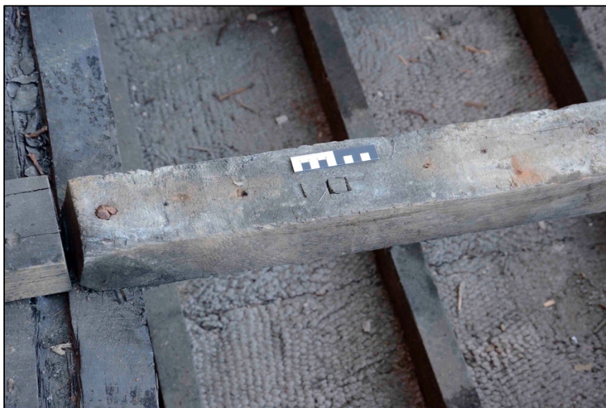
Appendix I.27: Detail of reused rafter with redundant square peg and chisel cut assembly mark.
