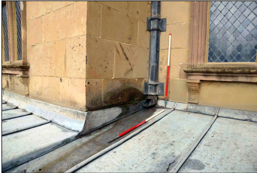
Appendix I.9: Detail of gutter outflow and flashing prior to repairs in October 2020, looking north-east.
