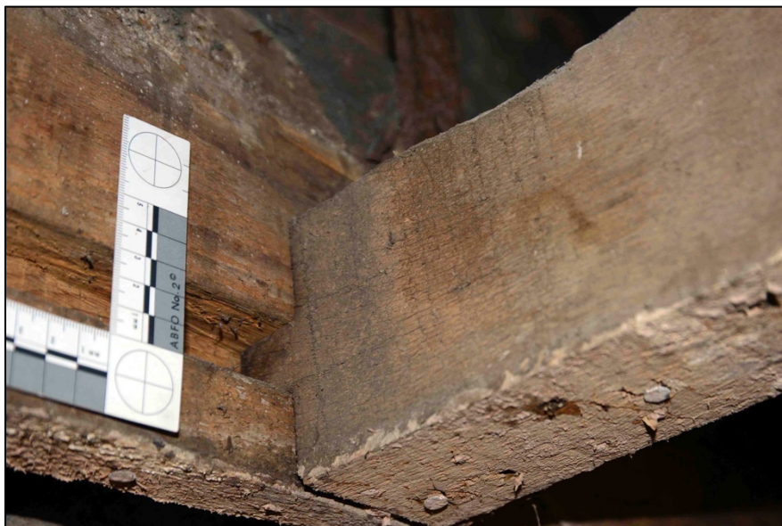
Appendix I.49: Detail of horizontal slot and tenon of lower ceiling joist in Area C ; note scored incision layout cuts.
