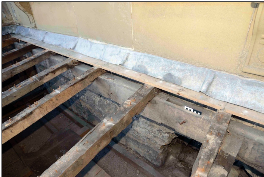
Appendix I.29: Detail of timber construction along the west wall of the Hall in Area A ; note rafters notched over timber bearer.
