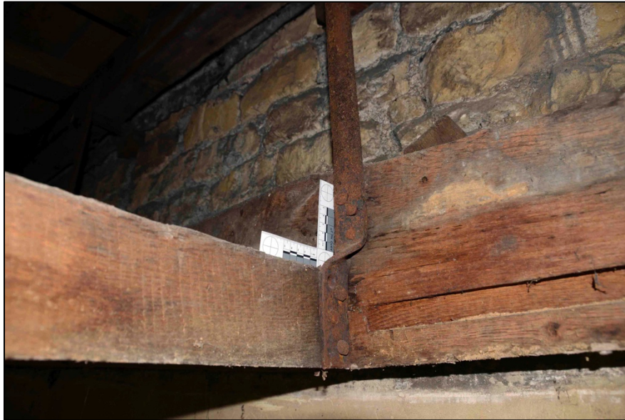
Appendix I.48: Detail of wrought iron strap within Area C ; note horizontal slot for tenon of lower ceiling joist.
