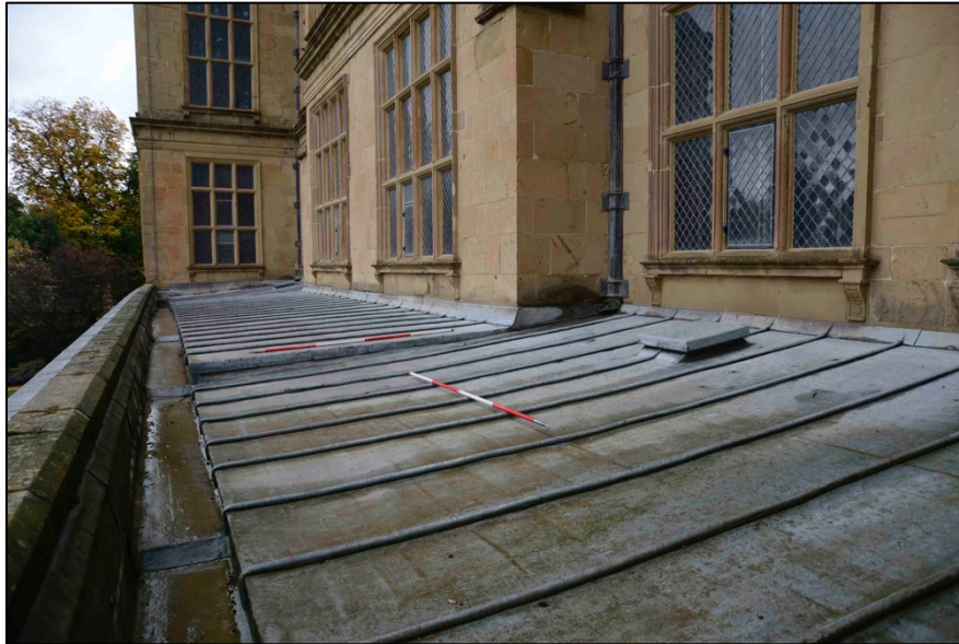
Appendix I.6: View of roof prior to repairs in October 2020, looking north-east.
