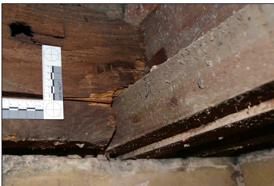
Appendix I.50: Detail of tenon of lower ceiling joist in Area C .
