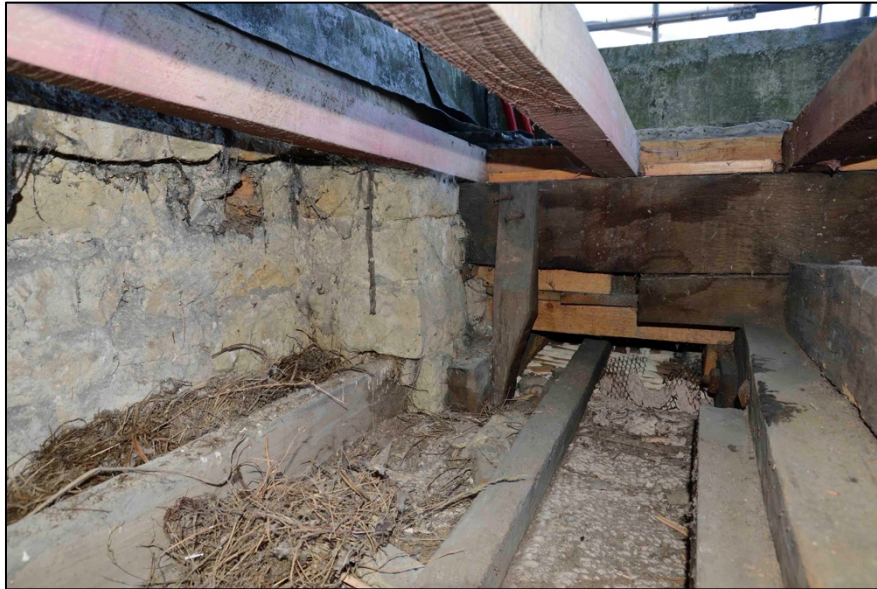
Appendix I.42: Detail of south-west corner of Area A ; note stone pier and replaced rafters.
