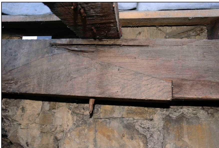
Appendix I.53: Detail of pegs and scarfed timber bearer beam against west wall of Hall in Area A .
