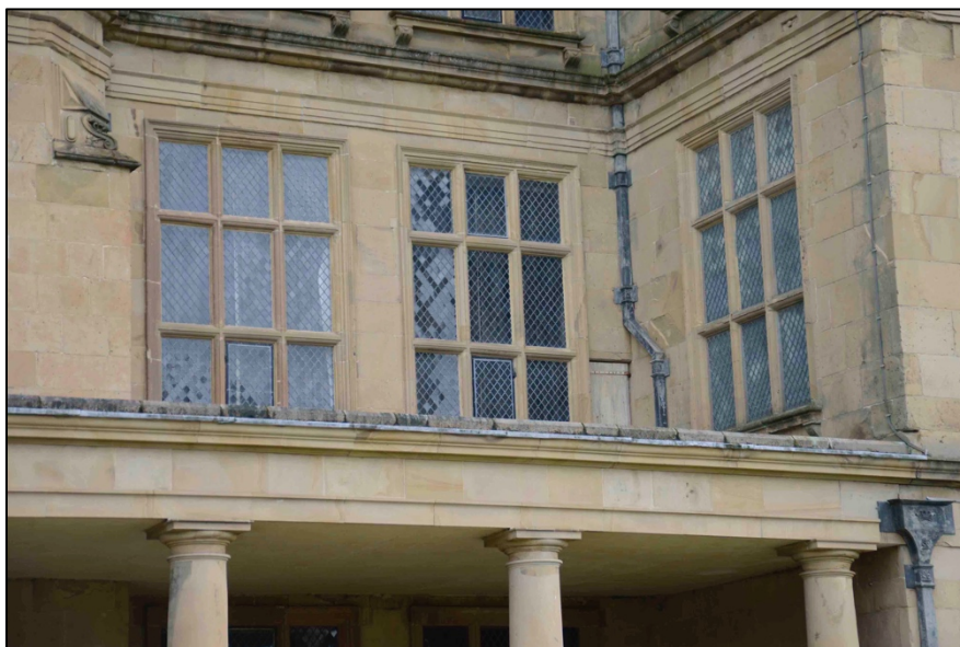
Appendix I.4: Detail of entablature above collonade prior to repairs in October 2020, looking south-east.
