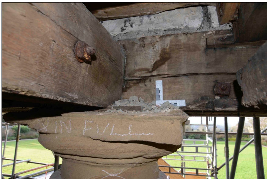
Appendix I.46: Detail of tie beam tenoned into entablature beam above column; note bolted fixings.
