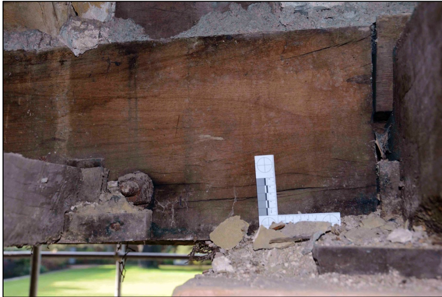
Appendix I.45: Detail of junction of timber beams and truss above column; note bolted fixing.
