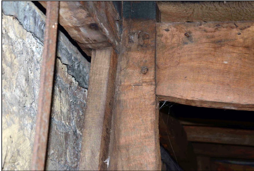
Appendix I.57: Detail of red painted letter 'B' on north face of post and principal joist of T2.
