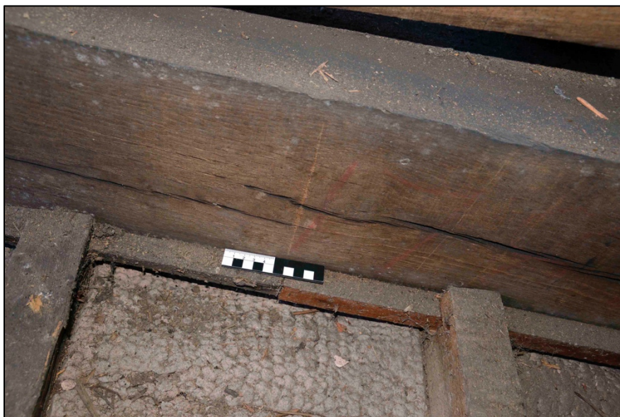
Appendix I.41: Detail of red painted marks (letters?) on south face of tie beam on T8.
