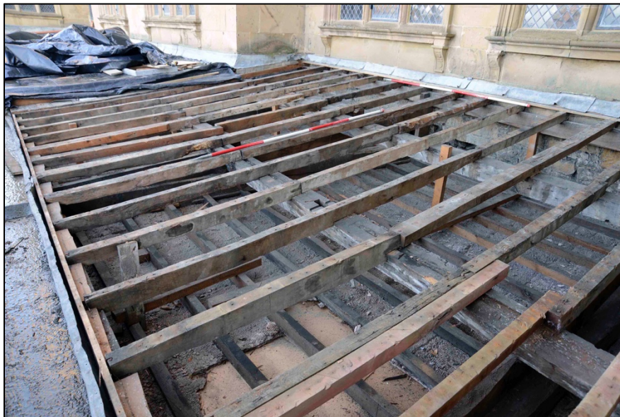
Appendix I.23: Detail of Area A following removal of boards, looking north.
