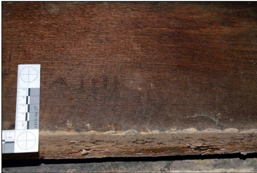
Appendix I.51: Detail of chisel cut assembly marks (VIII) on lower timber bearer against west wall of Hall in Area C .
