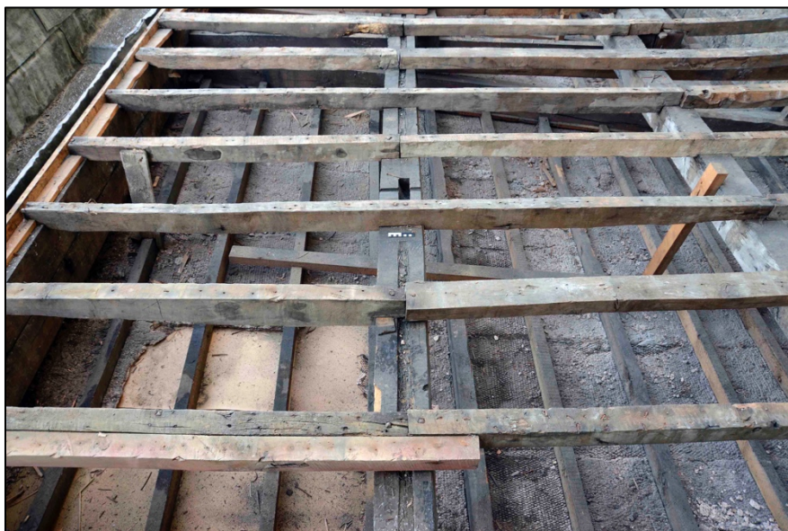
Appendix I.24: Detail of Area B following removal of boards, looking north; note reused prulin and patched hole in plaster ceiling below.
