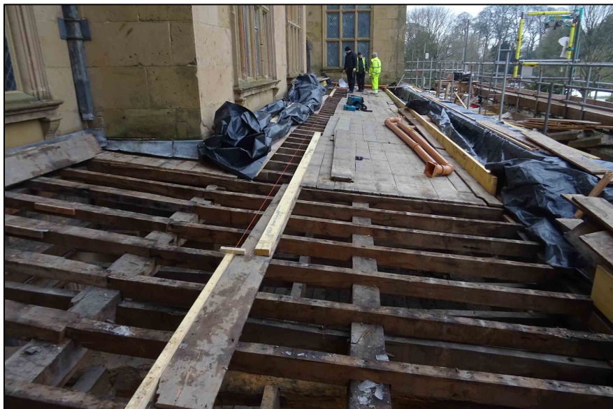
Appendix I.30: General view looking south across Areas B and C with partial removal of boards.
