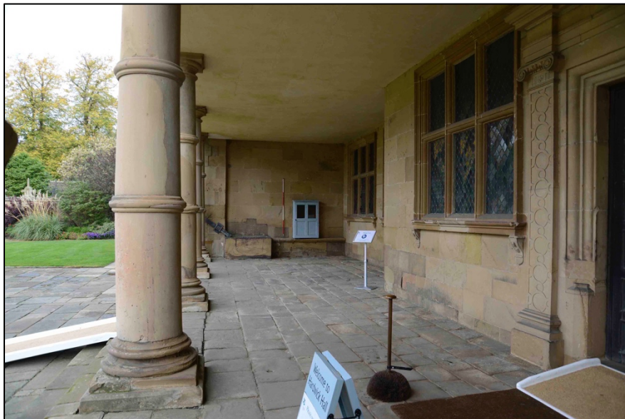
Appendix I.3: View of collonade prior to repairs in October 2020, looking north.
