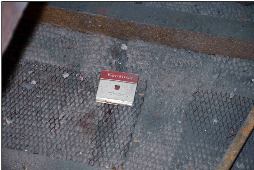
Appendix I.33: Detail of cigarette packet left within the roof void of Area A ; note expanded mesh for plasterwork below.
