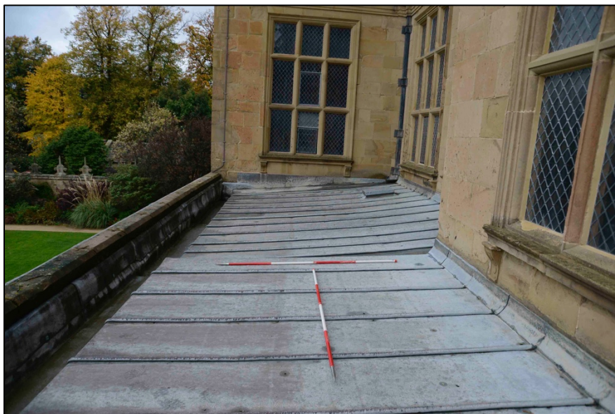
Appendix I.7: View of roof prior to repairs in October 2020, looking north.
