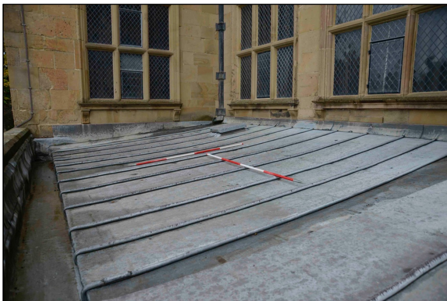
Appendix I.8: View of roof prior to repairs in October 2020, looking north-east.
