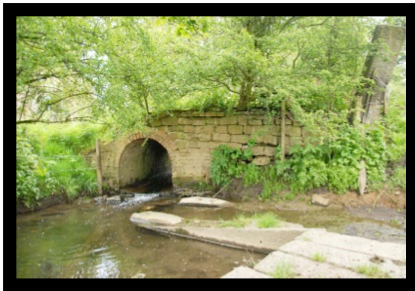
Photo: General view looking north; note use of brick for base of culvert
