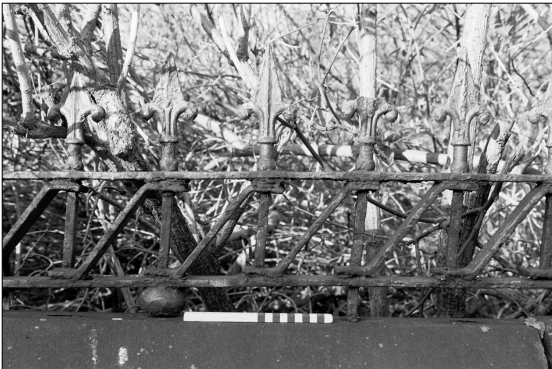
Appendix 5.8: Detail of railings on top of boundary wall, looking west (scale 20cm; Film 1.27).
