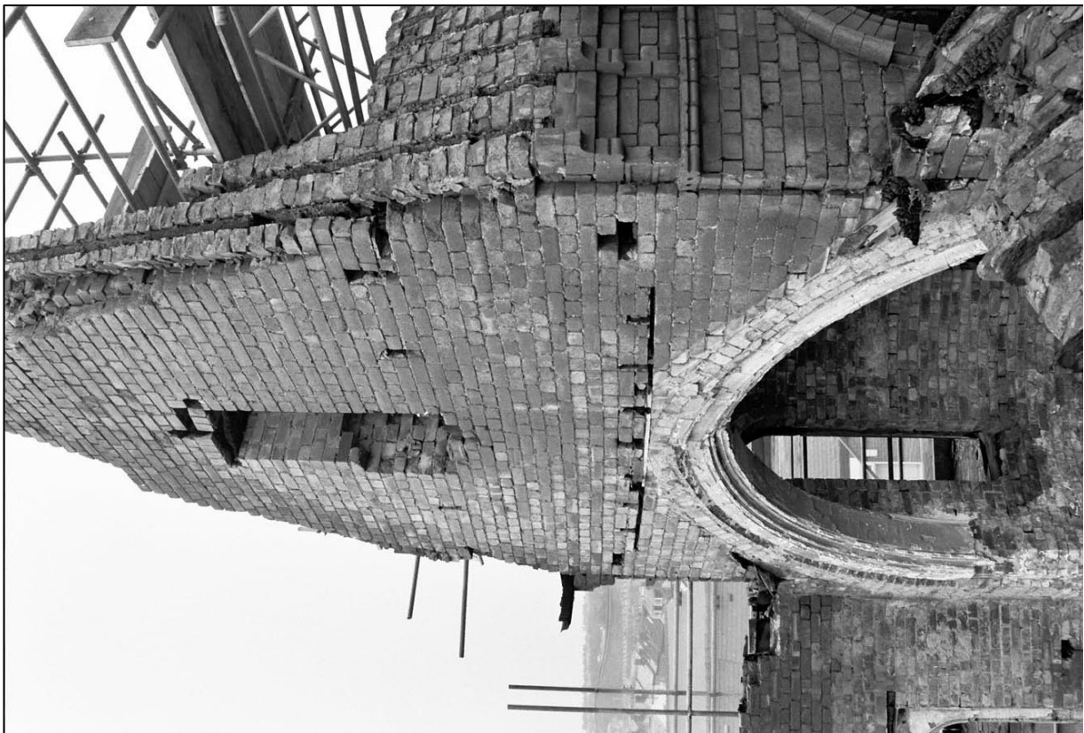
Appendix 5.27: Detail of upper section of internal brick gable to corner turret, looking east (Film 2.29).
