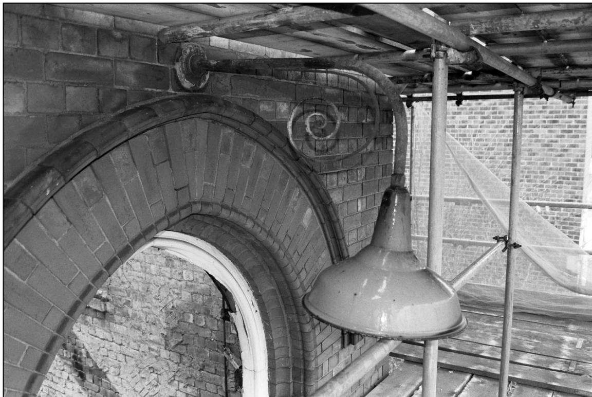
Appendix 5.14: Detail of decorative lighting bracket above first floor doorway on Vincent Road (Film 2.20).
