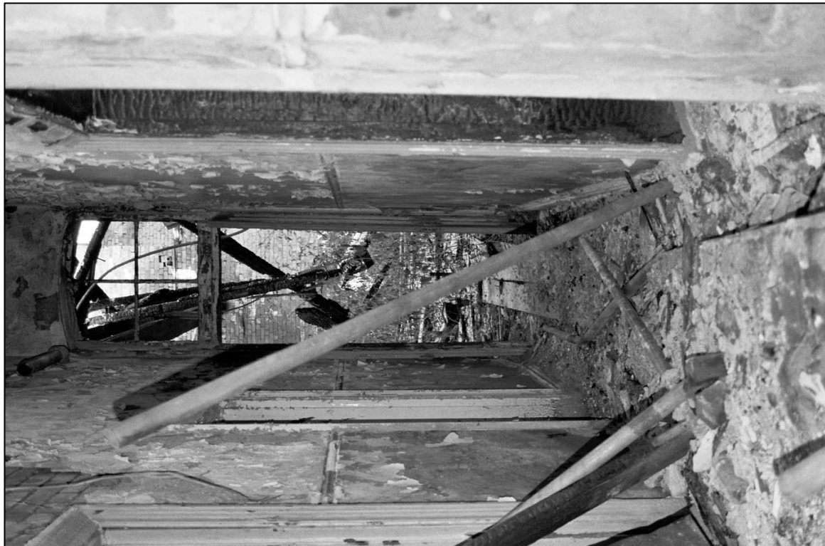
Appendix 5.21: General view of central north-south corridor on ground floor, looking north (Film 1.16).
