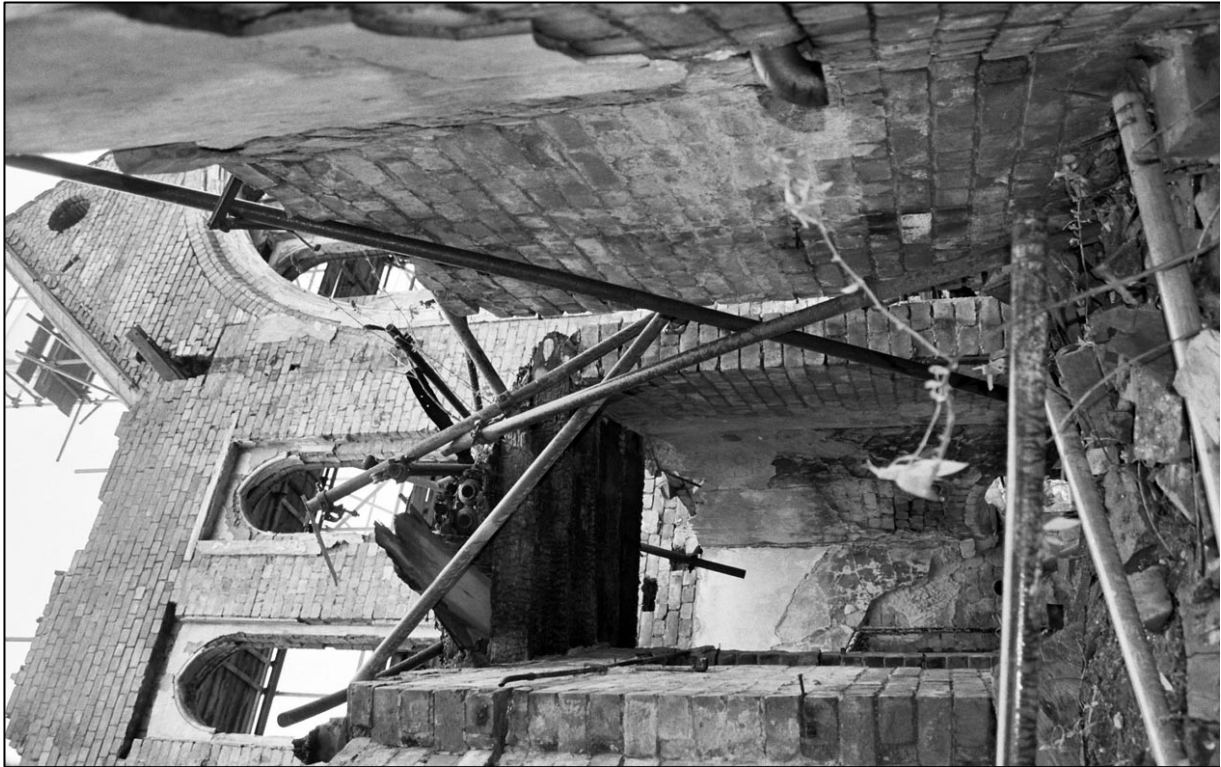
Appendix 5.26: General view of first floor corridor at south end of building, looking west (Film 2.7).
