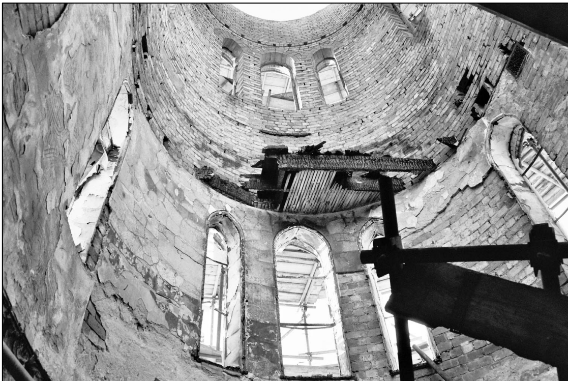
Appendix 5.20: View looking up inside the corner turret at south end of building (Film 1.23).
