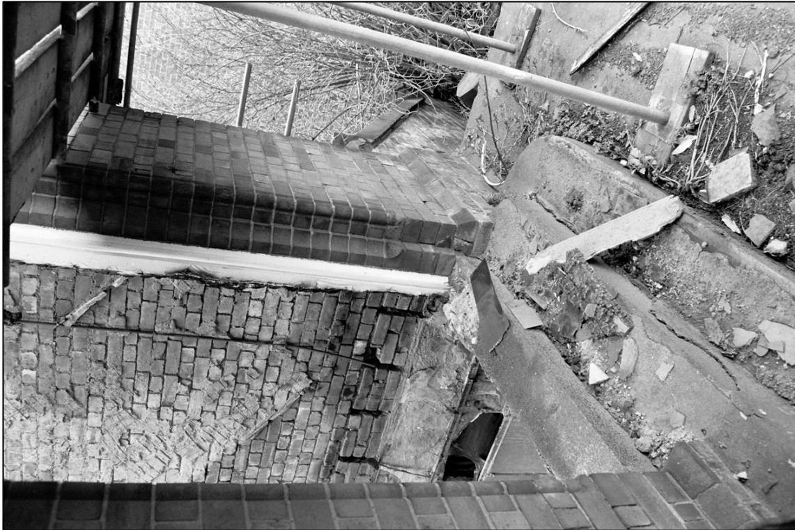
Appendix 5.11: Detail of door threshold of first floor entrance on Vincent Road, looking north (Film 2.13).
