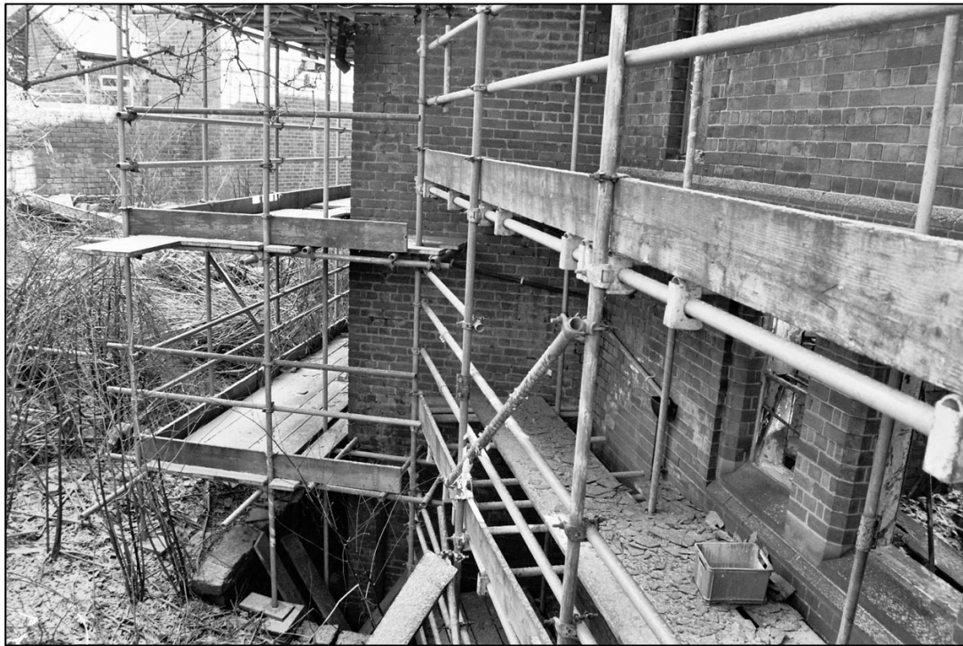
Appendix 5.9: General view of rear of site towards extension, looking north-east (Film 1.3).
