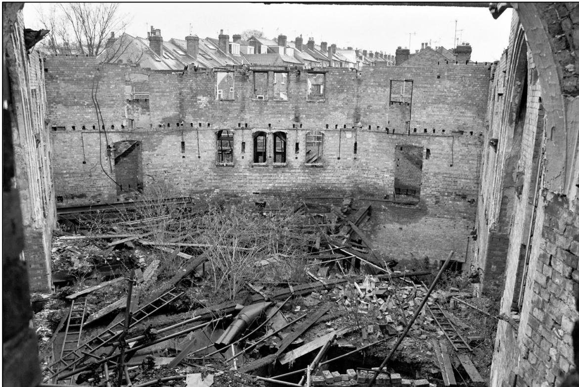
Appendix 5.29: General view from the south turret towards the rear of first floor, looking north (Film 2.22).
