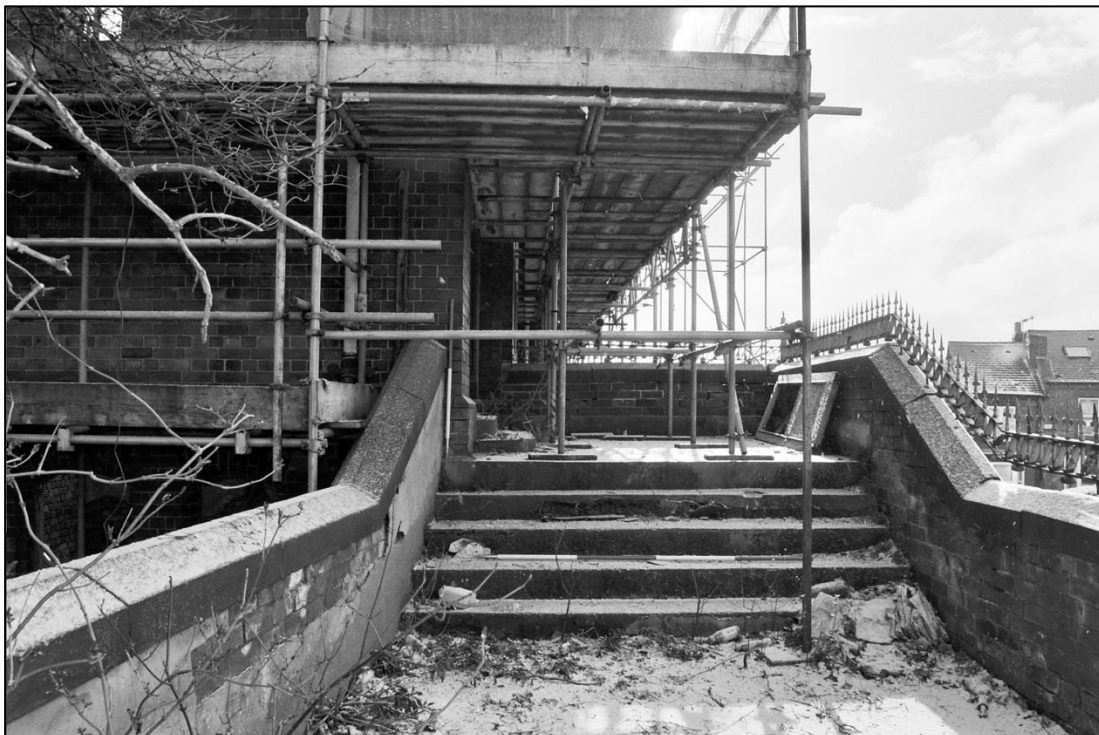
Appendix 5.10: First floor entrance steps on South View Road, looking south-east (Scale 1m/2m; Film 1.5).
