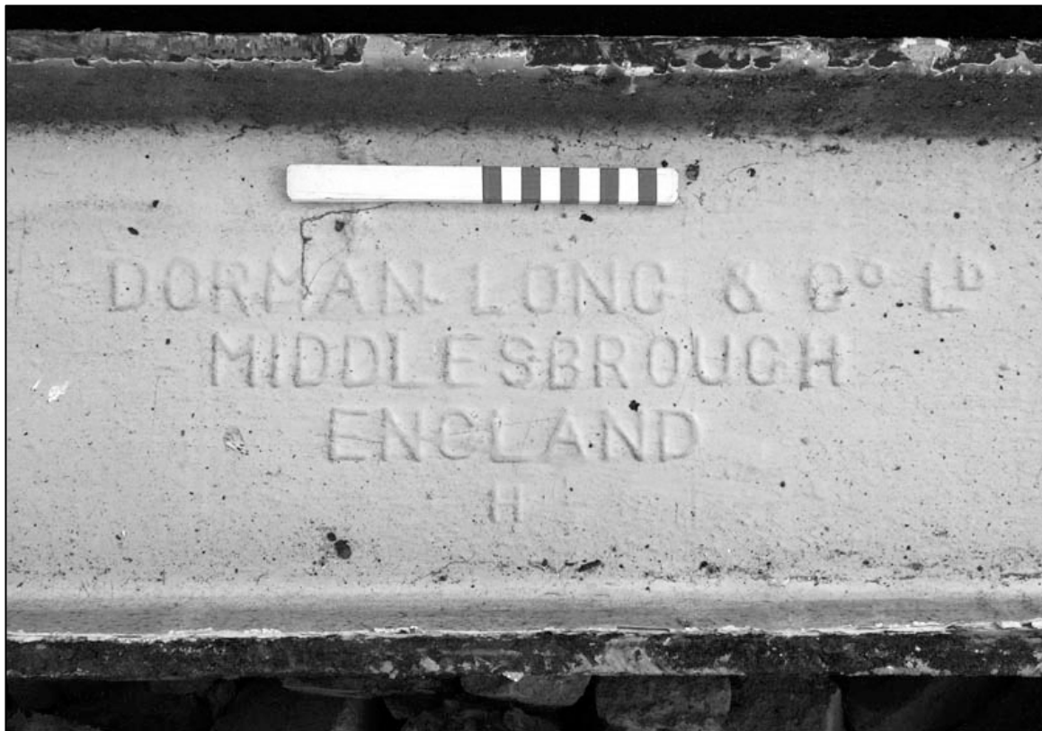
Appendix 5.25: Name stamp on beam used to support the first floor (Scale 20cm) (Digital Photograph).
