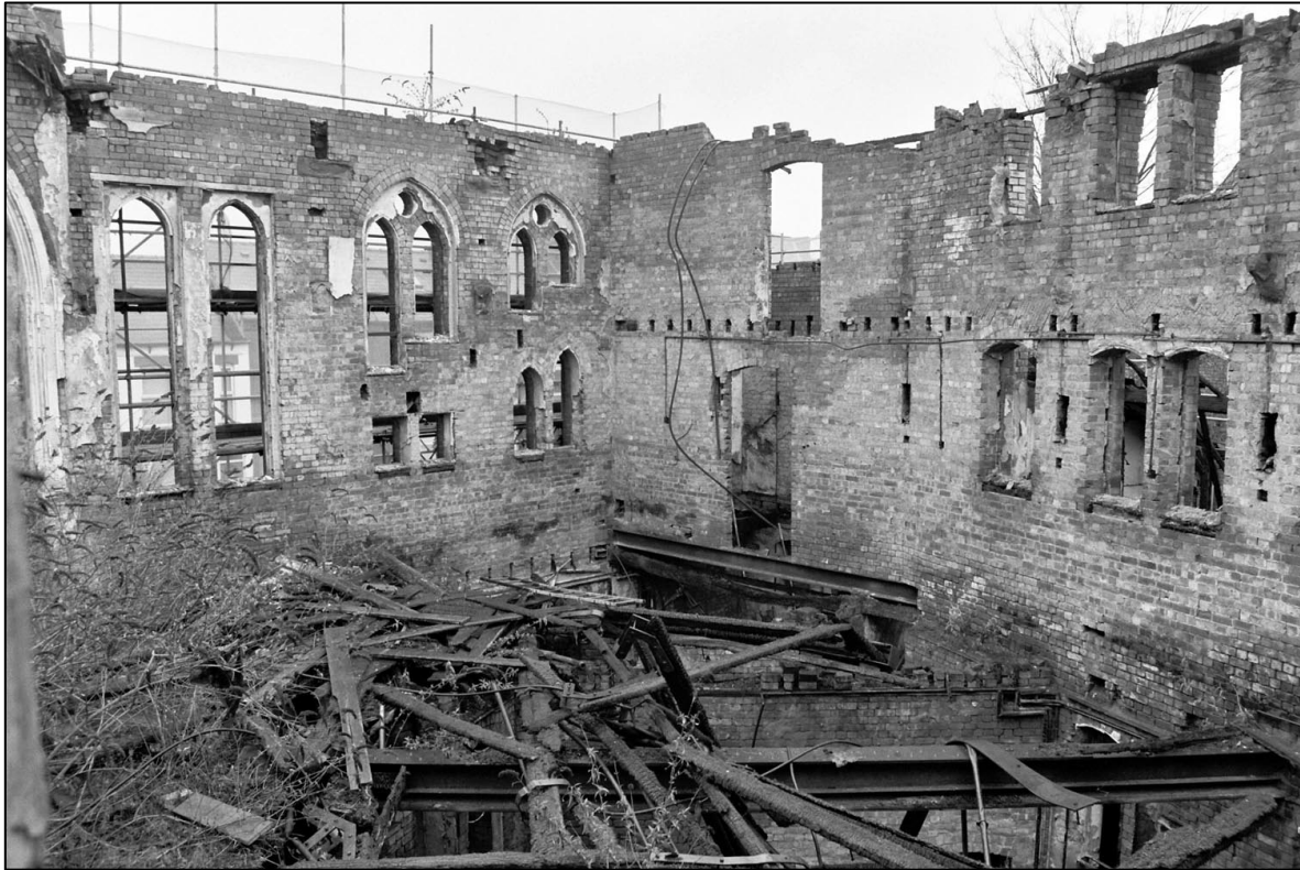
Appendix 5.28: General view of interior, looking west; note joist holes for former balcony (Film 2.18).
