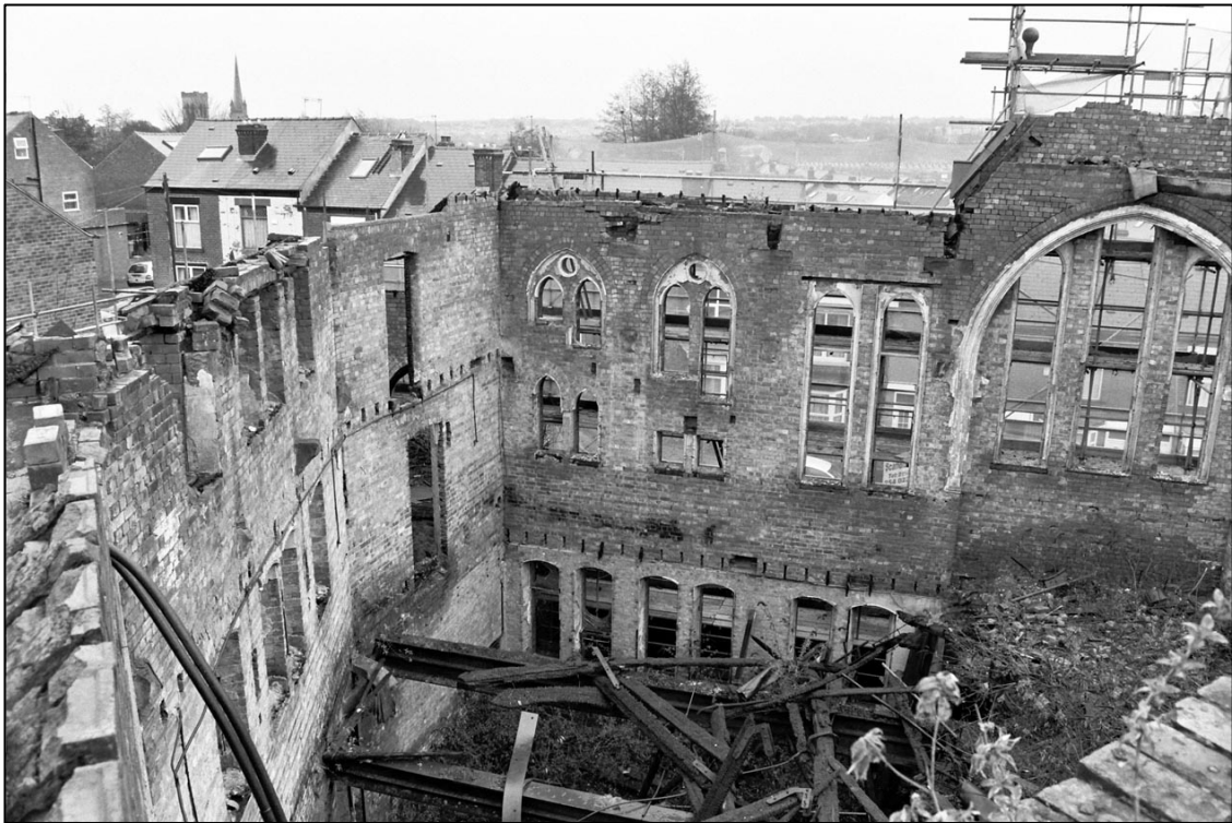
Appendix 5.33: General view of internal north-east corner; note angled joist holes for balcony (Film 2.33).
