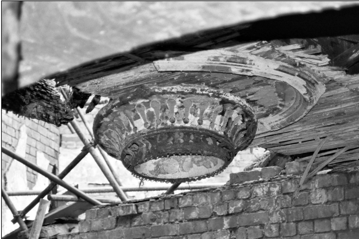
Appendix 5.24: Detail of ceiling mounted gas light holder on the ground floor, looking south-west (Film 2.9).
