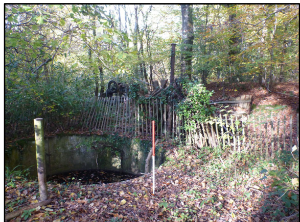
Appendix 3.18: Remains of pumping plant located on the southeast bank of the south pond.
