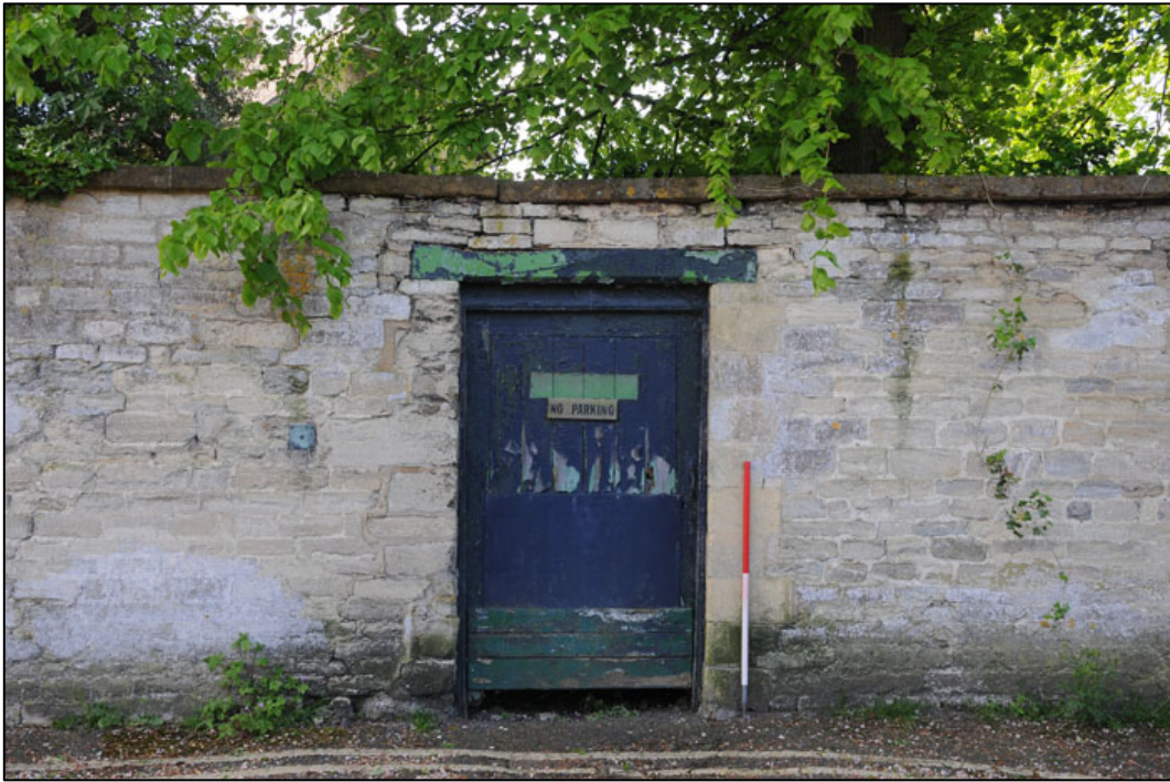
Appendix 3.33: Detail of pedestrian doorway HA9 in north boundary wall HA8 (1m scale).
