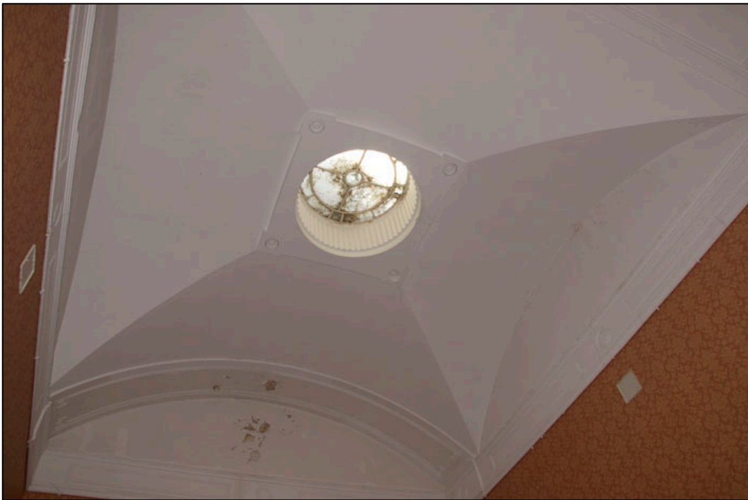
Appendix 3.8: Detail of vaulted ceiling and skylight above the main staircase in Woodstock House HA1 .
