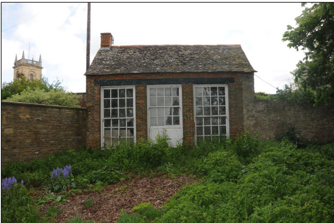
Appendix 3.20: Detail of northwest facing elevation of summer house HA3 (1m scale).
