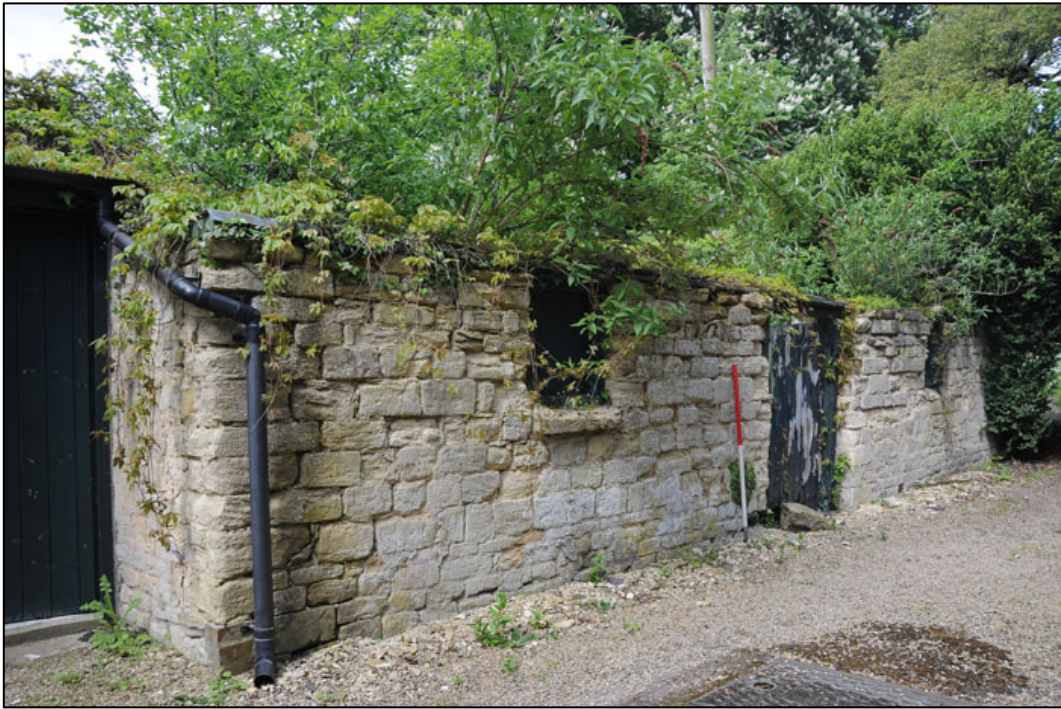
Appendix 3.19: General view of stone outbuilding HA1 , looking west; note advanced state of decay (1m scale).
