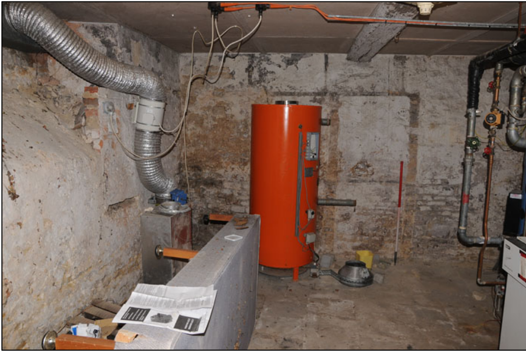
Appendix 3.3: General view of basement below Woodstock House HA1 ; note former light well to the left, and vertical wall scars in paintwork from former brick wine shelves (1m scale).
