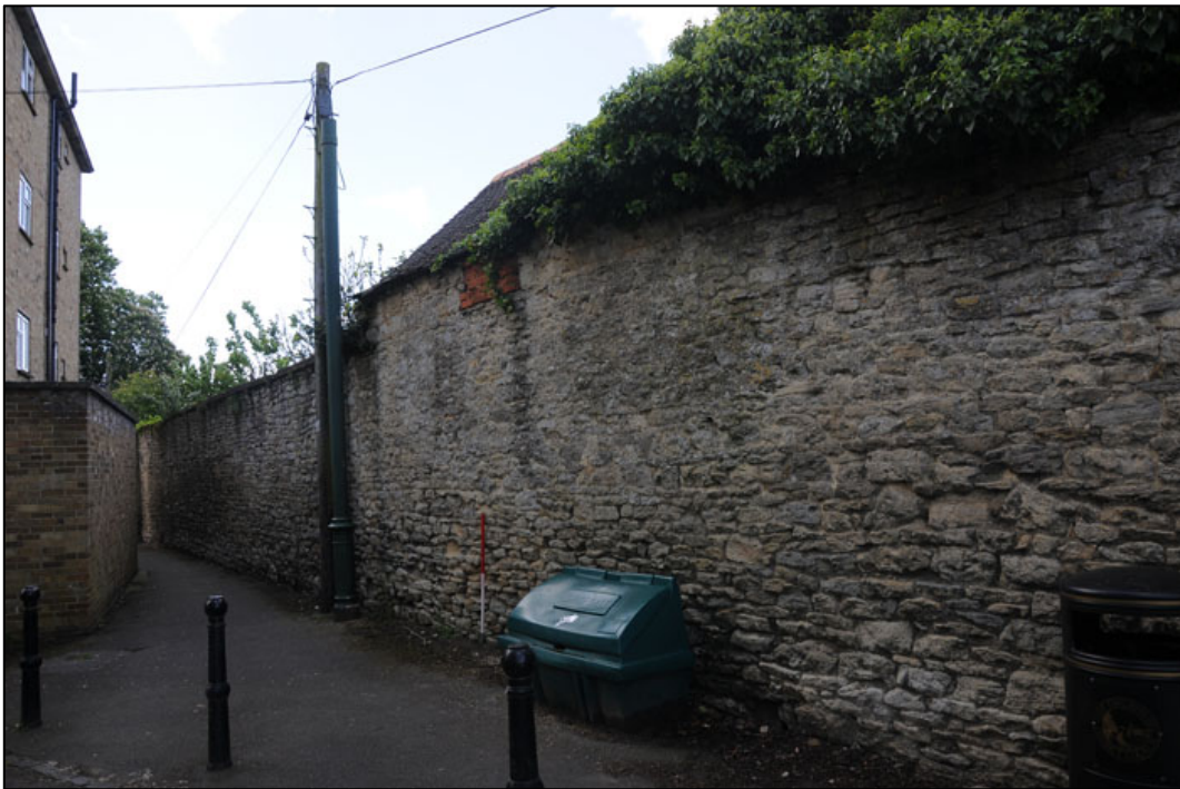
Appendix 3.34: General view along east boundary wall HA10 , looking southeast (1m scale).
