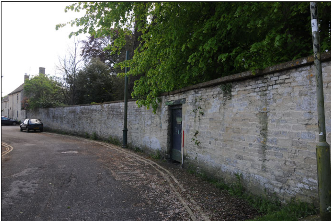
Appendix 3.32: General view along north boundary wall HA8 flanking Rectory Lane, looking southeast (1m scale).
