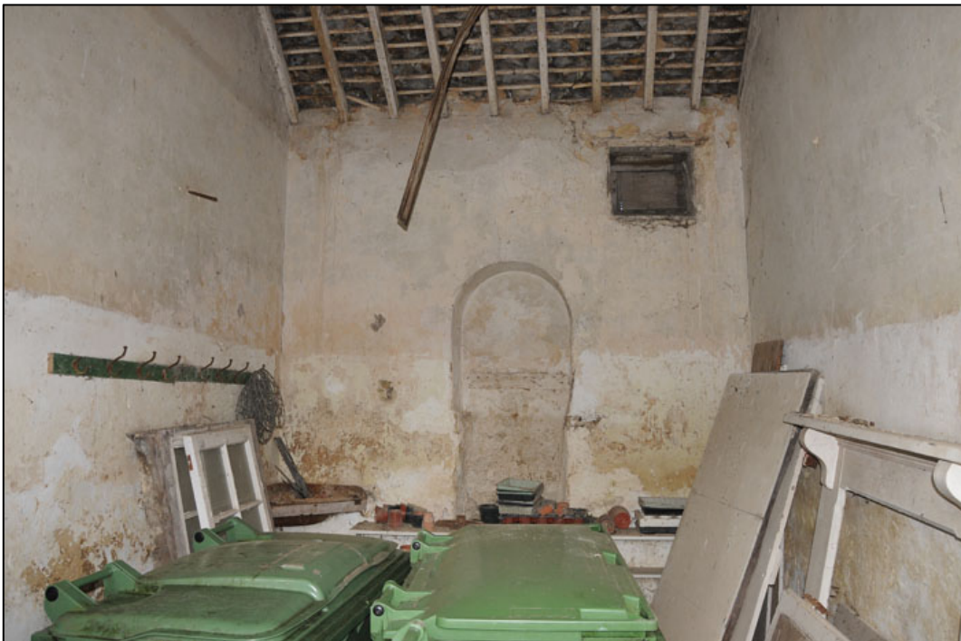
Appendix 3.28: Detail of interior of former loose box in stable block HA5 , looking north.
