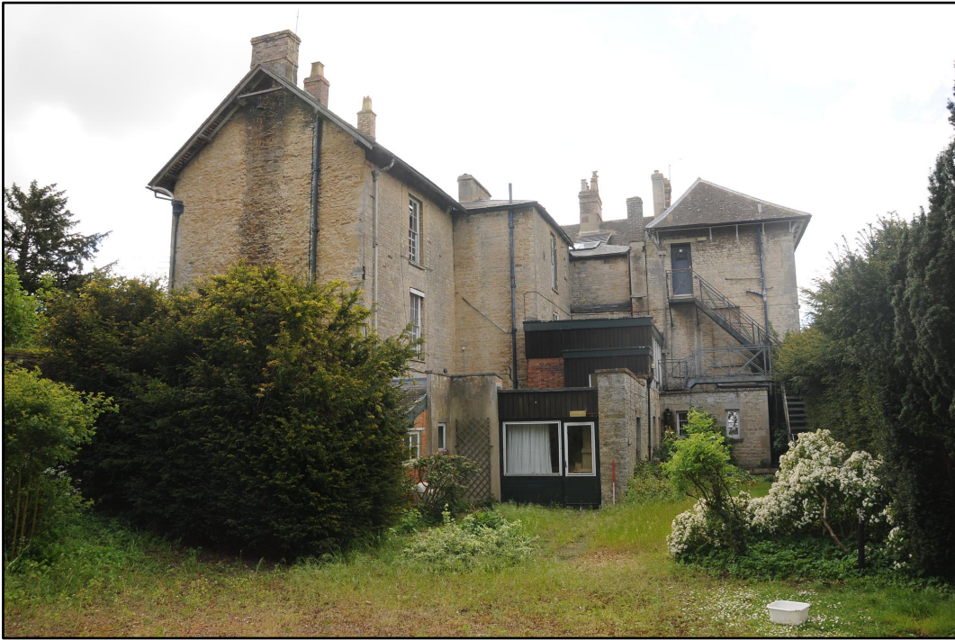
Appendix 3.55: General view of the northwest corner of Woodstock House, looking south (1m scale).
