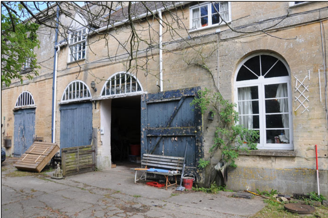
Appendix 3.22: Detail of looking northwest of coach doorways in south façade of Coach House HA4 (1m scale).
