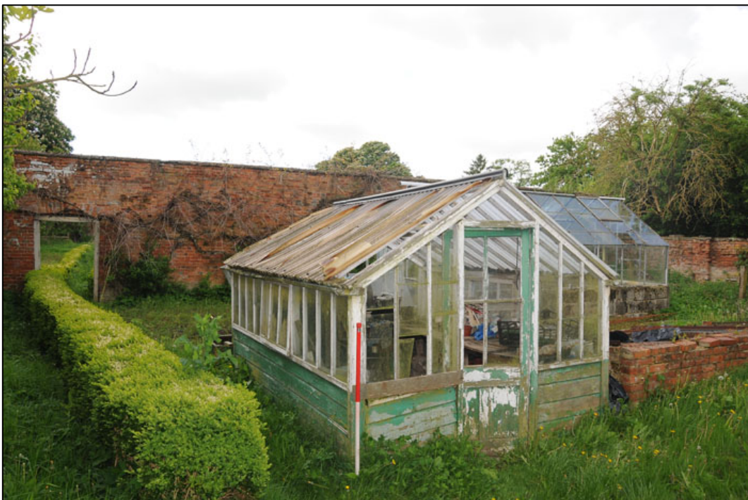
Appendix 3.40: Detail of wooden glass house in small walled garden HA14 , looking (1m scale).
