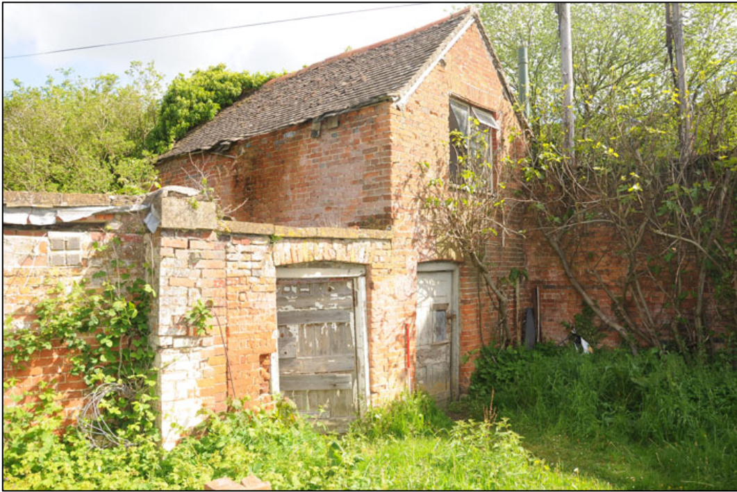
Appendix 3.29: General view of southwest corner of garden office/seed house HA6 , looking north (1m scale).
