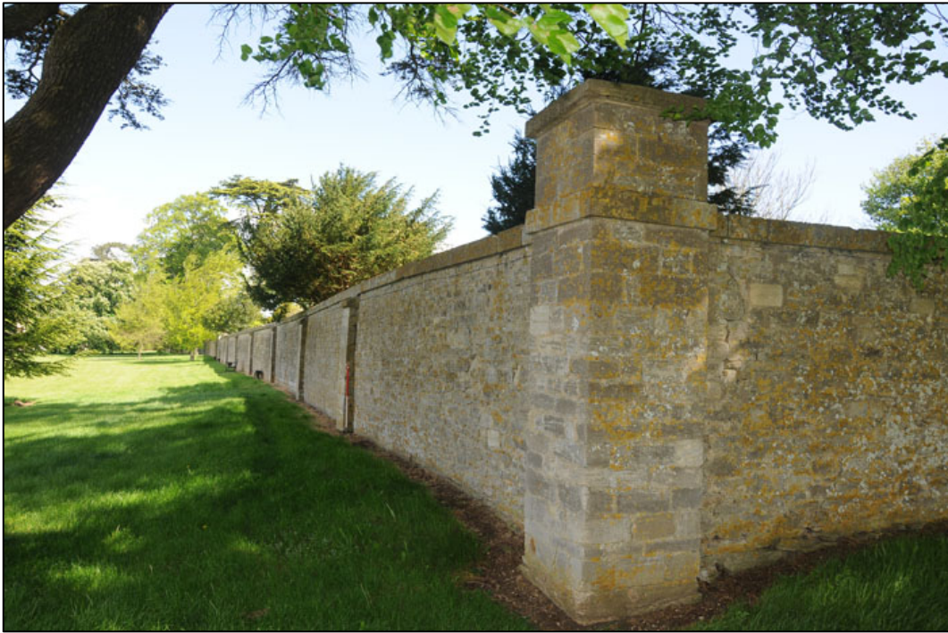
Appendix 3.35: General view of southwest corner of parkland boundary wall HA10 , looking north (1m scale).
