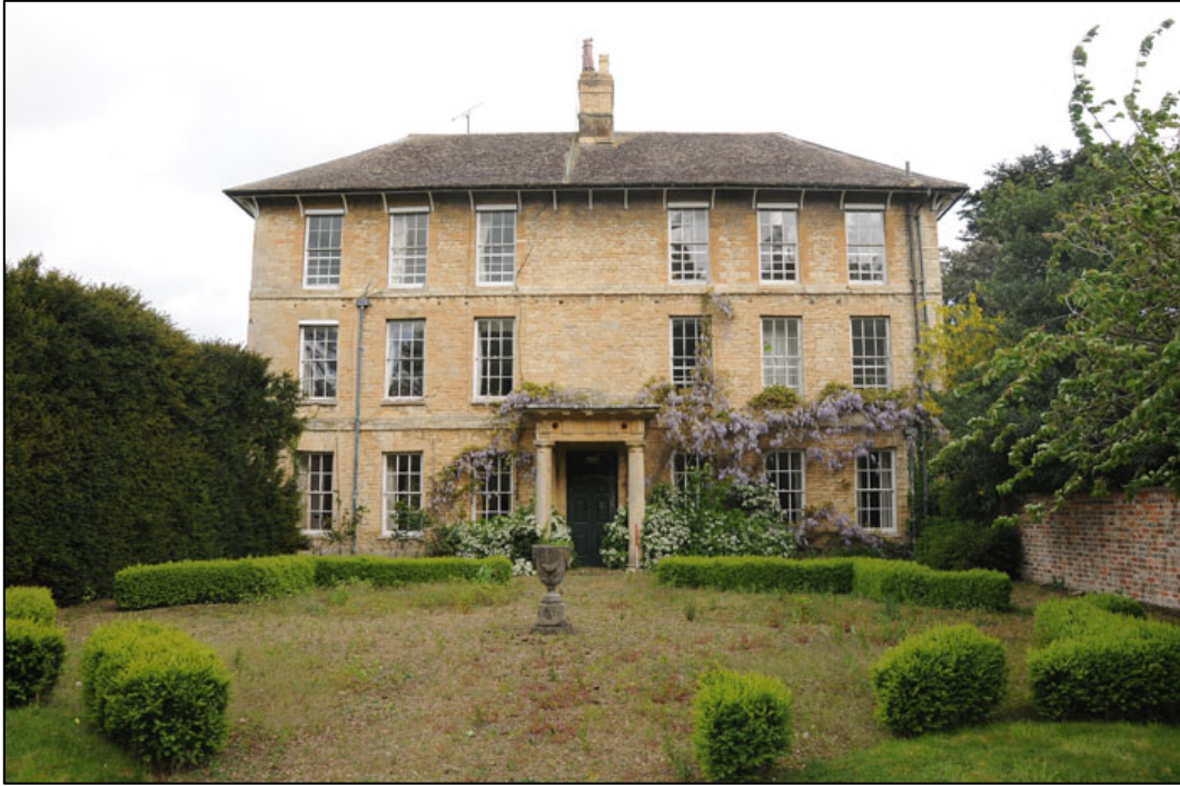
Appendix 3.1: General view of south elevation of Woodstock House HA1 ; note the row of timber sockets beneath the second floor string course (1m scale).
