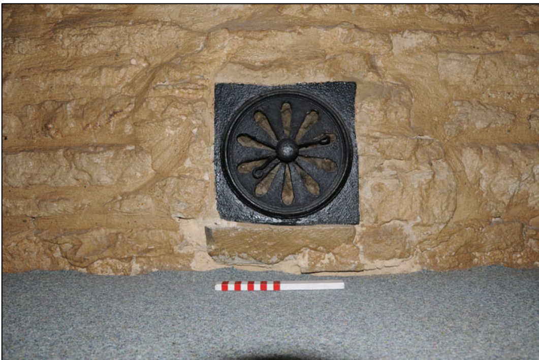
Appendix 3.26: Detail of in-situ cast-iron wall vent on first floor of Coach House HA4 (20cm scale).
