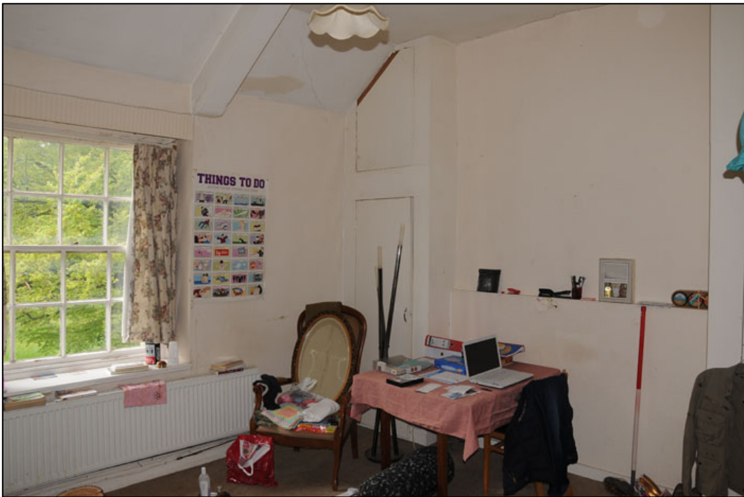
Appendix 3.24: Detail of interior room on first floor of Coach House HA4 (1m scale).
