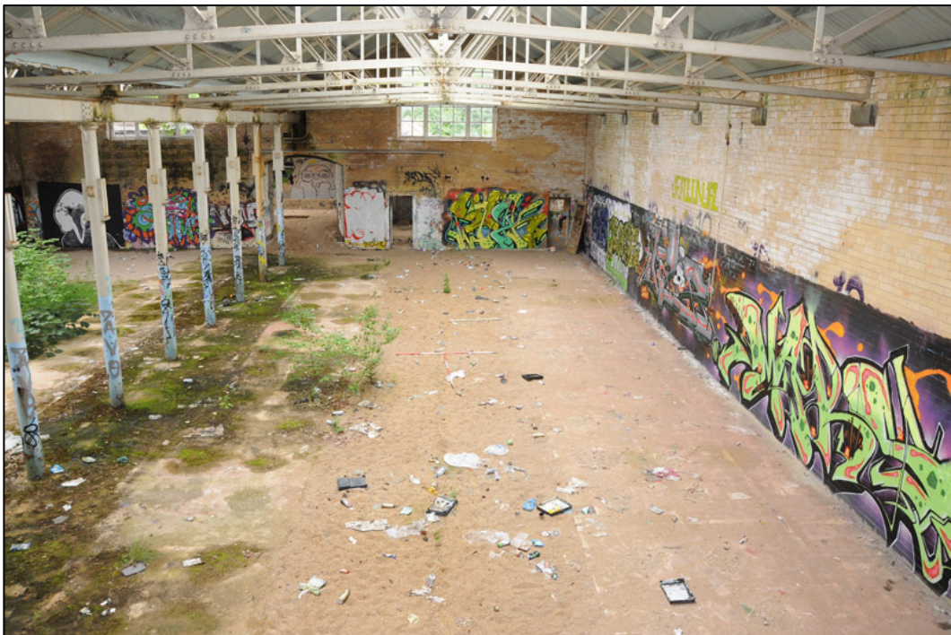
Appendix 2.33: General view of north floor bay of G6 ; note central area where pipework was located (2m scale).
