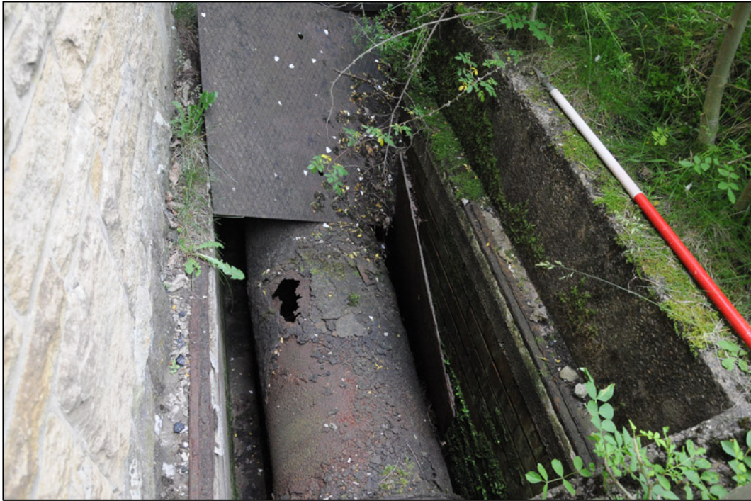
Appendix 2.13: Detail of in-situ water pipe alongside south external wall of G13 (1m scale).
