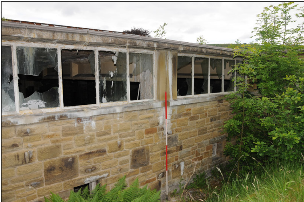
Appendix 2.12: Detail external stone walling and continuous upper glazing to G13 (2m scale).
