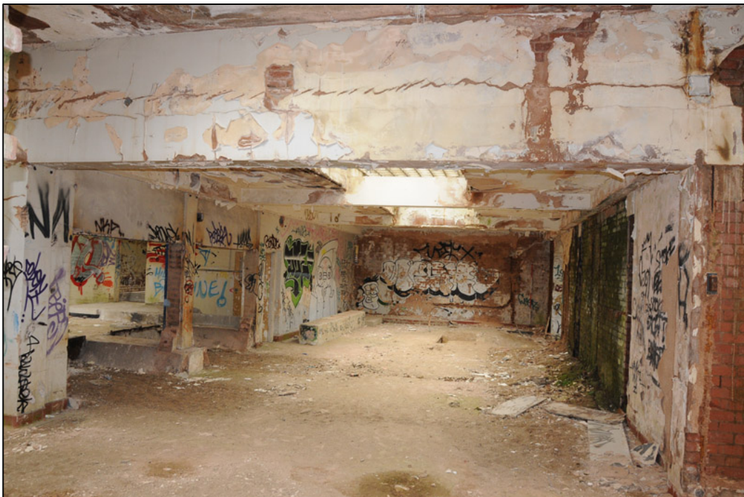
Appendix 2.18: General view of G10 , in West Extension; note concrete beams supporting roof (2m scale).
