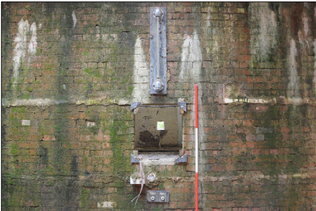
Appendix 2.20: Detail of pressure gauge and switches in south wall of G15 (2m scale).
