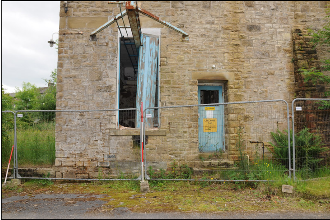
Appendix 2.7: Detail of taking-in door to G1; note inserted hoist (2m scale).
