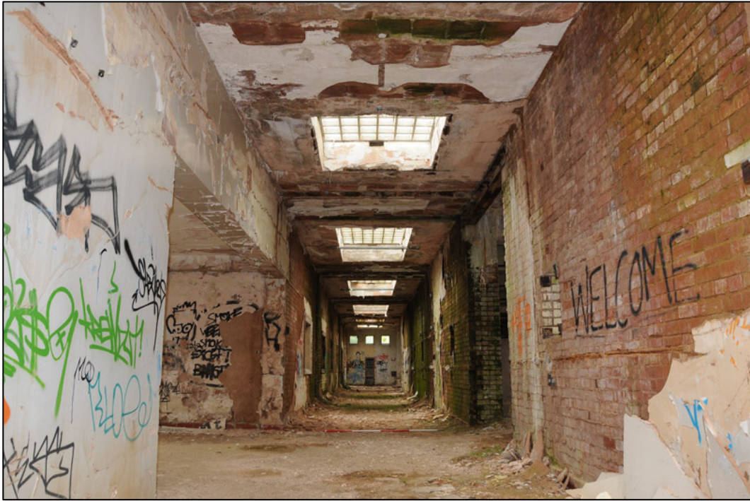
Appendix 2.17: General view of central corridor G15 , in South Extension (2m scale).
