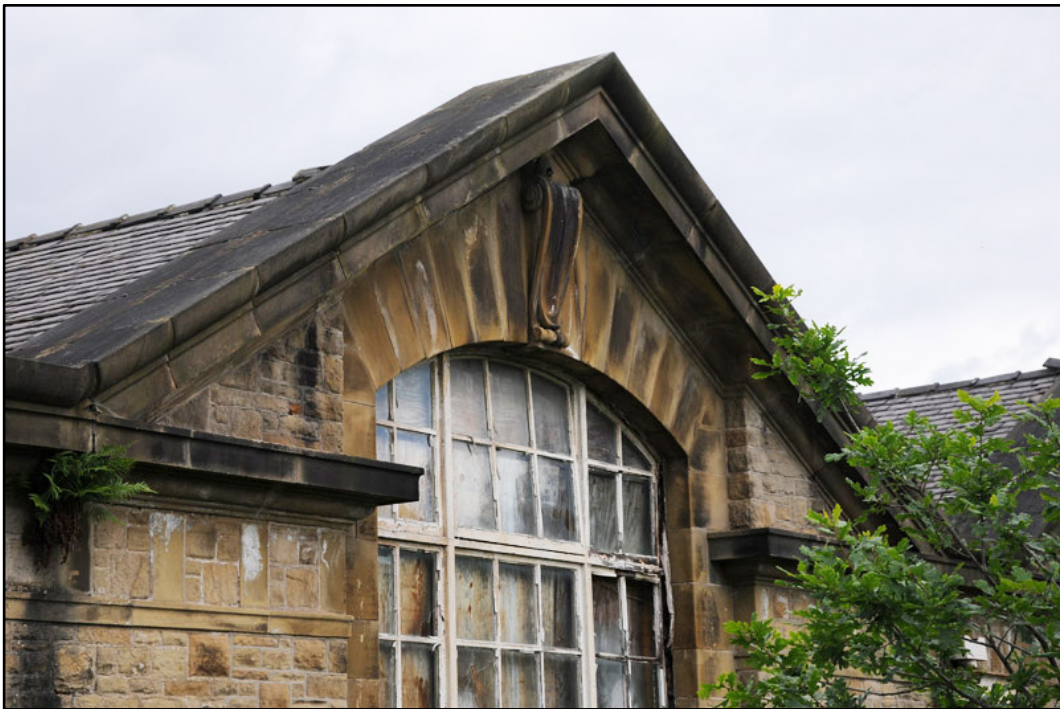
Appendix 2.6: Detail of keystone on Filtration Building in the form of a console bracket; note broken pediment.
