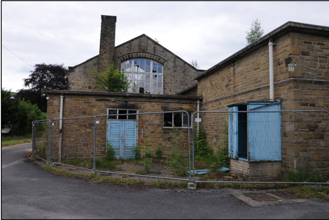
Appendix 2.9: General view of rear elevation of Filtration Building; note 1950s extension and chimney (2m scale).
