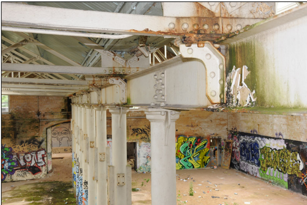
Appendix 2.35: Detail of central girder in G6; foreground represents site of removed column.
