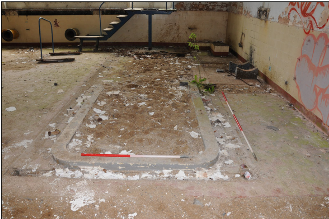
Appendix 2.22: Detail of foundations for removed plant in G14, looking east (1m/2m scale).
