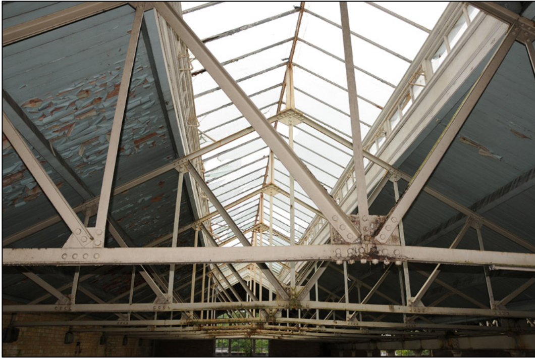
Appendix 2.32: Detail of metal roof truss above G6 ; note glazed clerestory windows forming skylight.
