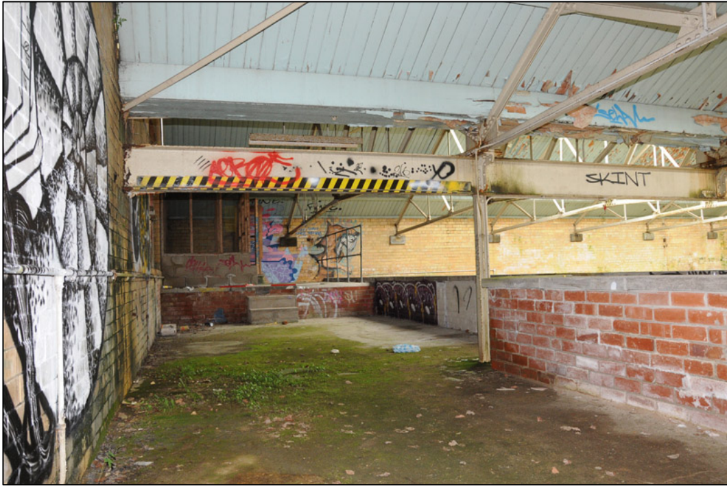
Appendix 2.34: General view of mezzanine level in G6; note wire cages against southeast corner (2m scale).
