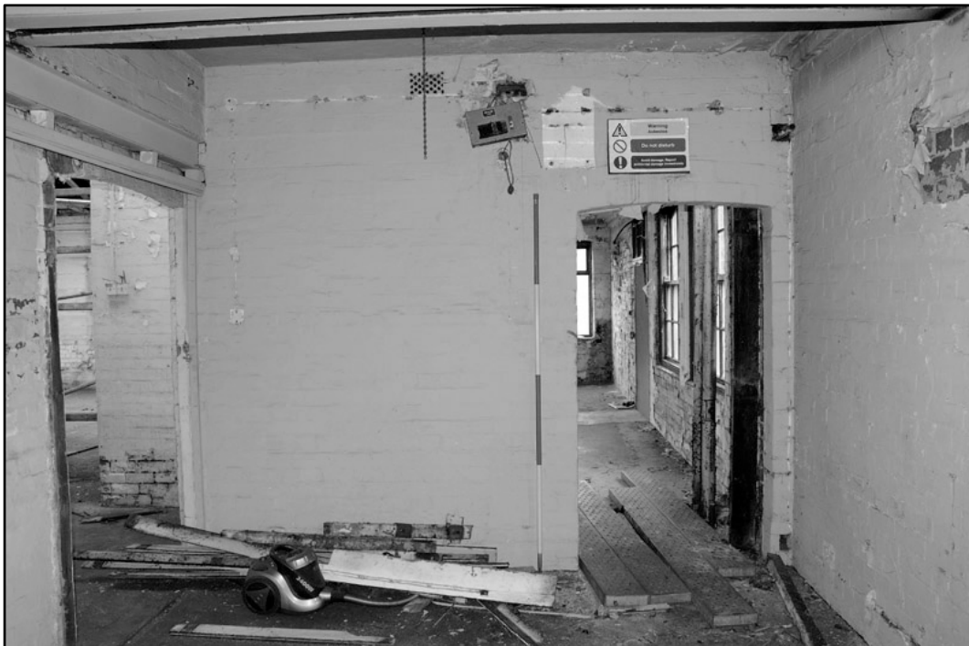
Appendix 4.28: General view of first floor room in frontage building, looking west; Film 1.31 (2m scale).
