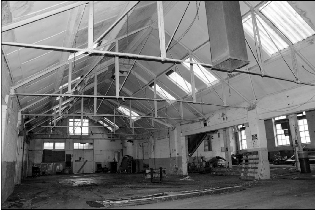
Appendix 4.15: Detail of metal roof trusses in central area, looking south; Film 1.17 (2m scale).
