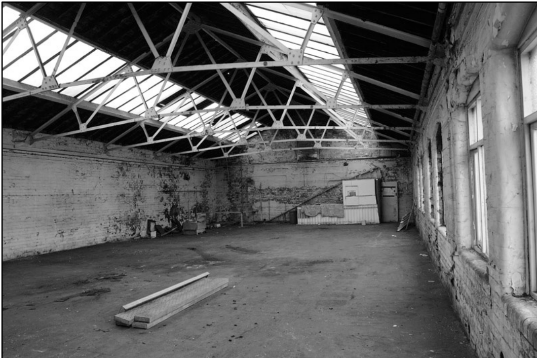
Appendix 4.26: General view of first floor of frontage building, looking southeast; Film 1.28 (2m scale).
