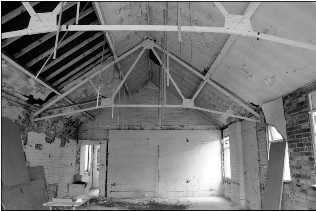
Appendix 4.23: General view of first floor offices in frontage building, looking east; Film 1.25 (2m scale).
