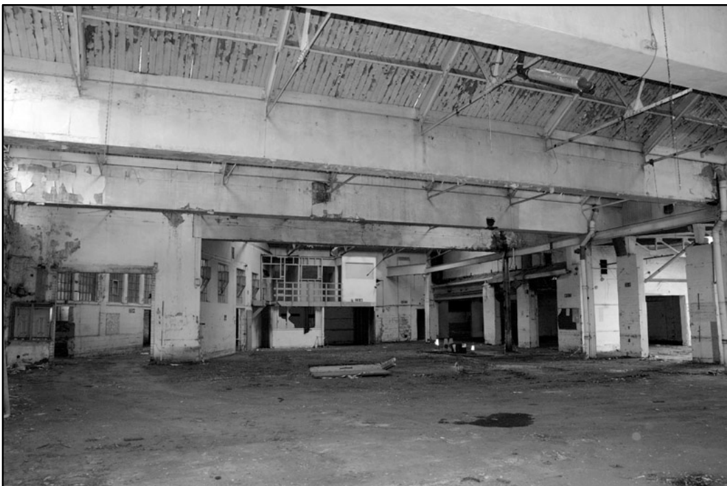
Appendix 4.10: Detail of north light roof structure, looking west; Film 1.12 (2m scale).
