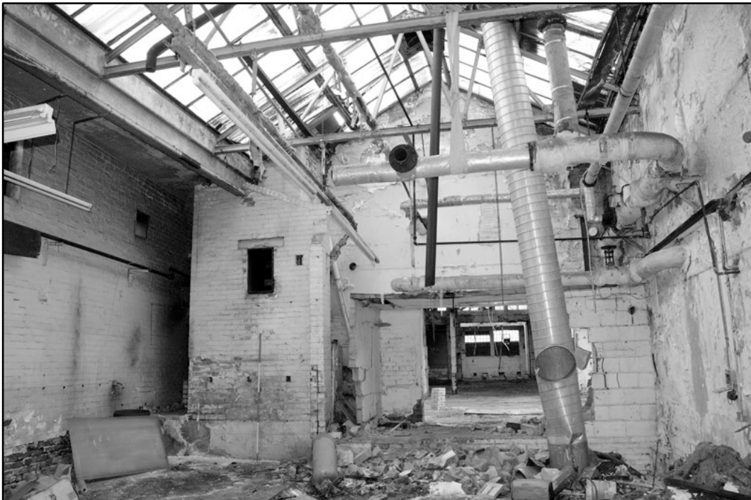
Appendix 4.16: Detail of remains of boiler house and chimney, looking east; Film 1.18 (2m scale).
