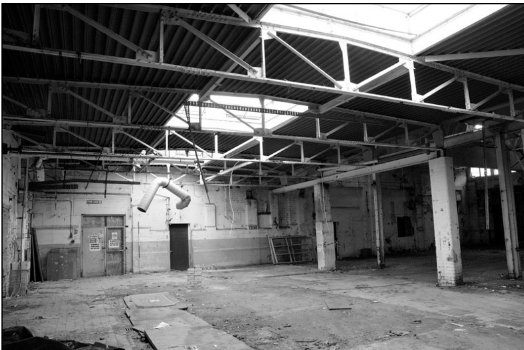
Appendix 4.12: General view of central area, looking northeast; note flat roof; Film 1.14 (2m scale).
