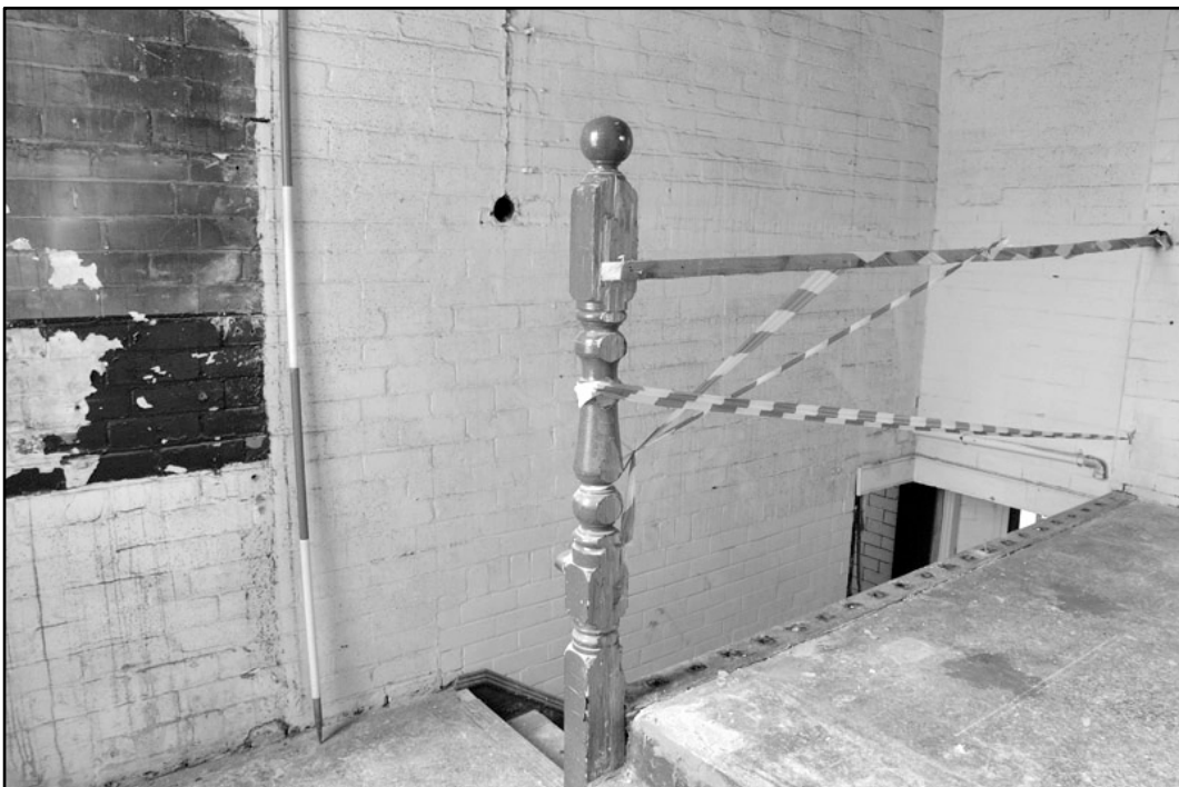
Appendix 4.24: Timber newel for rear staircase in frontage building, looking southeast; Film 1.26 (2m scale).
