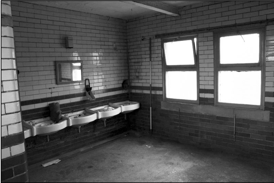
Appendix 4.32: Detail of first floor toilet in frontage building, looking southwest; Film 1.34 (2m scale).
