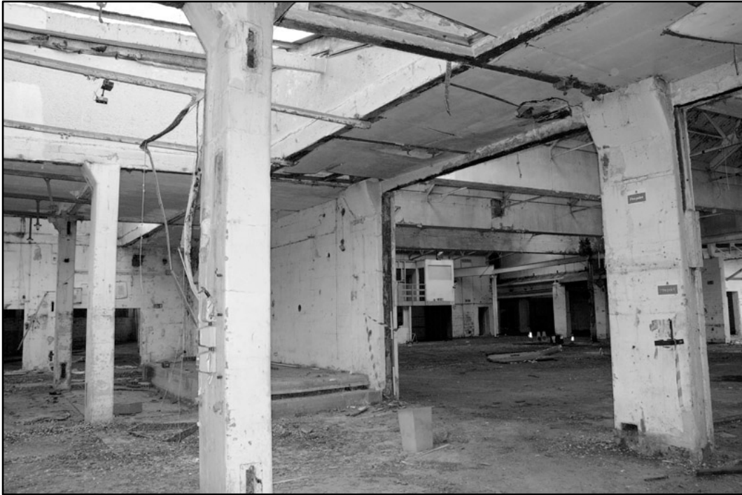
Appendix 4.9: General view looking into central section of the Site, looking southwest; Film 1.11 (2m scale).
