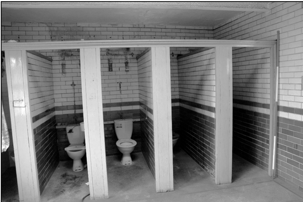
Appendix 4.33: Detail of first floor toilet in frontage building, looking northeast; Film 1.35 (2m scale).
