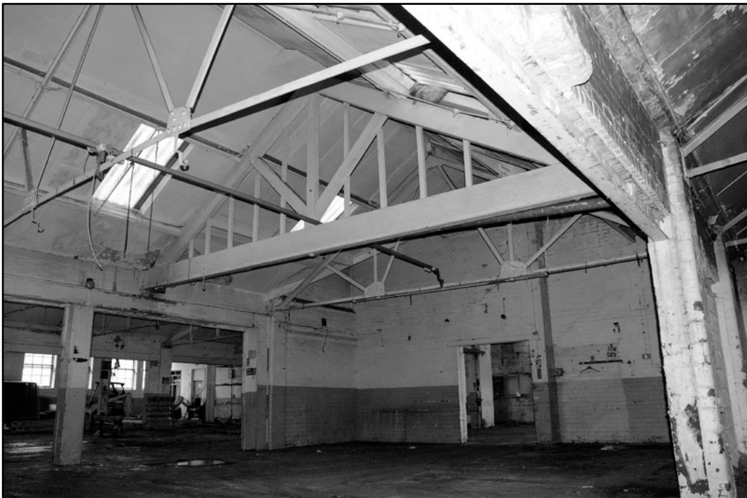
Appendix 4.14: Detail of timber roof truss in central area, looking northwest; Film 1.16 (2m scale).
