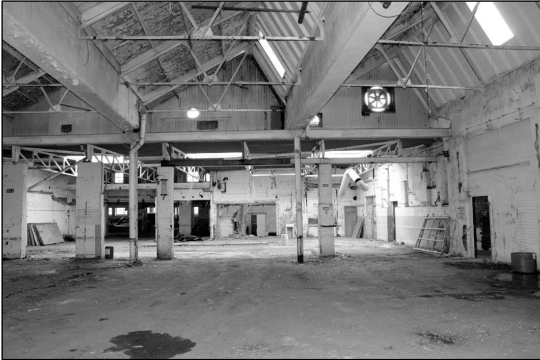
Appendix 4.11: Detail of north light roof structure, looking west; Film 1.13 (2m scale).
