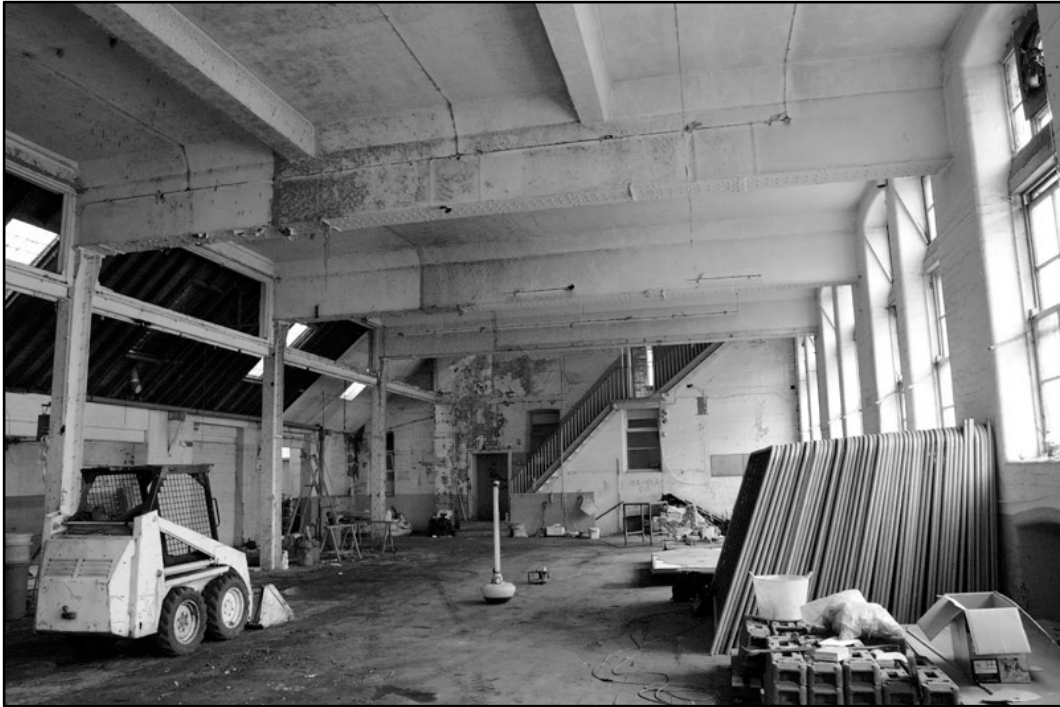
Appendix 4.19: General view of ground floor of frontage building, looking southwest; Film 1.21 (2m scale).
