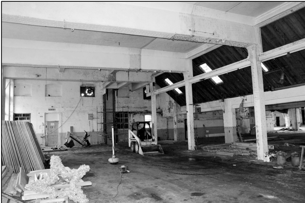
Appendix 4.18: General view of ground floor of frontage building, looking northeast; Film 1.20 (2m scale).
