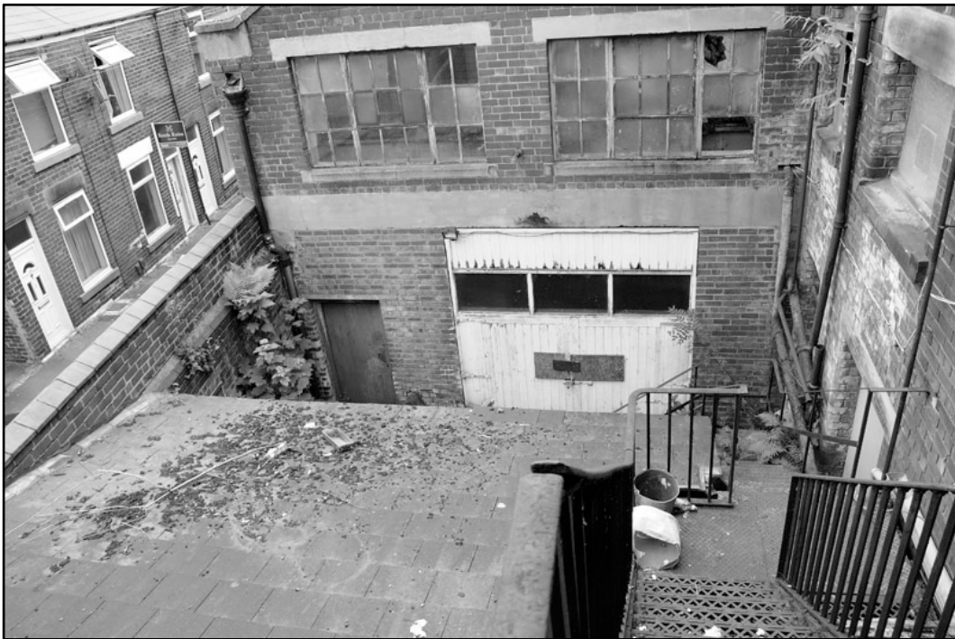
Appendix 4.31: General view of exterior of boiler house, looking east; note cast-iron staircase; Film 1.33.
