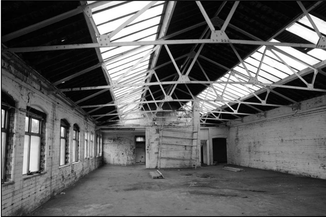
Appendix 4.25: General view of first floor of frontage building, looking northeast; Film 1.27 (2m scale).
