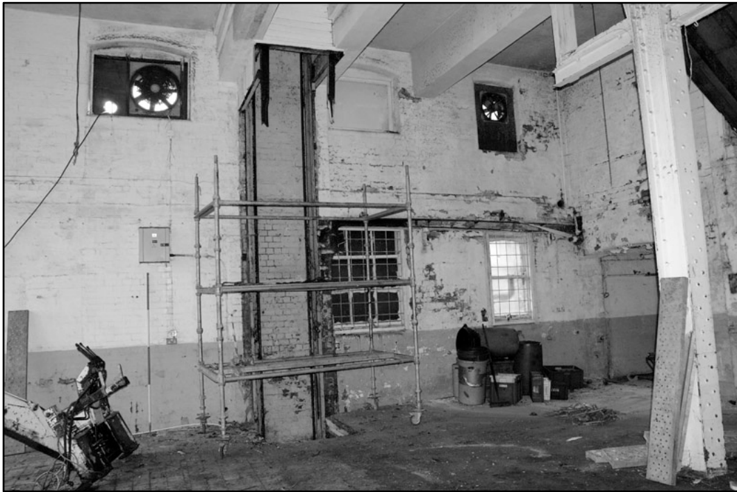
Appendix 4.17: Detail of remains of goods hoist in frontage building, looking north; Film 1.19 (2m scale).
