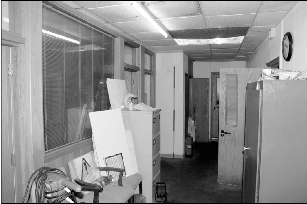
Appendix 4.21: General view of office partitions in frontage building, looking southwest; Film 1.23 (2m scale).
