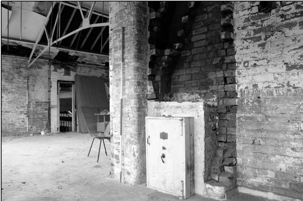
Appendix 4.22: General view of first floor office in frontage building, looking northeast; Film 1.24 (2m scale).
