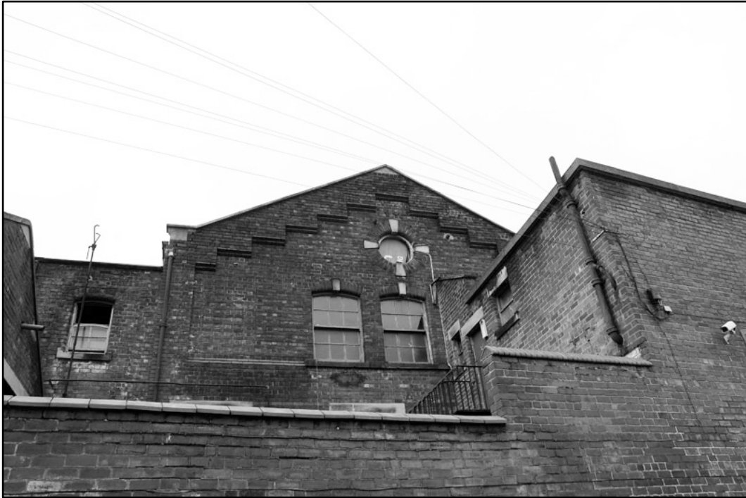
Appendix 4.3: Detail of decorated gable on frontage building, overlooking Coniston Terrace; Film 1.4 (2m scale).
