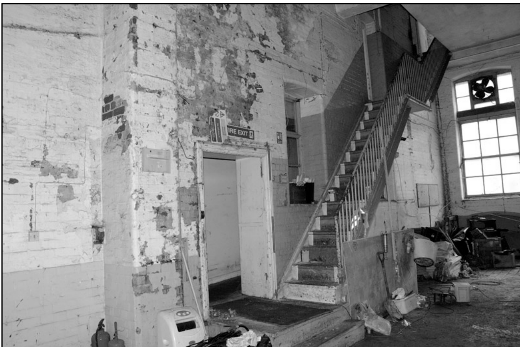
Appendix 4.20: Detail of staircase in frontage building, looking southwest; Film 1.22 (2m scale).
