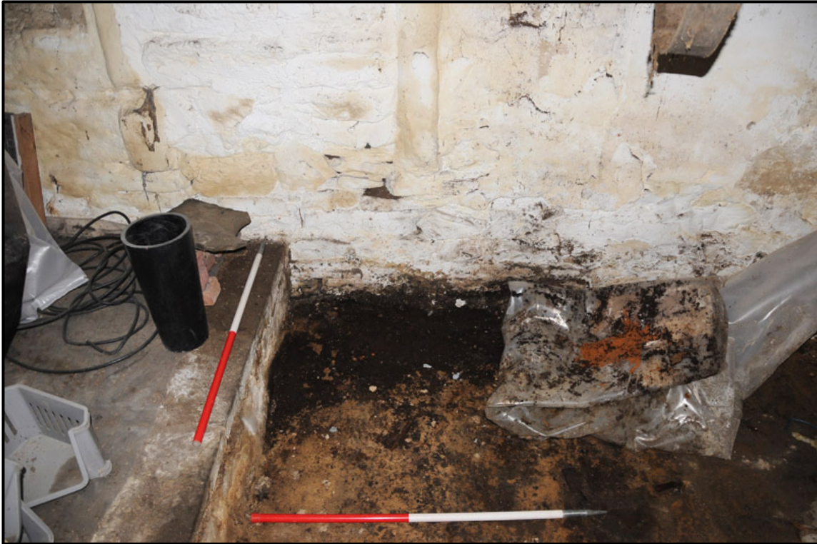
Appendix 3.1: General view of Trial Hole 1 before excavation, looking east (1m scale).
