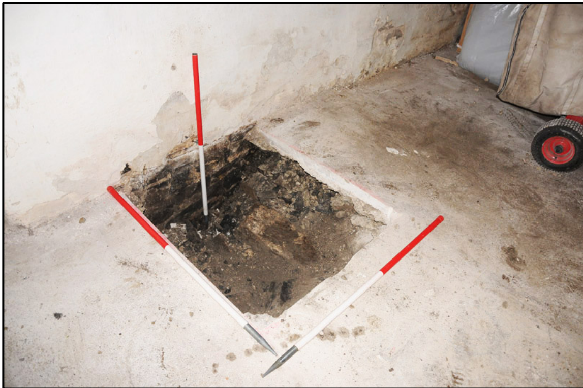
Appendix 3.6: Trial Hole 3 after excavation looking southeast; note wall face continues downwards (1m scale).
