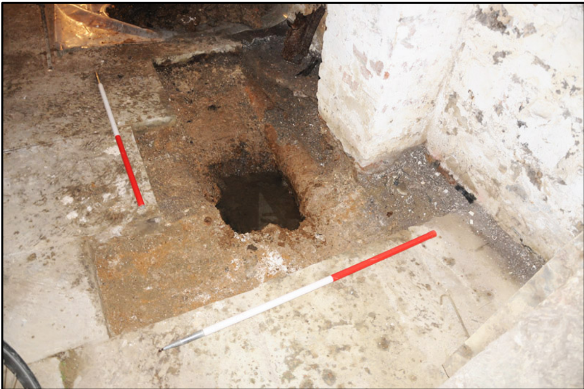
Appendix 3.4: General view of Trial Hole 2 after excavation looking south; note ceramic pipe (1m scale).
