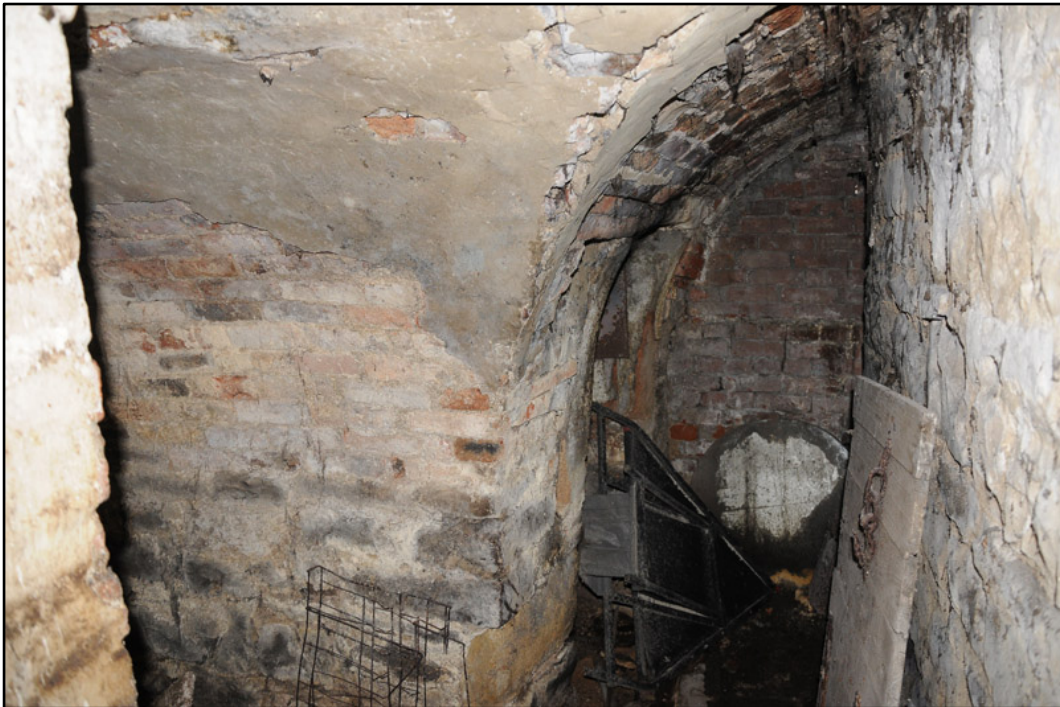
Appendix 5.25: Detail of vaulting supporting superstructure of corn drying kiln at east end of the south range.
