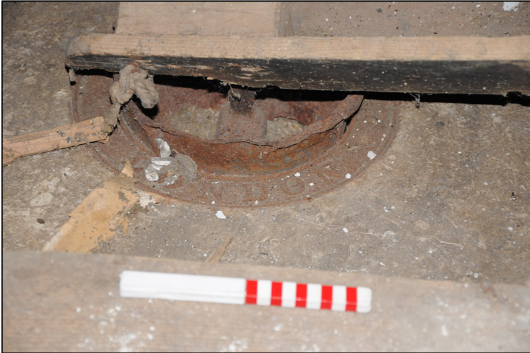
Appendix 5.31: Detail of central hub of grinding wheel on first floor, looking east (20cm scale).
