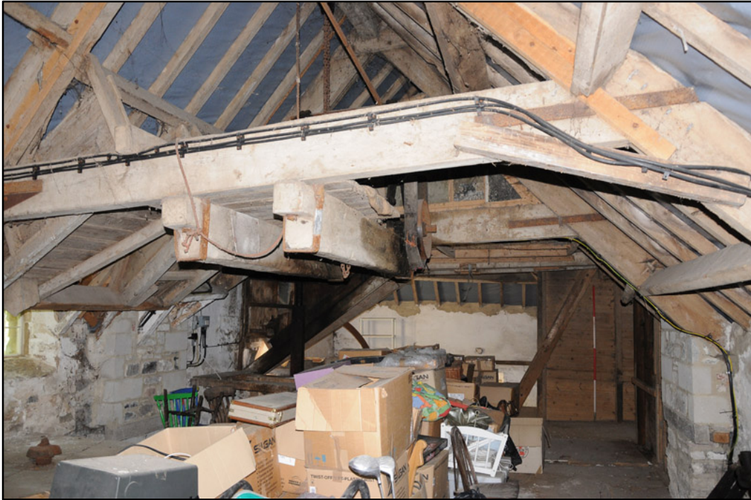
Appendix 5.26: General view of first floor of south range, looking west (2m scale).
