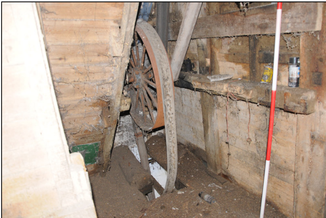
Appendix 5.34: Detail of belt driven transmission drives for trap door hoist on first floor of west range (2m scale).
