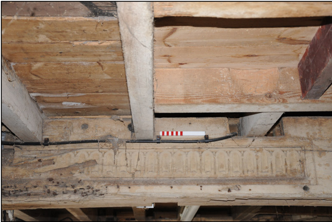
Appendix 5.21: Detail of reused timber beam to support first floor ceiling of south range (20cm scale).
