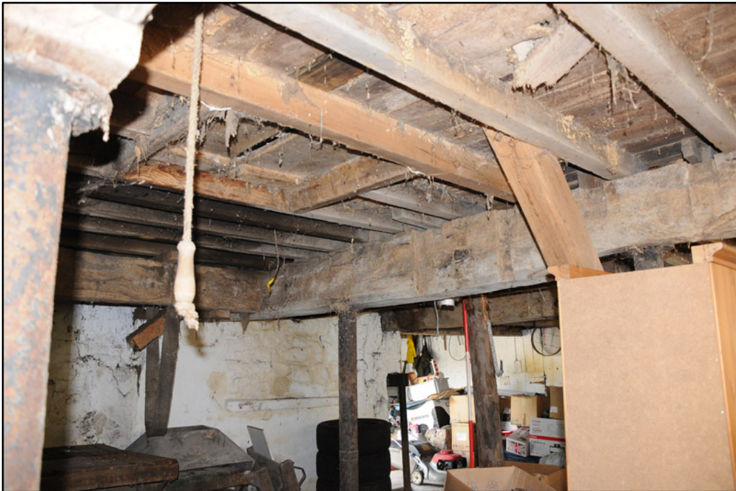
Appendix 5.16: General view of ground floor of west range, looking northeast; note trapdoor in ceiling (2m scale).
