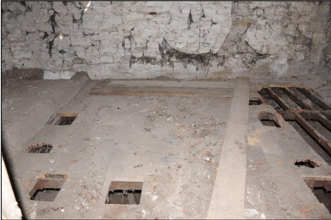
Appendix 5.28: General view of tiled floor of corn drying kiln, looking south; note metal girders.
