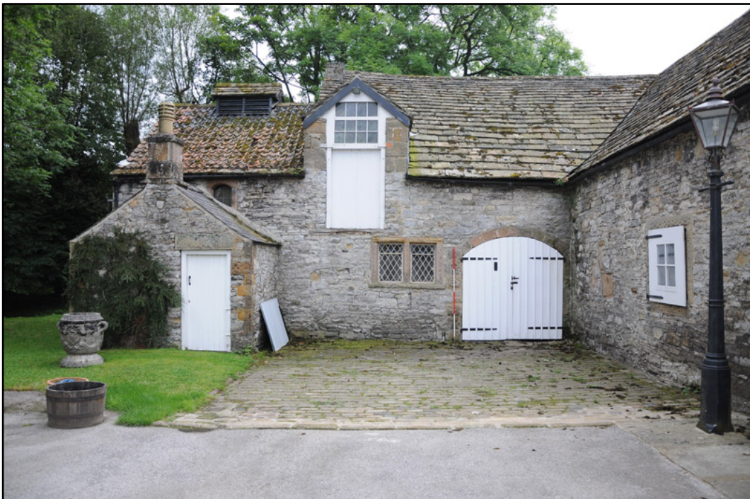
Appendix 5.2: Detail view of north elevation, looking south; note inserted taking-in door (2m scale).
