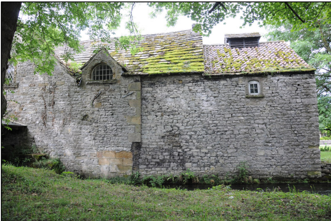
Appendix 5.8: Detail of south elevation alongside the river; note changes in stonework.
