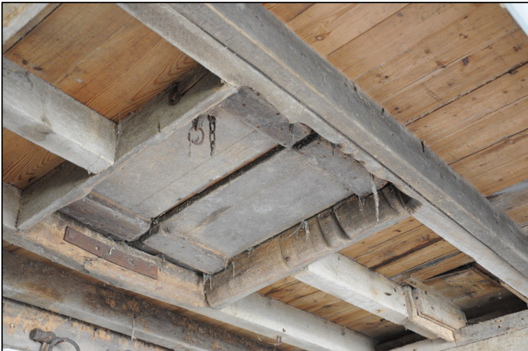
Appendix 5.22: Detail of trap door to first floor of the south range; note wear marks from pulley ropes.
