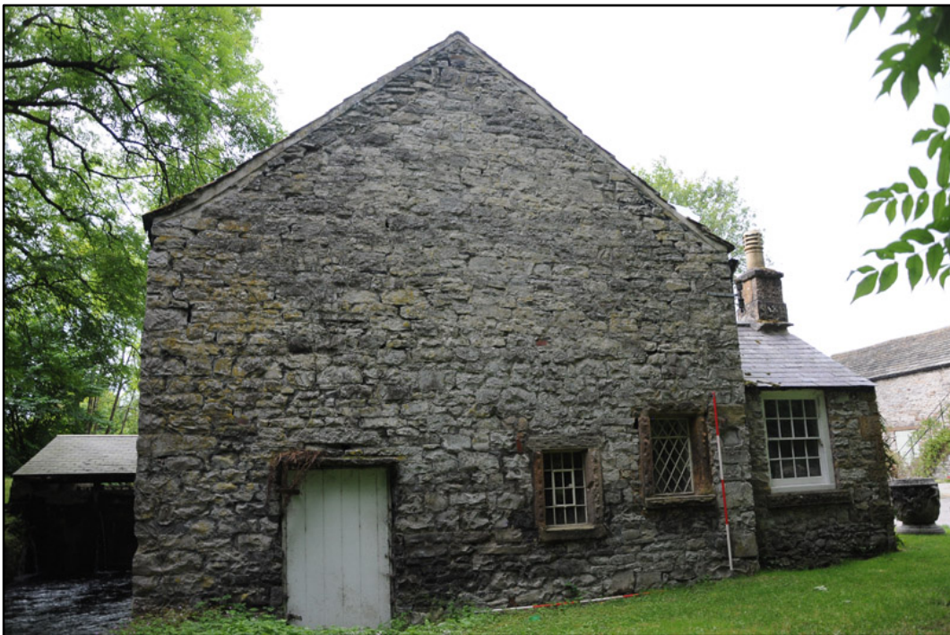
Appendix 5.10: General view of east elevation of south range, looking west (2m scale).
