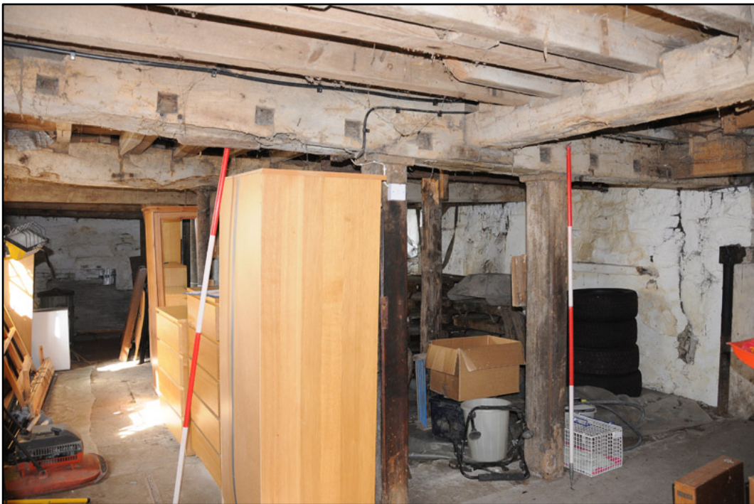
Appendix 5.18: General view of ground floor of west range, looking north; note redundant mortices (2m scale).
