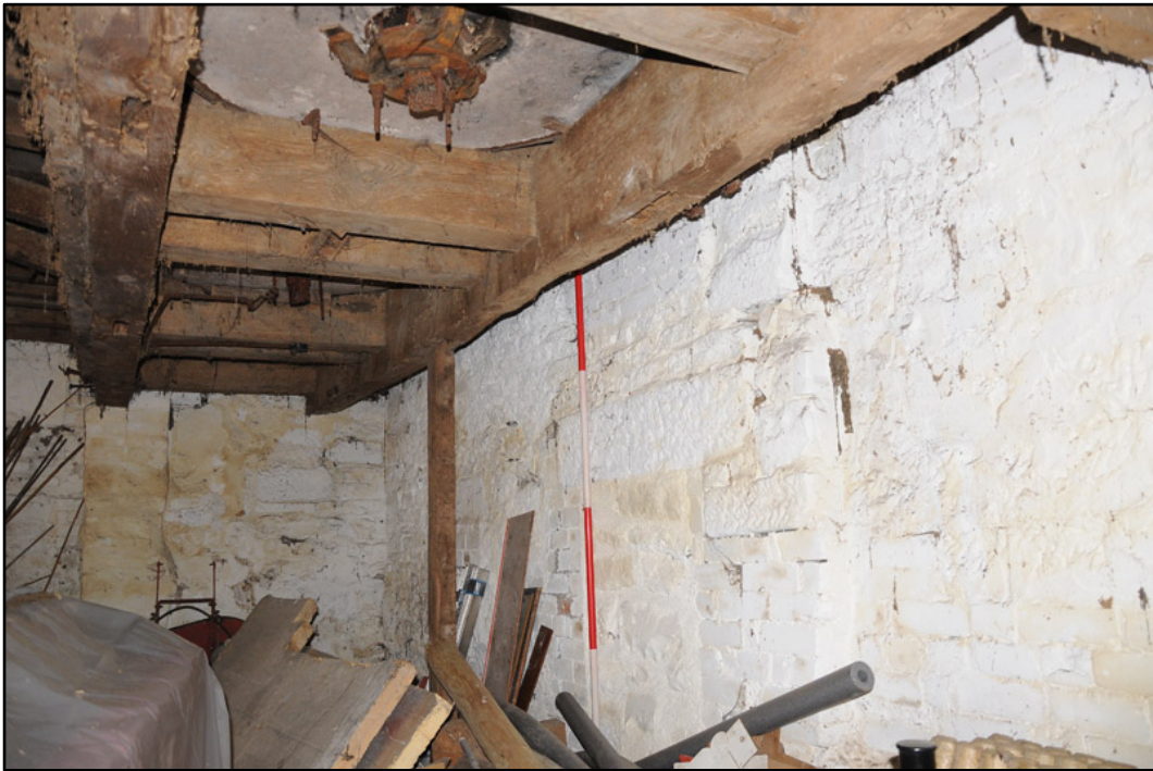
Appendix 5.15: Detail of internal north wall of west range, looking northwest; note blocking (2m scale).
