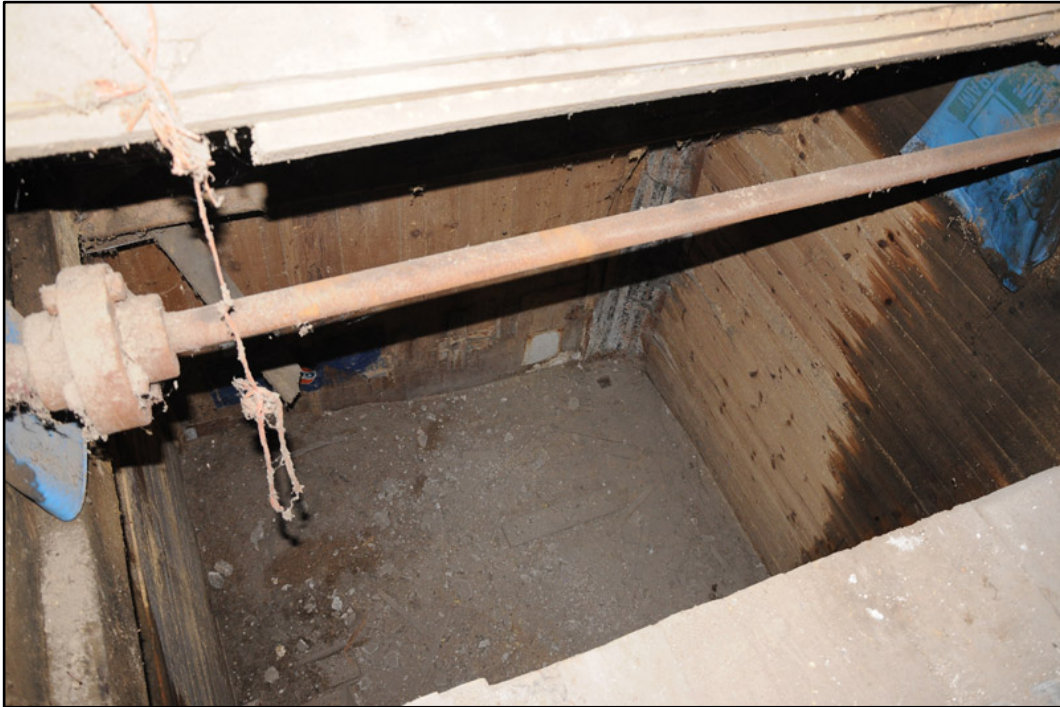
Appendix 5.37: View looking down into timber grain storage bin on first floor of west range.
