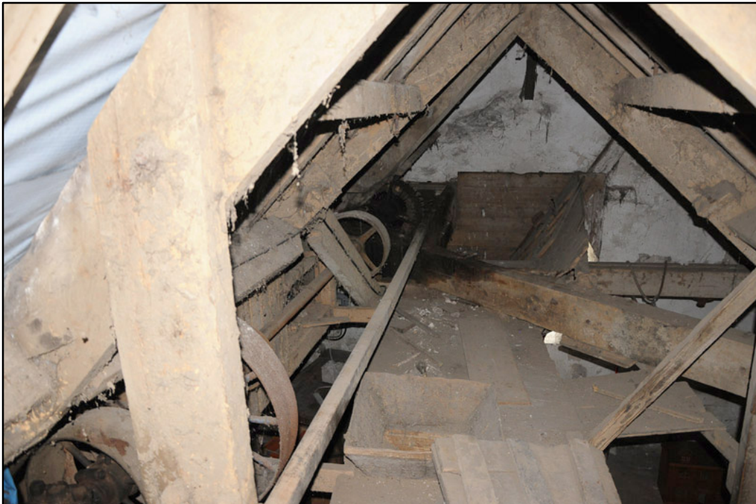
Appendix 5.38: General view looking south along second floor walkway above west range.
