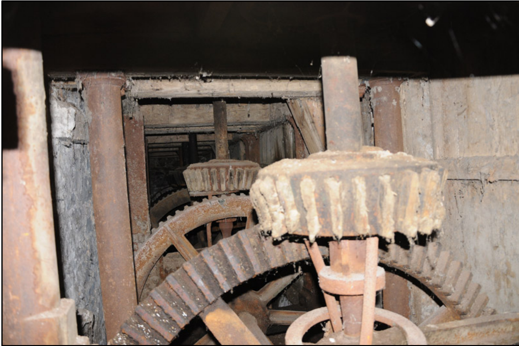
Appendix 5.24: Detail of in-situ machinery along south wall of south range, looking west.
