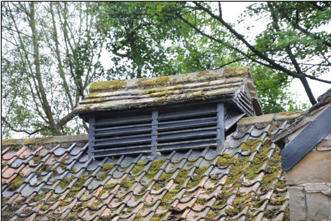
Appendix 5.6: Detail of louvered vent above kiln in east end of the building.
