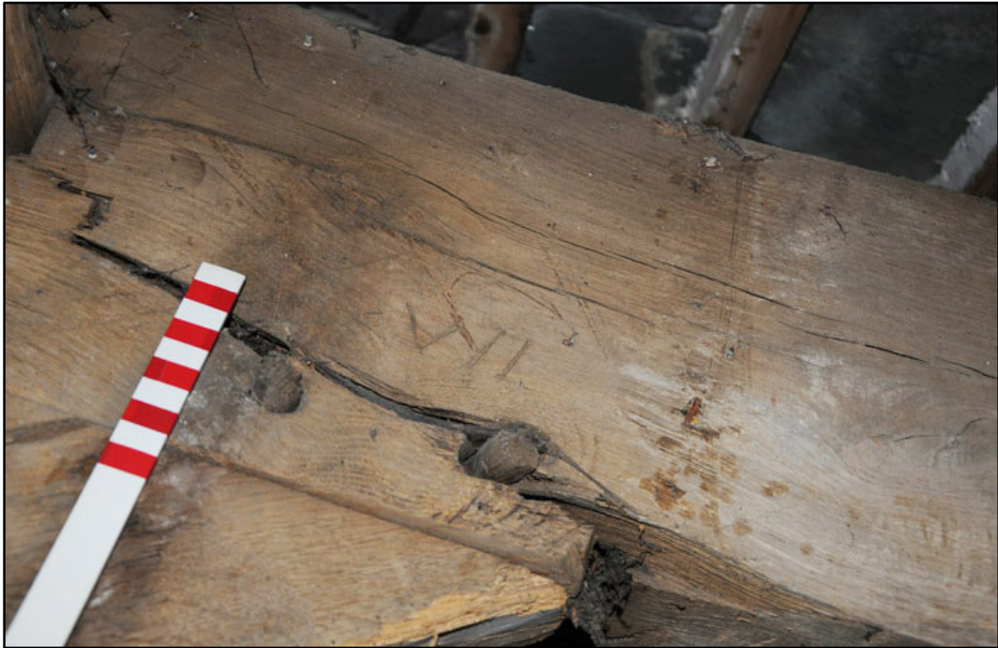
Appendix 3.33: Detail of assembly marks and fixing pegs on roof truss in T1 (10cm scale).
