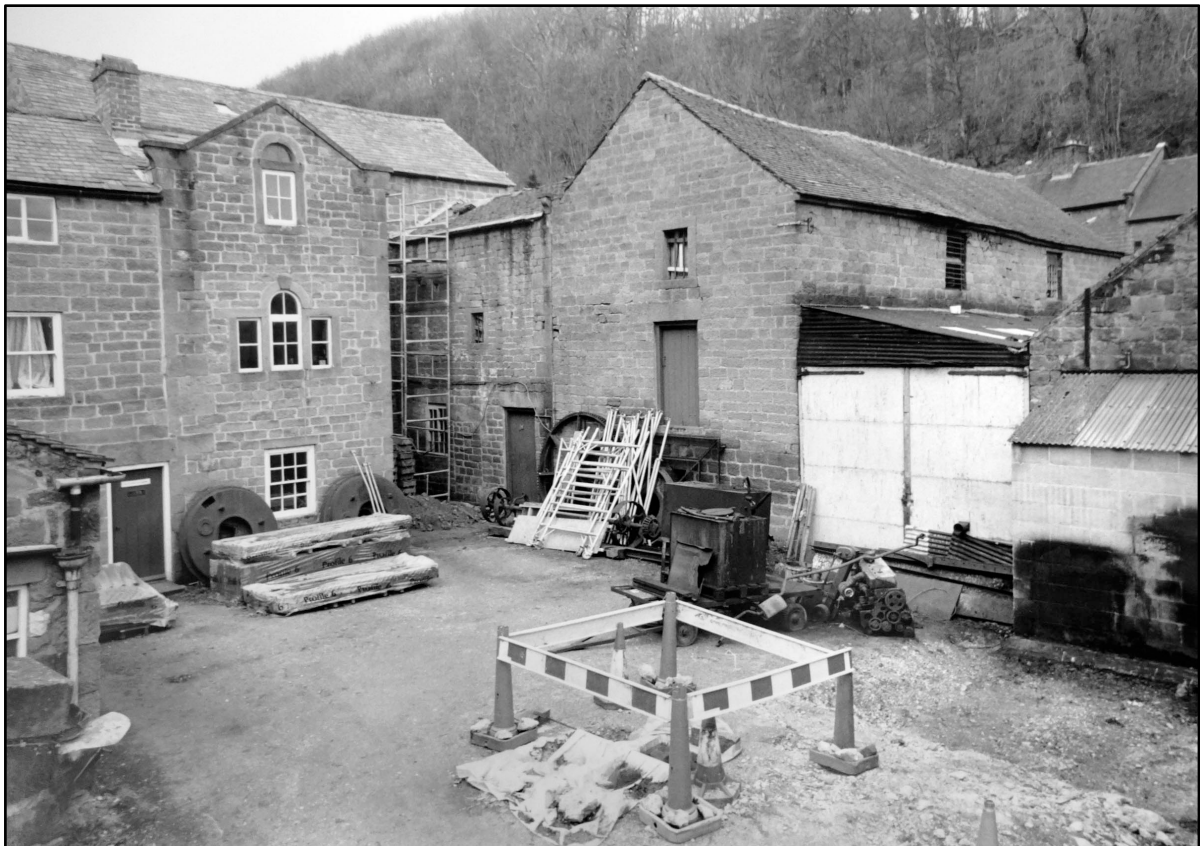
Appendix 2.4: View of east yard during repairs to adjacent buildings in 1994 © R. Freestone and Derbyshire Record Office
