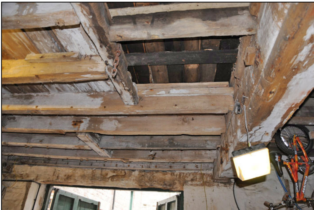
Appendix 3.8: Detail of exposed ceiling joists of G1, looking east; note trapdoor opening and rope scars.
