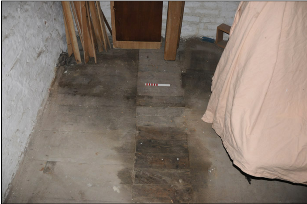
Appendix 3.28: Detail of blocked floor opening in the southeast corner of SI (20cm scale).
