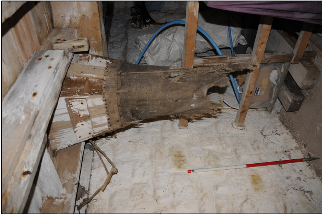
Appendix 3.18: Detail of hopper chute in ceiling of FI, looking east (1m scale).
