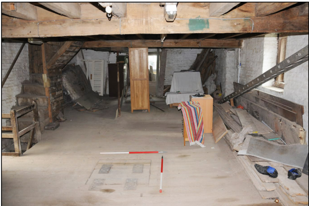
Appendix 3.23: General view of SI, looking north; note staircase up to TI and trapdoor in the floor (1m scale).
