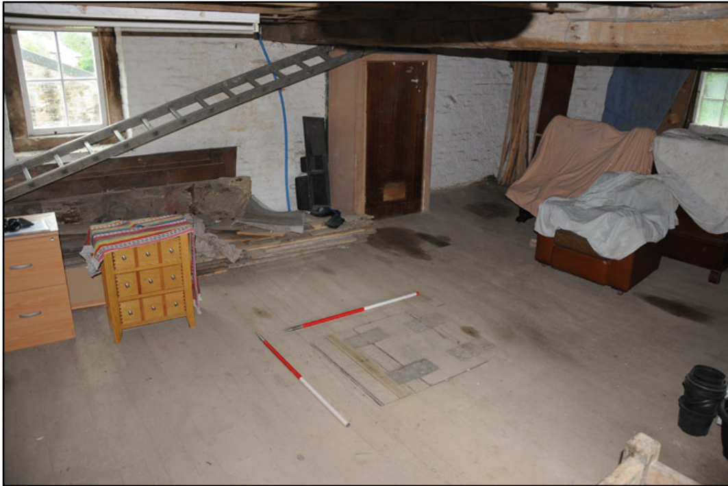
Appendix 3.22: Detail of southern end of SI, looking south; note in-situ trap door (1m scale).
