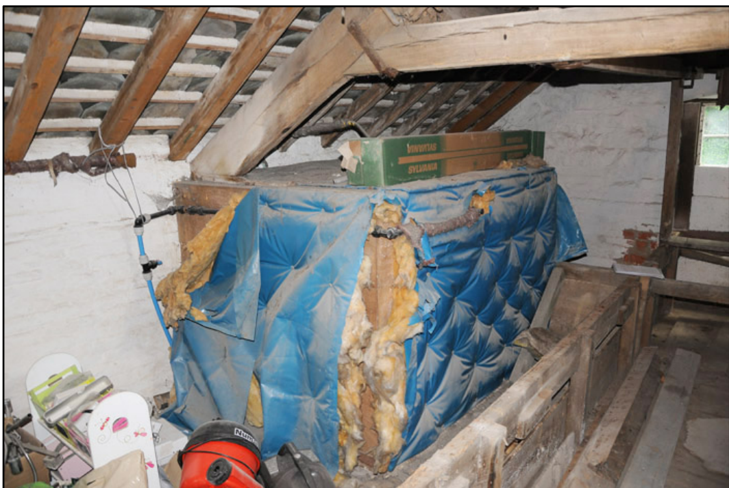
Appendix 3.36: Detail of modern water tank against east wall of TI; note raised tie beam secured with iron strap.
