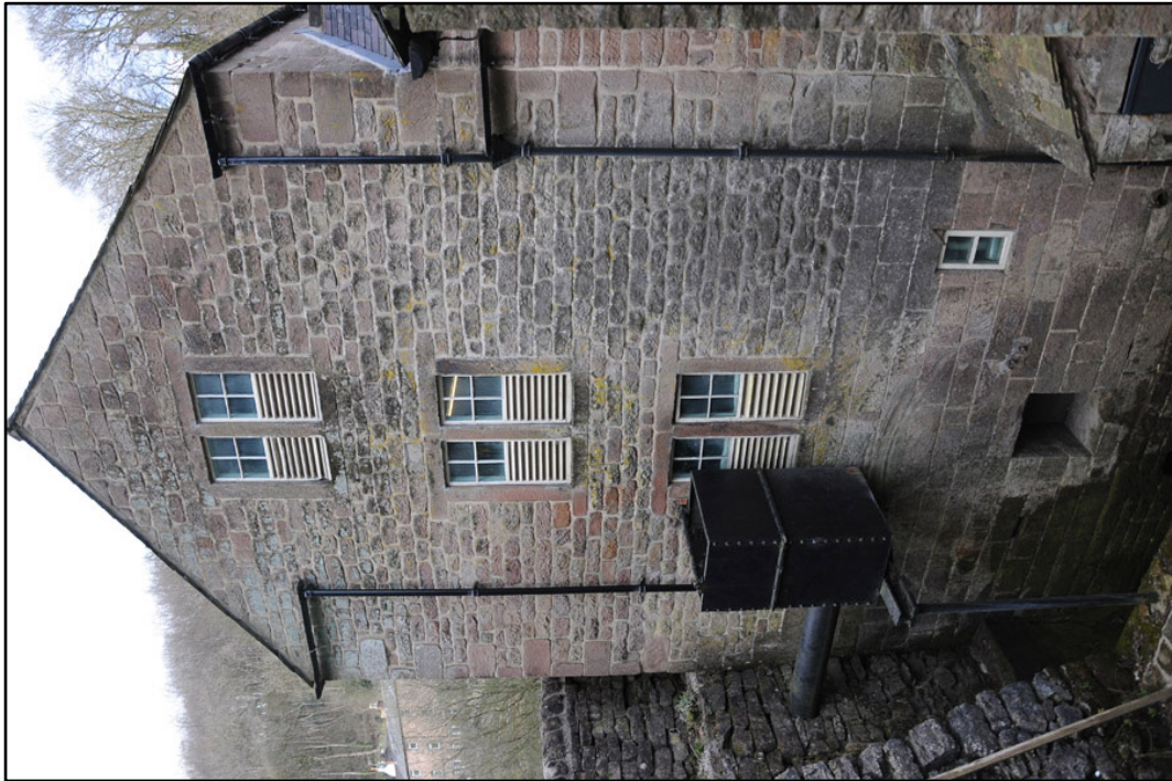
Appendix 3.5: View of south gable; note centrally positioned windows with louvers and tank forming pentrough.
