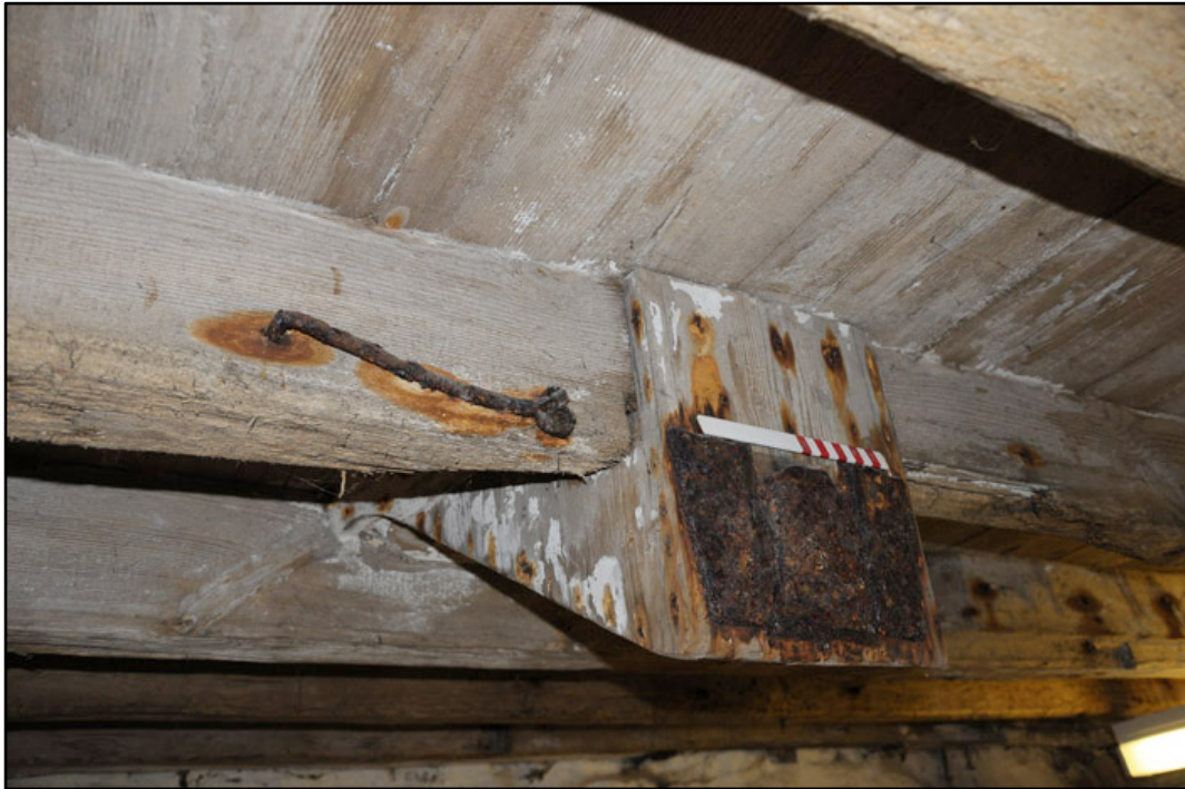
Appendix 3.16: Detail of hopper feed from former grain chute on the ceiling of FI (20cm scale).
