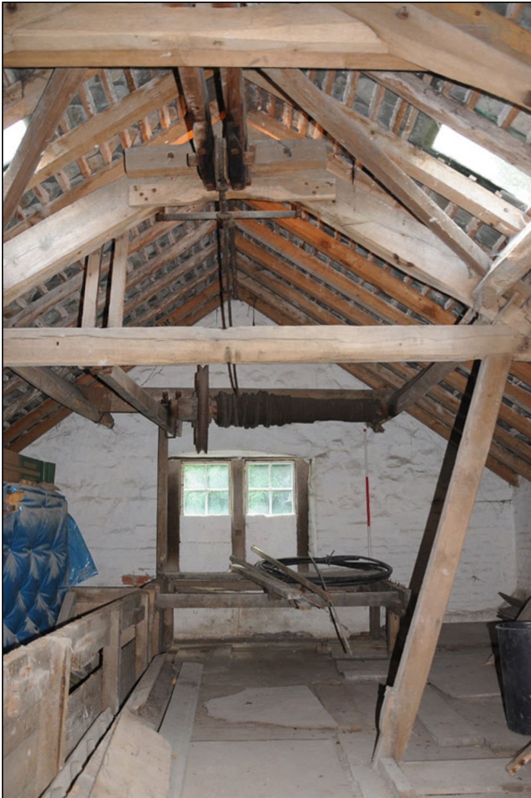
Appendix 3.30: General view of south end of T1; note ceiling mounted winch for sack hoist (2m scale).
