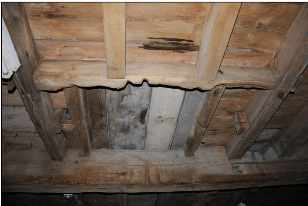
Appendix 3.25: Detail of trapdoor opening in ceiling of S1; note grooves from rope of sack hoist (1m scale).
