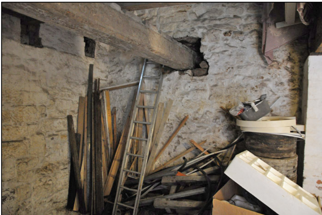
Appendix 3.13: Detail of southwest corner of G1; note recently inserted beam and empty joist sockets (1m scale).
