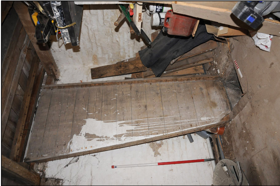
Appendix 3.26: Detail of surviving section of former grain chute in southwest corner of S1 (20cm/1m scale).
