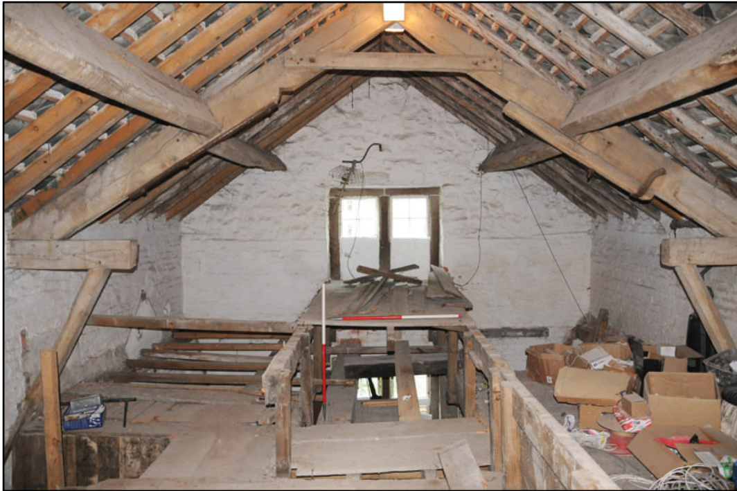
Appendix 3.35: General view of TI, looking north; note inserted platform and sawn off tie-beam (1m scale).
