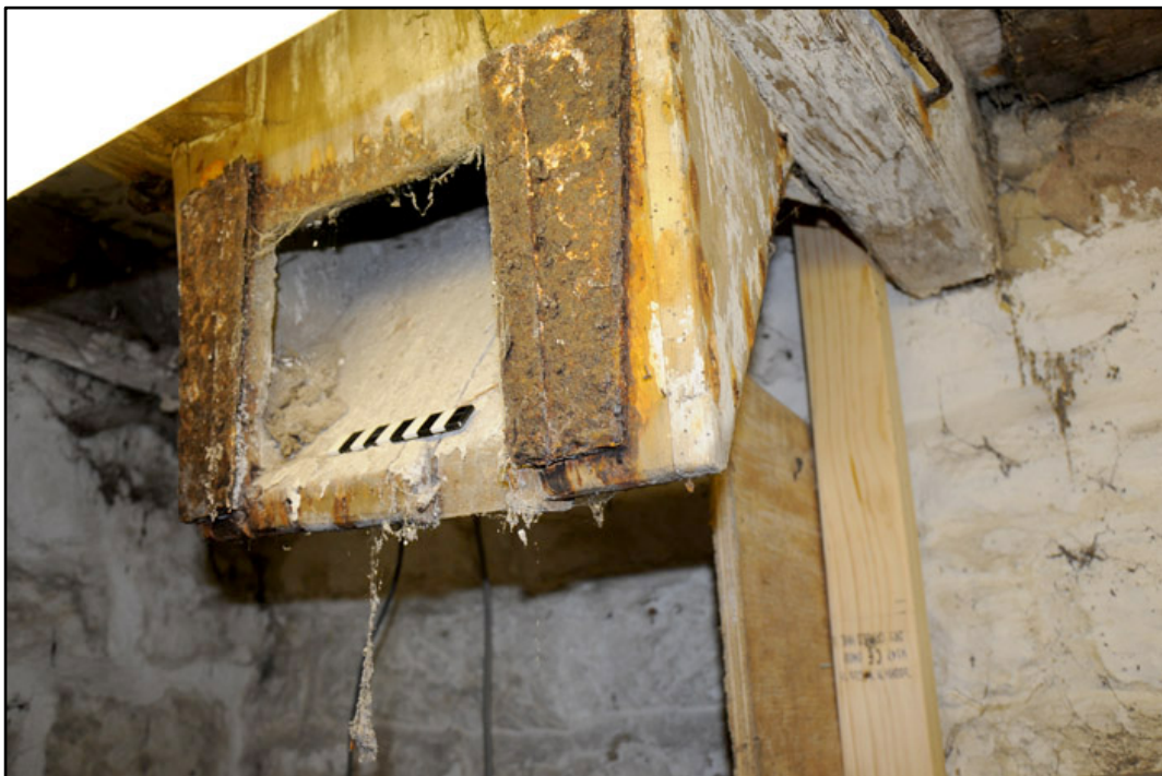
Appendix 3.17: Detail of hopper feed from former grain chute on the ceiling of FI (10cm scale).
