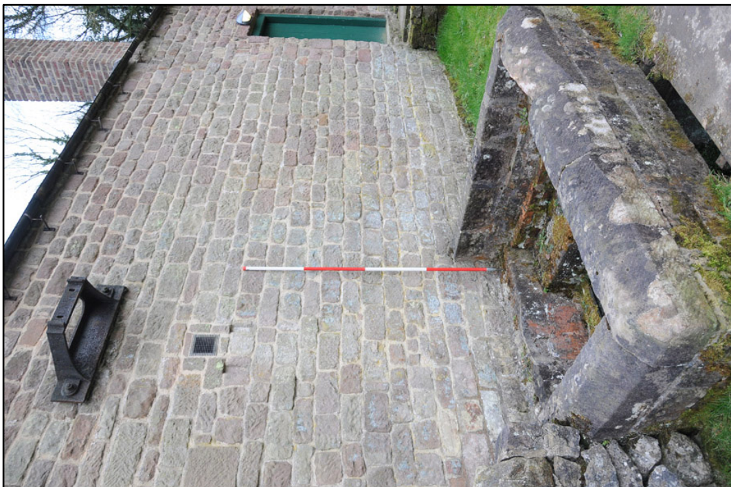
Appendix 3.6: Detail of external vertical driveshaft bracket and location of former power drive on west elevation (2m scale).
