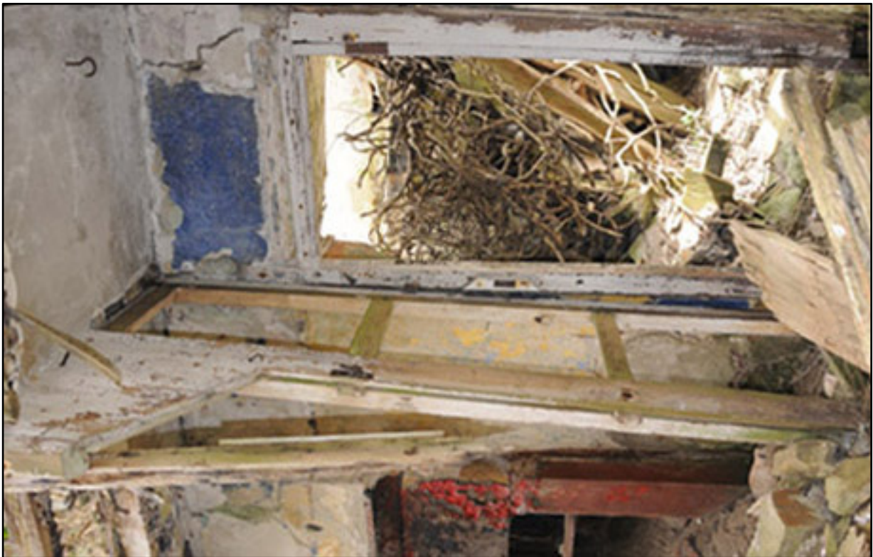
Appendix 3.8: Detail of doorway between G1 and G2 ; note surviving traces of blue.
