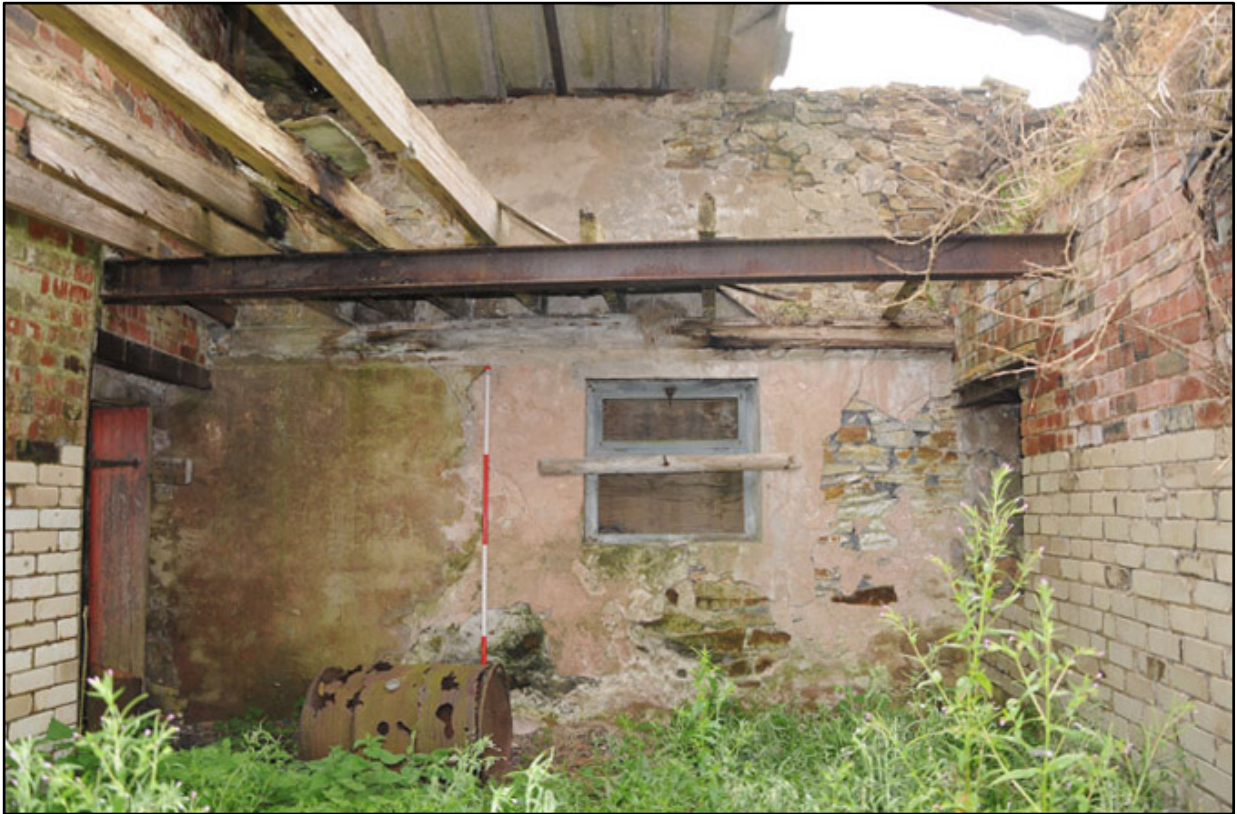
Appendix 3.17: General view looking south of room G5 ; note RSJ and glazed tiles (2m scale).
