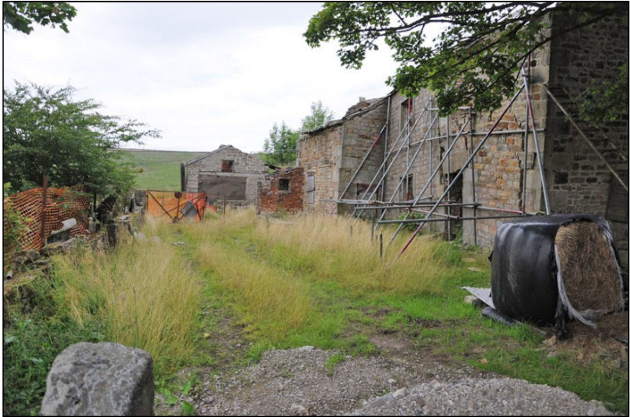
Appendix 3.3: General view looking west into yard along the south side of Smelters Cottage.
