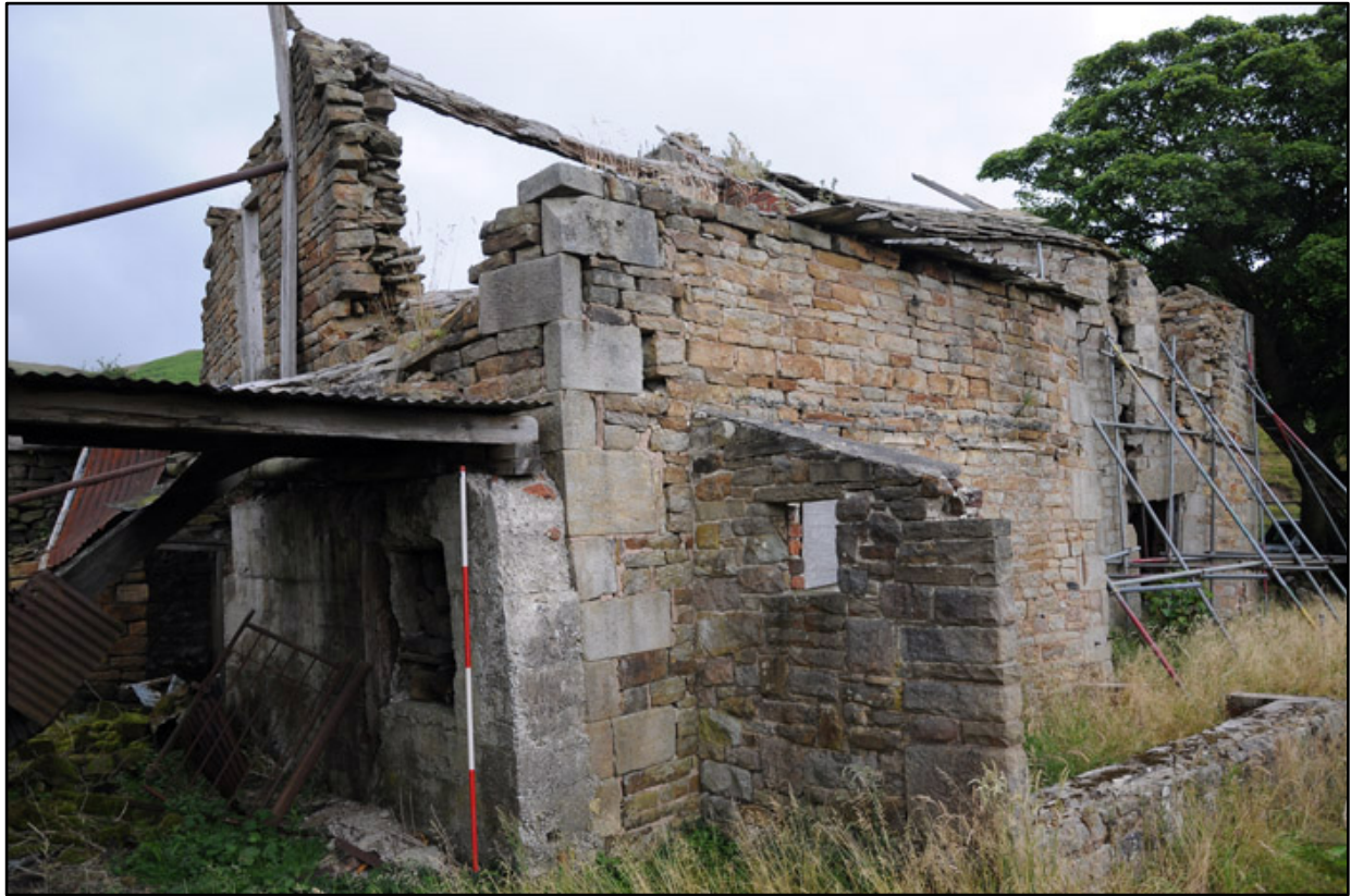
Appendix 3.15: Detail of southwest corner of extension G5 and F5 , and lean-to G6 (2m scale).
