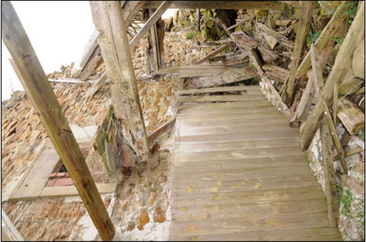
Appendix 3.7: Interior view of room G2 , looking northwest; note matchboard paneling and upper floor fireplace.
