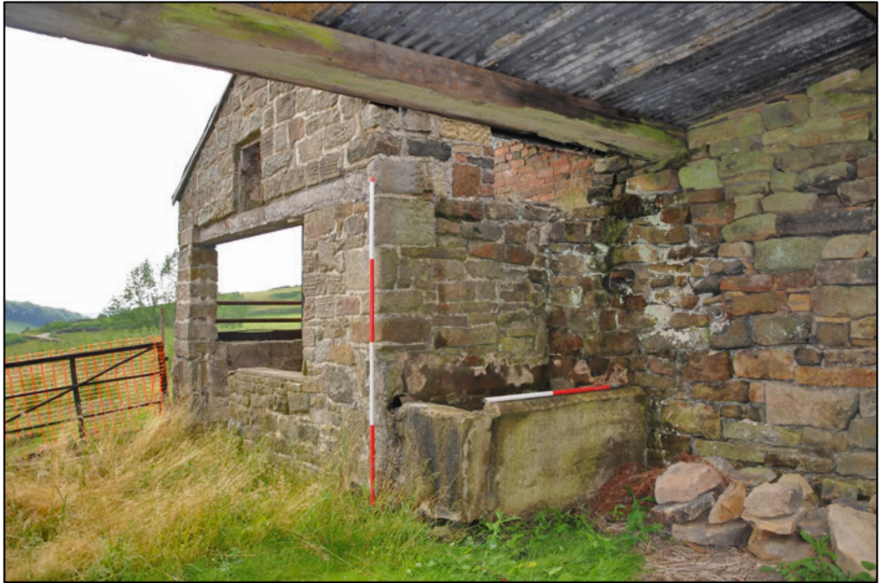
Appendix 3.21: General view of northeast corner of out-building G9 and drinking trough; note secondary roof (2m scale).
