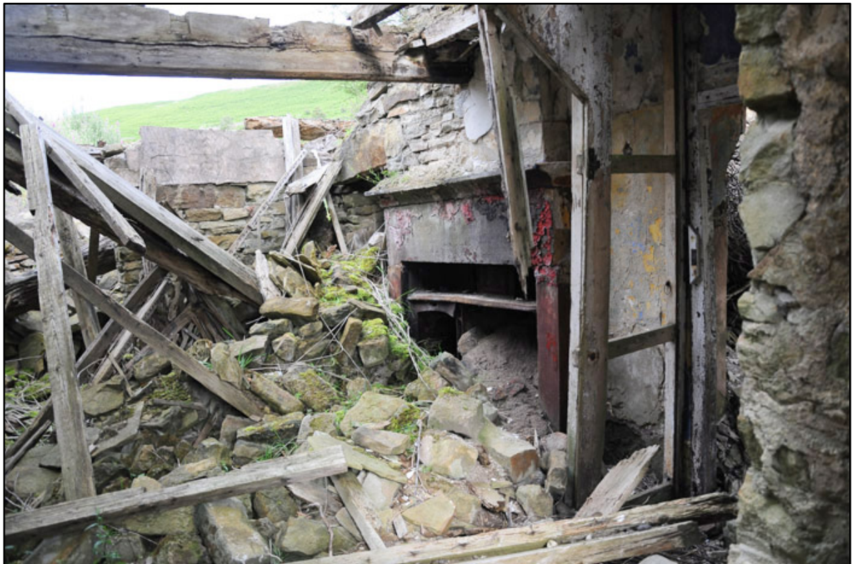
Appendix 3.6: Interior view of room G2, looking northeast; note fireplace and remains of baffle partition to doorway.
