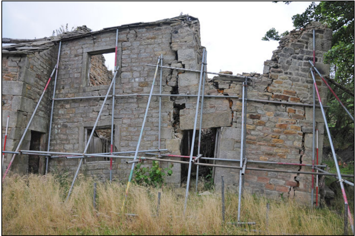
Appendix 3.5: Detail of south elevation; note structural cracking (2m scale).
