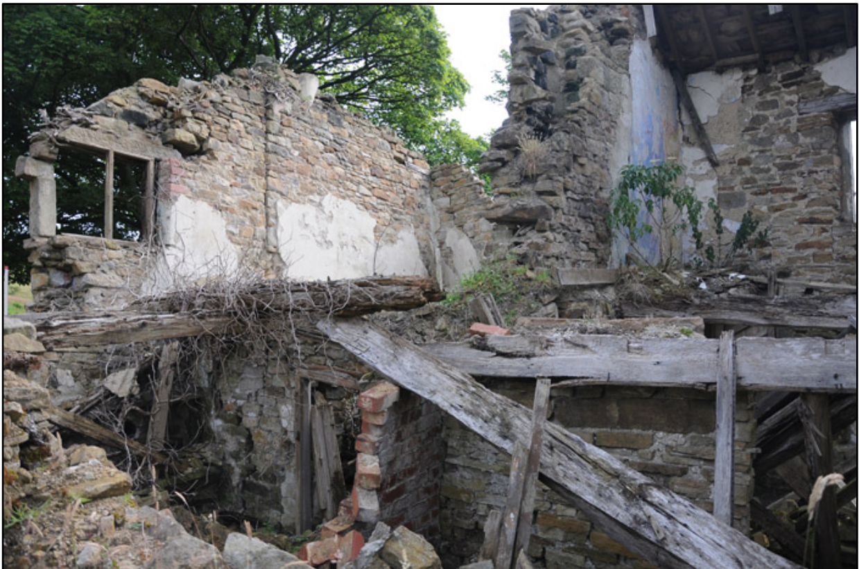
Appendix 3.10: General view looking into the interior of rooms G3, G4 and F3, F4 .
