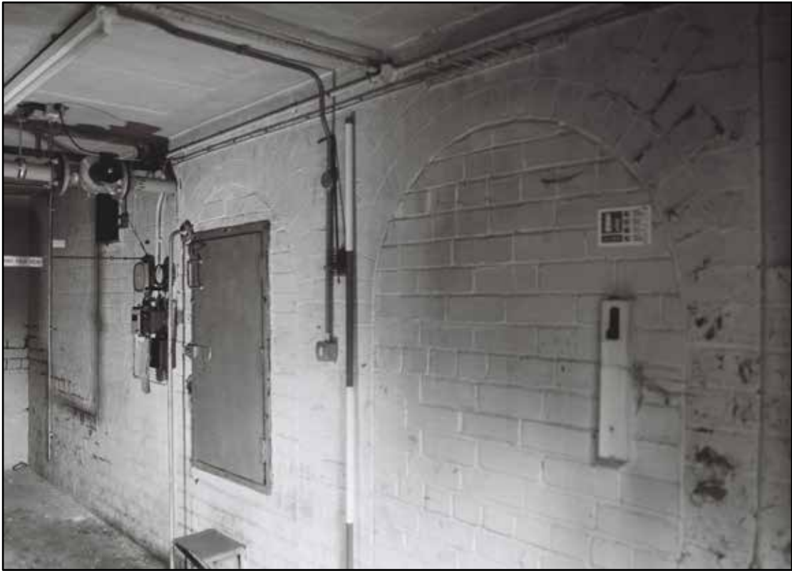
Appendix 5.98: General view of north wall in boiler room B2 with blockings (2m scale) (Film 20.10)
