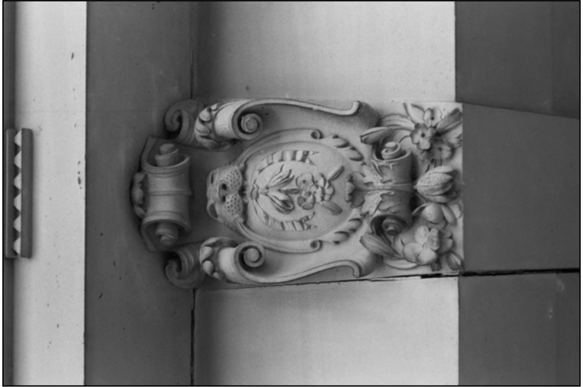
Appendix 5.73: Detail of exterior carving of a seal and wreath on keystone on south elevation (Film 32.16)
