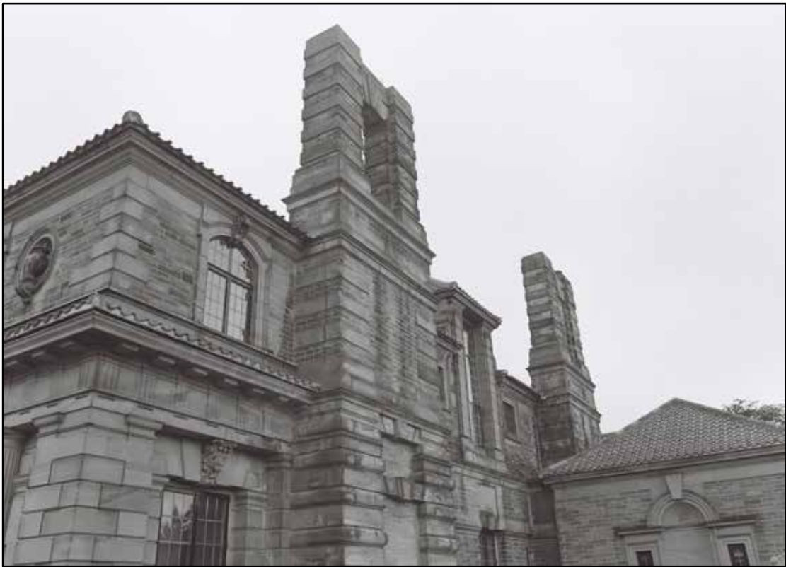
Appendix 5.60: Detail of external chimney stack along east elevation of house (Film 6.15)
