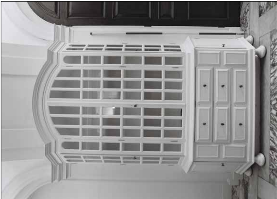
Appendix 5.126: Detail of original display cabinet in G7, looking east (2m scale) (Film 27.15)
