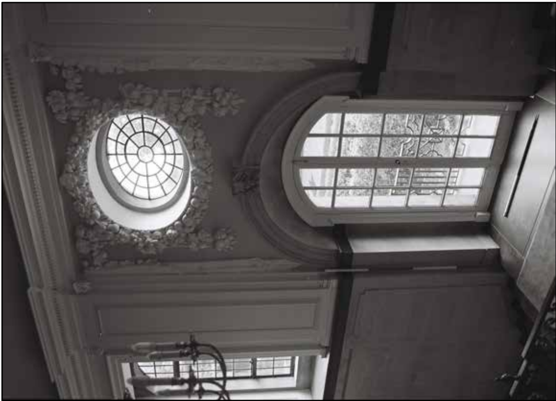
Appendix 5.166: Detail of half landing and balcony on staircase in F2, looking west (1m/2m scale) (Film 18.06)
