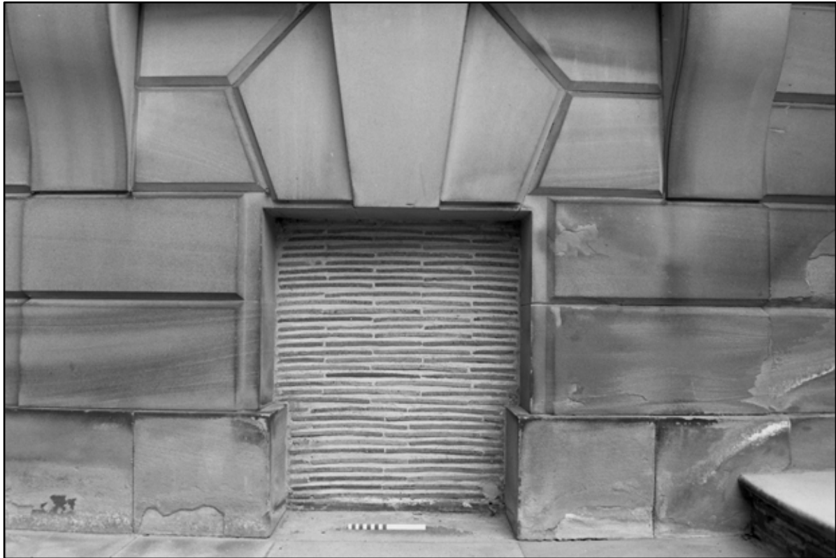
Appendix 5.52: Detail of blocked basement window on north elevation of house (20cm scale) (Film 32.07)
