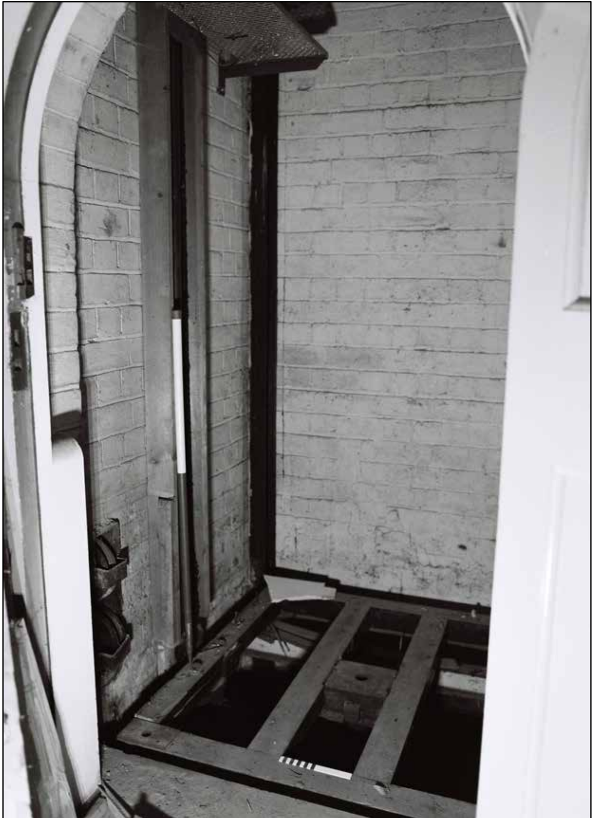
Appendix 5.107: Detail of base of lift shaft in basement (20cm/1m scale) (Film 23.06)
