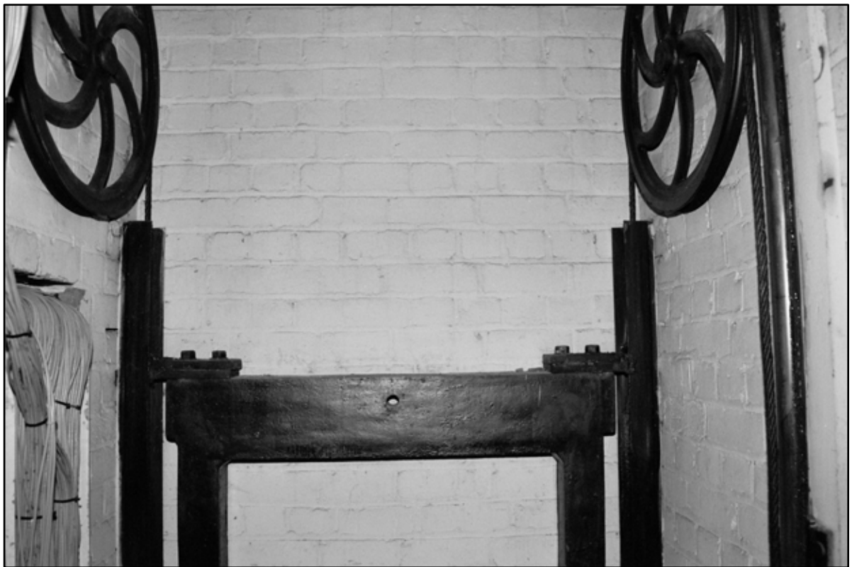
Appendix 5.221: Detail of upper part of lift shaft S2; note wheels and counterweight (Film 33.07)
