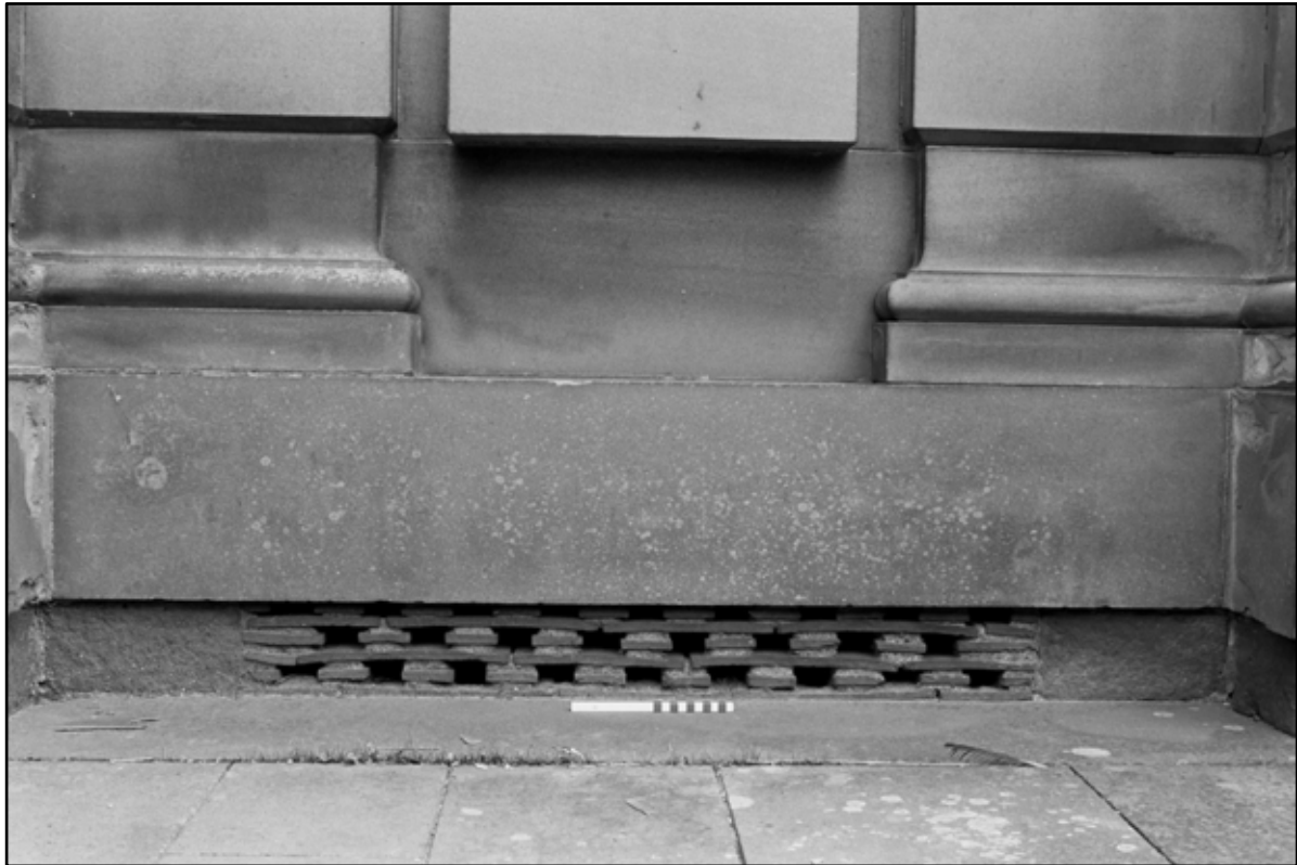
Appendix 5.79: General view across entrance forecourt of north elevation of house (20cm scale) (Film 32.25)
