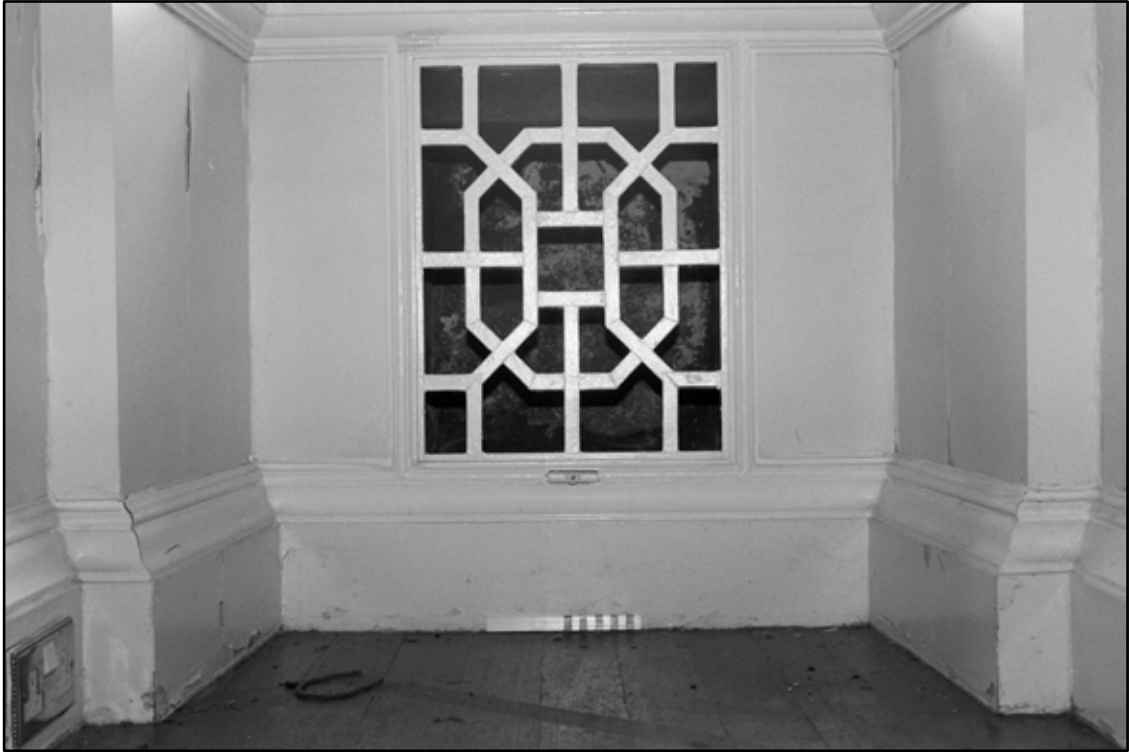
Appendix 5.130: Detail of fretwork heating vent in south wall of G7 (20cm scale) (Film 33.29)
