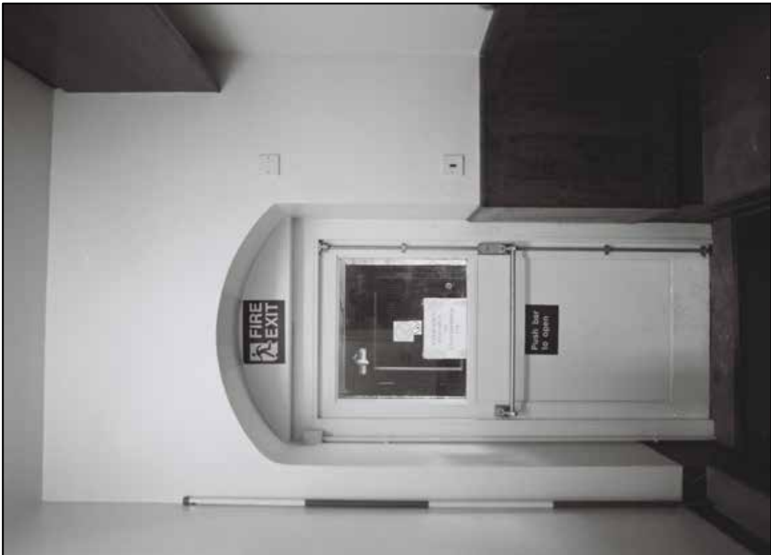
Appendix 5.163: General view of service entrance doorway in G12, looking north (2m scale) (Film 30.12)
