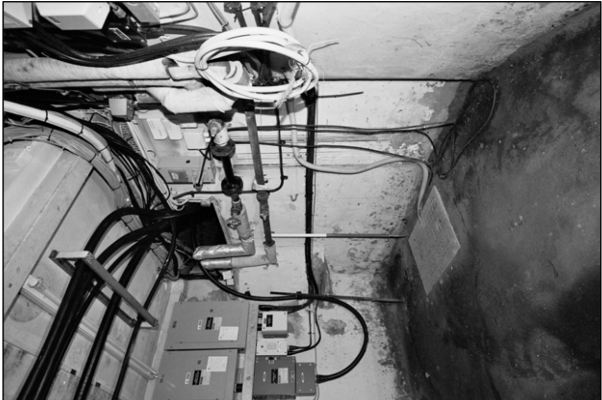
Appendix 5.234: General view of A10, looking southwest; note high level hatch to vaulted tunnel (1m scale) (Film 22.22)
