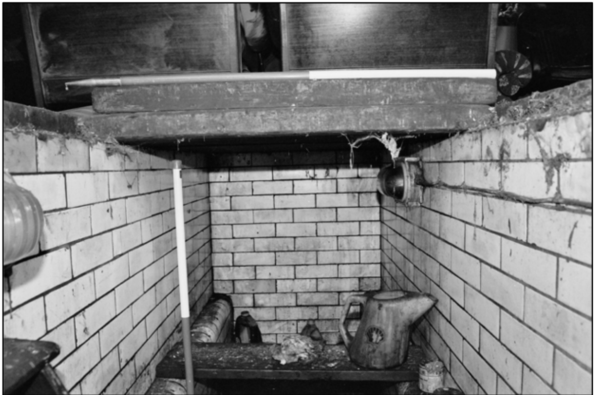
Appendix 5.254: Detail of glazed tiles inside inspection pit GA4, looking north (1m scale) (Film 21.10)
