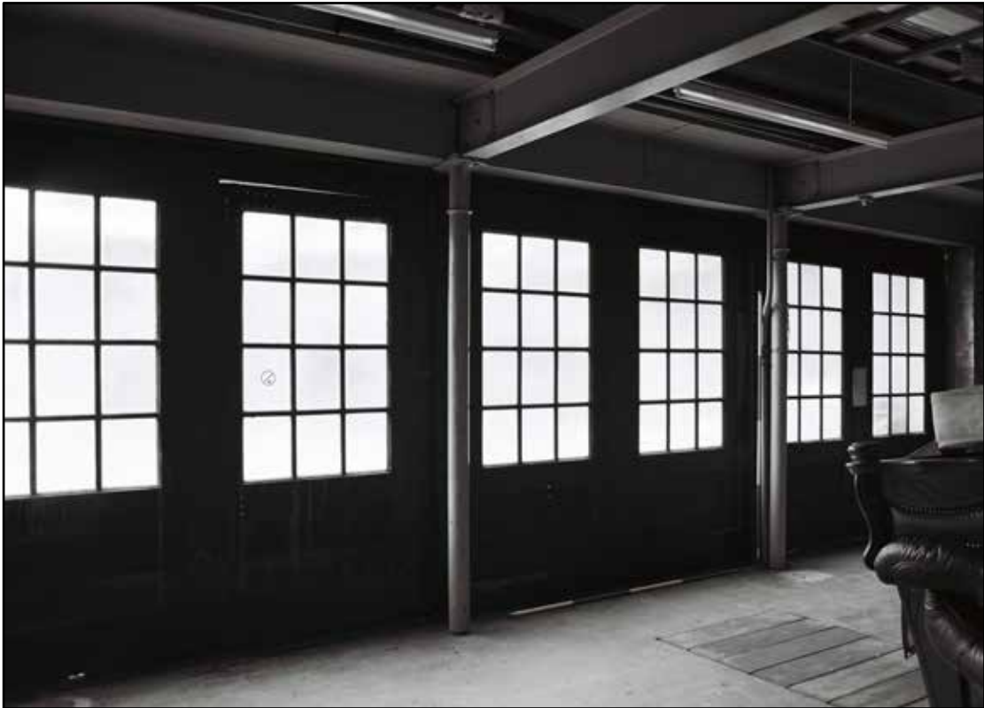
Appendix 5.247: General view of the glazed sliding doors to vehicle garage GA4 in motor house (2m scale) (Film 20.07)
