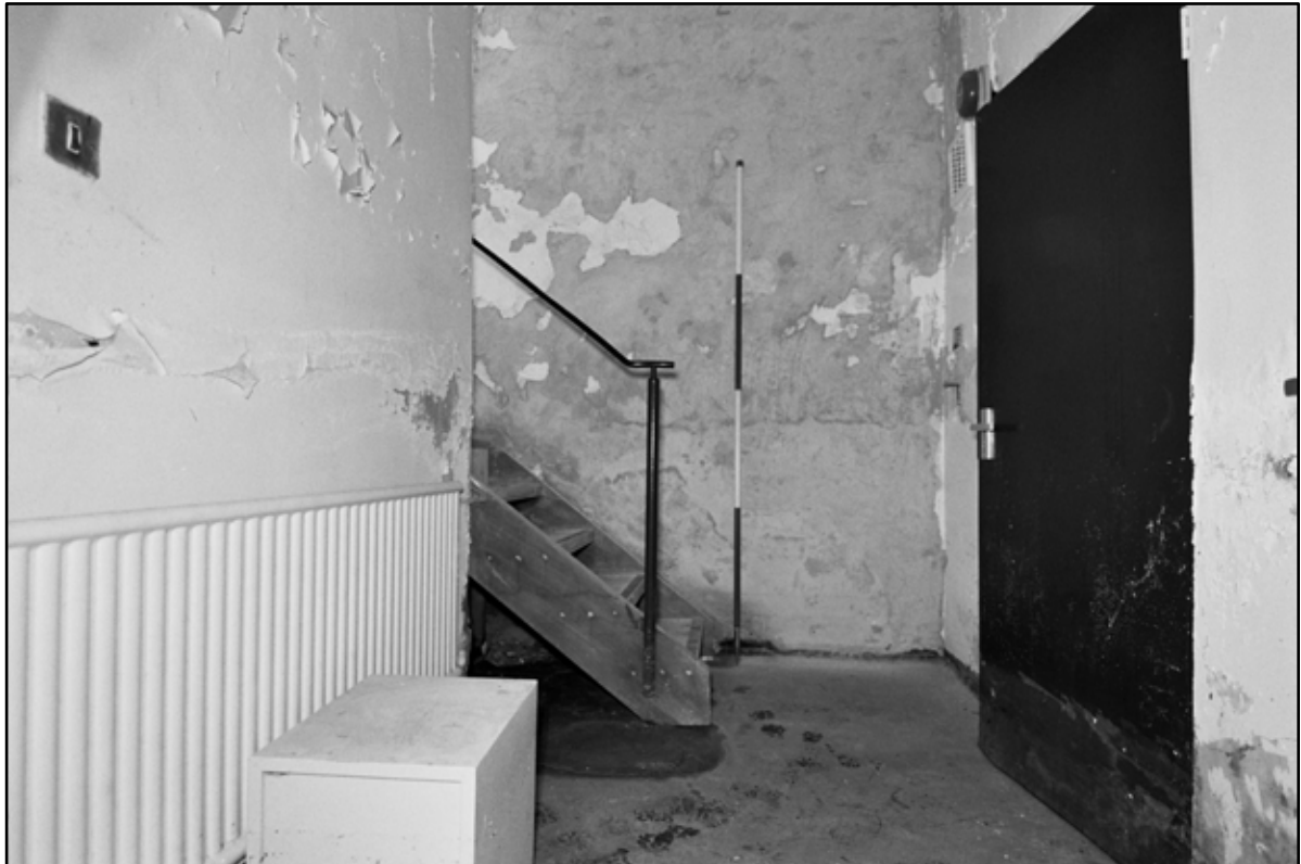
Appendix 5.230: General view looking south of basement stairwell in Annex (2m scale) (Film 22.21)
