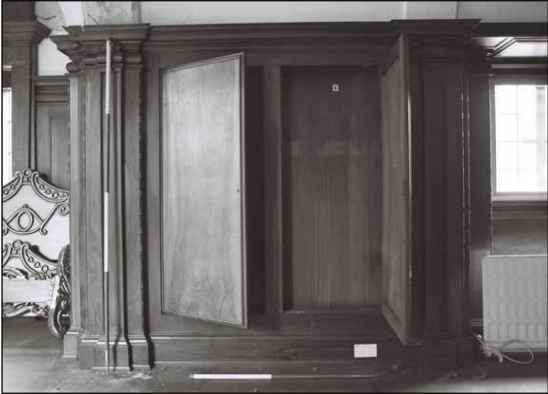
Appendix 5.145: Detail of built-in cupboard for billiard cues in north wall of G1 (1m/2m scale) (Film 25.09)
