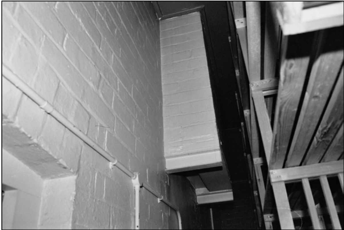
Appendix 5.269: Detail of high level chimney breast in west wall of GA2, looking north (Film 21.25)
