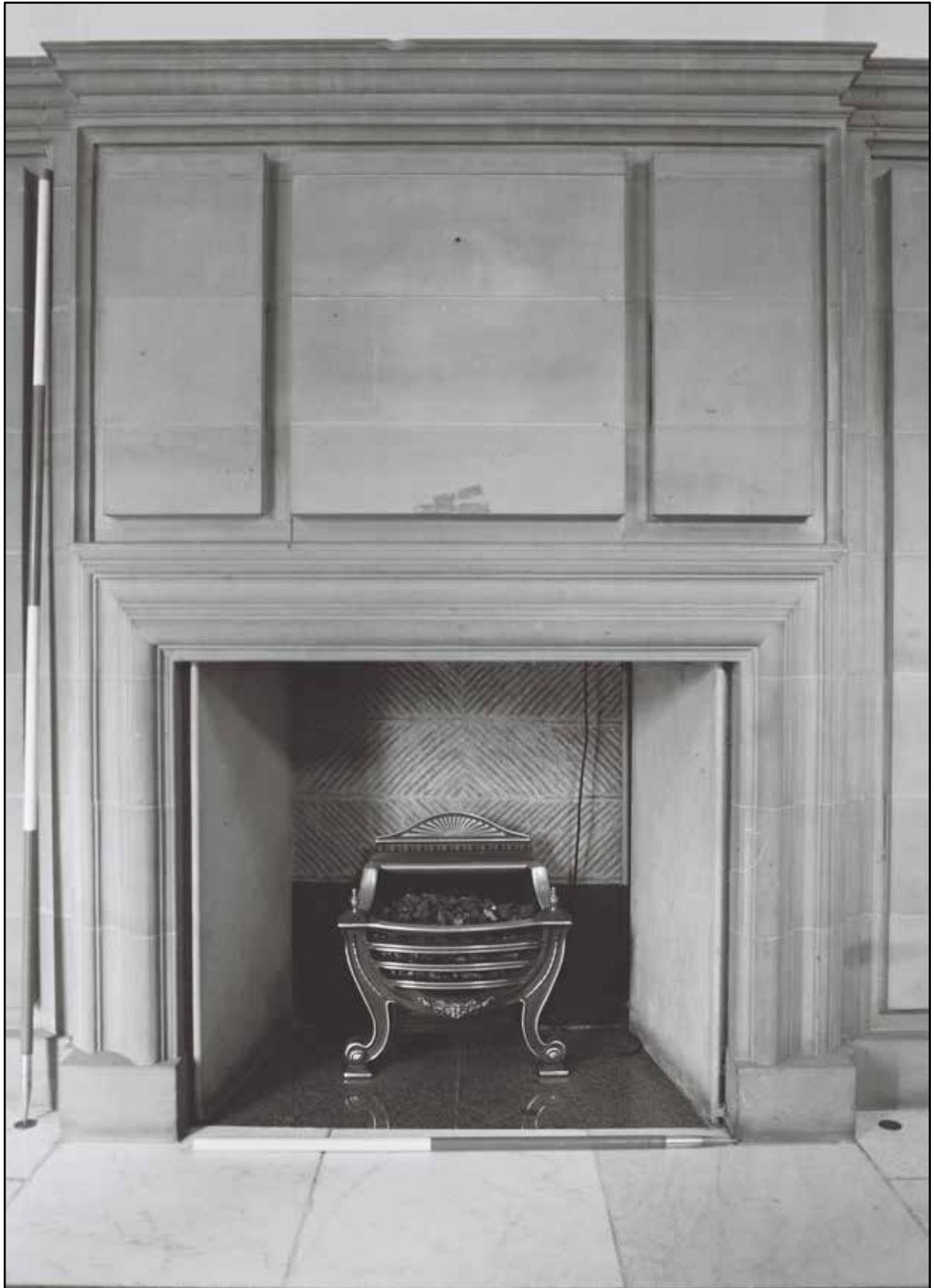
Appendix 5.112: Detail of fireplace in south wall of entrance hall G4 (1m/2m scale) (Film 28.14)
