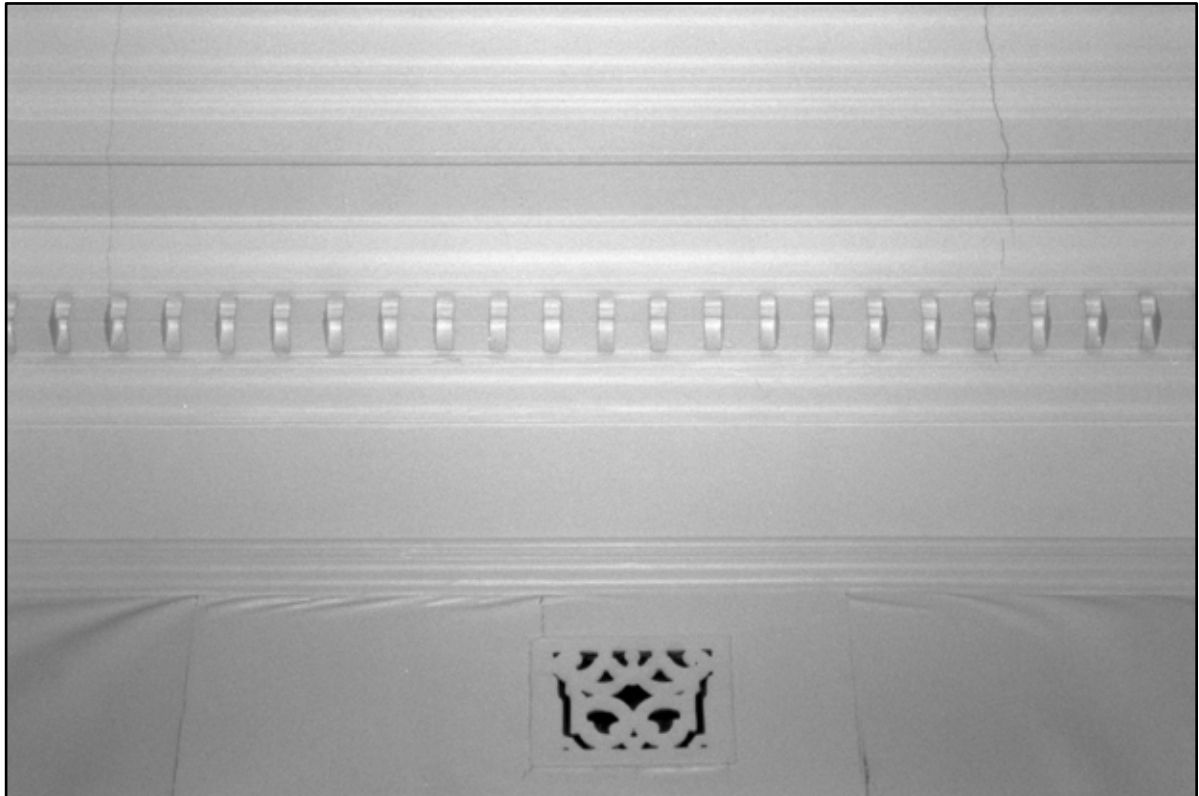
Appendix 5.117: Detail of cornice and metal high level vent in G8 (Film 33.31)
