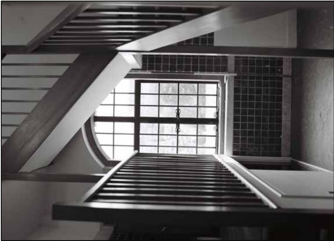
Appendix 5.195: General view of former bathroom F8; note inserted stairwell (2m scale) (Film 13.06)
