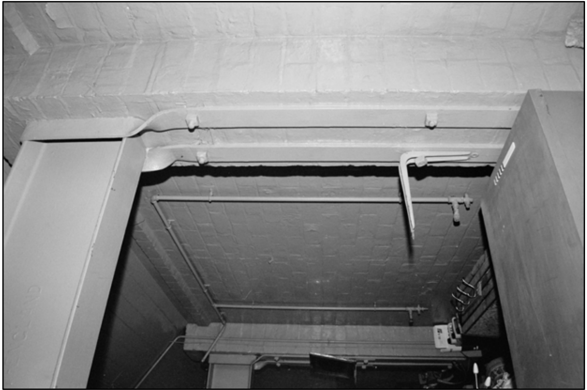
Appendix 5.249: Detail of metal conduit and shelving bracket on north wall of motor house (20cm scale) (Film 21.03)
