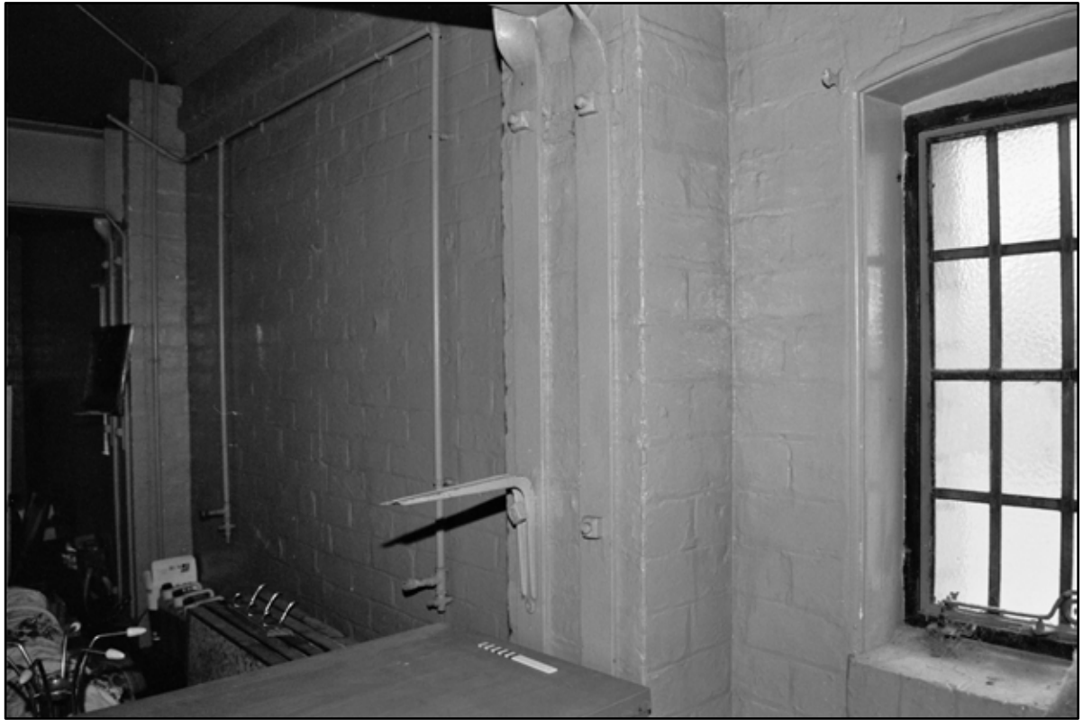
Appendix 5.251: Detail of metal conduit on north wall of motor house (20cm scale) (Film 21.02)
