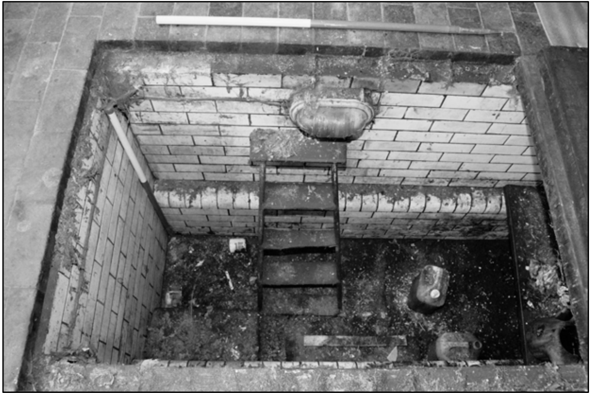
Appendix 5.255: Detail from above of inspection pit in GA4 (1m scale) (Film 21.12)
