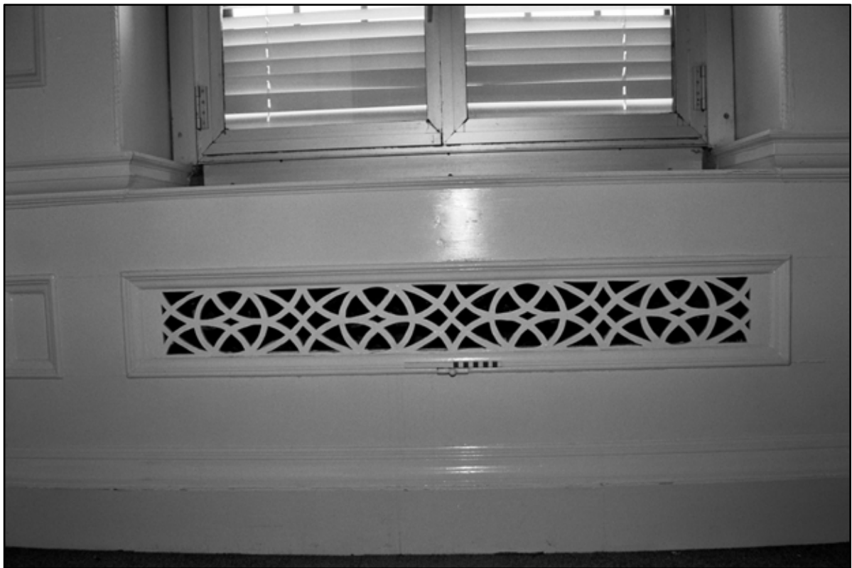
Appendix 5.118: Detail of fretwork heating vent in east wall of G8 (20cm scale) (Film 33.32)
