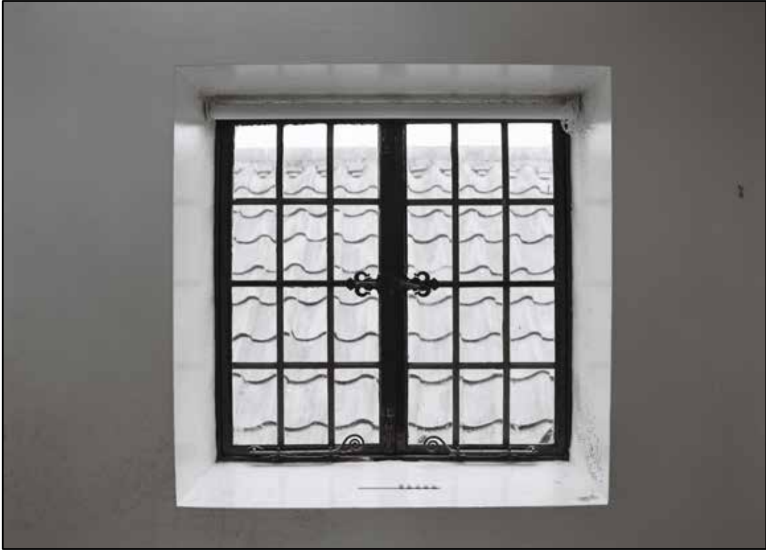
Appendix 5.208: Detail of metal framed window in S8, looking east (20cm scale) (Film 11.15)
