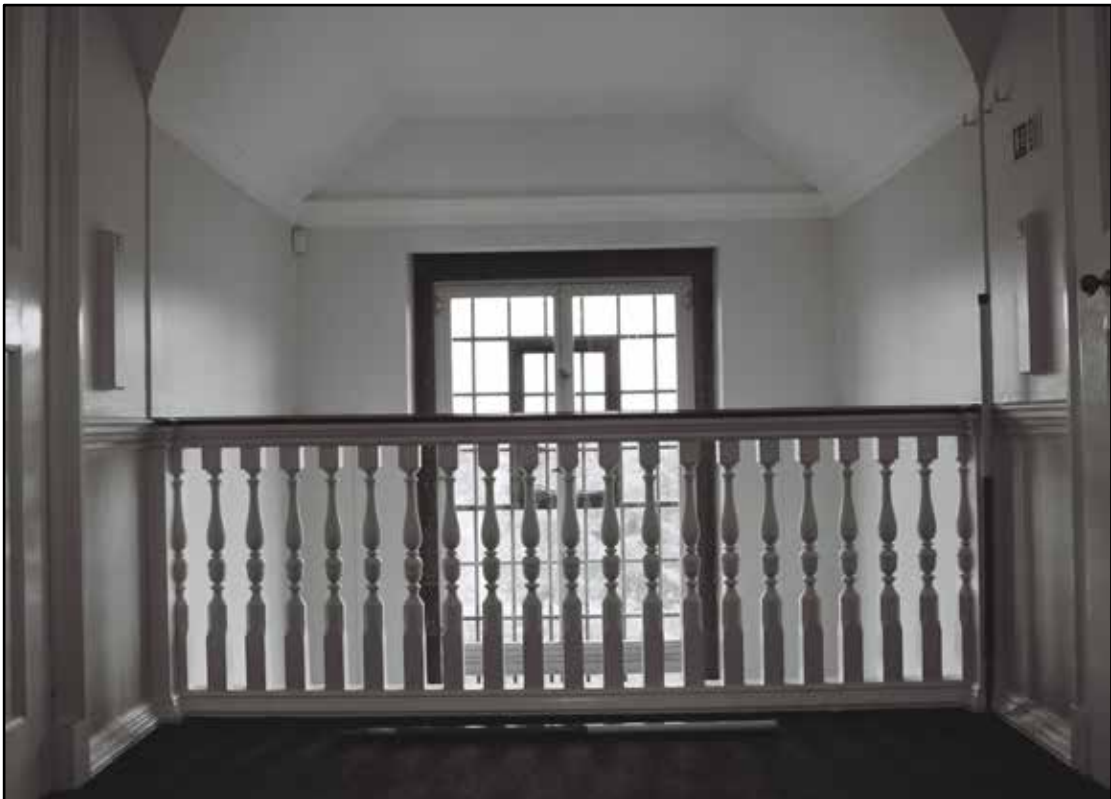
Appendix 5.205: General view of balcony on second floor landing S1, looking east (1m scale) (Film 11.11)
