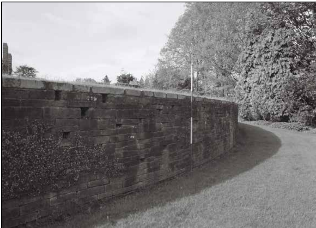
Appendix 5.31: Curved retaining wall forming lower edge to south lawn; note holes for planting (2m scale) (Film 2.09)
