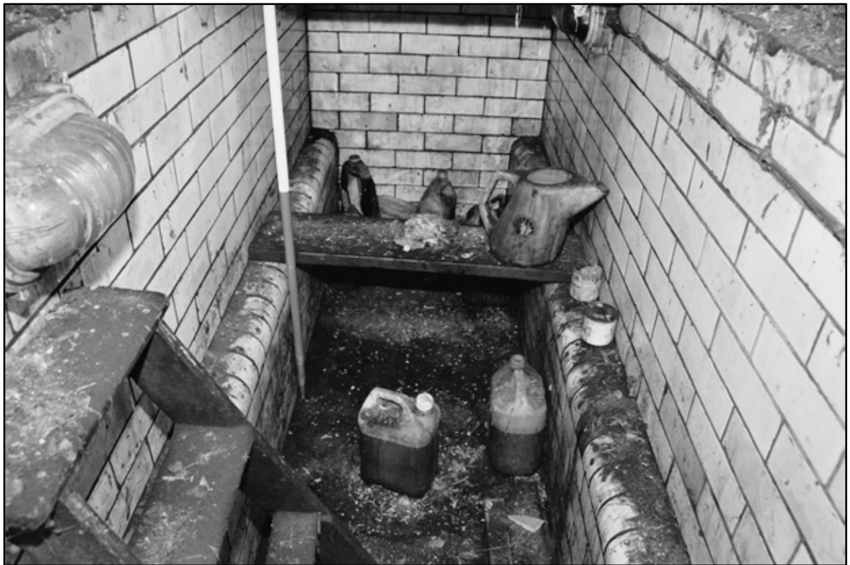
Appendix 5.256: General view of interior of inspection pit in GA4, looking north (1m scale) (Film 22.11)
