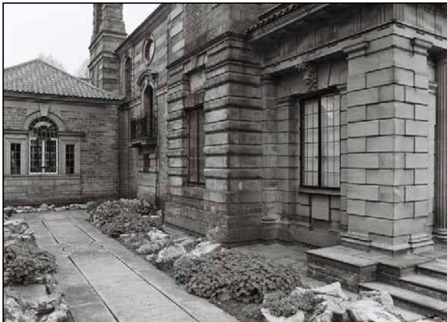
Appendix 6.8: Comparative view of exterior of the House on 25 th May 2015 (Film 8.09).
