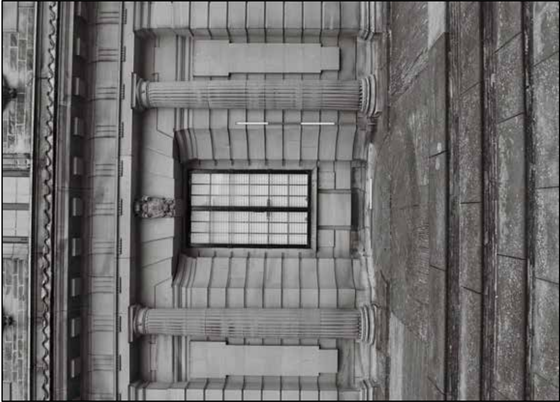
Appendix 5.67: Detail of the ground floor of the south elevation of house (1m/2m scale) (Film 7.07)
