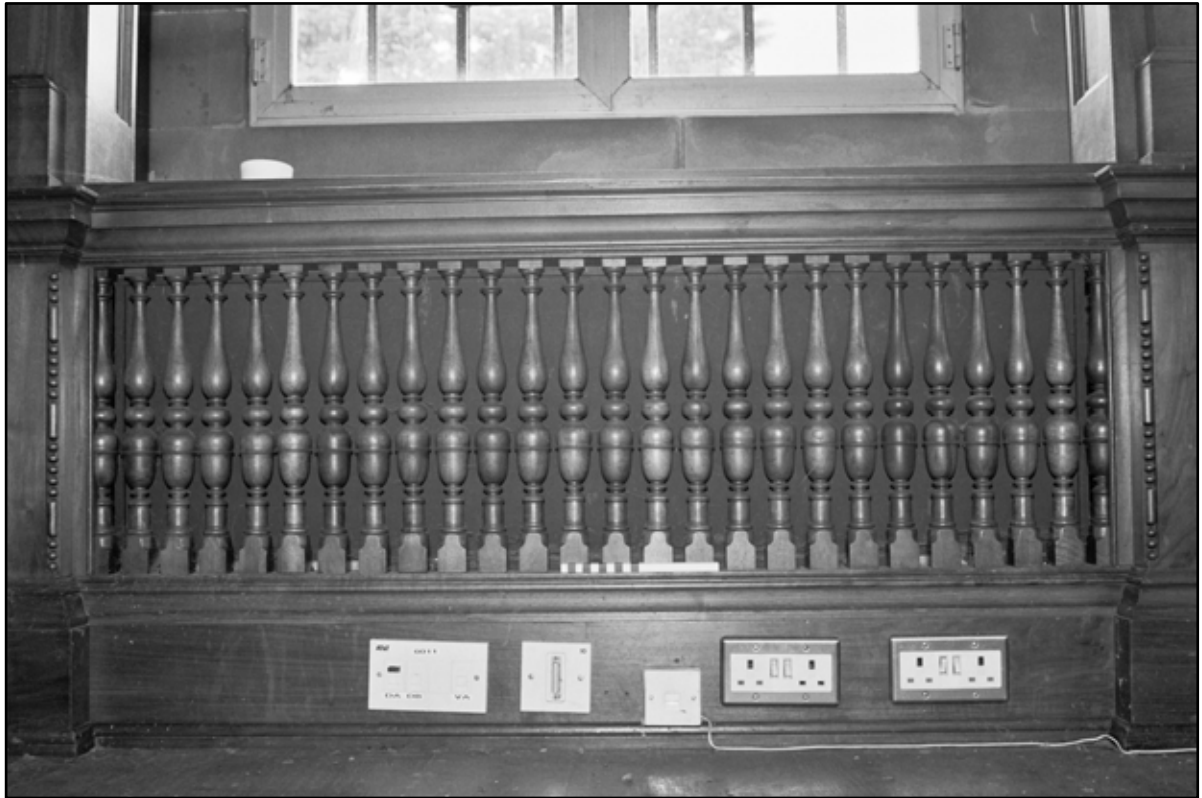
Appendix 5.148: Detail of ventilation grill in west wall of GI (20cm scale) (Film 33.24)
