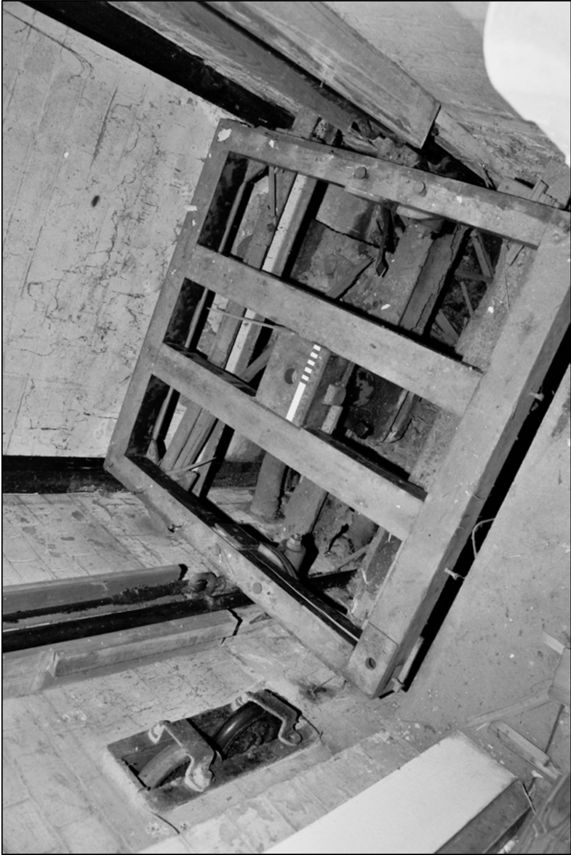
Appendix 5.108: Detail of remains of lift car in basement (20cm scale) (Film 33.34)
