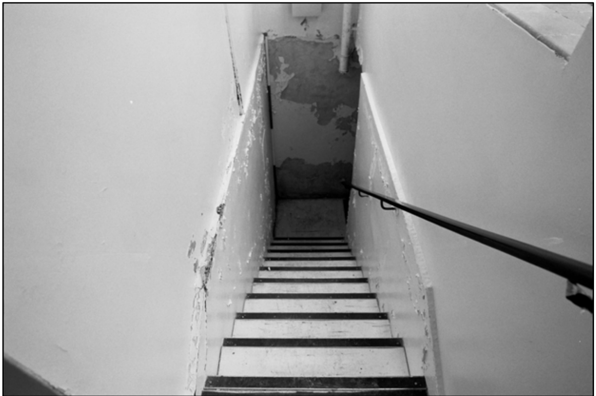
Appendix 5.229: General view looking down stairwell A1 to basement of Annex (Film 22.09)
