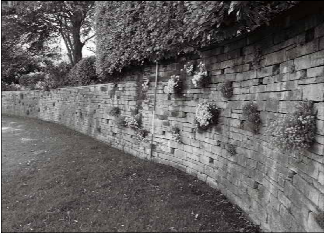
Appendix 5.30: Curved retaining wall northwest garden; note holes for planting (2m scale) (Film 1.13)
