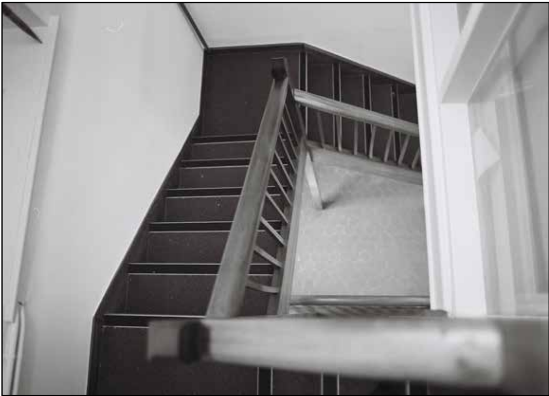
Appendix 5.214: View looking down inserted stairwell in S6 (2m scale) (Film I3.05)
