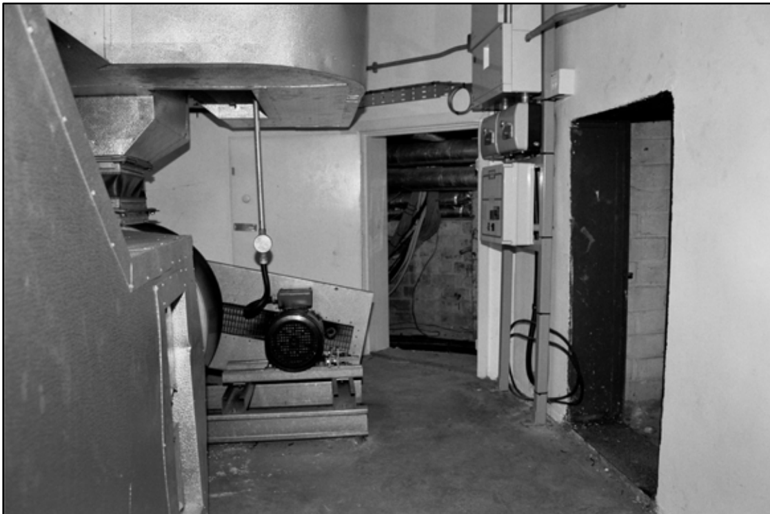
Appendix 5.91: Interior of former plenum chamber in basement; note modern ducts (Film 22.31)
