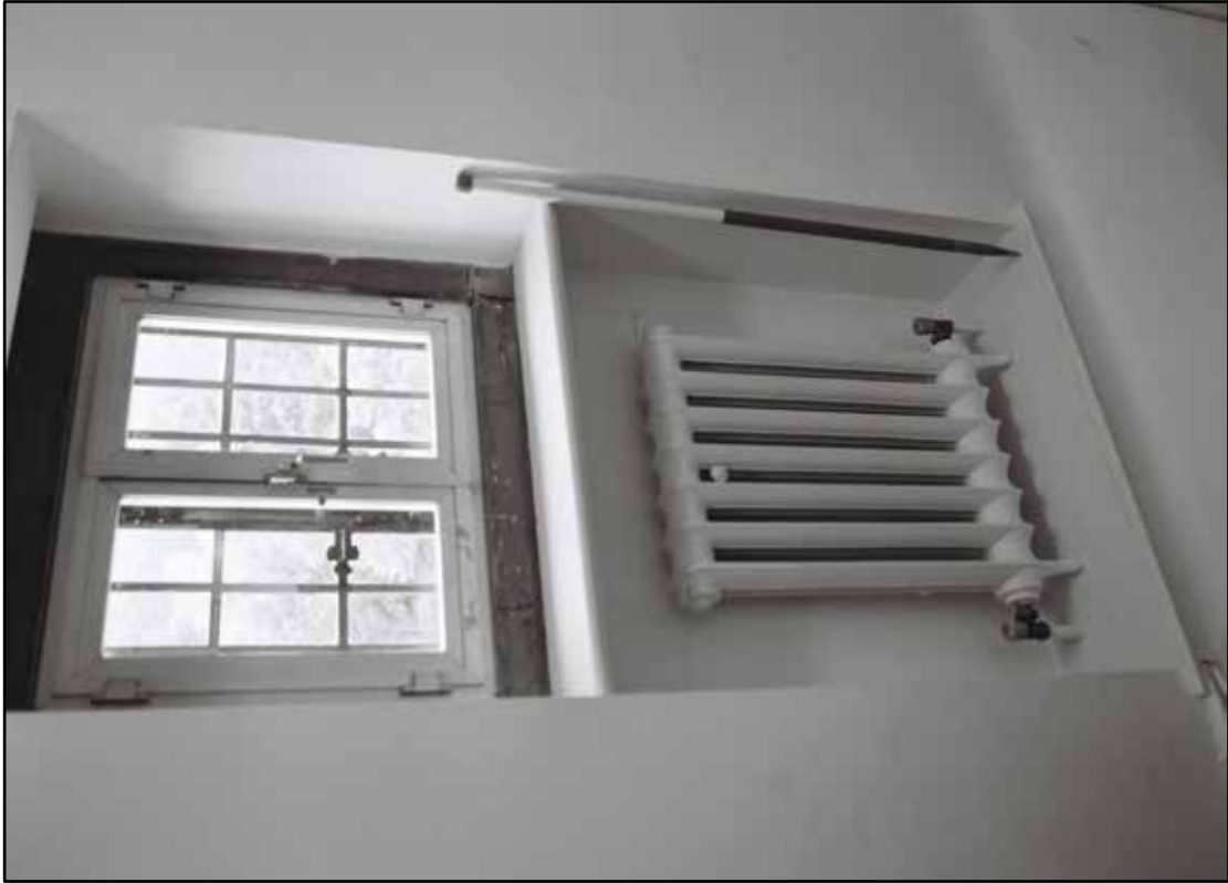
Appendix 5.213: Detail of radiator in the inserted stairwell S6 (1m scale) (Film I3.03)
