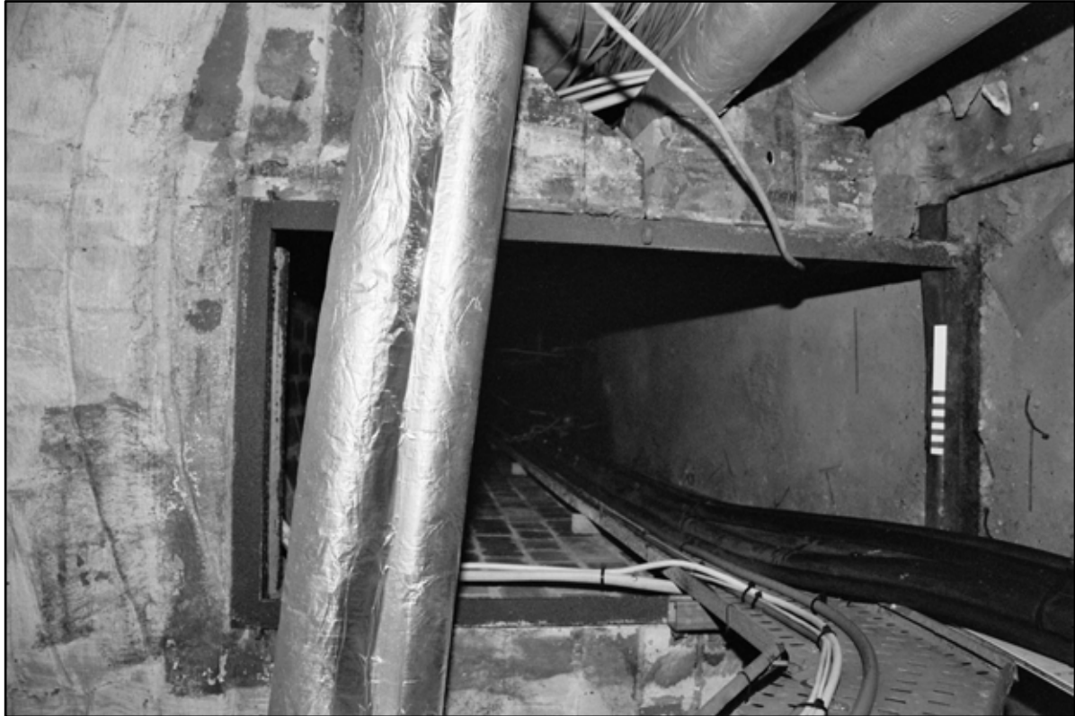
Appendix 5.92: General view of entrance to ducting tunnels in basement (20cm scale) (Film 22.33)
