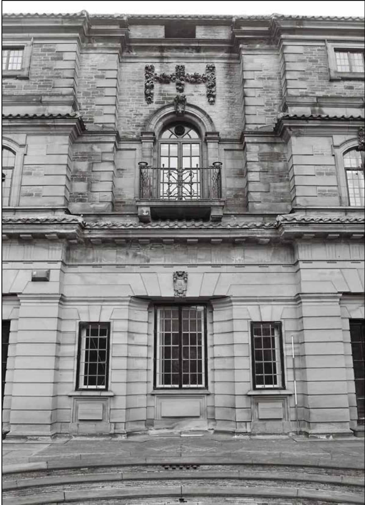
Appendix 5.69: Detail of central bay of south façade of house (1m/2m scale) (Film 7.11)
