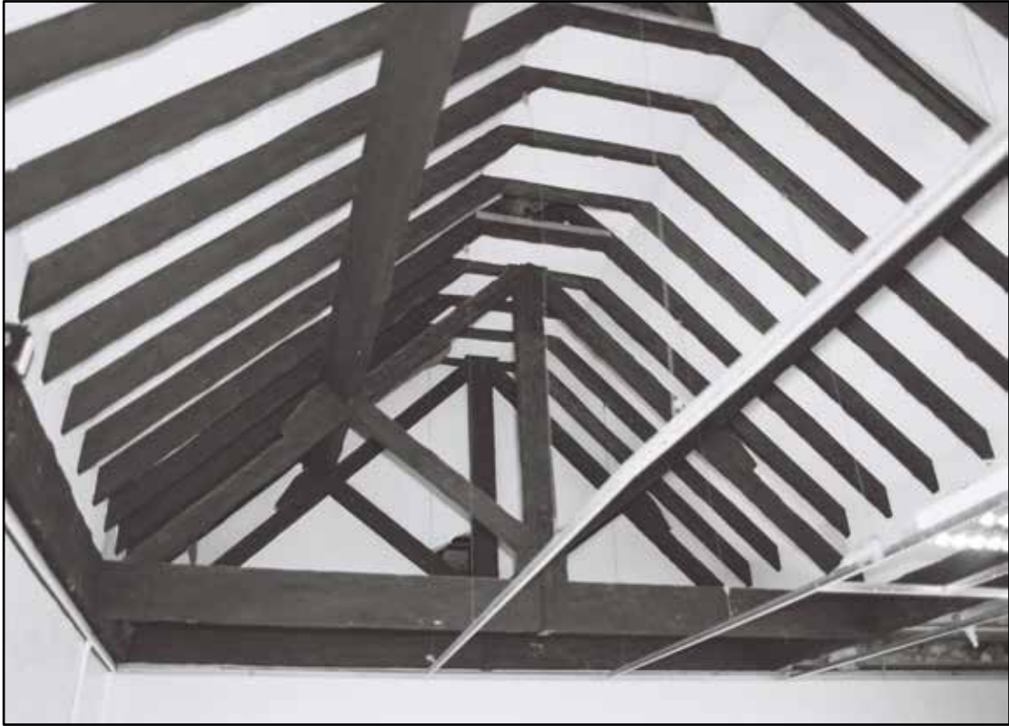
Appendix 5.215: General view of exposed roof timbers in S5; note black staining (Film 12.07)
