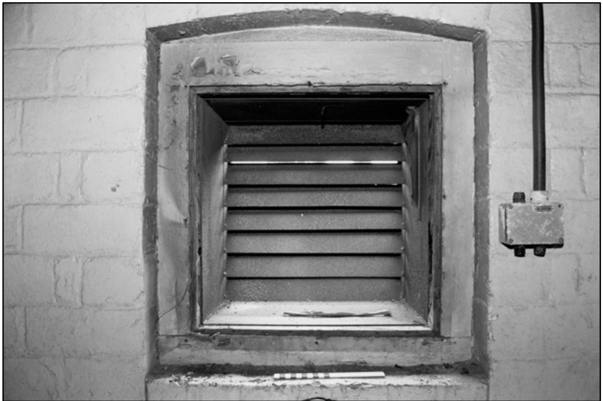
Appendix 5.241: Detail of interior of high level window in GAI of motor house (20cm scale) (Film 21.32)
