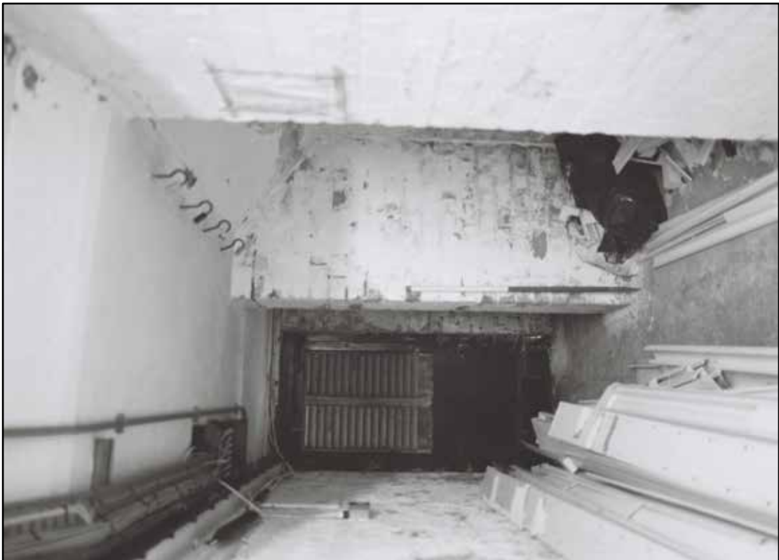
Appendix 5.97: General view of corridor B6; note hooks in ceiling (1m scale) (Film 24.10)
