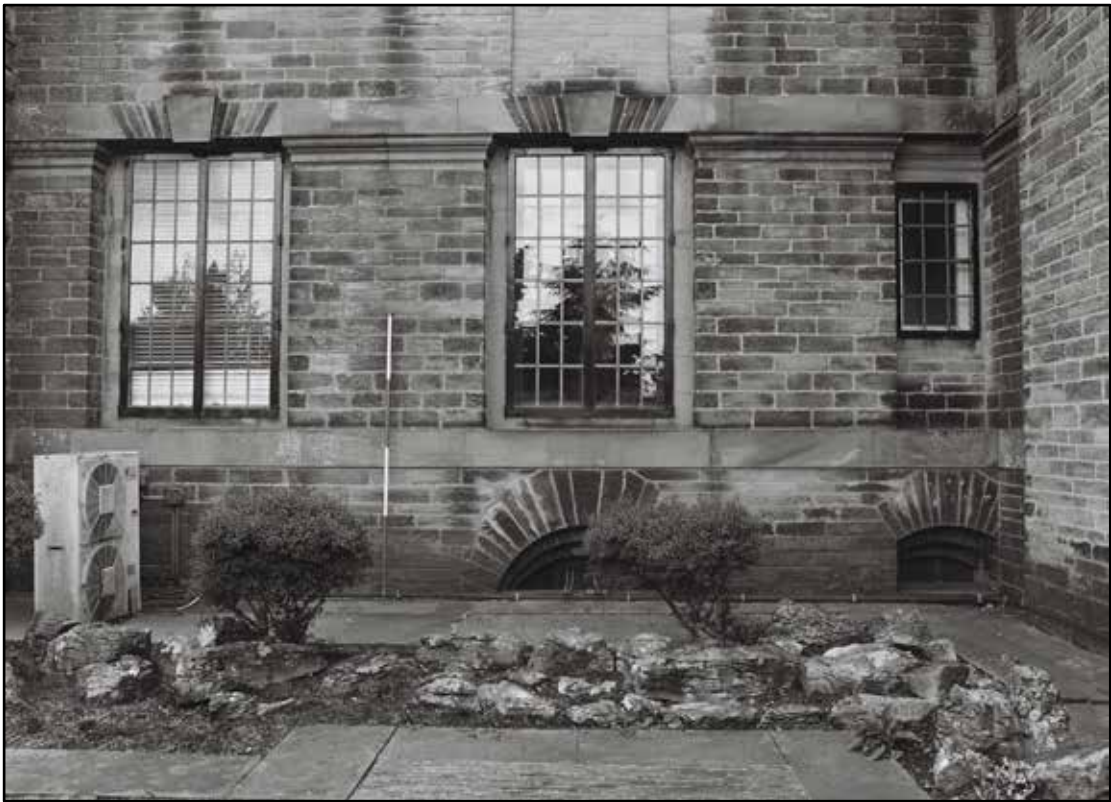
Appendix 5.63: General view of east wall of house; note basement windows (2m scale) (Film 6.09)
