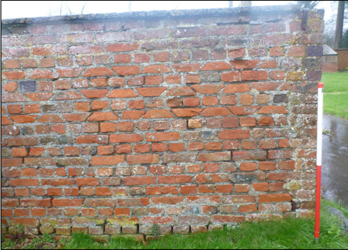
Appendix 3.17: Detail of decorative wall surrounding walled garden, looking north F17 (1m scale).
