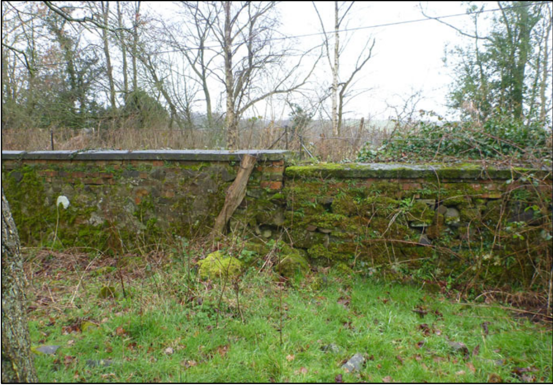
Appendix 3.29: Detail of vertical joint in estate boundary wall F4 , looking south.
