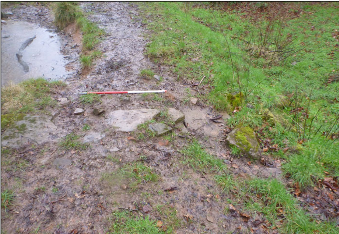
Appendix 3.26: Detail of sluice culvert through the western embankment of pond F3 , looking south (1m scale).
