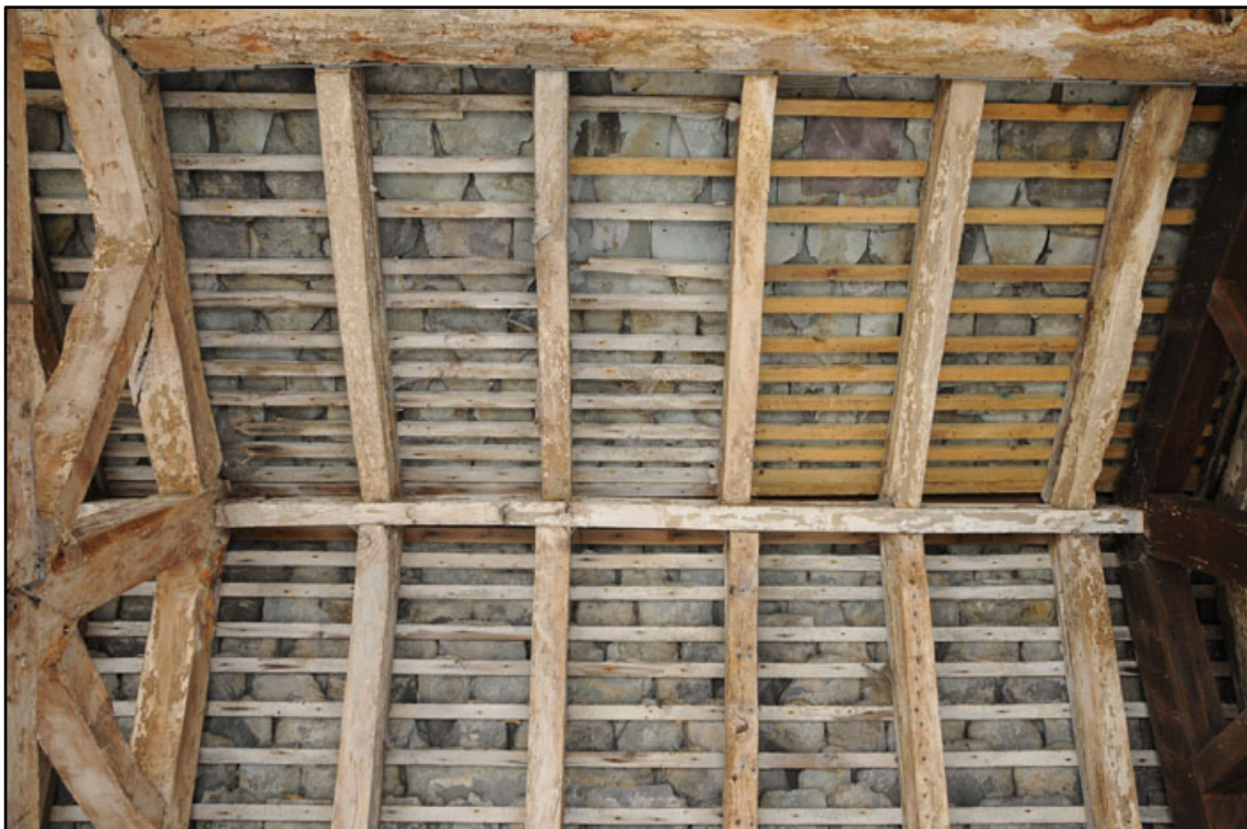
Appendix 2.57: General view of roof construction between T6 and T7 in G3; note painted timbers.
