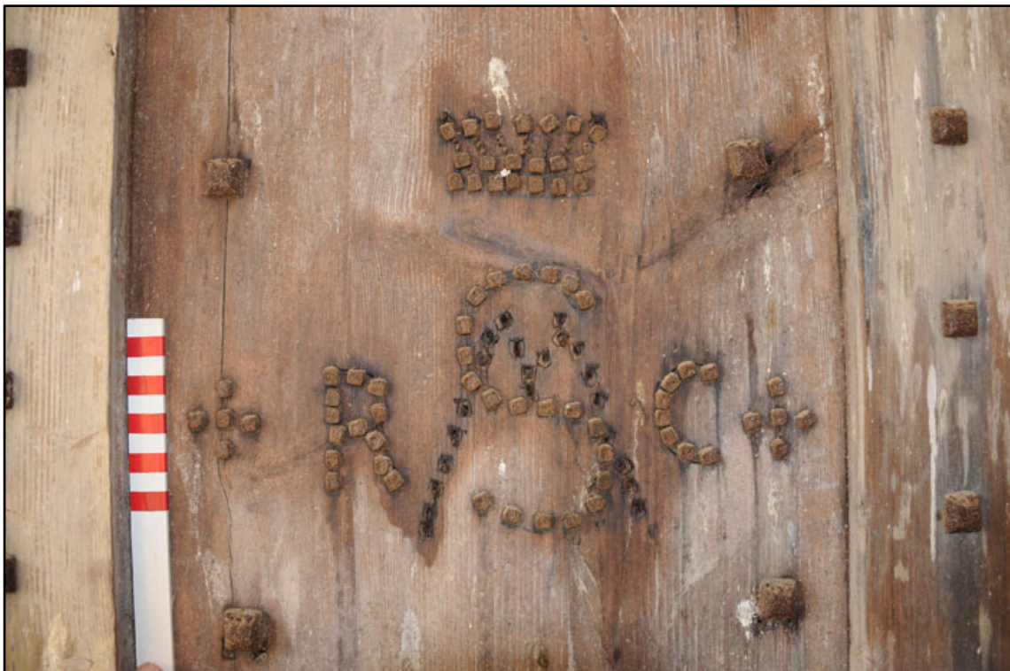
Appendix 2.69: Detail of stud decoration on door D4 in G3 ; note alteration in design (10cm scale).
