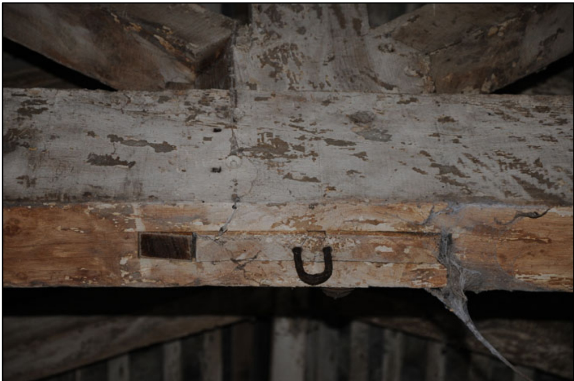
Appendix 2.61: Detail of metal staple and truss construction on underside of T7 in G3.
