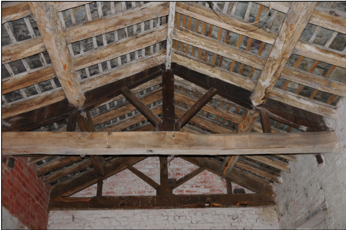
Appendix 2.52: Detail of roof construction at west end of G3 ; note junction of painted and unpainted roof timbers.
