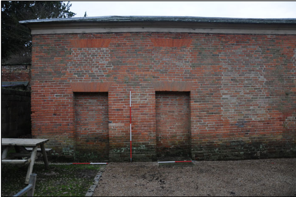
Appendix 2.11: Detail of blocked doorways D6 and D7 on north elevation; note bricked up openings (2m scale).
