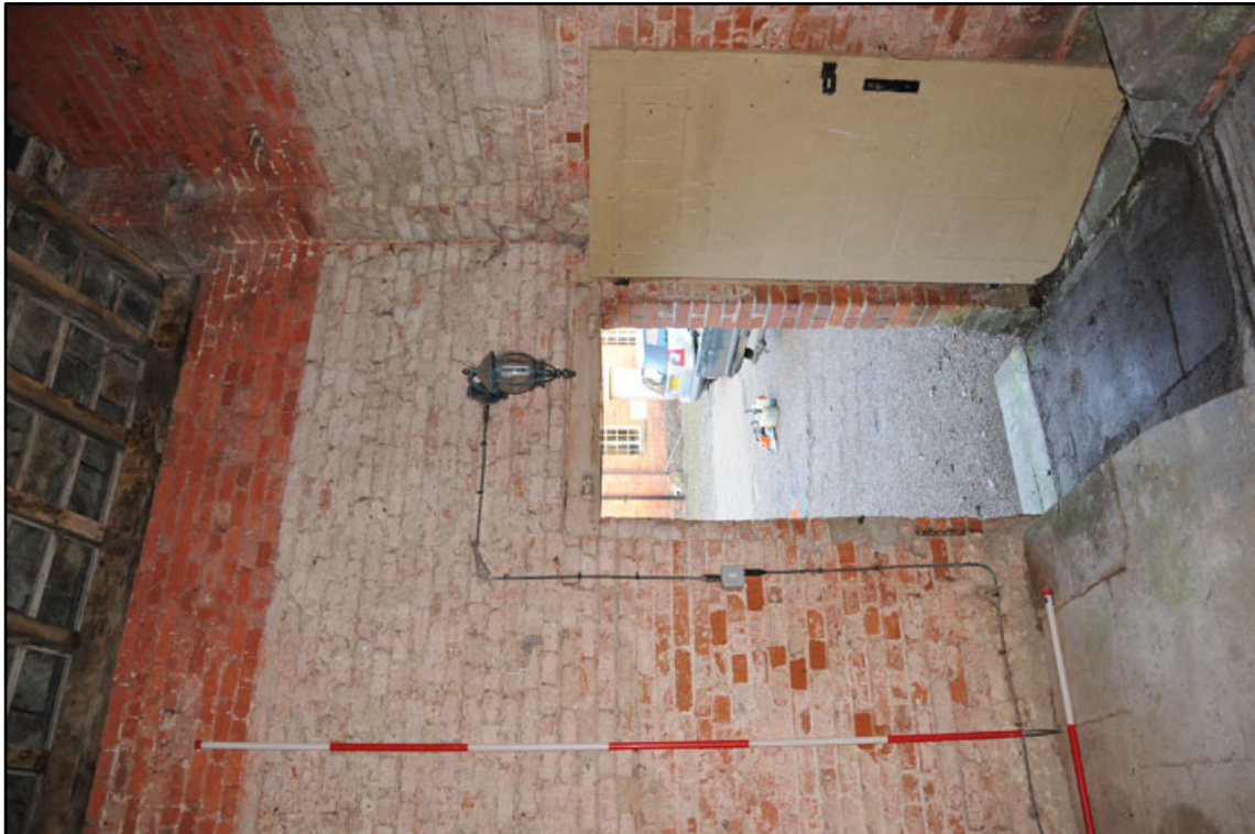
Appendix 2.35: General view of northeast corner of G2 and inserted doorway to Brewhouse Yard (1m/2m scale)
