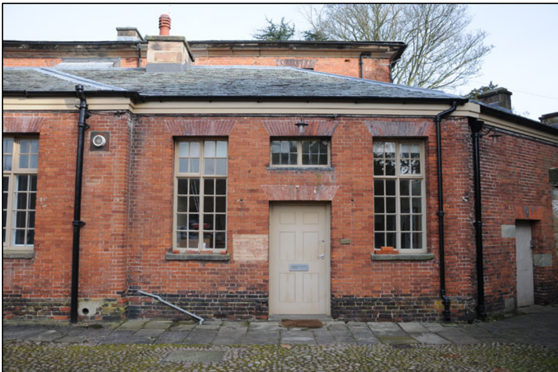
Appendix 2.12: General view of doorway and high level window on laundry on opposite side of Brewhouse Yard.
