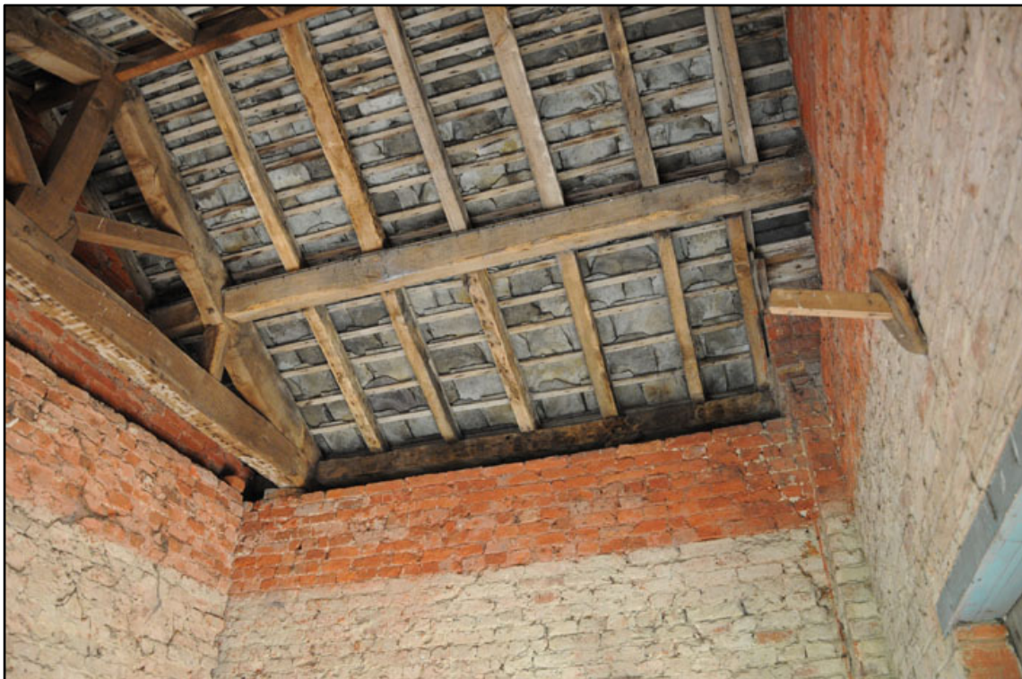
Appendix 2.42: Detail of roof structure in G2, looking north; note surviving exposed section of wall-plate.
