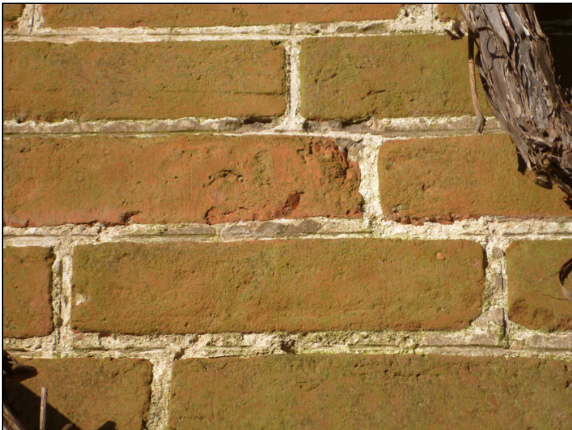
Appendix 2.16: Detail of wheel struck pointing in lime mortar on south façade.
