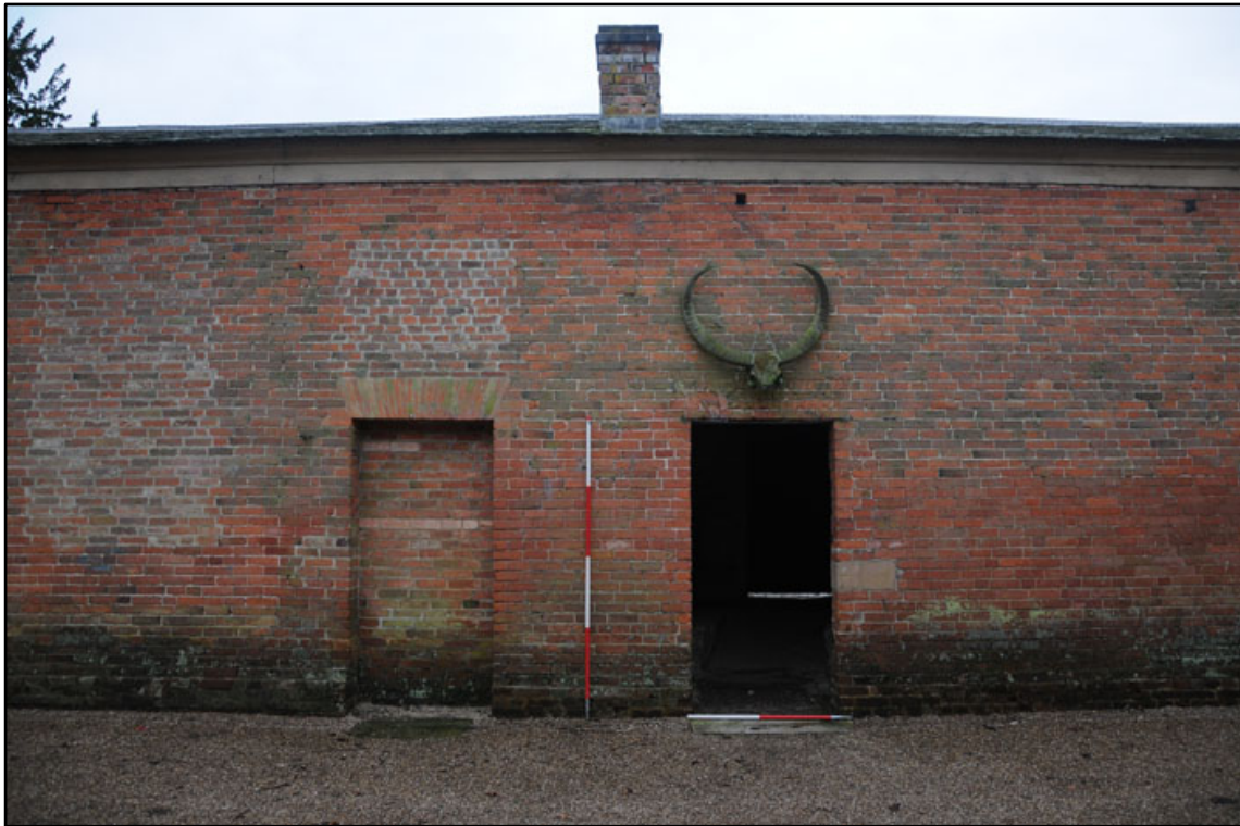
Appendix 2.13: General view of D2 and blocked D5 on north elevation – door open (2m scale).
