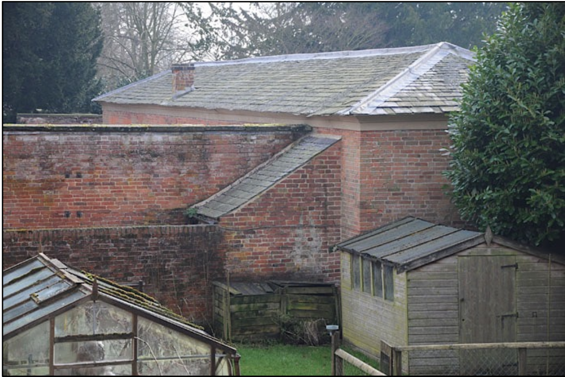
Appendix 2.5: General view of northwest corner of the South Range, looking southeast.
