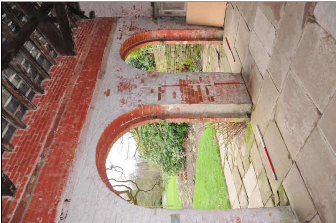
Appendix 2.28: Detail of southwest corner of G1 ; note inserted timber above arches (1m/2m scale).
