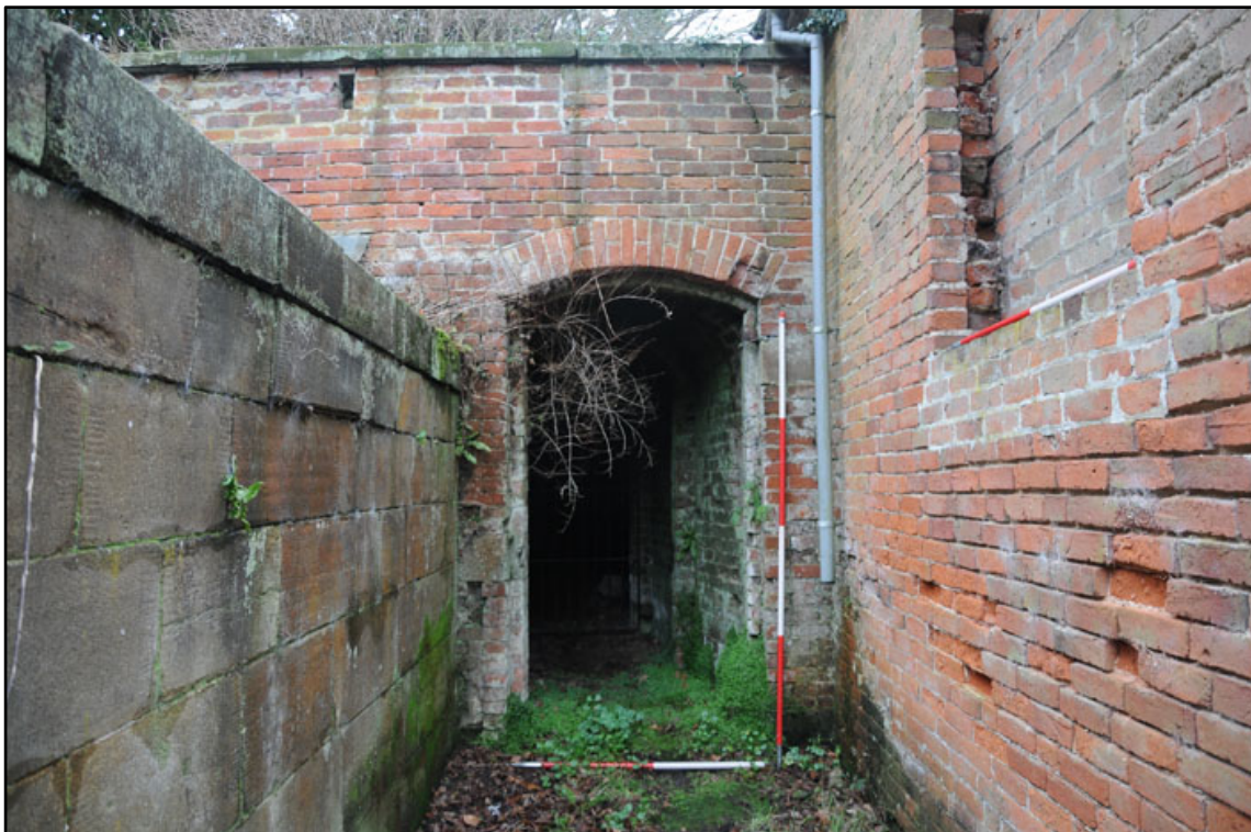
Appendix 2.8: Detail of entrance to Ice House; note bricked up joist holes at top of wall (2m scale).
