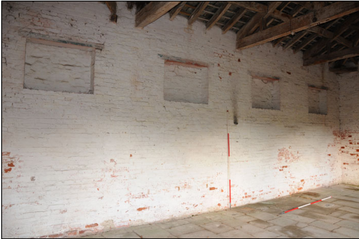
Appendix 2.47: General view of north wall of G3, looking east; note blocked in windows (2m scale).
