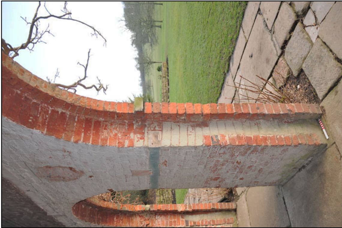
Appendix 2.27: Detail of cement repair to jamb of A2 , looking east (20cm scale).
