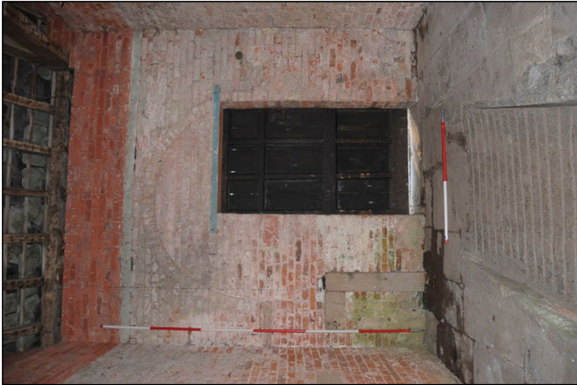
Appendix 2.37: General view of south wall of G2; note exposed timber wall-plate (1 m/2m scale).
