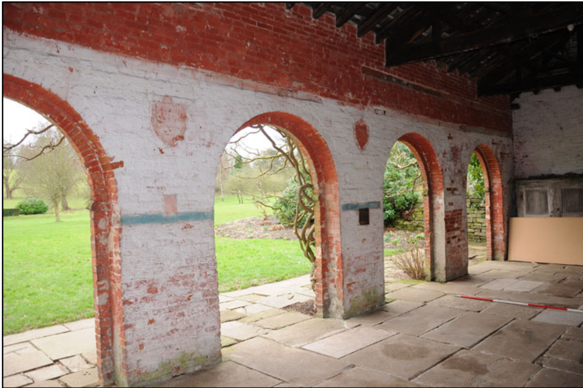
Appendix 2.23: General view of internal south elevation of G1 , looking southwest (2m scale).
