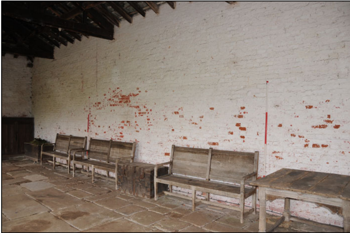
Appendix 2.25: General view of rear blind wall of GI, looking northwest (2m scale).
