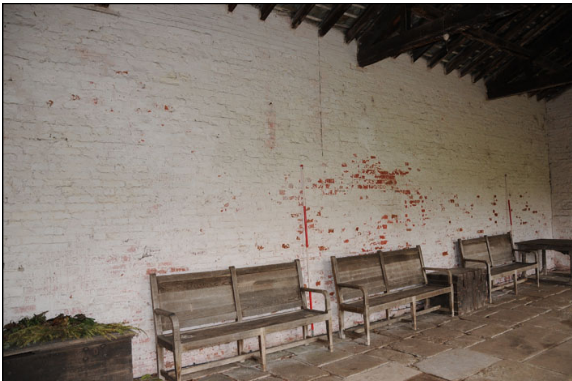
Appendix 2.26: General view of rear blind wall of GI, looking northeast (2m scale).
