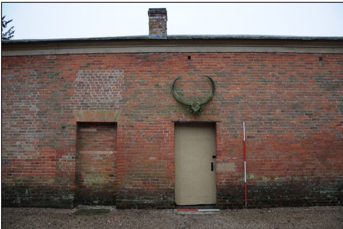
Appendix 2.14: General view of D2 and blocked D5 on north elevation – door closed (2m scale).
