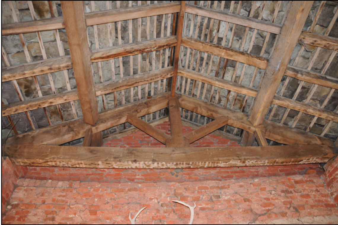
Appendix 2.41: Detail of truss T4 in in G2, looking west; note lath and plaster scars on underside of tie-beam.
