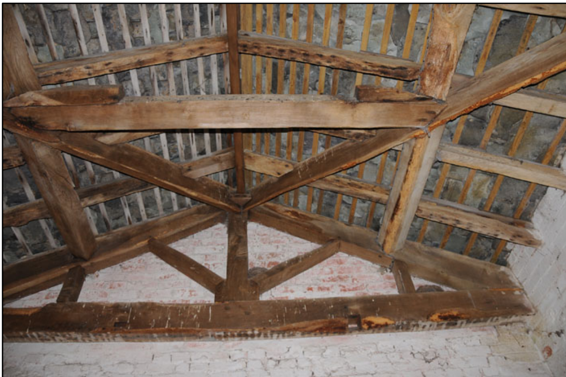
Appendix 2.53: Detail of roof construction at west end of G3 ; note former sloping timbers from removed hip roof.
