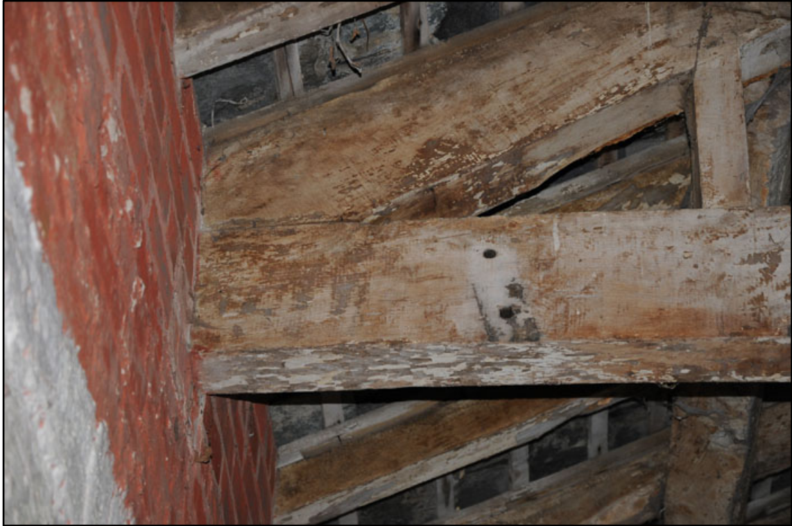
Appendix 2.60: Detail of site of former fixing bracket on underside of T7 in G3..
