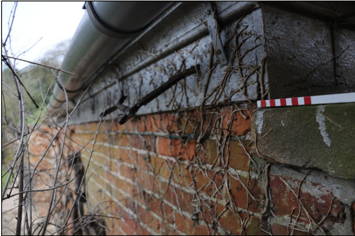
Appendix 2.19: Detail of surviving in-situ gutter bracket with V-profile at southeast end of south facade (20cm scale).
