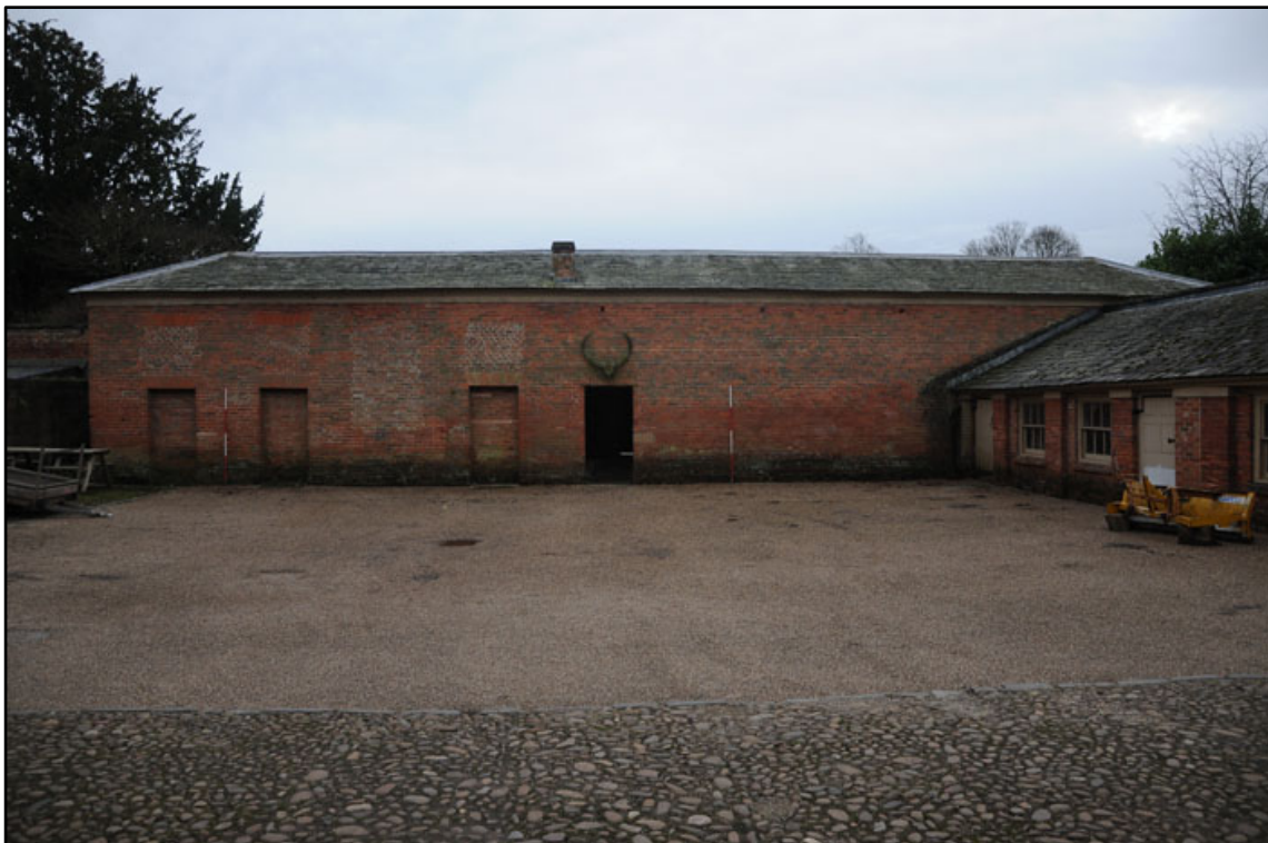
Appendix 2.10: General view of north elevation, looking south across Brewhouse Yard (2m scale).
