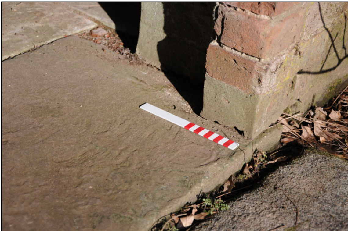
Appendix 2.32: Detail of paving continuing beneath brick jamb of A2, in A1; note cement repair (20cm scale).
