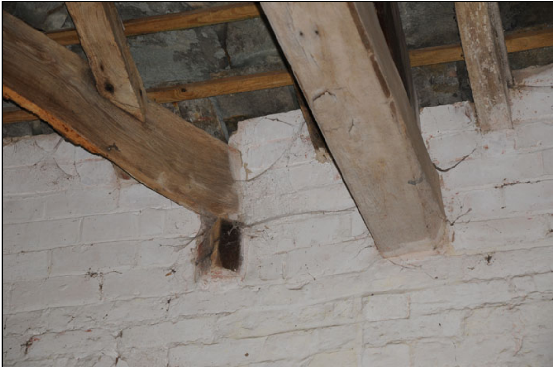
Appendix 2.54: Detail of sawn off corner tie adjacent to T6 in north wall of G3; note replaced tie beam.
