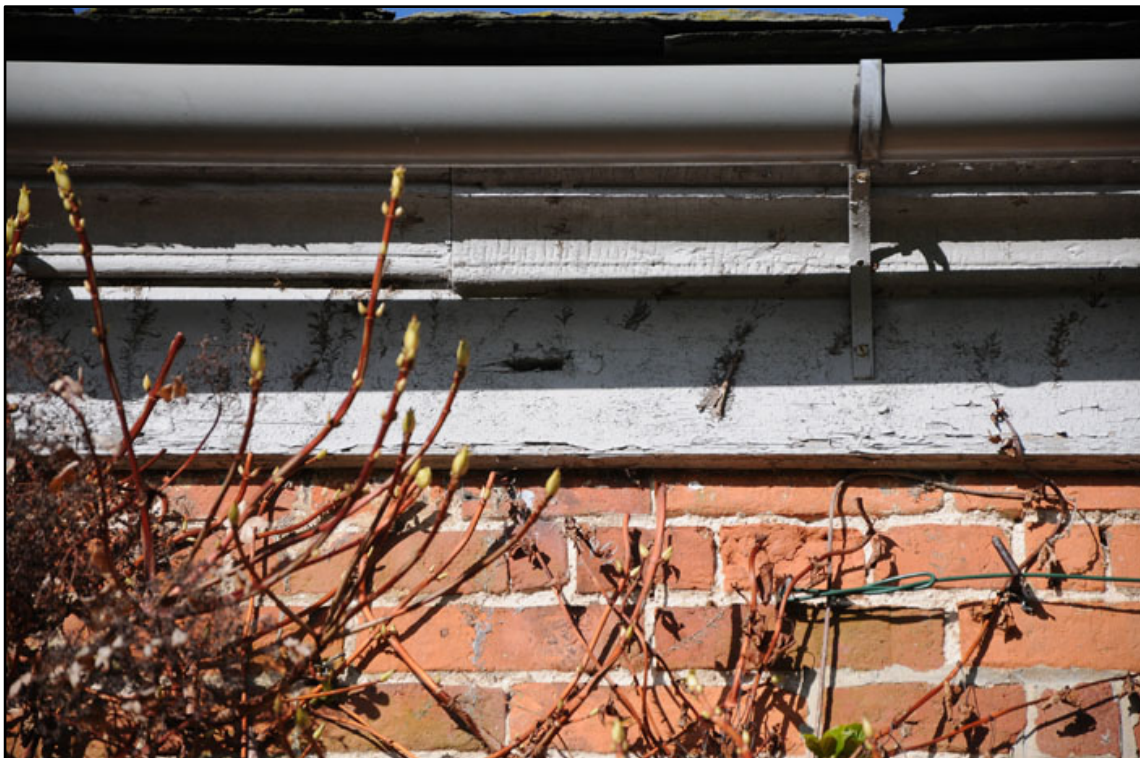
Appendix 2.20: Detail of fixing hole for former gutter bracket on soffit board of south facade.
