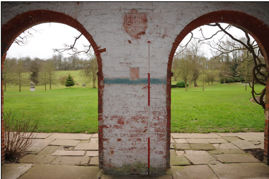
Appendix 2.24: Detail of arcade openings and pier between A3 and A4 in G1 ; note sawn off timber (2m scale).
