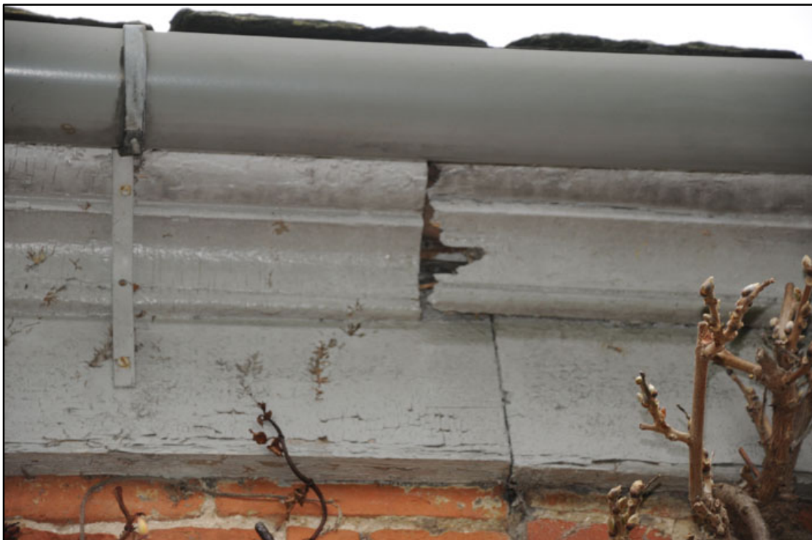
Appendix 2.18: Detail of timber mouldings at eaves level of south façade; note modern gutter fixing.
