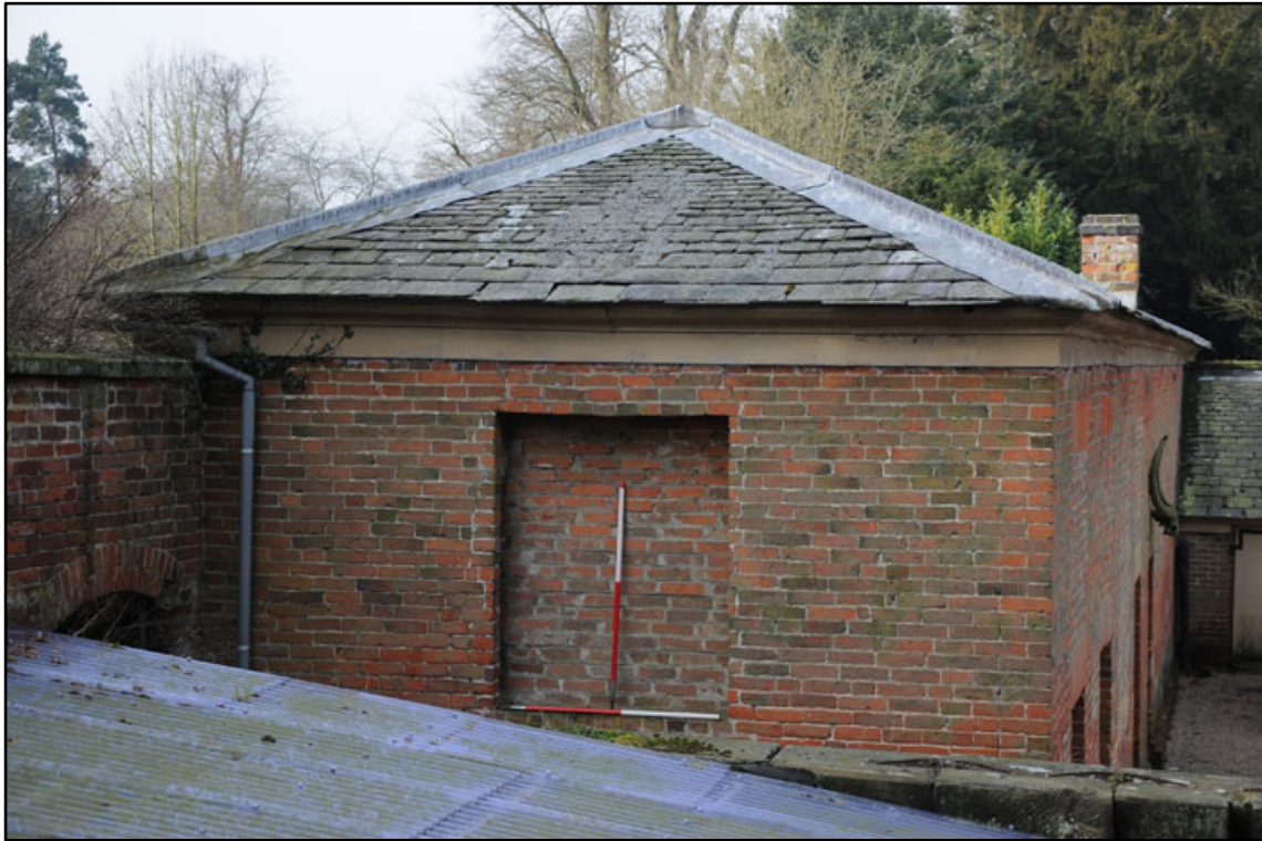
Appendix 2.7: Detail of false window W5 in east elevation; note lack of lintel detail (1m scale).
