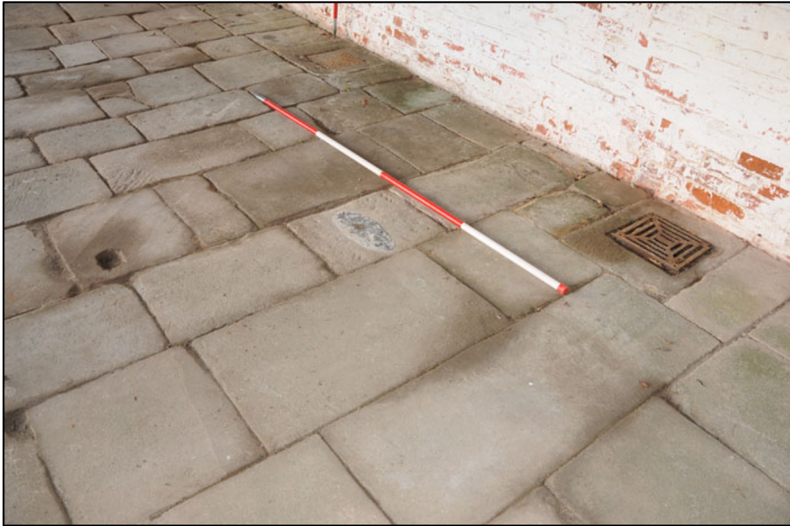
Appendix 2.49: General view of Drain and sockets in paving along north wall of G3 (2m scale).
