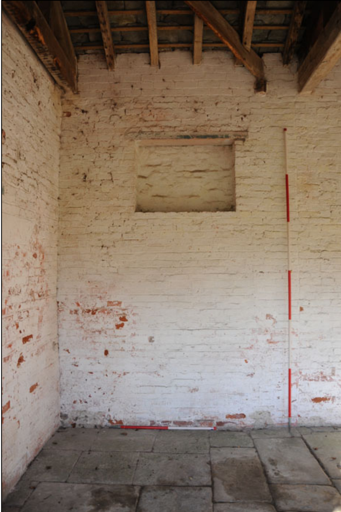
Appendix 2.51: Detail northwest corner of G3; note vertical joint to the right of ranging pole (1m/3m scale).
