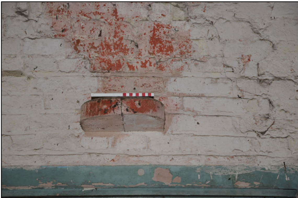
Appendix 2.59: Detail of inserted timber ledge above D4 in G3 (20cm scale).
