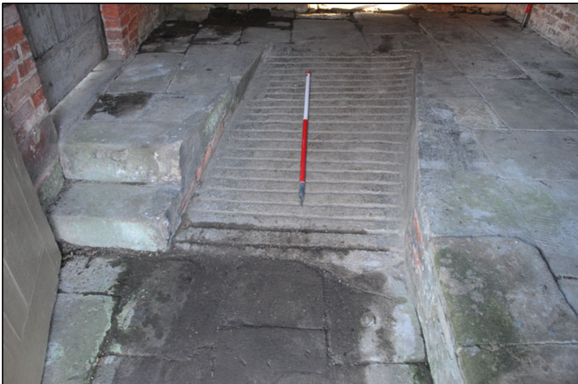
Appendix 2.40: General view of inserted concrete ramp in G2, looking south (1m scale).
