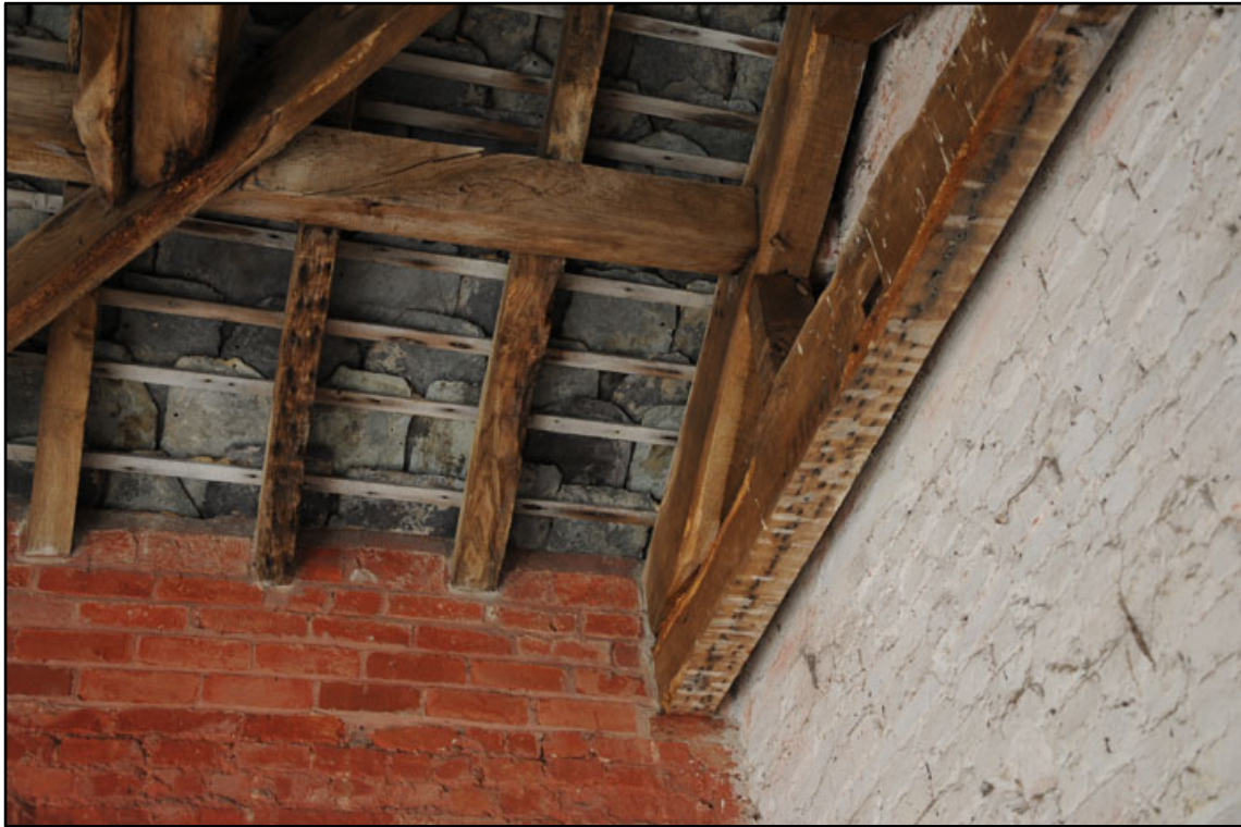
Appendix 2.58: Detail of underside of truss T5 in G3 ; note lath and plaster scars from removed ceiling.
