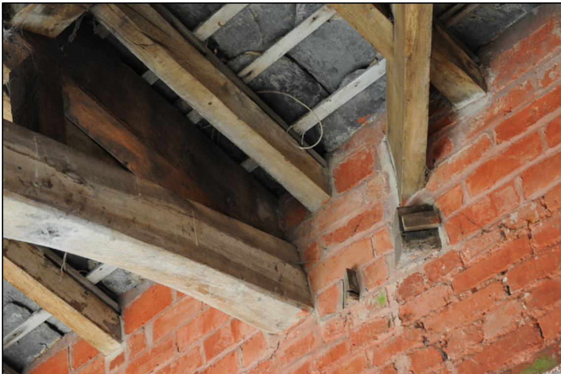
Appendix 2.55: Detail of sawn off corner tie adjacent to T6 in south wall of G3; note replaced tie beam
