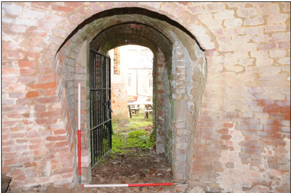
Appendix 2.71: General view looking along entrance passage G4 into Ice House, looking northwest (2m scale).
