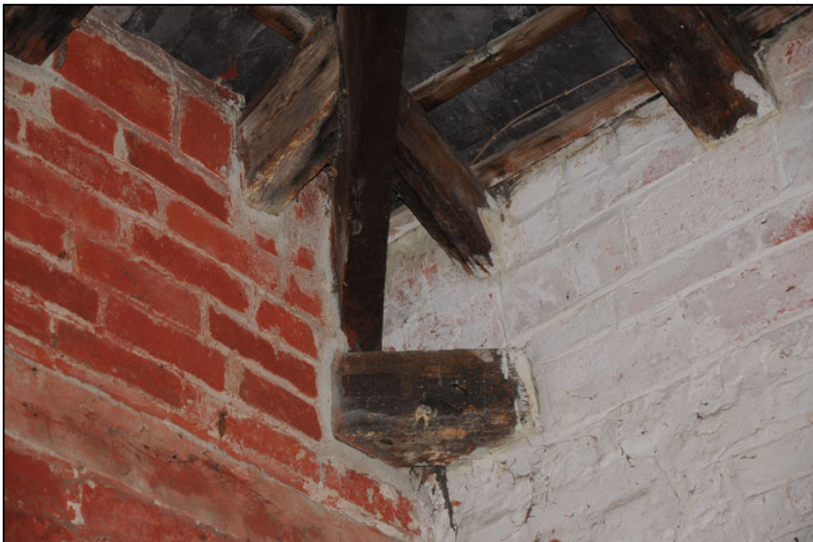
Appendix 2.34: Detail of corner tie in northwest corner of GI; note bricked up upper section of walling.
