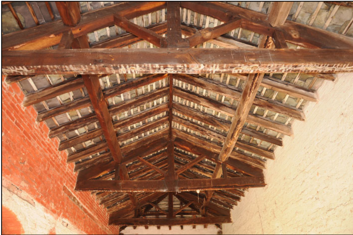
Appendix 2.33: General view of roof structure in GI; note dark coloured, unpainted timbers.
