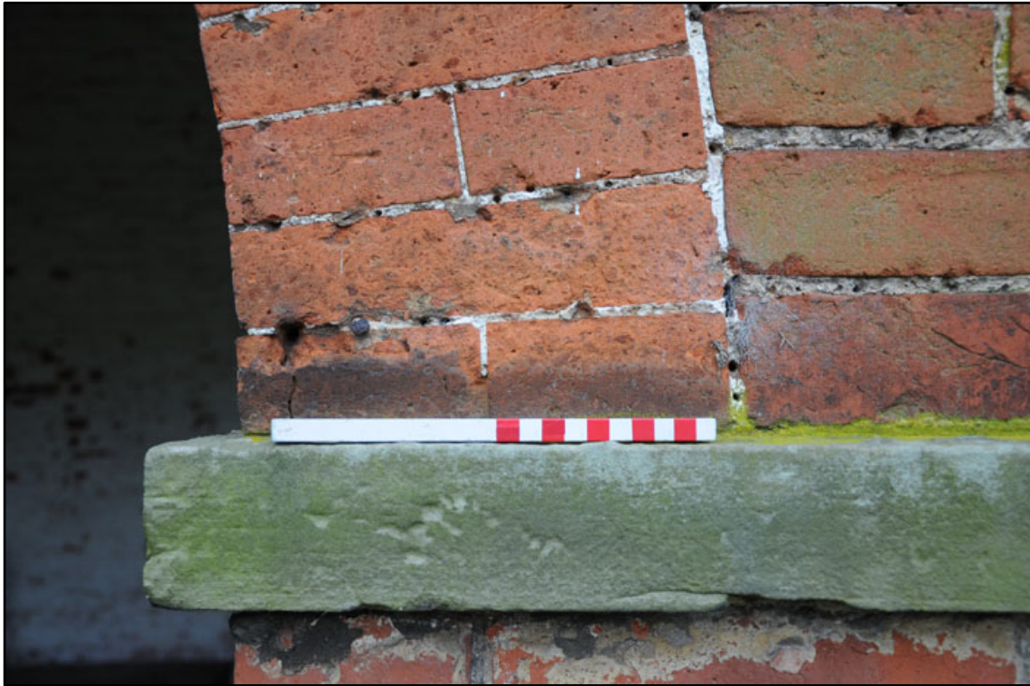
Appendix 2.15: Detail of rubbed brick detailing of arch with thin joints on south facade (2m scale).
