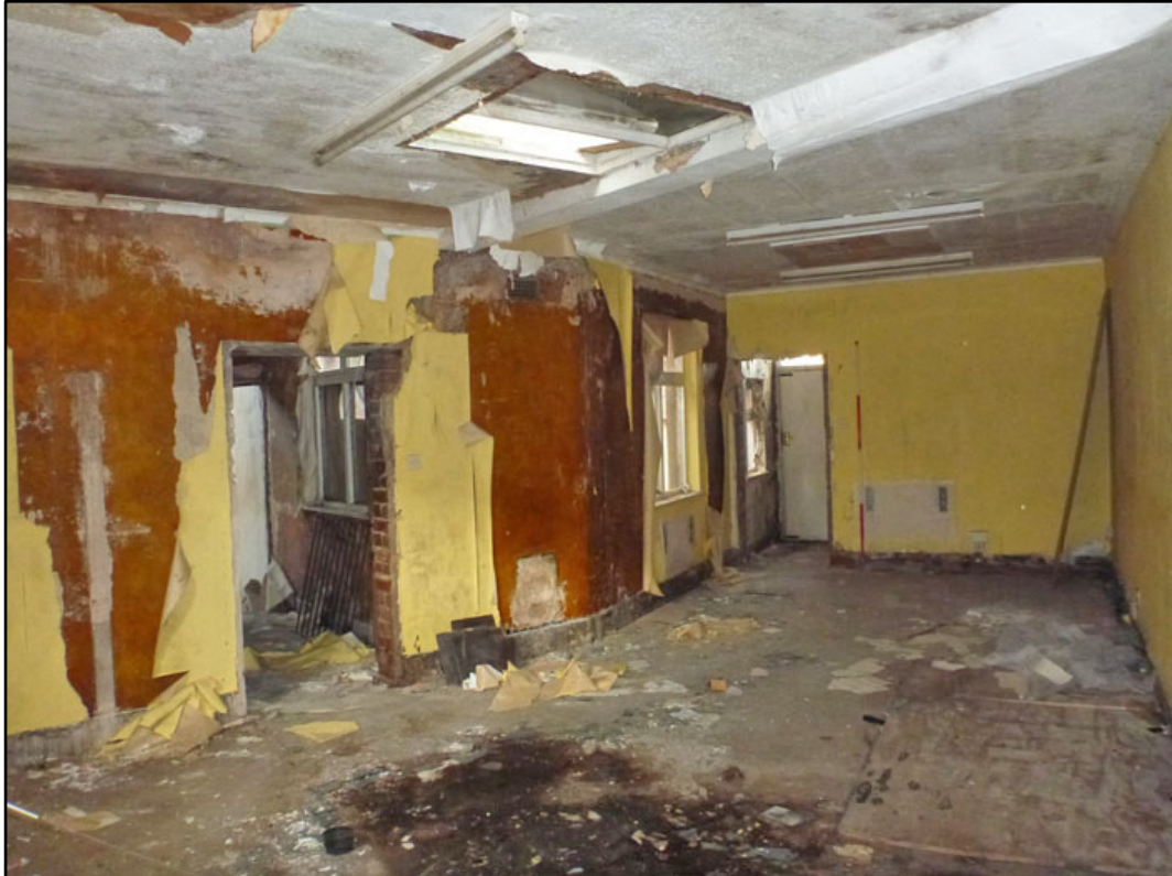
Appendix 3.10: General view of flat roofed section of ground floor, looking north (2m scale).
