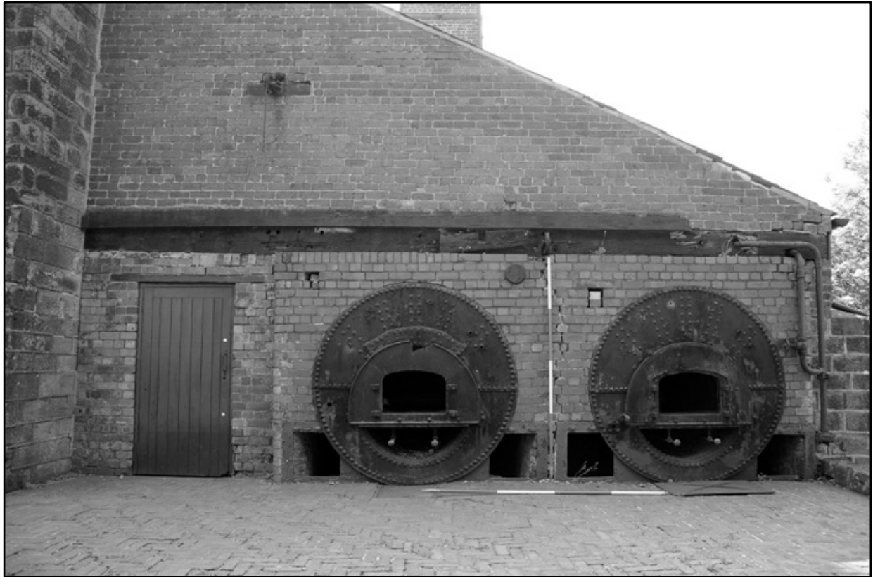
Appendix 2.8: Detail of north elevation, looking south; note structural crack and timber lintel. Film 1.23.
