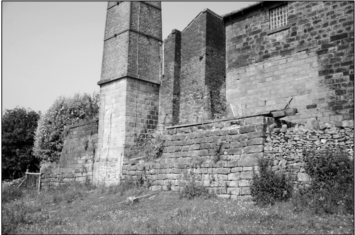
Appendix 2.4: General view of south elevation and chimney, looking northwest (3m scale). Film I.9.
