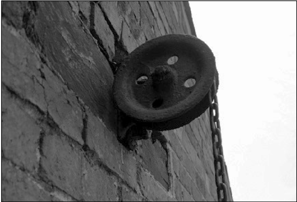
Appendix 2.11: Detail of pulley wheel above boilers in gable of north elevation.
