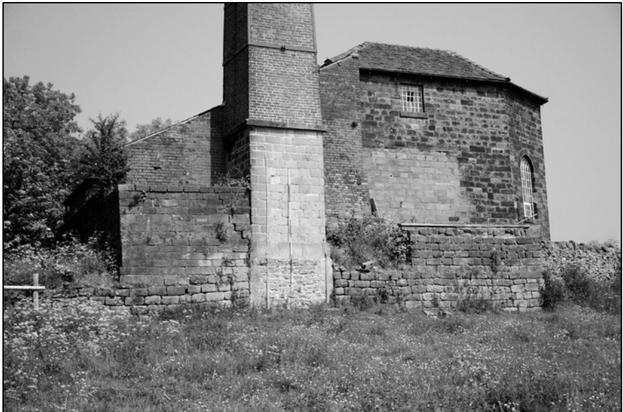
Appendix 2.5: General view of south elevation and chimney, looking northeast (3m scale). Film I.12.
