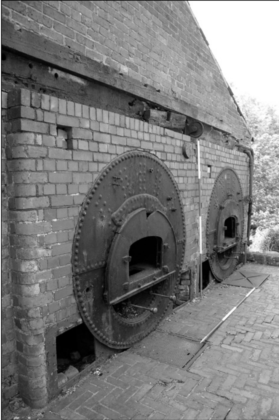
Appendix 2.10: Detail of north elevation, looking southwest; note boilers with brick walling (2m scale). Film 1.27.
