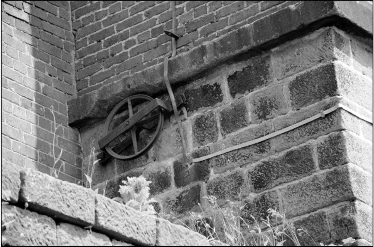
Appendix 2.6: Detail of wheel (for possible damper) on southwest side of chimney. Film 1.14.
