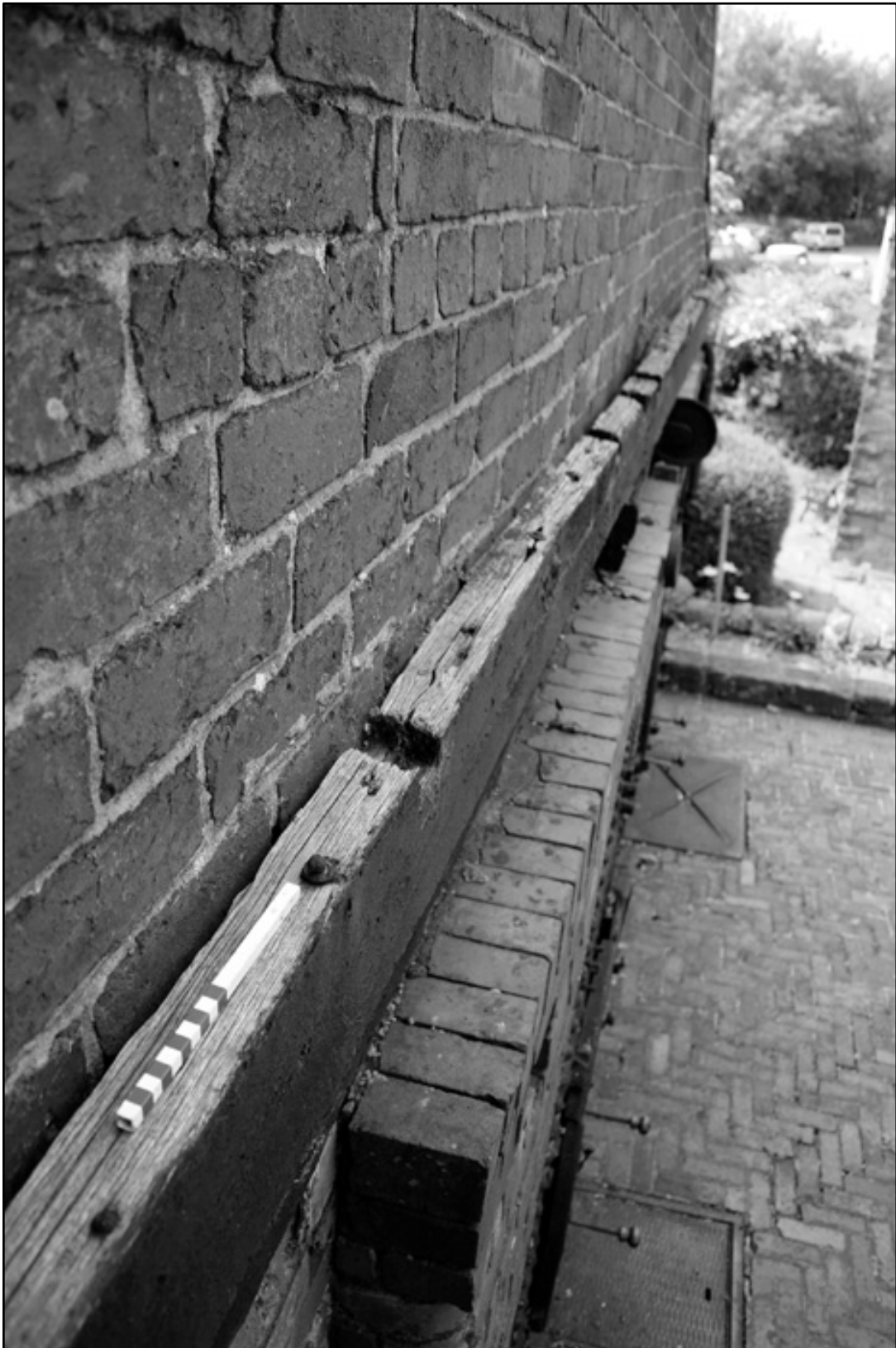
Appendix 2.13: Detail of timber beam along north elevation from above; note empty slots for roof joists (20cm scale). Film I.29.
