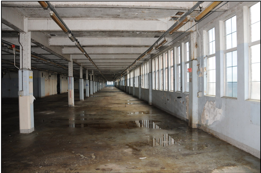
General view of sixth floor of Cream Block, looking north (2m scale))
