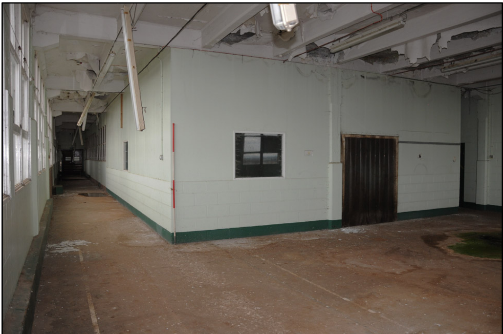
Detail of sixth floor of Almond Block; note inserted modern partition (2m scale)
