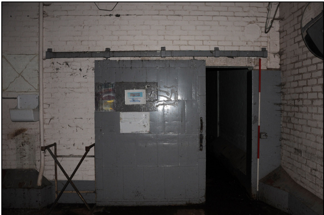
Detail of sliding door on fifth floor of Almond Block; note metal sheets (2m scale)
