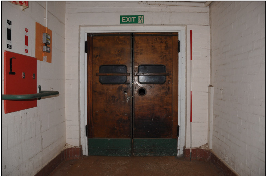
Detail of wooden swing doors on forth floor of Almond Block (2m scale)
