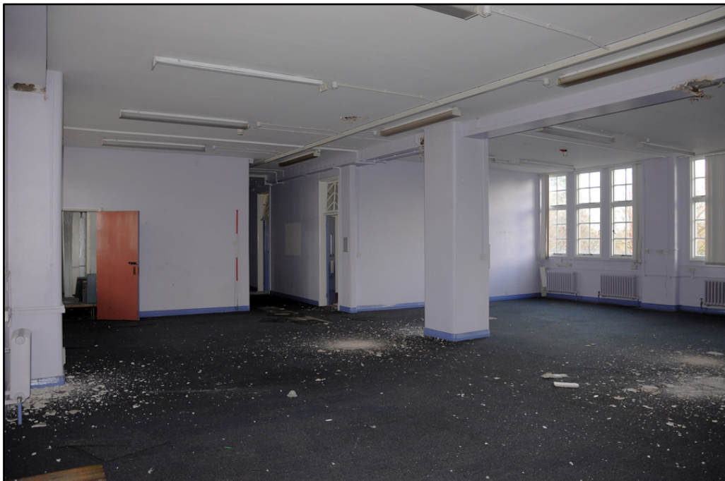
Detail of second floor rooms in 1936 three-storey section of the Cream Block (2m scale)
