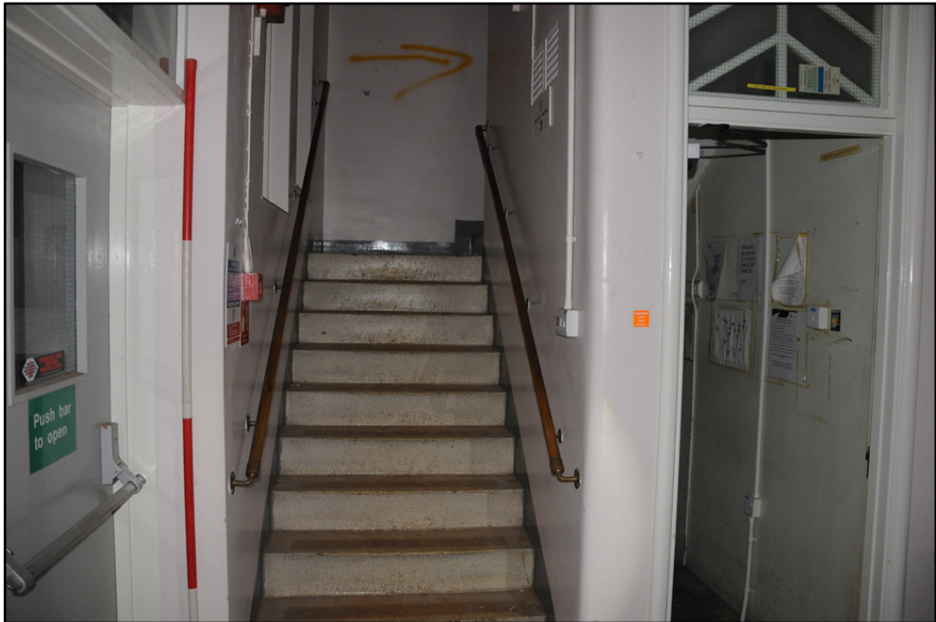
View of staircase at north end of three-storey section of Cream Block; note timber handrails (2m scale)
