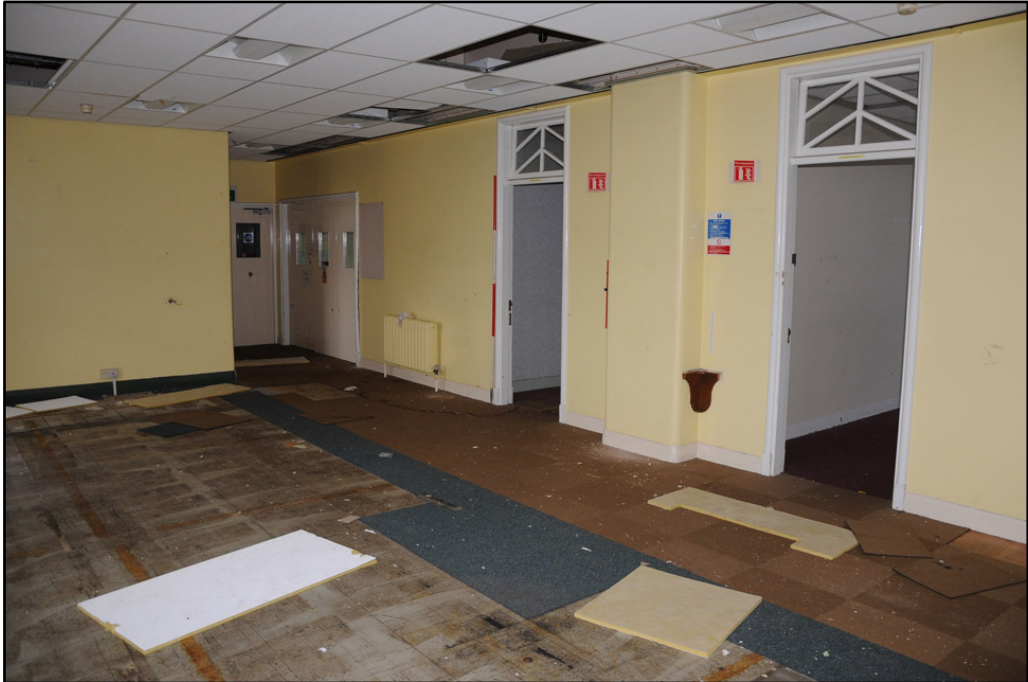
Detail of first floor rooms in 1936 three-storey section of the Cream Block (2m scale)
