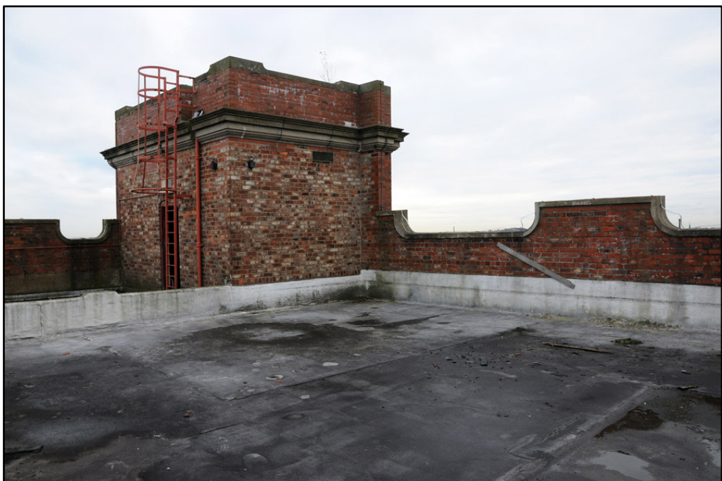
Detail of southeast corner turret on Almond Block; note ashlar cornice and decorative parapet
