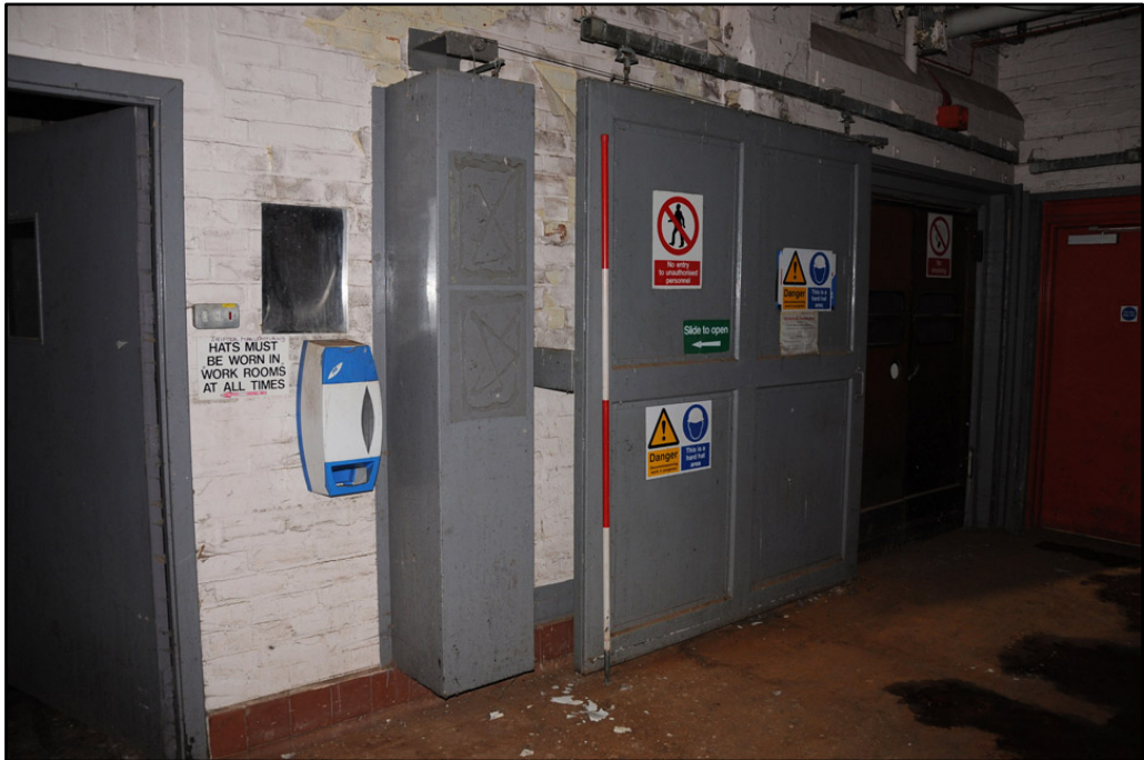
Detail of sliding door on forth floor of Almond Block (2m scale)
