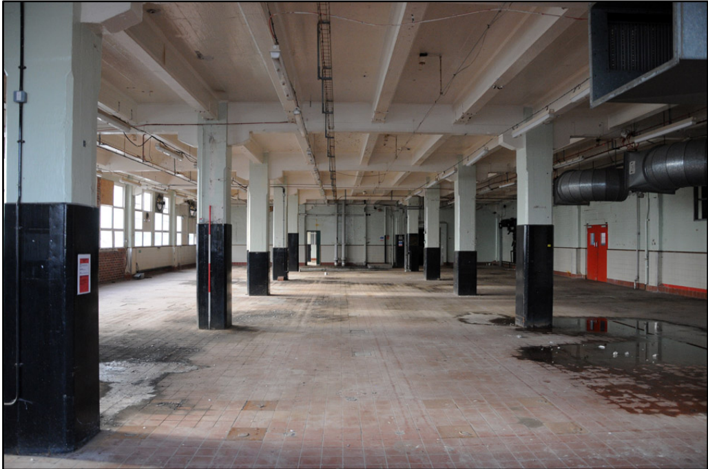
General view of third floor of Almond Block; note exposed concrete superstructure (2m scale)
