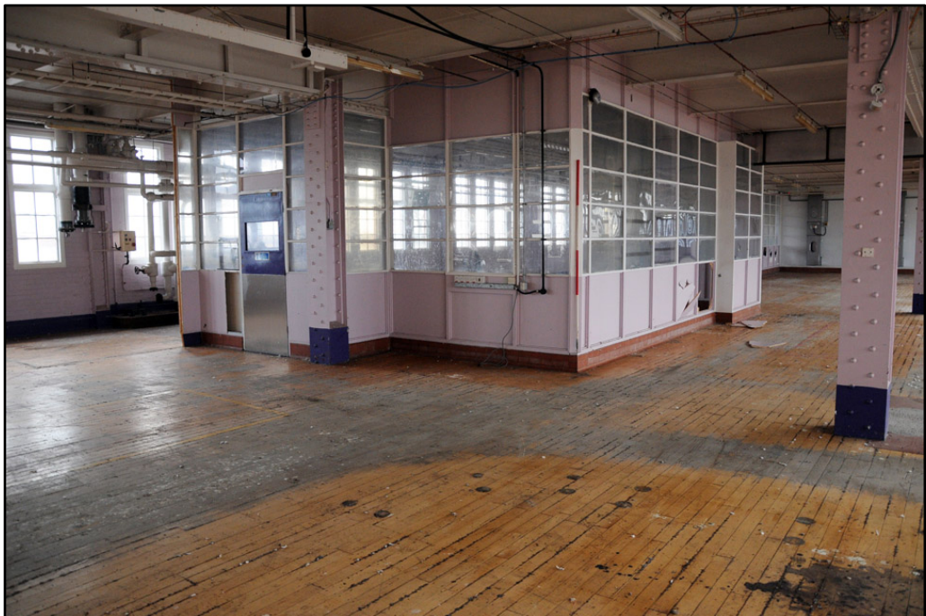
Detail of inserted office within fifth floor of Cream Block; note ware pattern in floor (2m scale)
