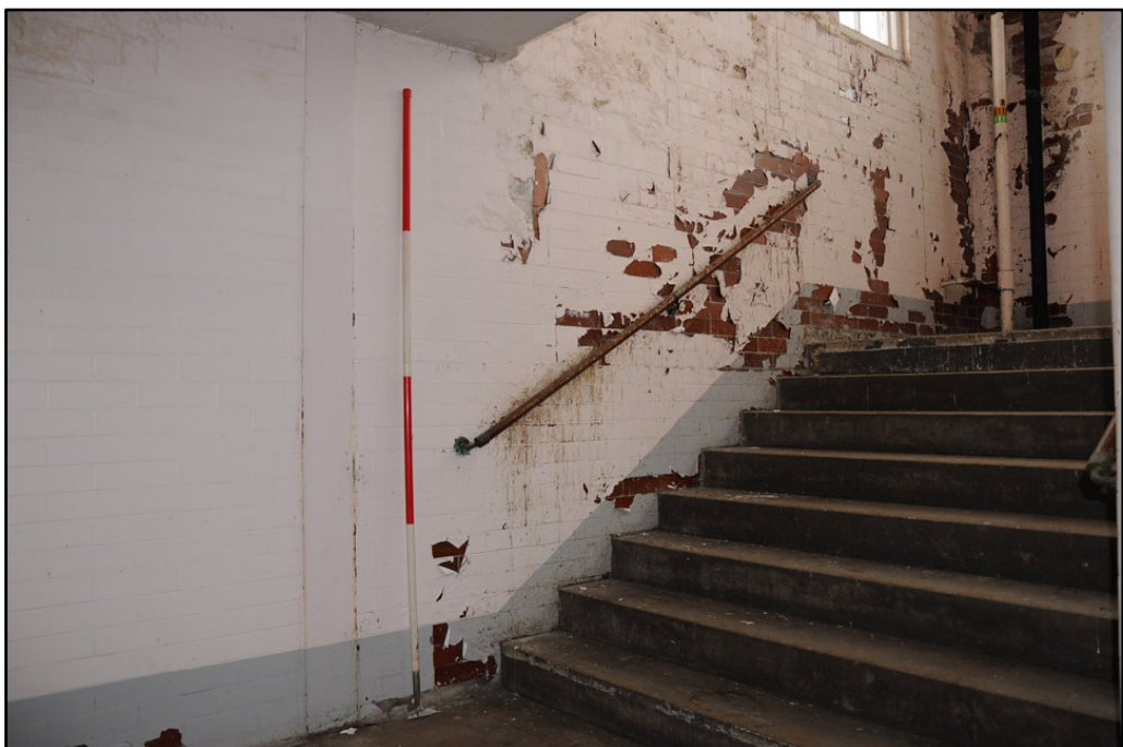
Detail of north stairwell on fifth floor of Cream Block; note brown glazed tiles (2m scale)
