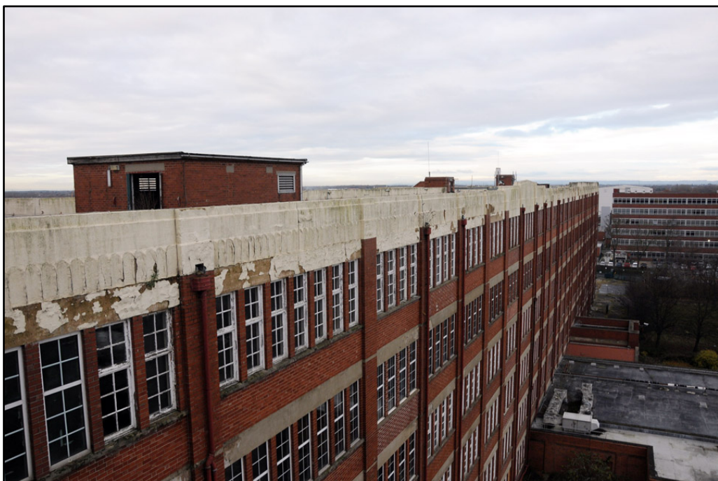
General view of upper part of east elevation of Cream Block, looking northwest
