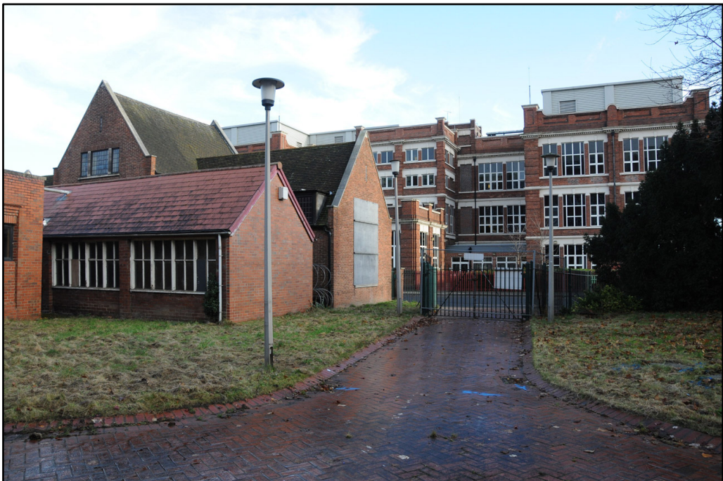
View looking northeast of the external elevation of the subway corridor; note extensive fenestration
