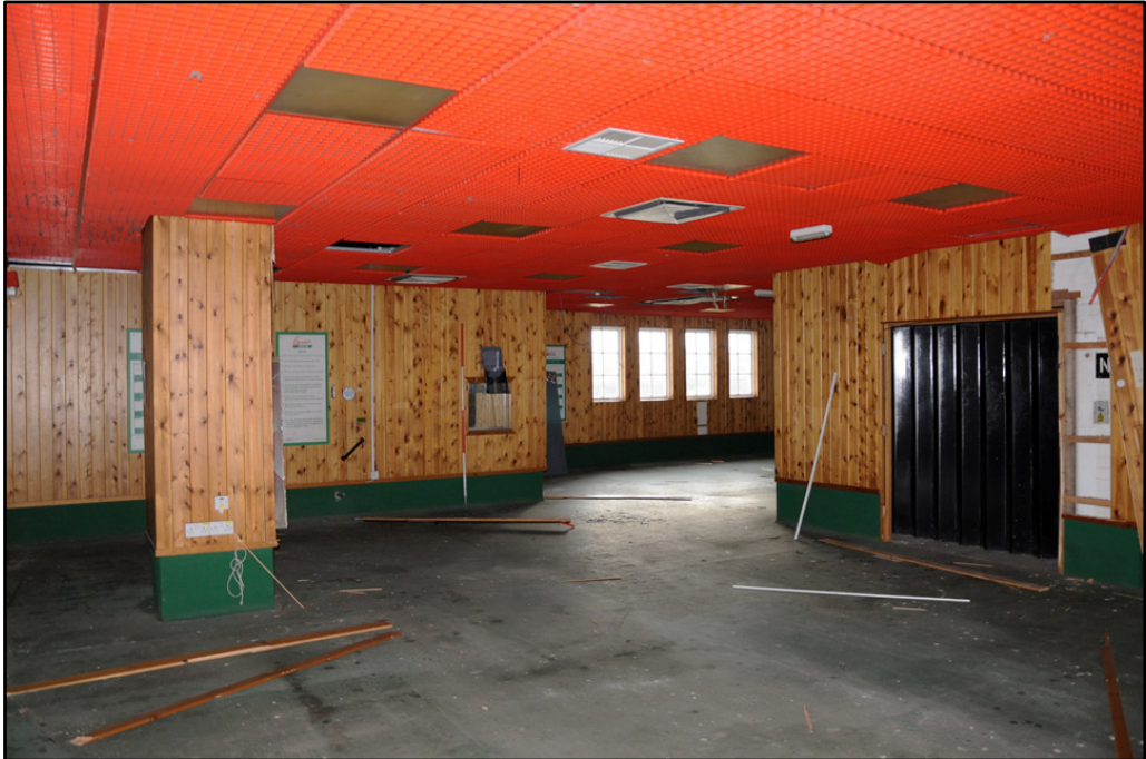
General view of fourth floor gym in northwest area of fourth floor of Cream Block (2m scale)
