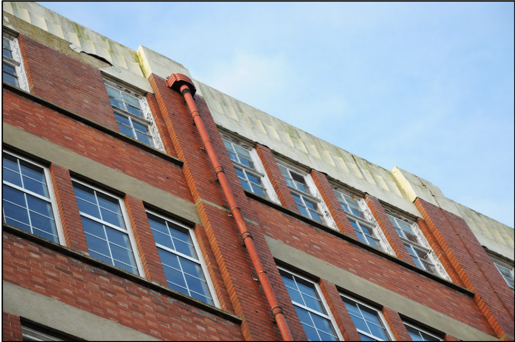
Detail of downpipes and deco inspired hopper heads on east elevation of Cream Block
