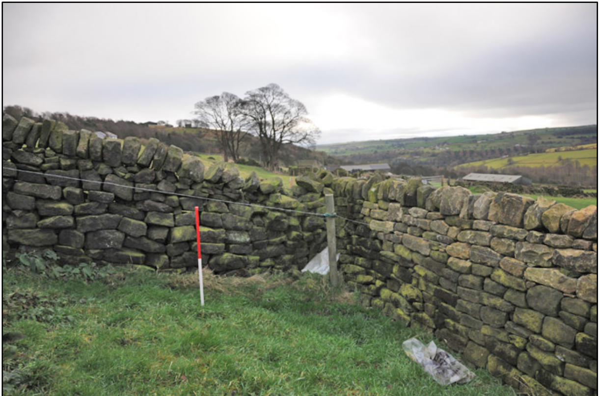
Appendix 3.4: Detail of wall junction in southeast corner of field F1b , looking east (1m scale).
