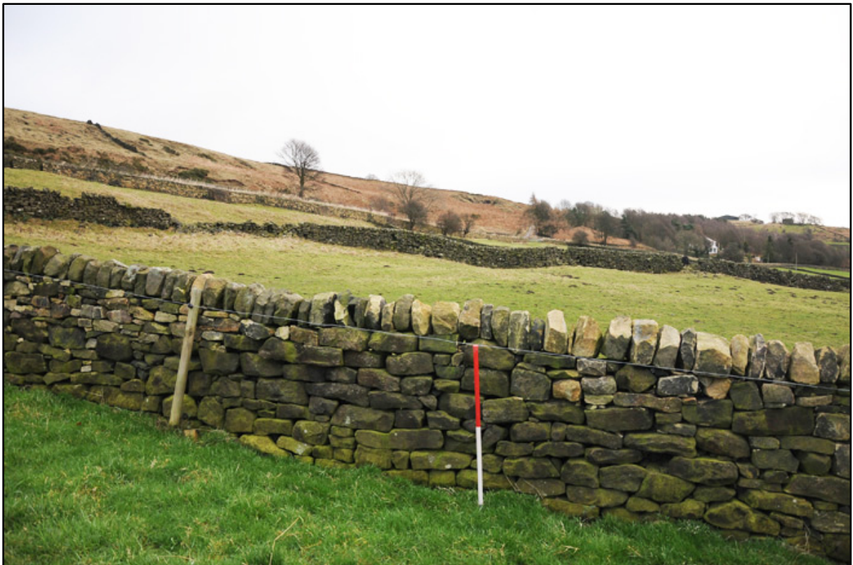
Appendix 3.2: Detail of section of wall in field F1b , where new opening will be made for proposed roadway (1m scale).
