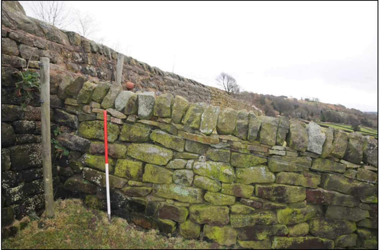
Appendix 3.3: Detail of wall junction in northeast corner of field F1a , looking east (1m scale).
