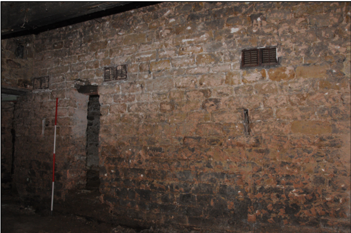
Appendix 5.67: General view of south wall of cart shed G8, looking southeast; note inserted vents (2m scale)
