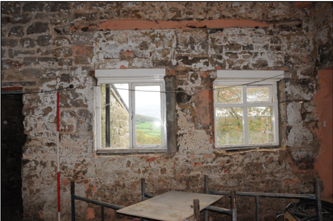
Appendix 5.65: Detail of altered windows in north wall of G4 , possibly associated with former stable (2m scale)
