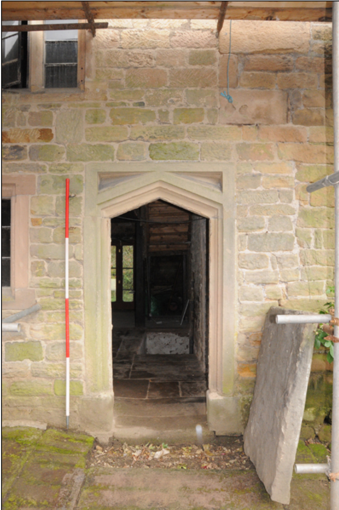
Appendix 5.11: Detail of doorway into room G1; note truncated quoins from phase I house (2m scale)
