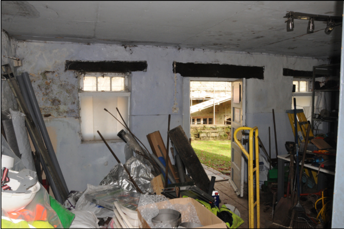
Appendix 5.72: General view of ground floor of former stable in T-shaped barn, looking north
