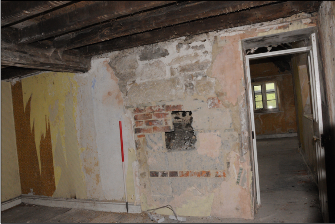
Appendix 5.42: General view of FI, looking northeast; note blocked fireplace (1m scale)
