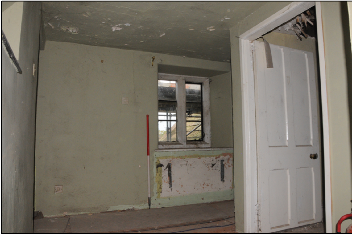
Appendix 5.40: General view of inserted landing (phase 9) at west end of F4, looking north (1m scale)
