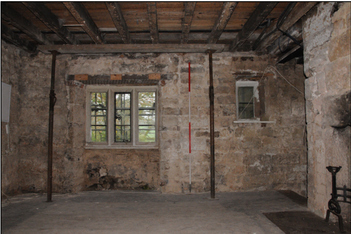
Appendix 5.19: General view of altered window (phase 7) in north wall of GI (2m scale)
