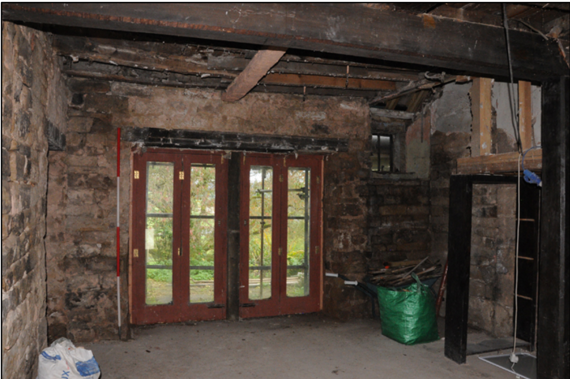
Appendix 5.29: Detail of inserted (phase 9) doors in north wall of G3; note overhead beam marking former partition (2m scale)
