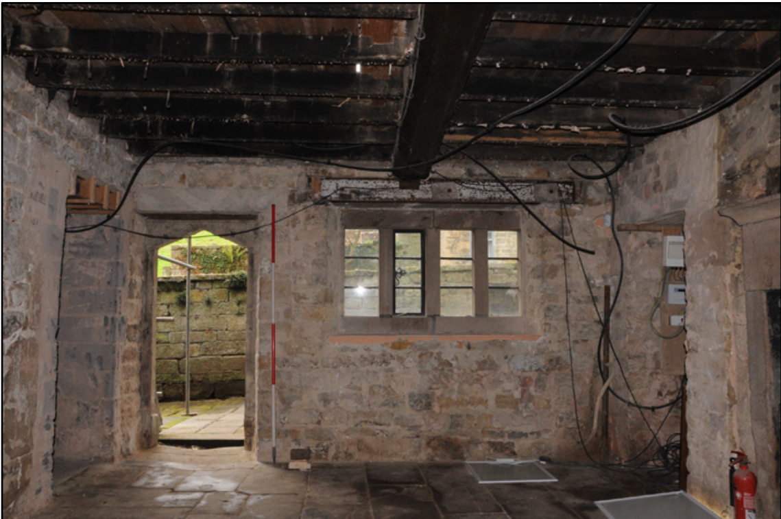
Appendix 5.27: General view of south wall and inserted window (phase 7) in G3 (2m scale)
