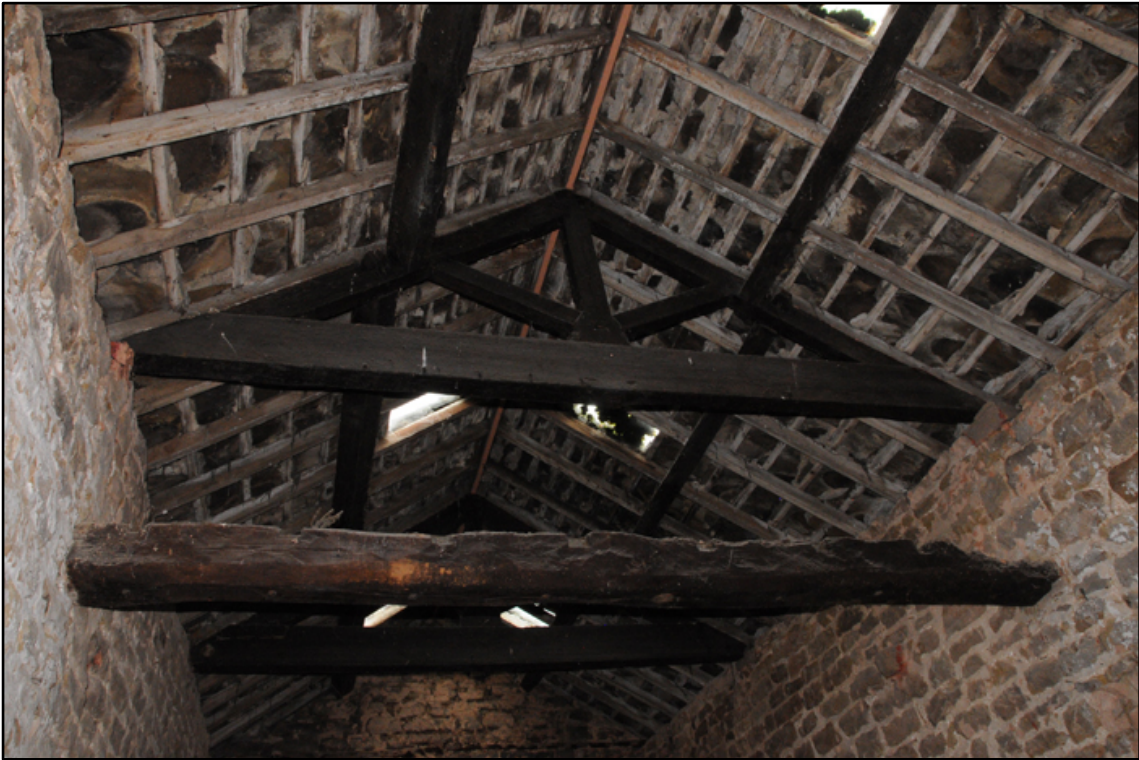
Appendix 5.62: General view inserted beam and roof trusses in F5, looking west
