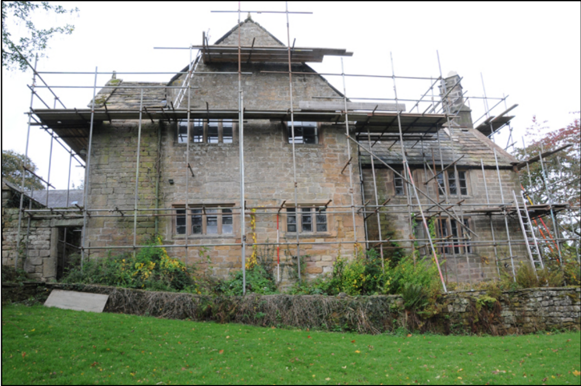
Appendix 5.12: General view of east elevation of the hall, looking west; note post 1950s terrace (2m scale)
