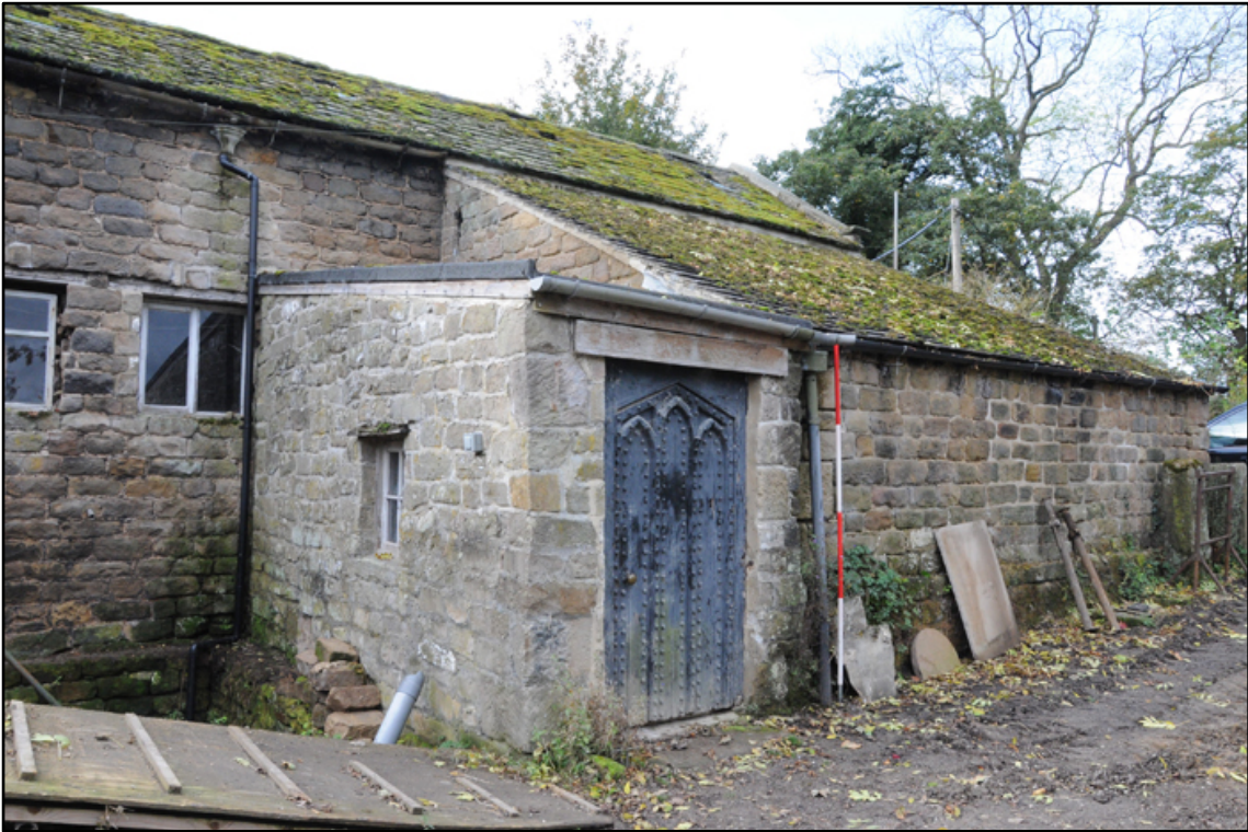
Appendix 5.60: General view of rear of cart shed G8 and passageway G10; note reused doorway from G3 (2m scale)
