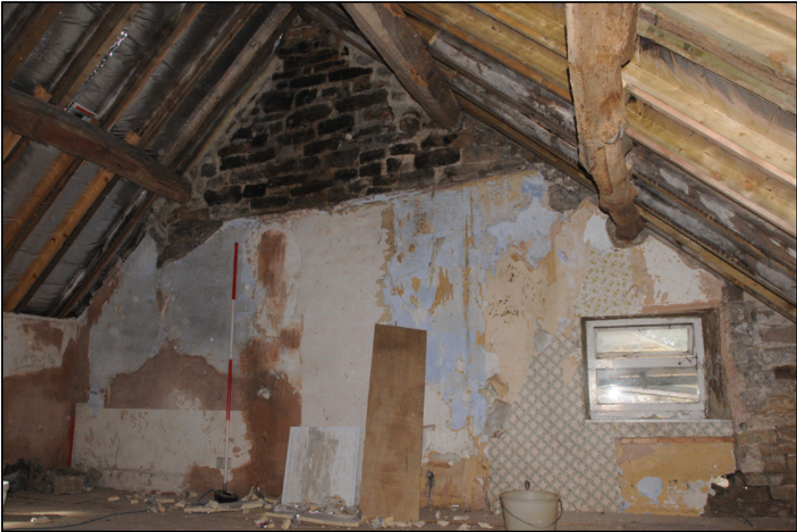
Appendix 5.48: General view of west wall of F3; note blocked doorway behind ranging pole (2m scale)
