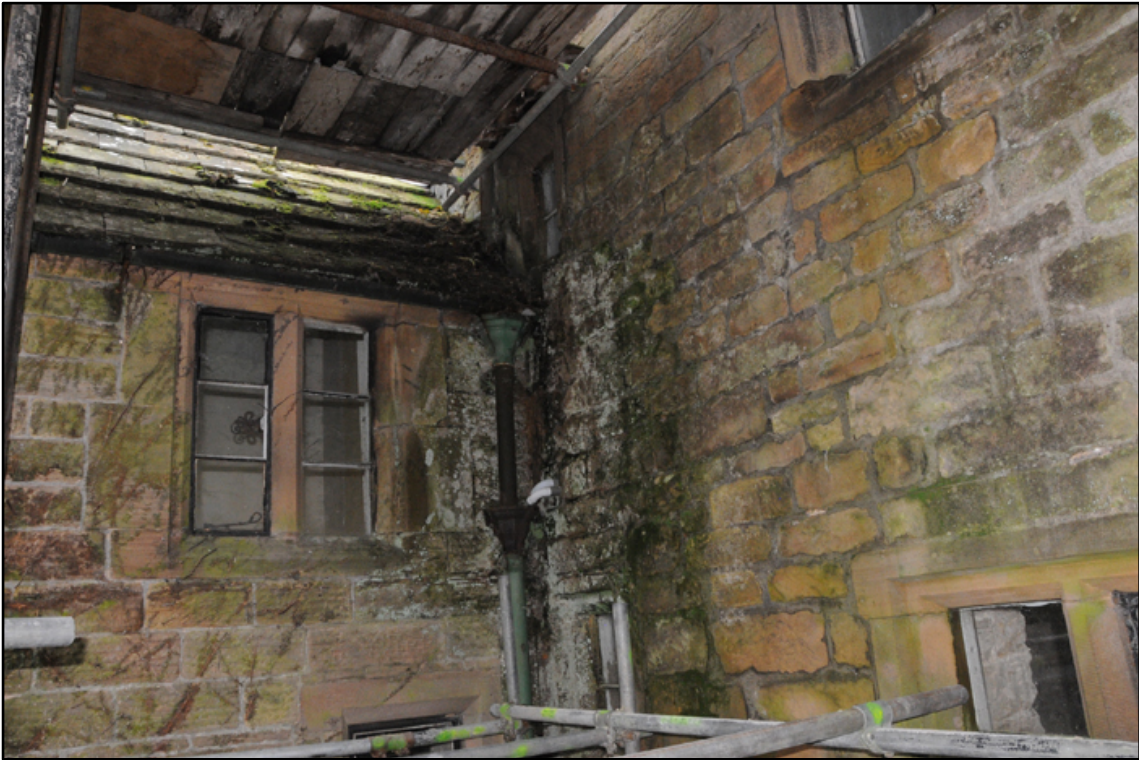
Appendix 5.14: Detail of external junction of F4 and F6; note change in coursing and size of window
