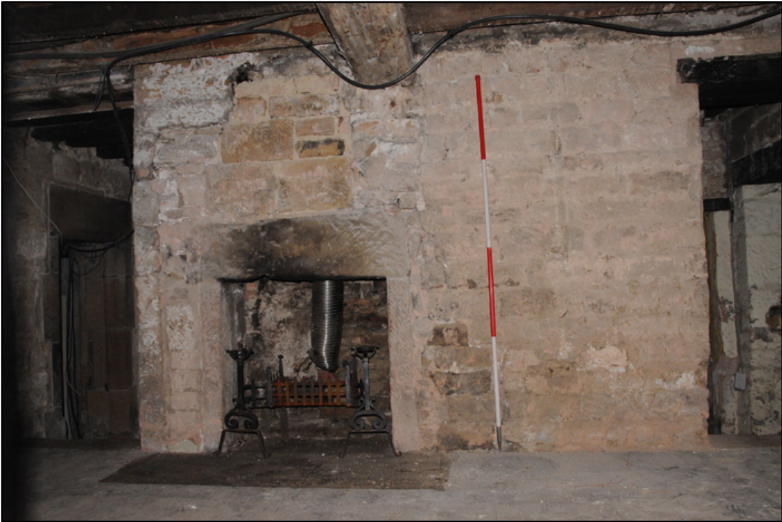
Appendix 5.18: General view of altered fireplace in GI, looking west (2m scale)
