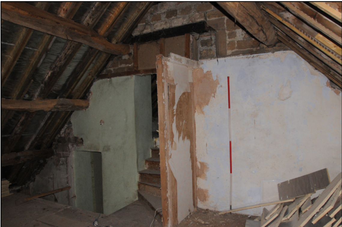
Appendix 5.49: General view of east wall of F3; note truncated (phase 1) window in apex of roof (2m scale)
