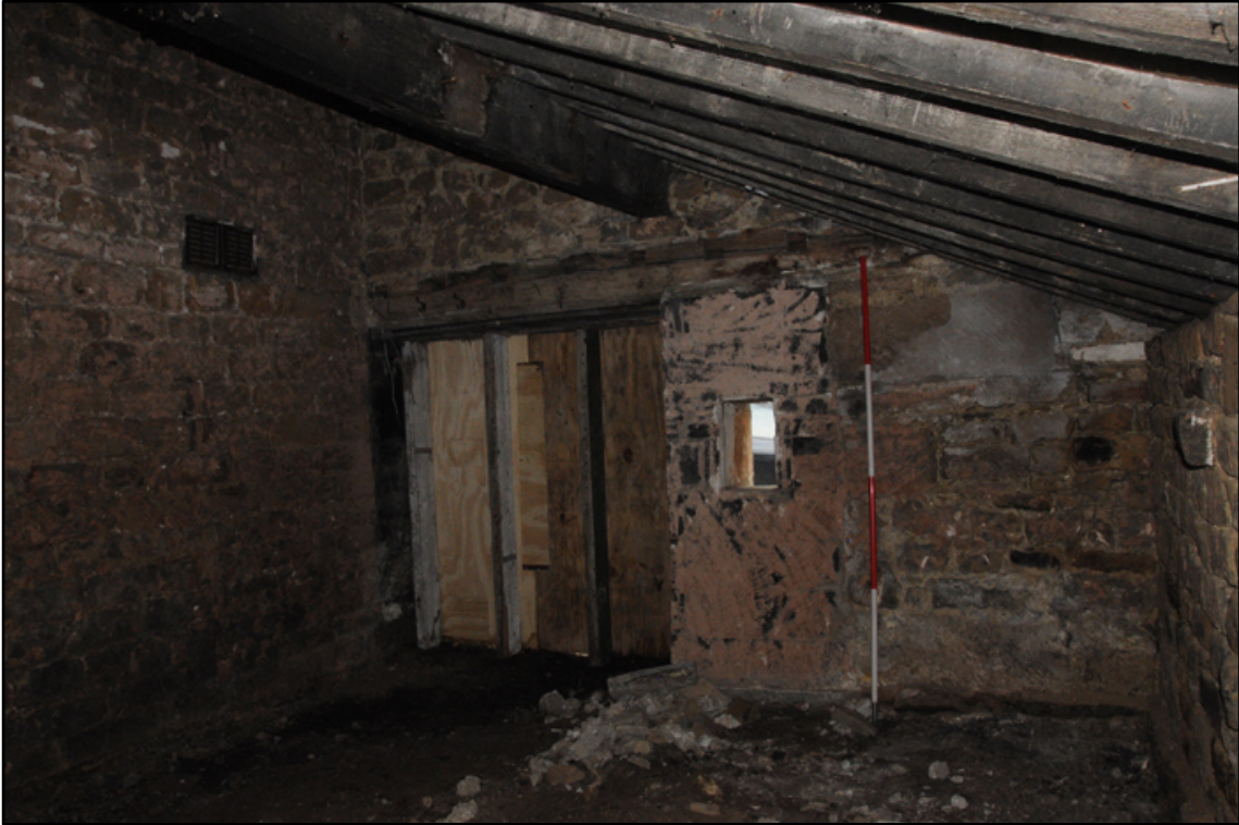
Appendix 5.66: General view of west end of cart shed (phase 5) (2m scale)
