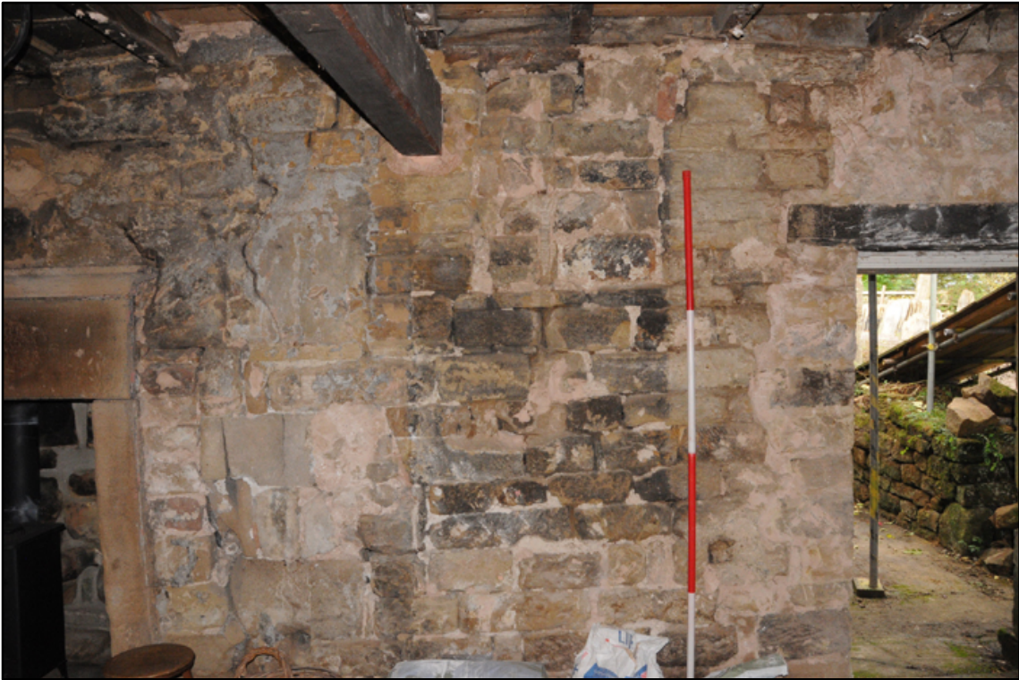
Appendix 5.30: Detail of blocked high level window in west wall of G3 (possibly reused?); note inserted door (2m scale)
