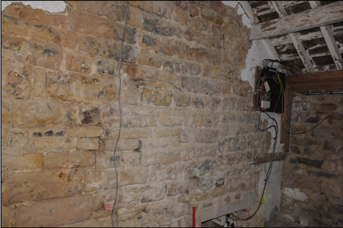
Appendix 5.38: General view of east gable of hall in G9; note vertical scar from former doorway (2m scale)
