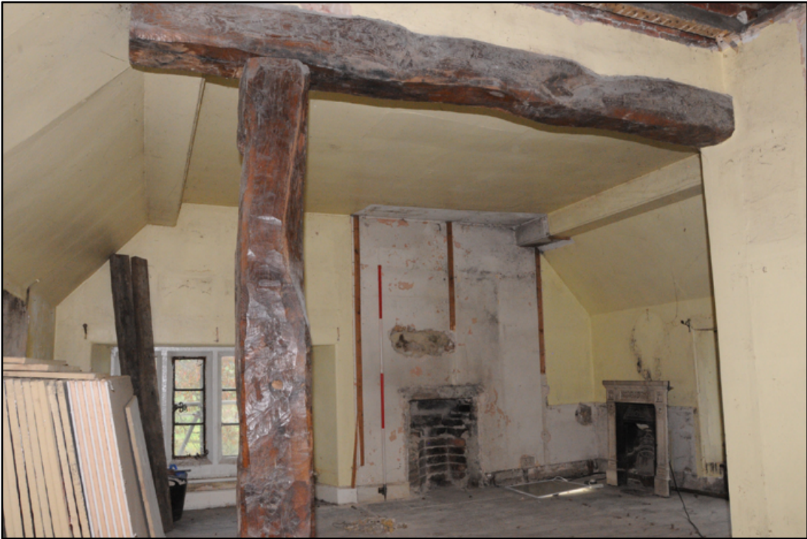
Appendix 5.44: General view of F6, looking north; note inserted timber beam (phase 7) (2m scale)
