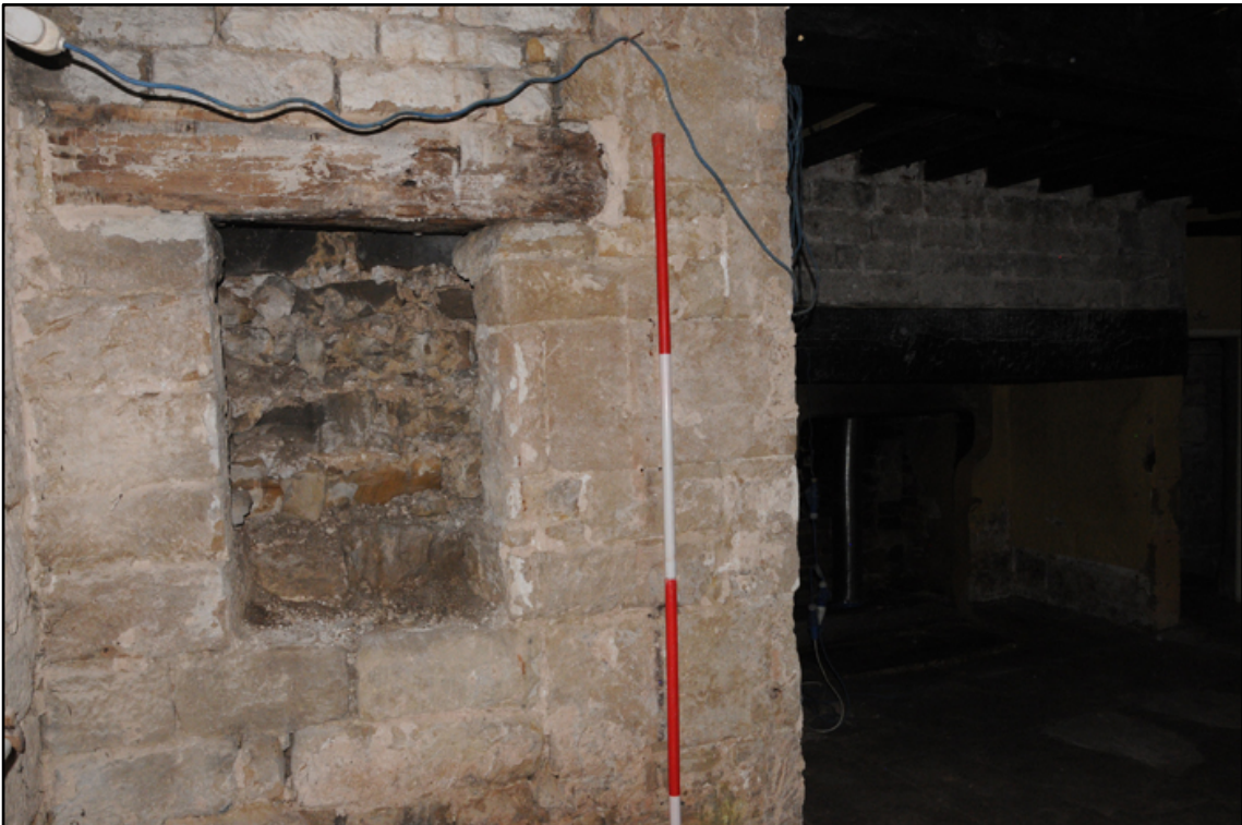
Appendix 5.25: Detail of blocked narrow window in west wall of G2 that originally looked up the entrance walkway (2m scale)
