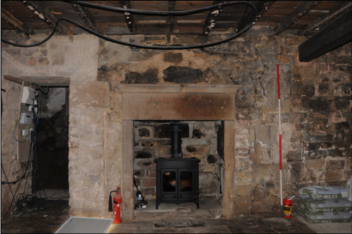
Appendix 5.26: General view of altered fireplace in west wall of G3; note truncated lintel in secondary doorway (2m scale)
