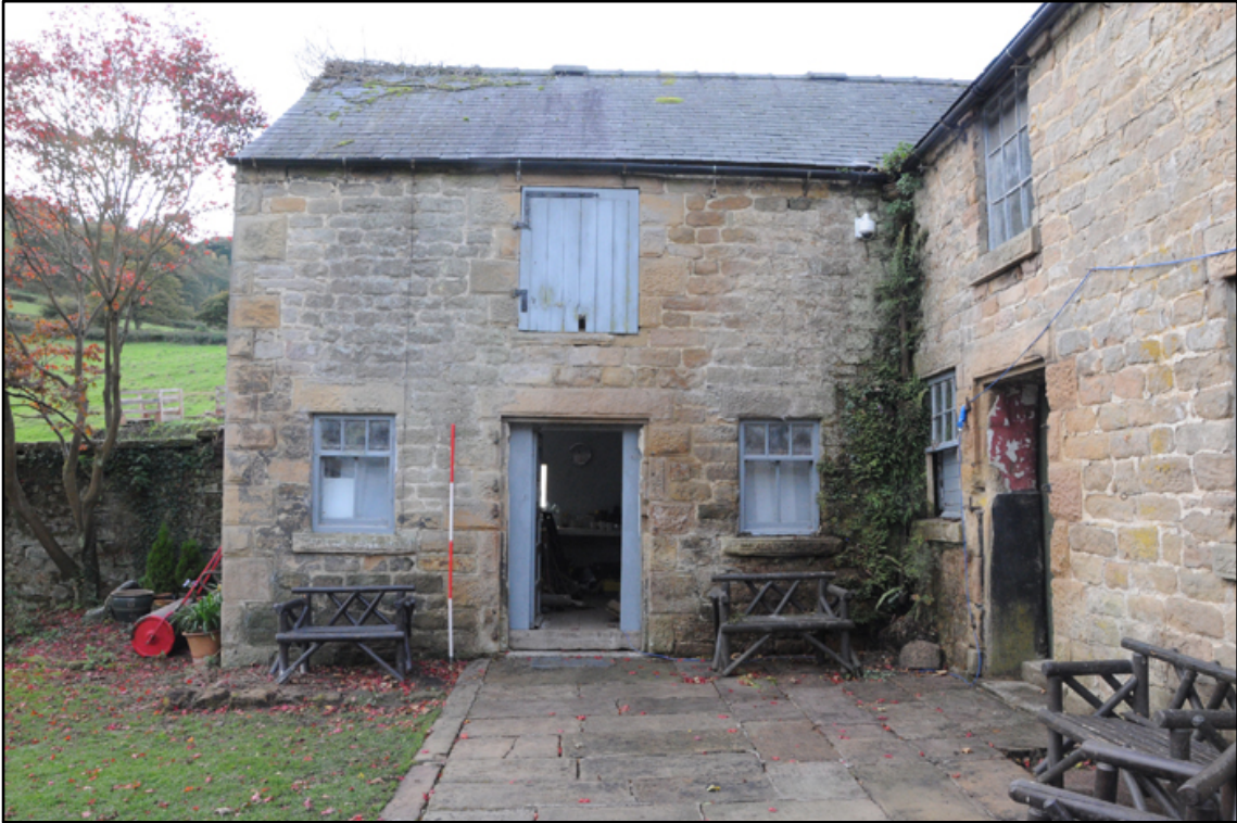
Appendix 5.70: General view of north elevation of T-shaped barn; note first floor pitching door (2m scale)
