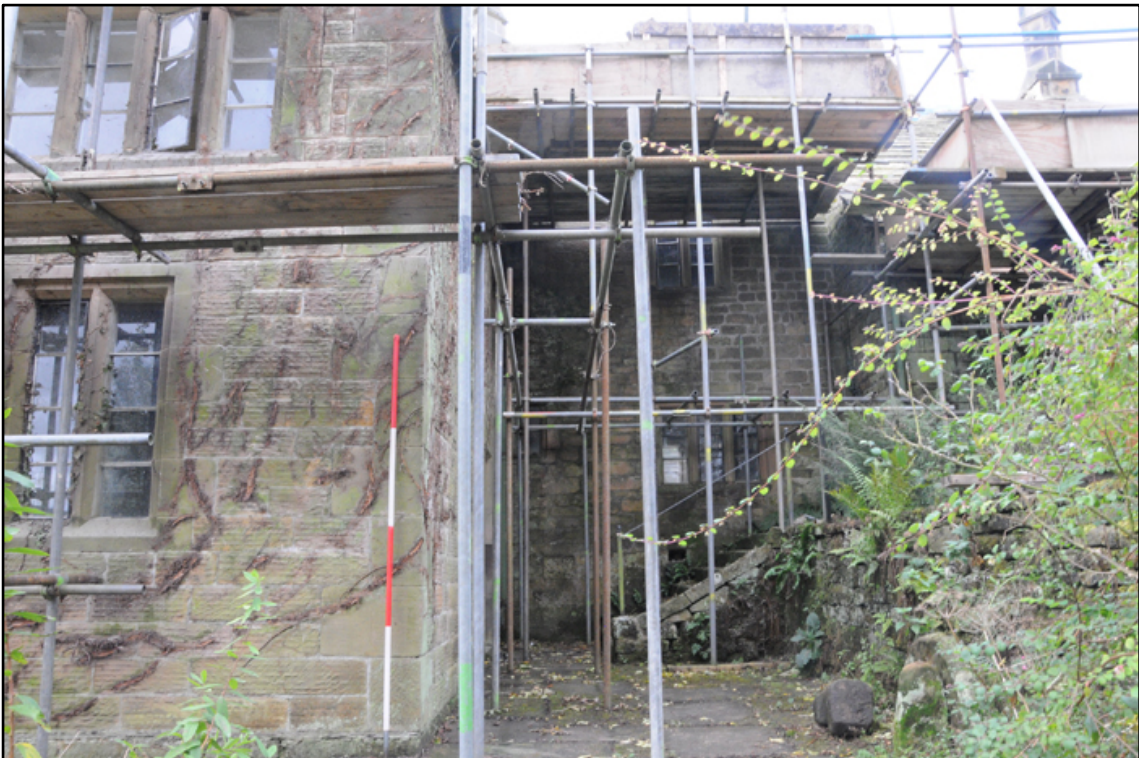
Appendix 5.13: Detail of northwest corner of northern extension (phase 6), looking south (2m scale)
