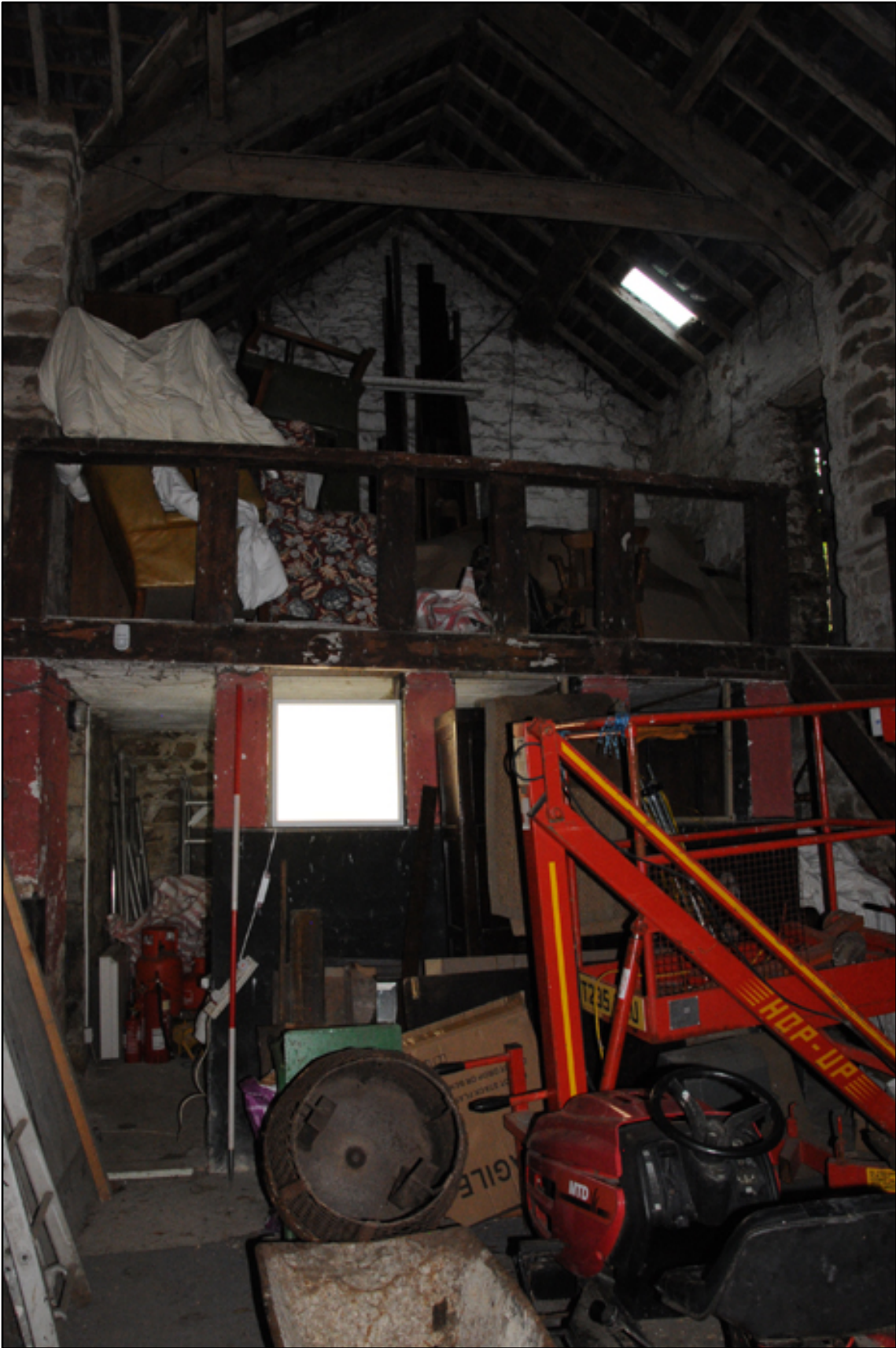
Appendix 5.74: General view of south end of T-shaped barn; note inserted concrete floor for upper level (2m scale)
