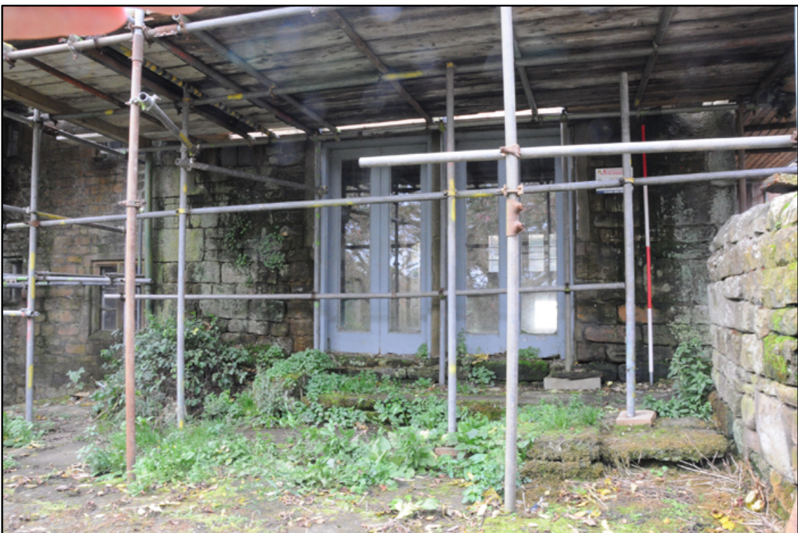
Appendix 5.15: General view of inserted doors (phase 9) in north wall of G3, looking south (2m scale)
