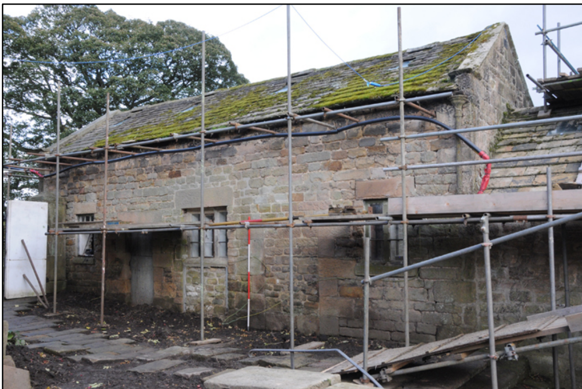
Appendix 5.59: General view of south elevation of G4; note blocked doorway and inserted opening (2m scale)
