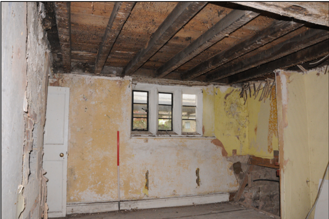
Appendix 5.43: General view of south wall of FI; note inserted wall (phase 9) to right (1m scale)
