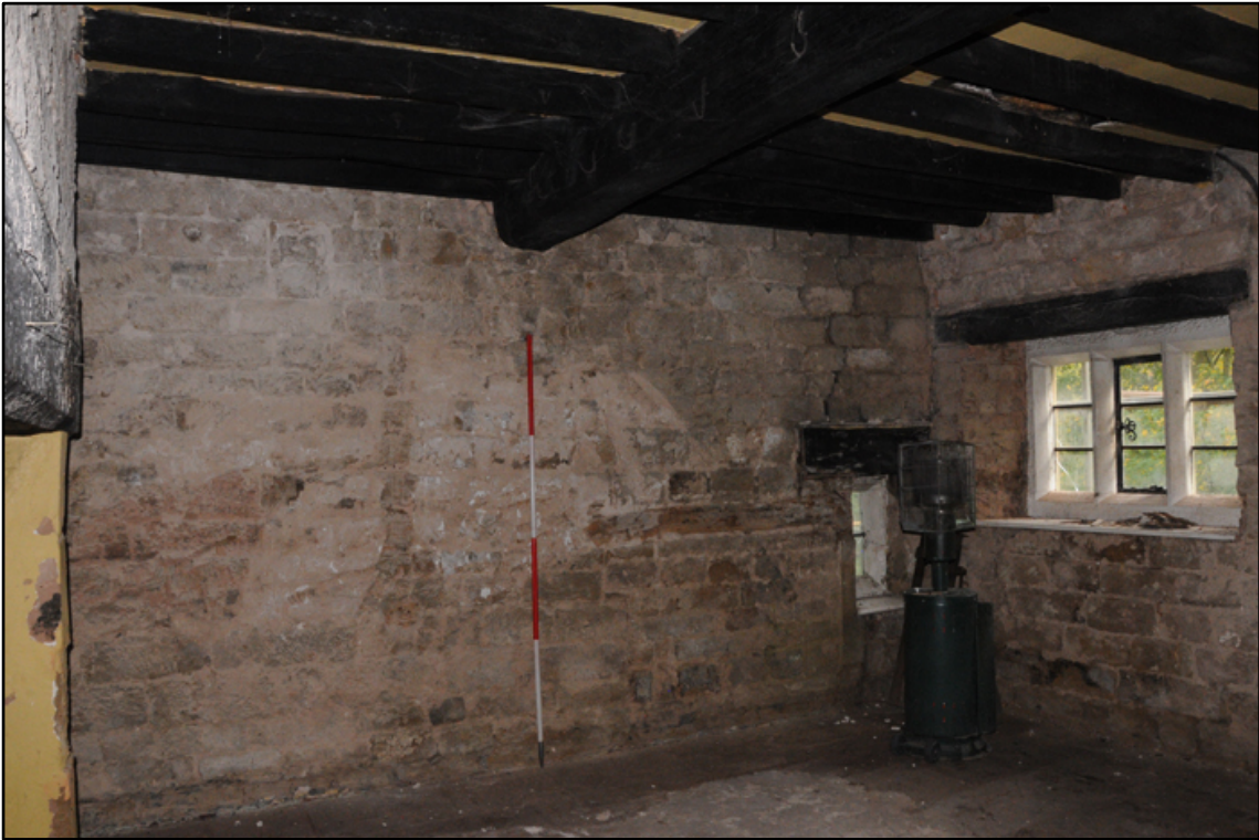
Appendix 5.22: General view of north wall of G2; note blocked opening (phase 7) and narrow window (2m scale)
