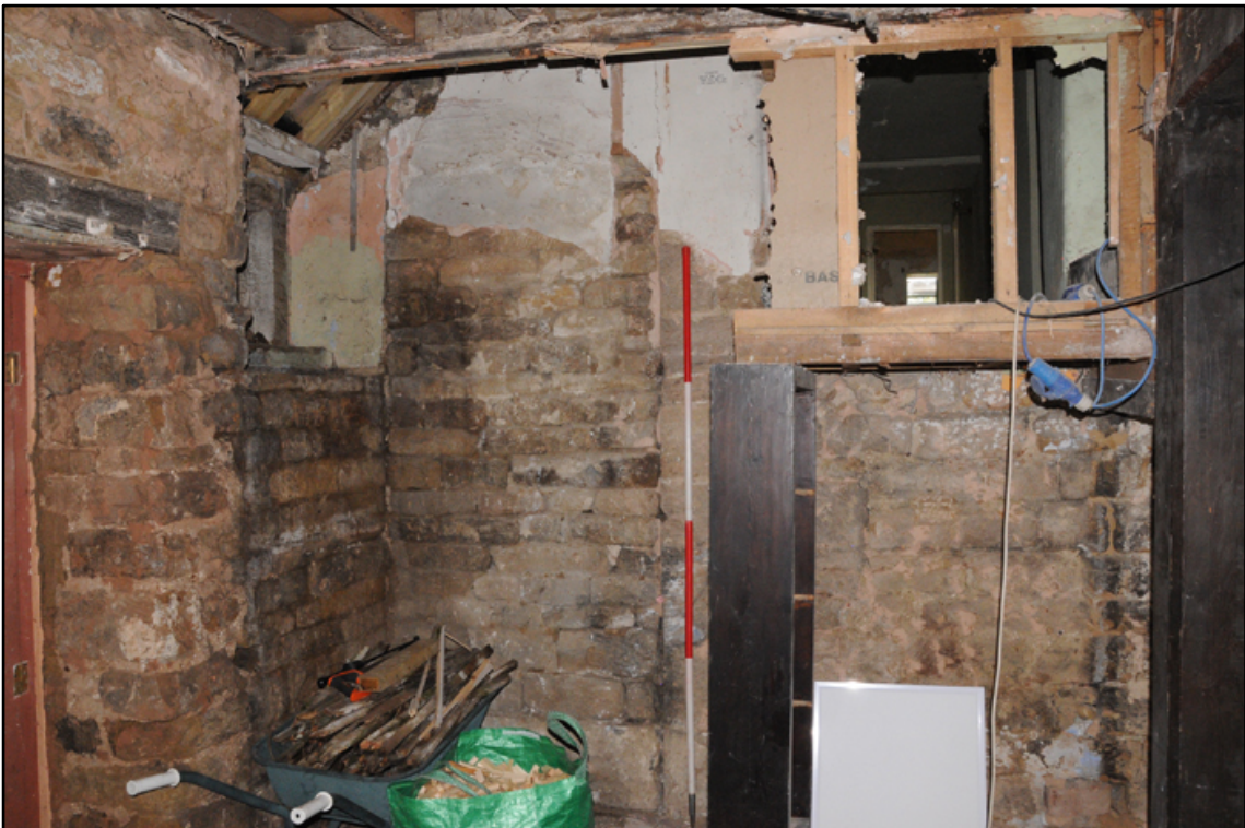
Appendix 5.31: Detail of vertical construction break in northeast corner of G3 ; note remains if winder stair (2m scale)
