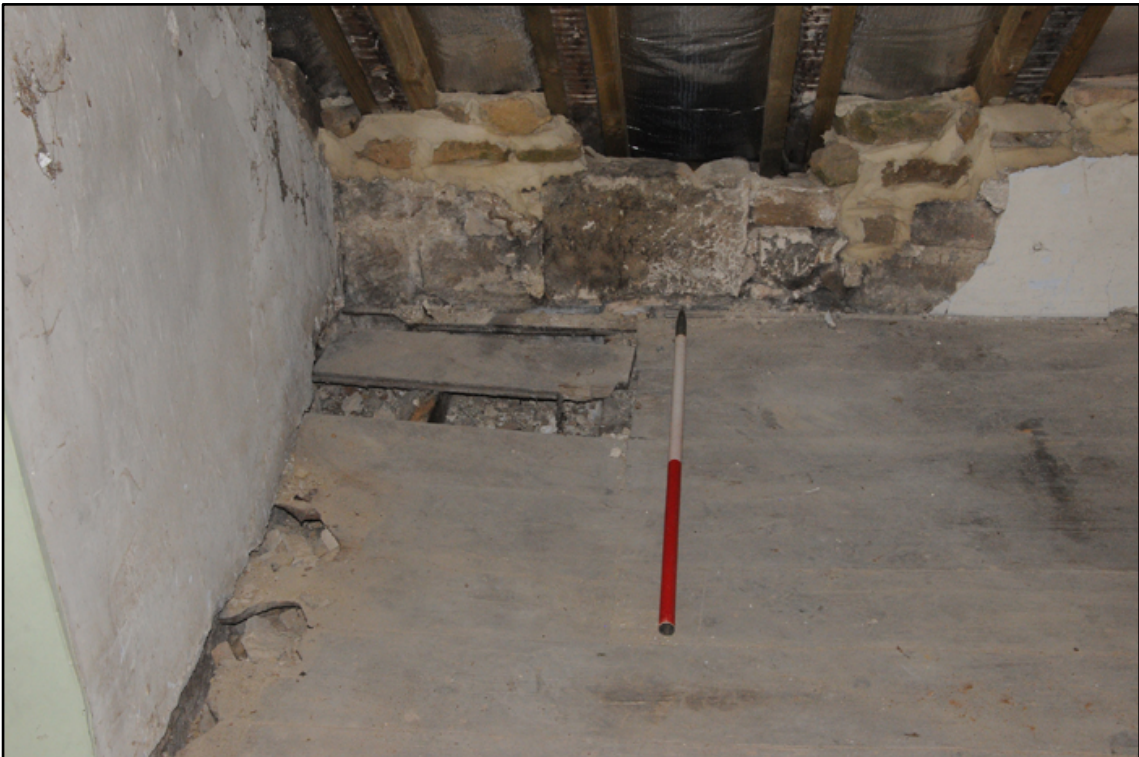
Appendix 5.51: Detail of floor scar in northwest corner of SI; possible access hatch for ladder stair (1m scale)
