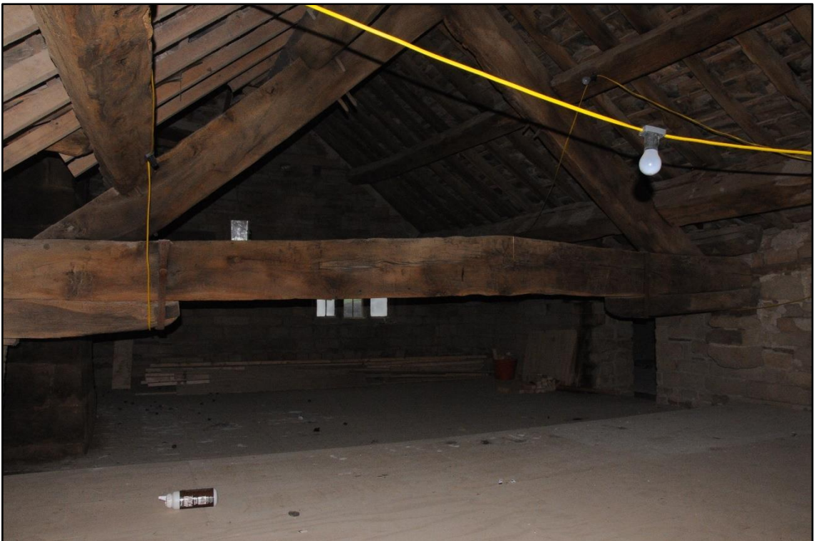
Appendix 2.10: View of truss in the eastern bay of Woodseats Farmhouse (Building 1)
