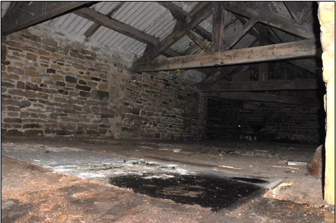
Appendix 2.14: View of first floor of northeast-southwest range of Building 2, looking south
