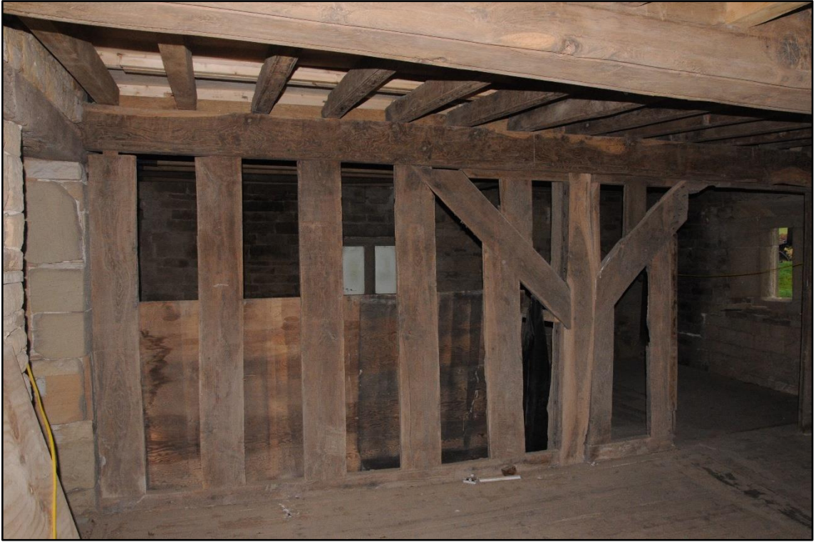
Appendix 2.9: View of timber screen between chambers on first floor of Woodseats Farmhouse (Building 1)
