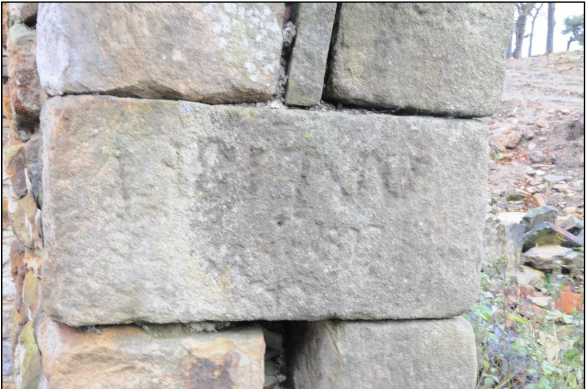
Appendix 2.16: Detail of inscription on door reveal of Building 3 (possible date of 1877)
