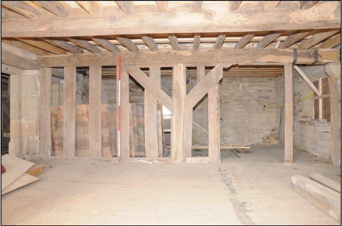
Appendix 2.33: Timber partition wall between F1 and F2, looking northwest (2m scale)
