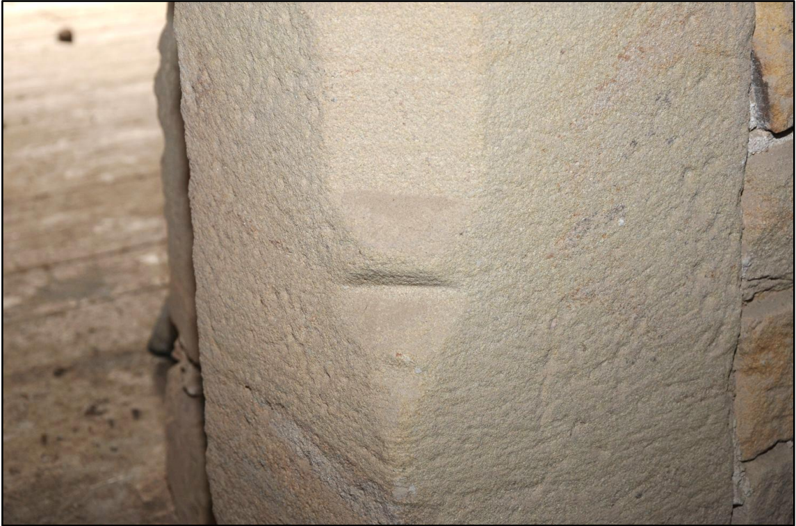
Appendix 2.29: Detail of stop to chamfer on surround to doorway between F3 and F4 , looking south
