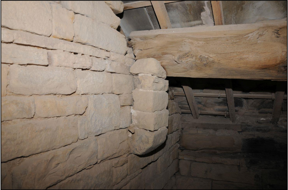
Appendix 2.41: Detail of added corbel supporting purlin on north wall of SI, looking northeast
