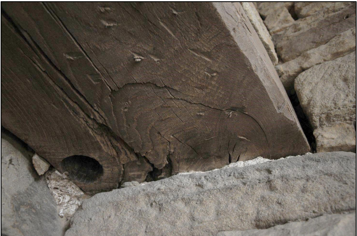
Appendix 2.20: Detail lintel with hinge socket to doorway between G3 and G4, looking north
