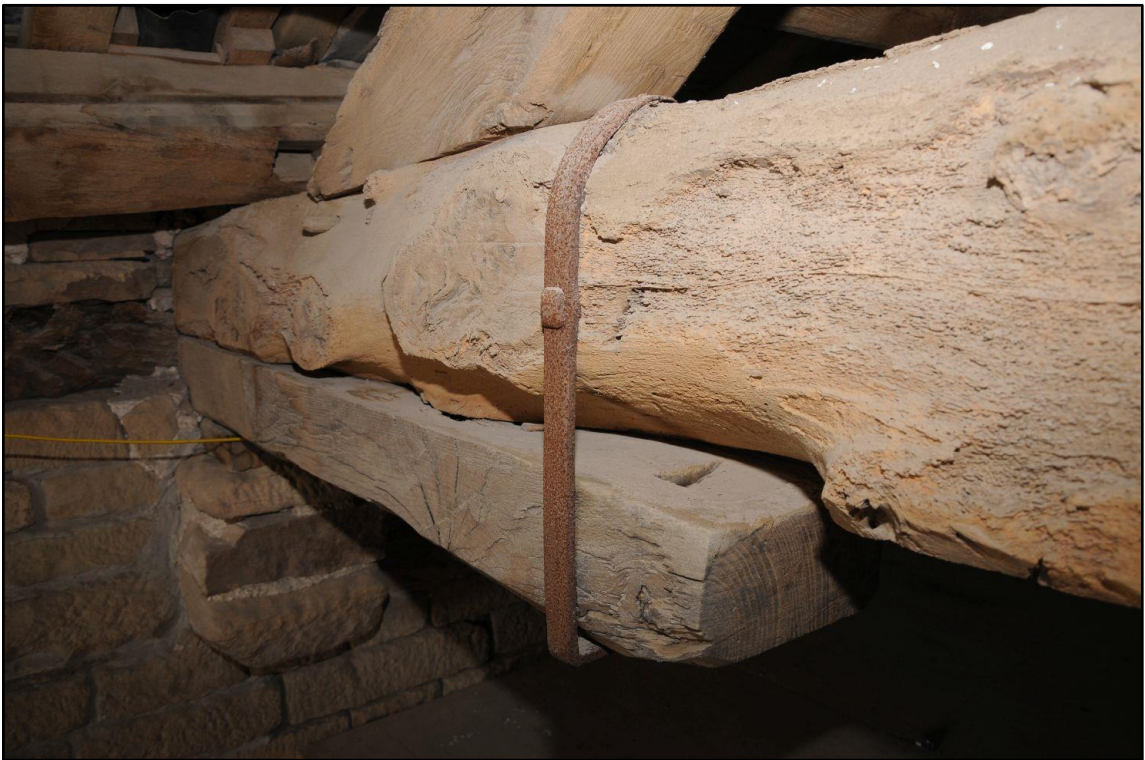
Appendix 2.40: Detail of strap and support to truss in SI, looking west
