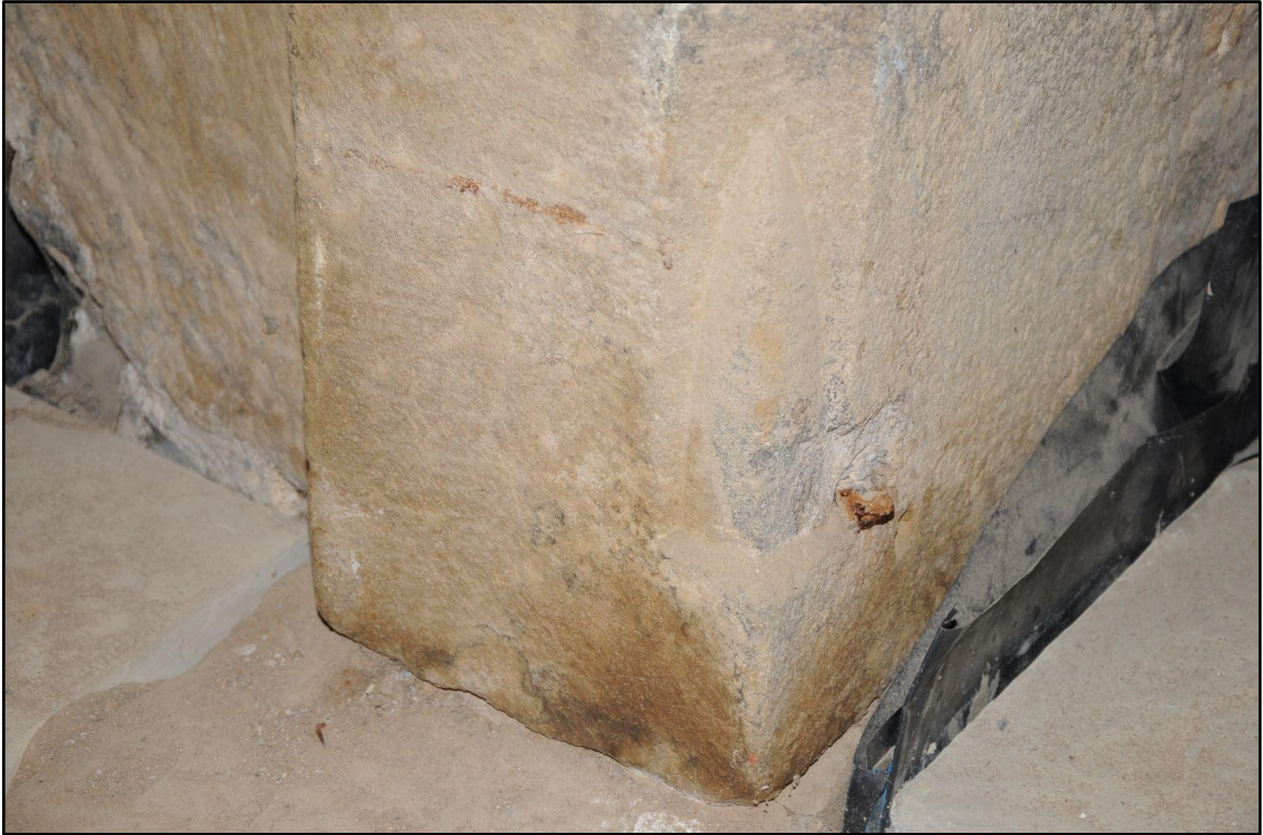
Appendix 2.19: Detail of chamfered stop to doorway between G3 and G4, looking south
