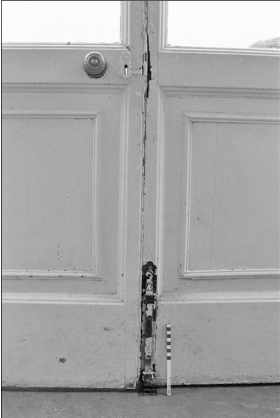
Appendix I.13: Detail of door furniture on inner face of external doors to Porch (20cm scale). Film I.19.
