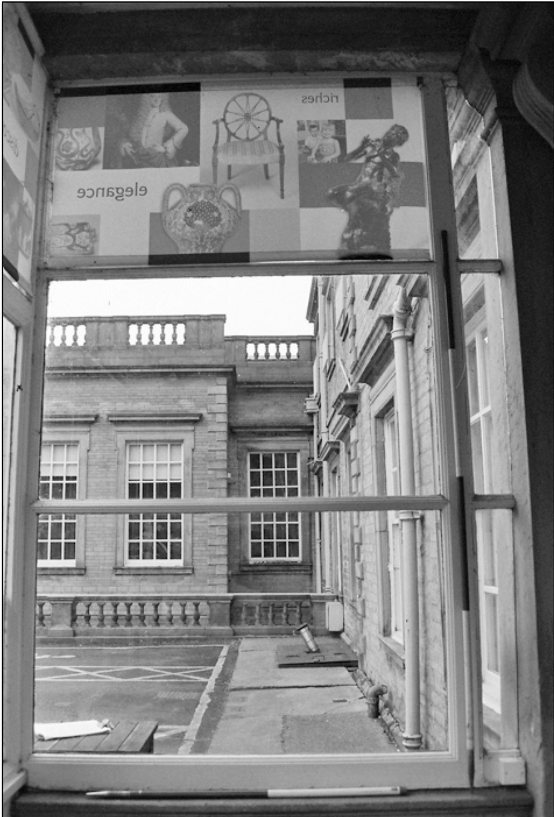
Appendix I.16: Internal view of east elevation and glazing (1m/2m scale). Film I.22.
