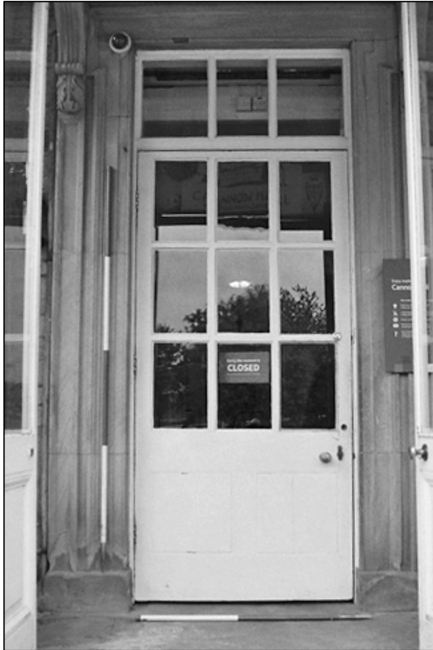
Appendix I.8: Detail of inner door into Hall (1m/2m scale). Film I.18.
