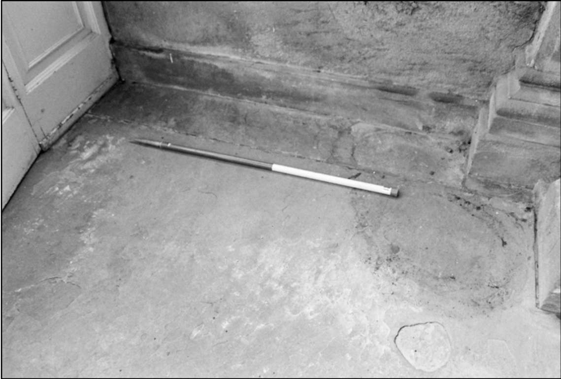
Appendix I.24: Detail of southwest floor of Porch (1m scale). Film I.29
