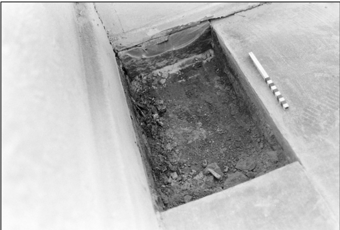
Appendix I.23: Detail of excavated trial hole I, following removal of slab (20cm scale). Film I.34
