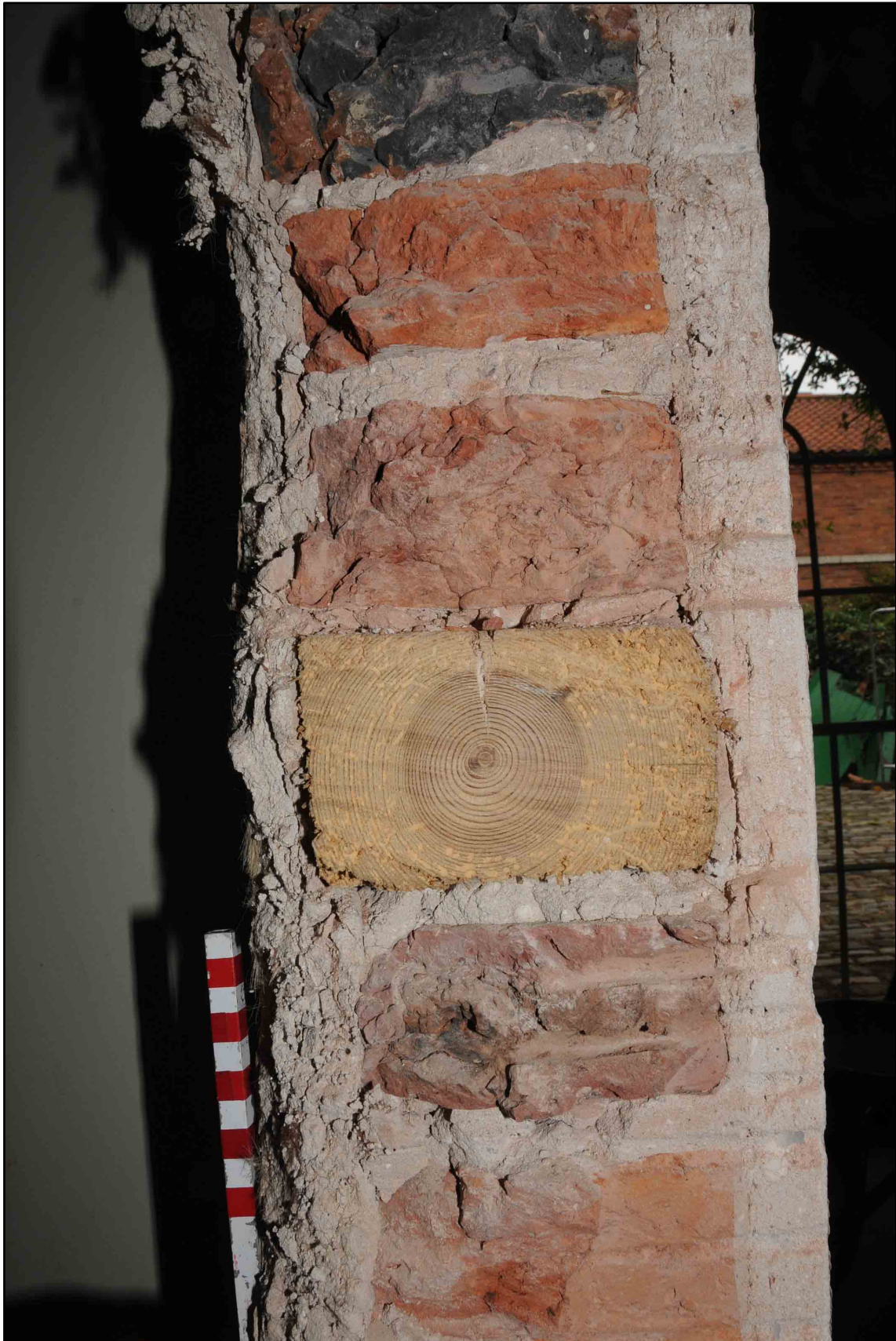
Appendix I.16: Detail of inset timber in wall between G2 and G7 ; note single brick thick (10cm scale).
