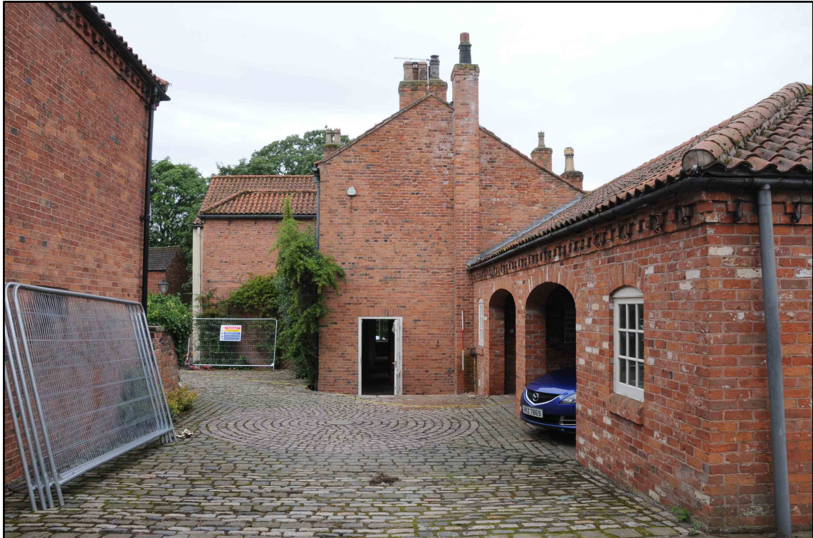
Appendix I.3: General view of rear of property, looking south-west (2m scale).
