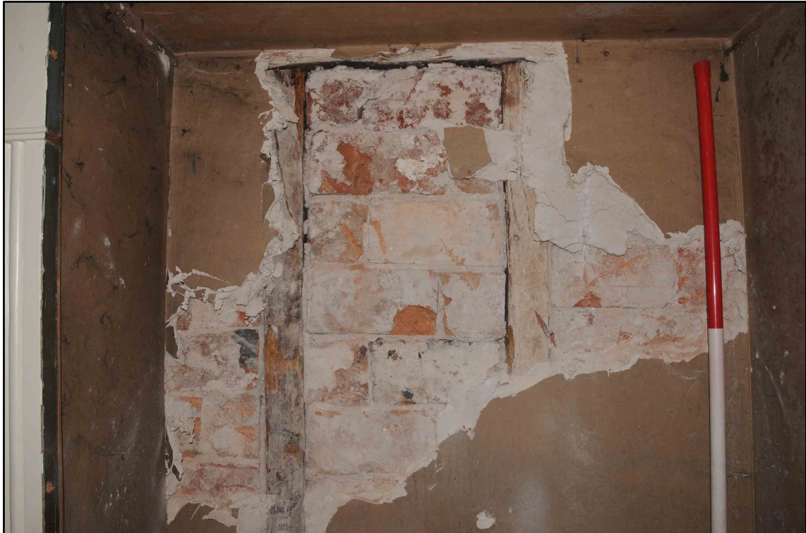
Appendix I.11: Detail of exposed timber studs and brick fill in cupboard in G2 (0.5m scale).
