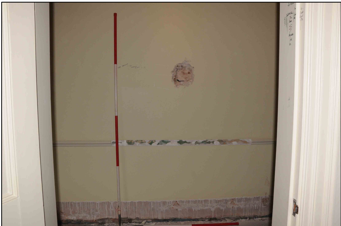
Appendix I.10: General view of south wall of corridor G5 (1m/2m scale).
