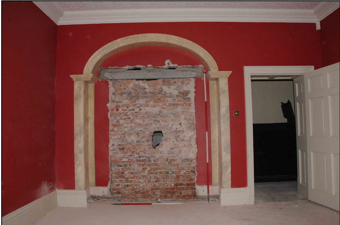
Appendix I.5: Detail of north wall of G3 with plaster removed (1 m/2m scale).
