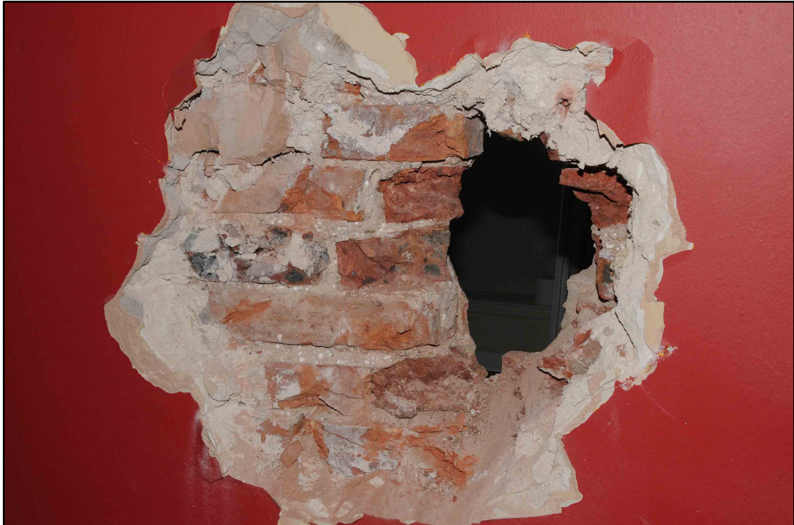
Appendix I.7: Detail of brick wall between G3 and G4 ; note single brick thickness.
