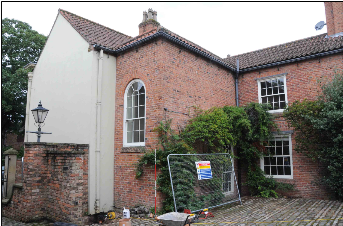
Appendix I.4: General view of exterior of staircase with round headed window (2m scale).
