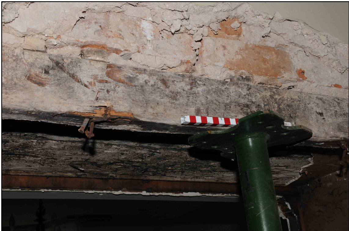
Appendix I.12: Detail of re-used timber forming lintel in south wall of corridor G5 (10cm scale).
