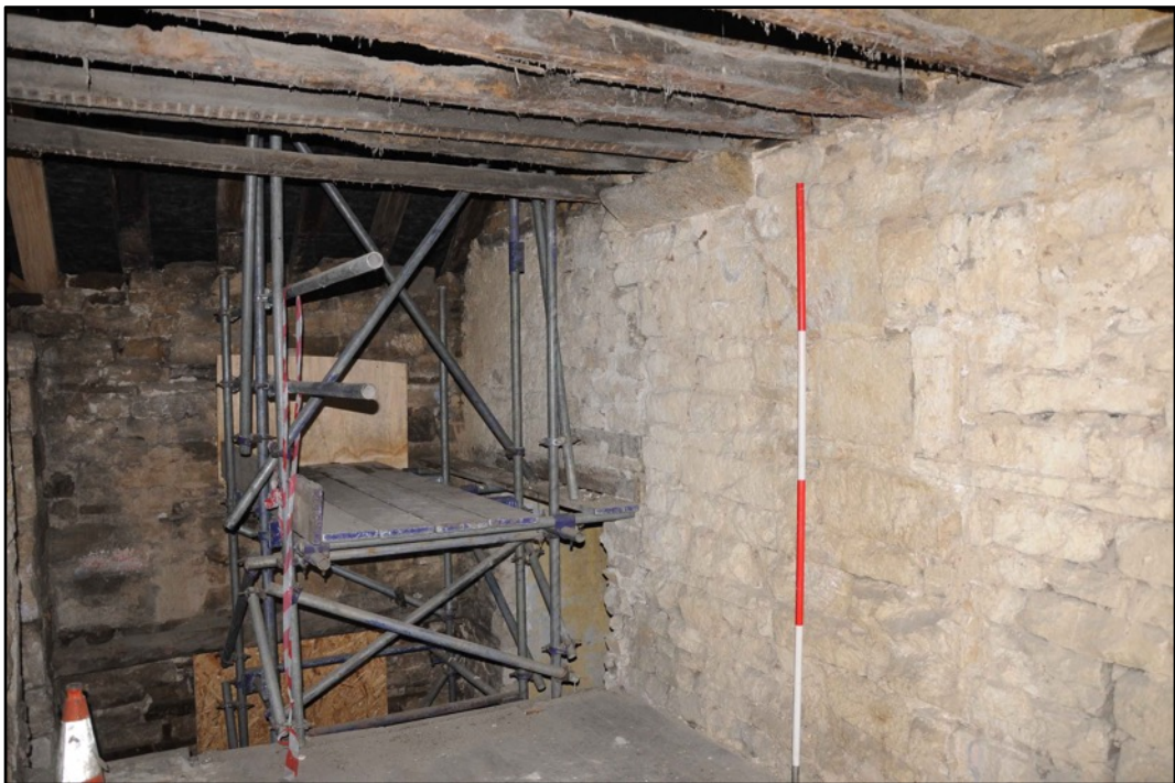
Appendix 2.44: General view of F3 looking north; note alterations to righthand wall (2m scale)
