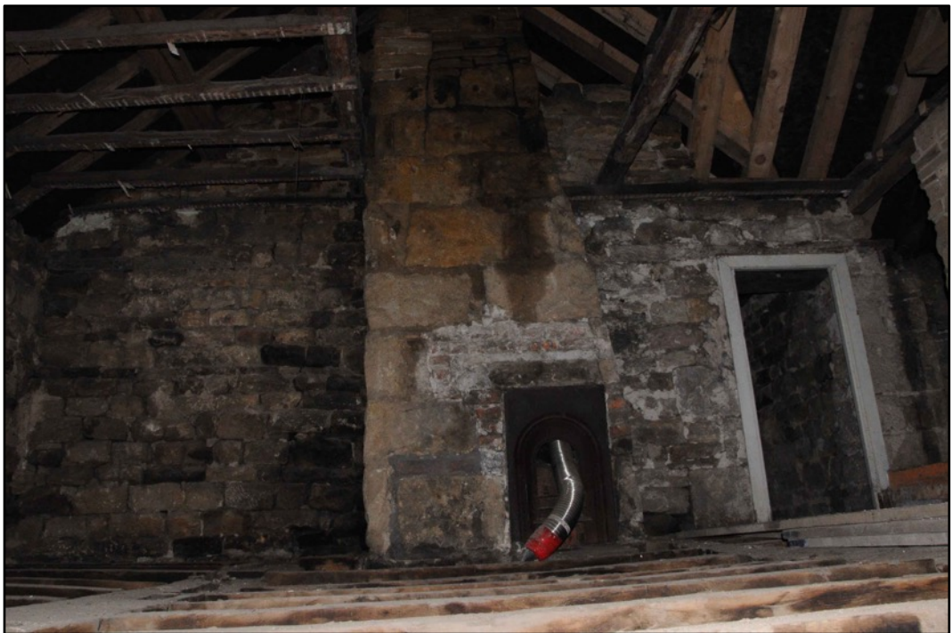
Appendix 2.36: General view of F1, looking north (no access taken from floor below)
