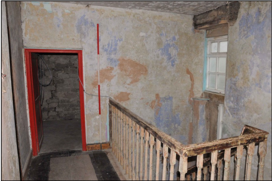
Appendix 2.21: General view of landing F7, looking west; note inserted wall (2m scale)
