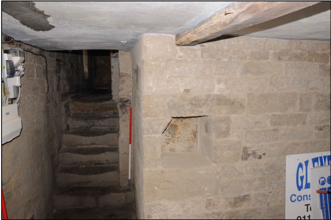
Appendix 2.37: Detail of steps down to CI, looking northwest; note stone cupboard (1m scale)
