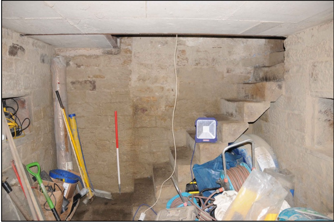
Appendix 2.39: View of north wall of C2; note blocked lightwell (1m scale)
