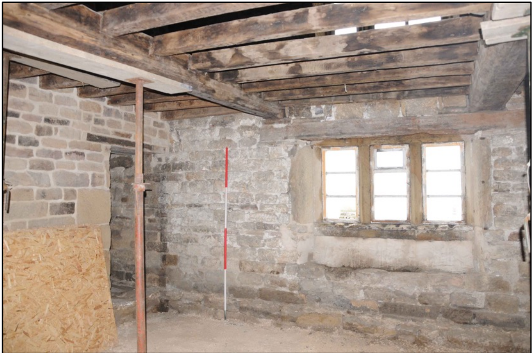
Appendix 2.34: View of south wall of G1; note recess below window (2m scale)
