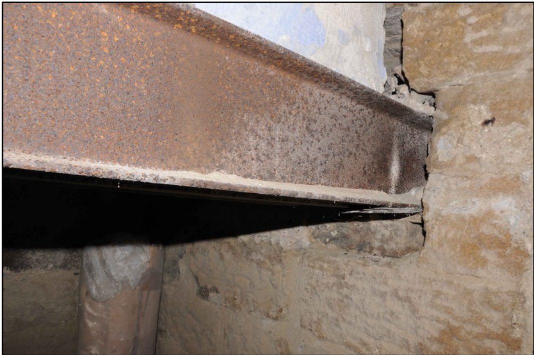
Appendix 2.40: Detail of inserted RJC and slate packing in C2, looking north
