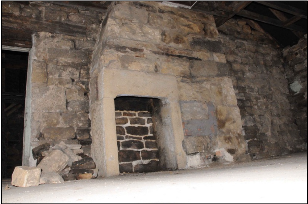
Appendix 2.35: General view of F2, looking south (no access taken from floor below)
