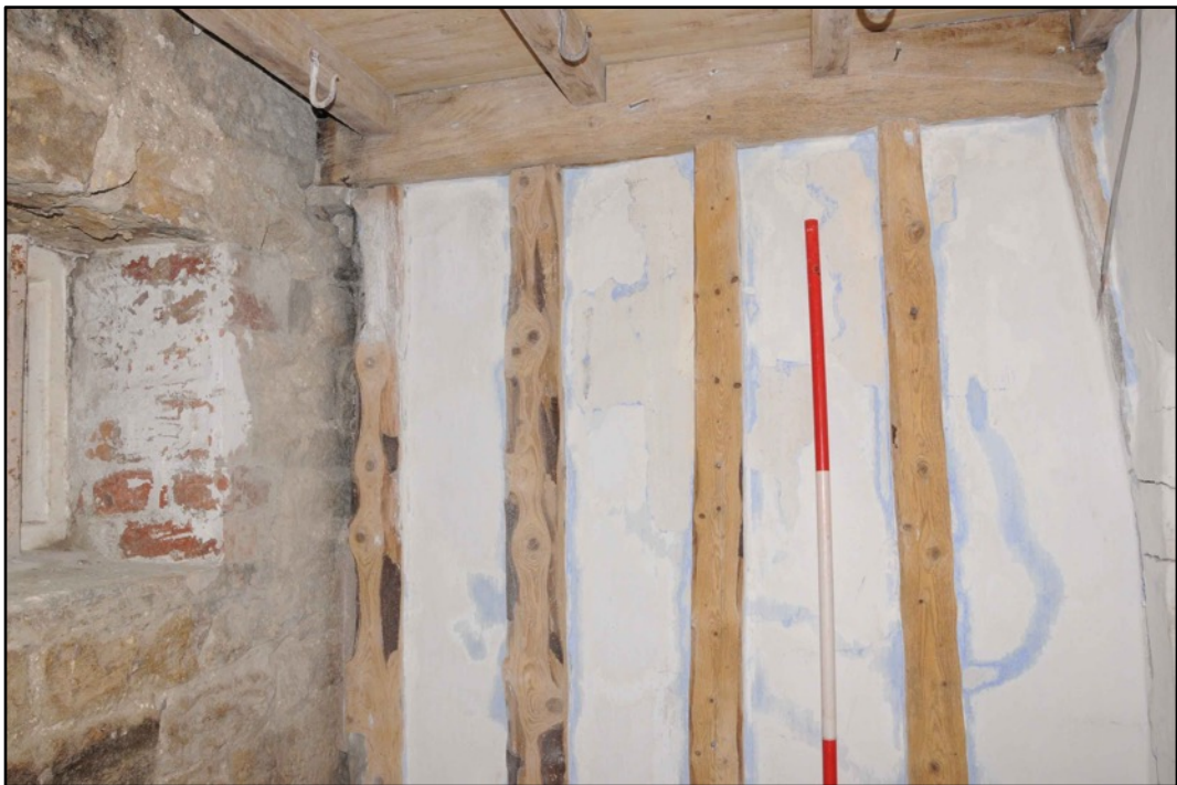
Appendix 2.20: Detail of inserted wall in G7, looking east (0.5m scale divisions)
