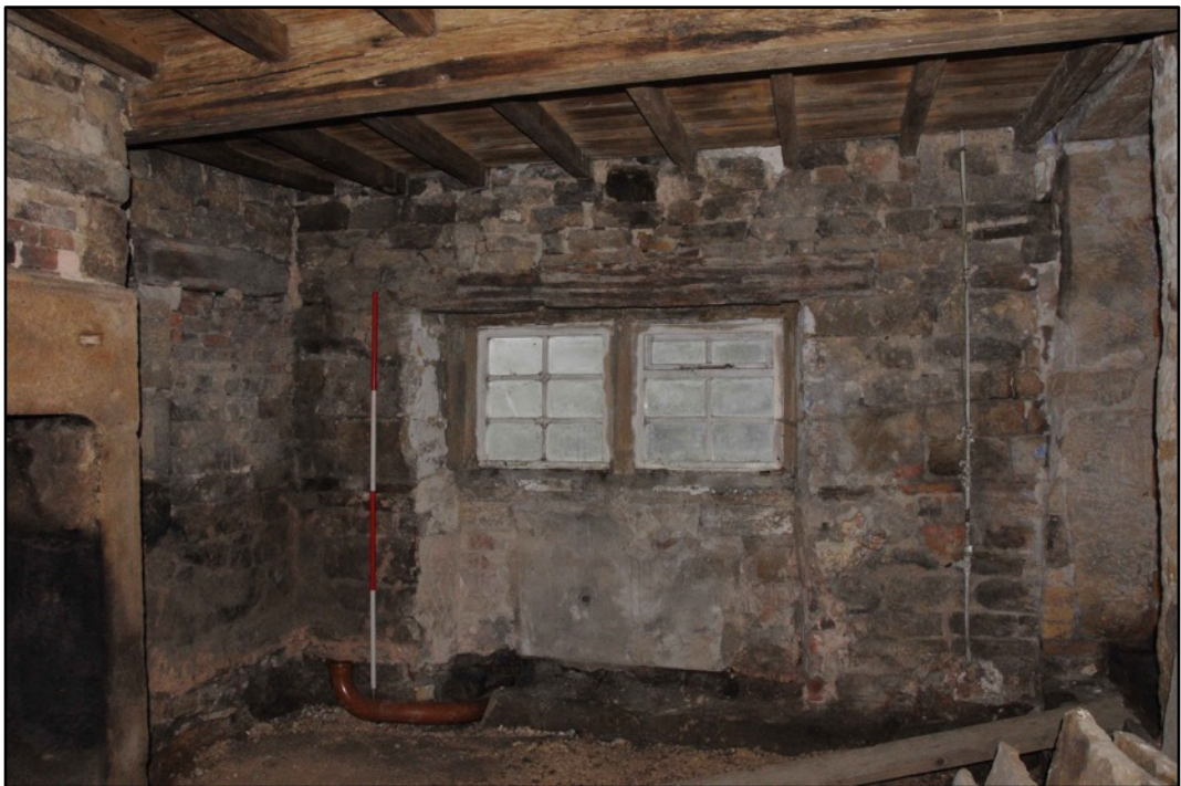
Appendix 2.28: View of west wall of G2; note recess created under window for sink (2m scale)
