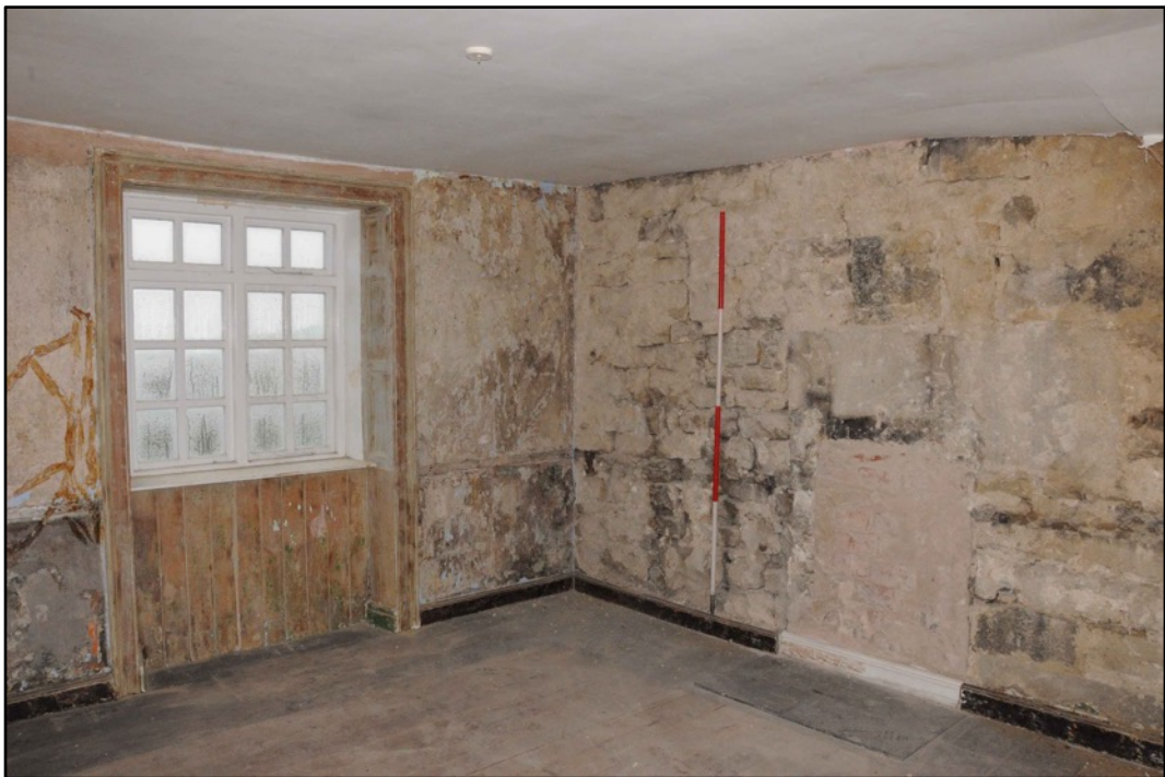
Appendix 2.24: General view of F4, looking southwest; note blocked fireplace (2m scale)
