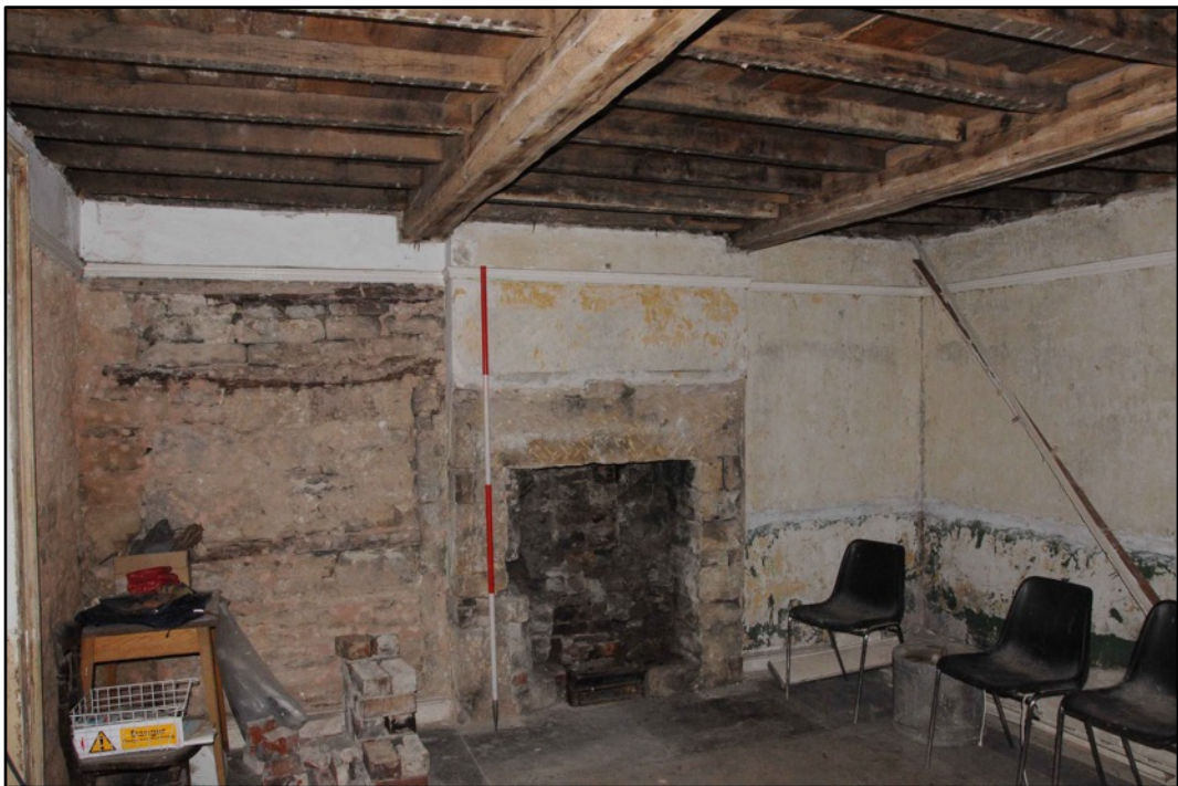
Appendix 2.18: General view of G5, looking west; note blocking on left of fireplace (2m scale)
