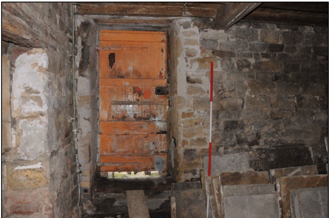
Appendix 2.30: Detail of inserted doorway in northwest corner of G2 (2m scale)
