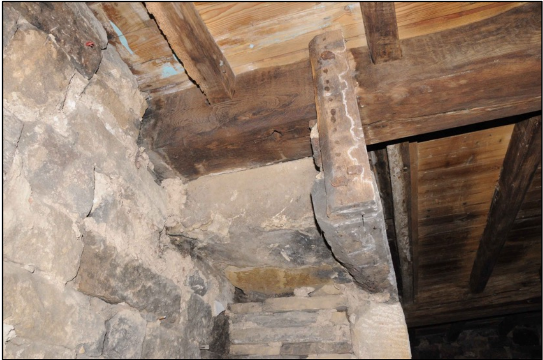
Appendix 2.29: Detail of chamfered beam on east side of fireplace in G2; note alterations
