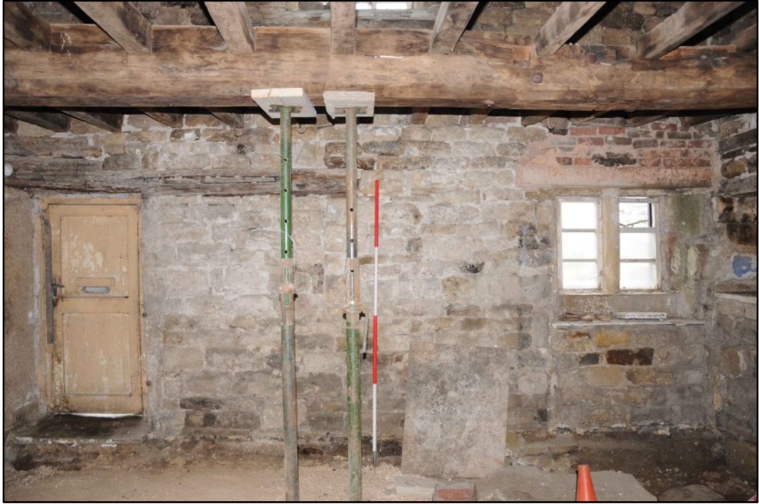
Appendix 2.33: View of west wall of G1; note blocked window and door (2m scale)
