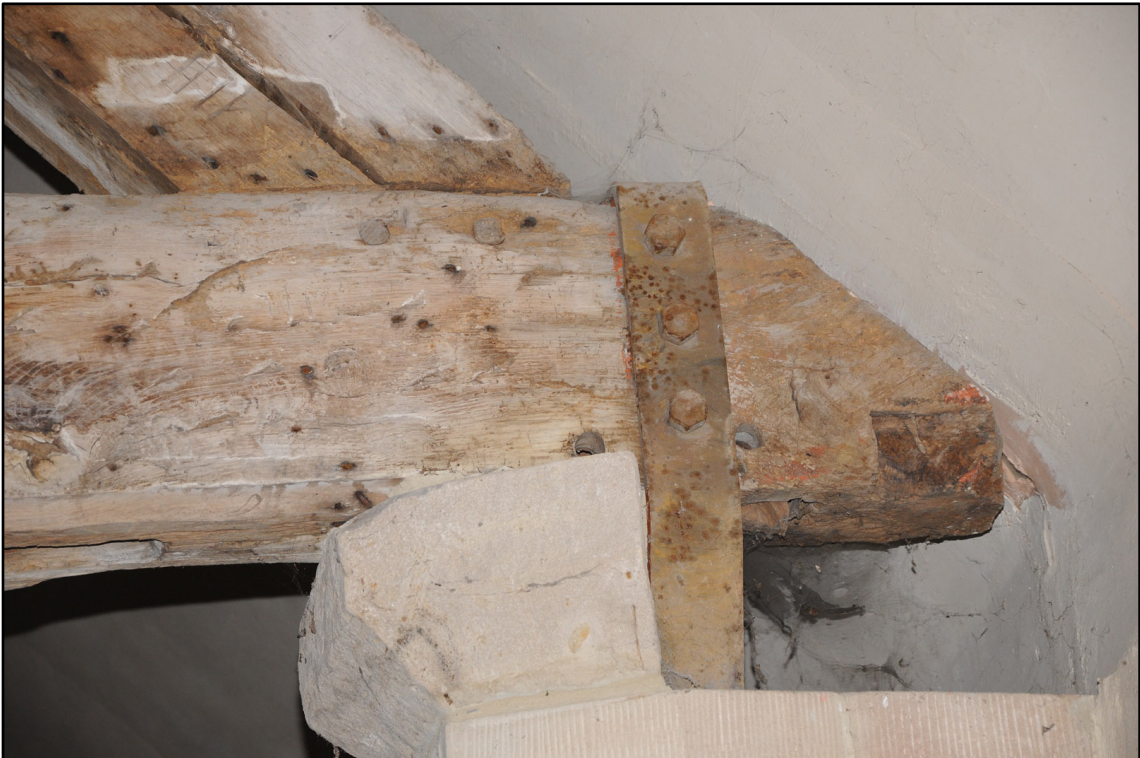
Appendix 5.139: Detail of end of tiebeam in F13 ; note mortise for post ( Photo 163 )
