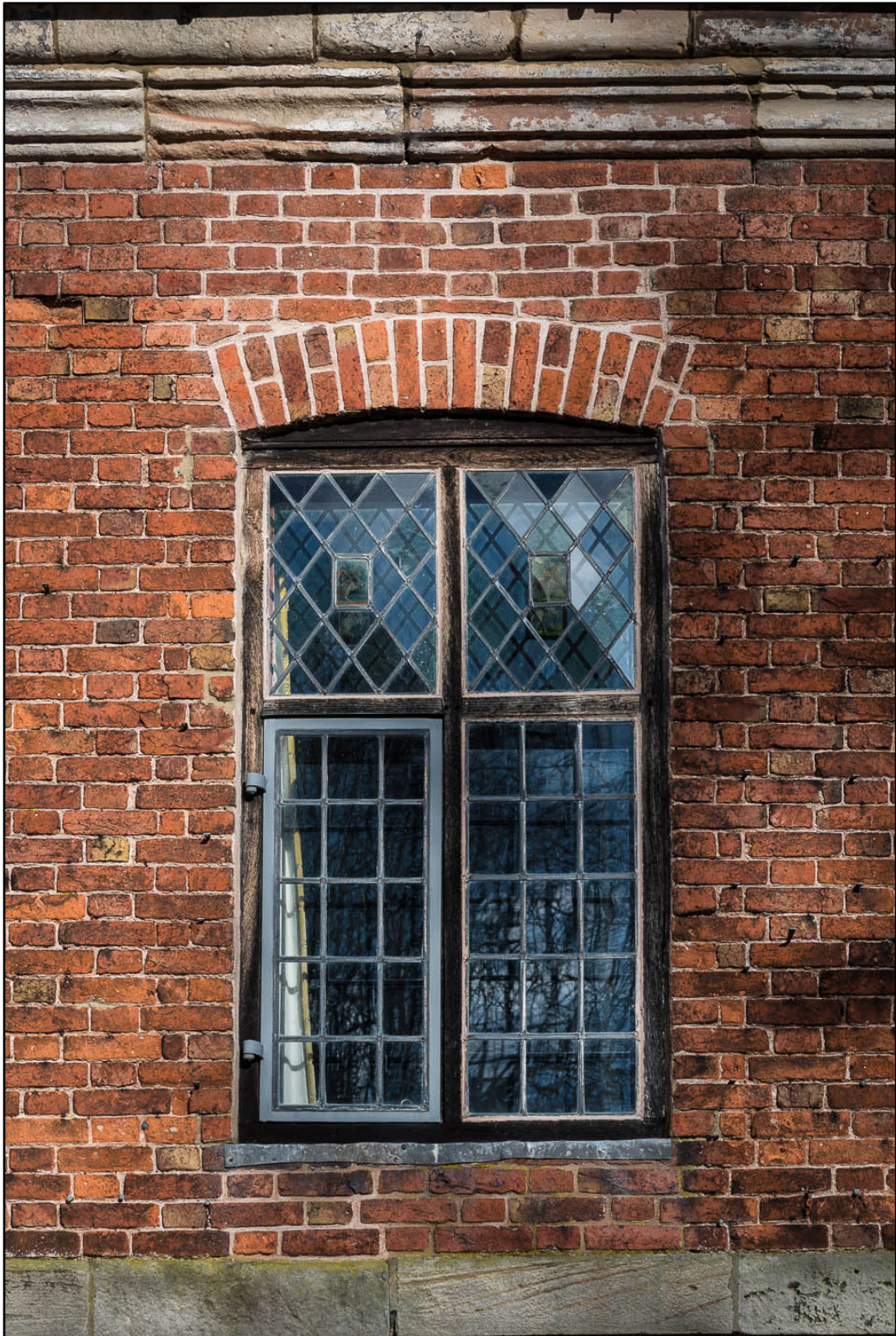
Appendix 5.19: Detail of restored 1 st floor window in façade of Building 1 (Photo 32)
