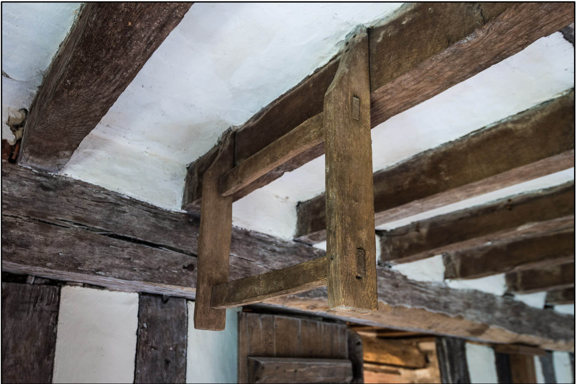
Appendix 5.II0: Detail of ladder hanger attached to ceiling in G10 (Photo 84)
