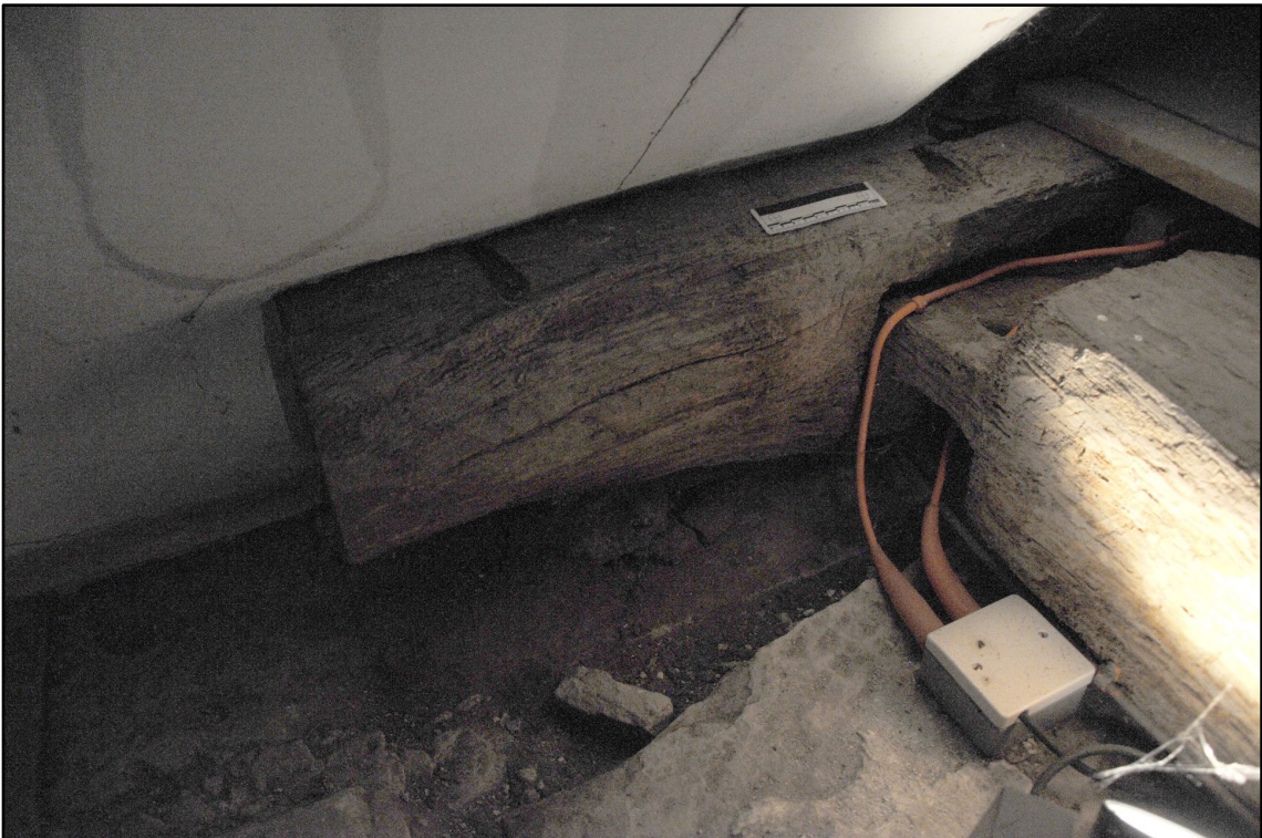
Appendix 5.140: Detail of re-used tiebeam in F13 ; note empty holes (10cm scale) ( Photo 162 )
