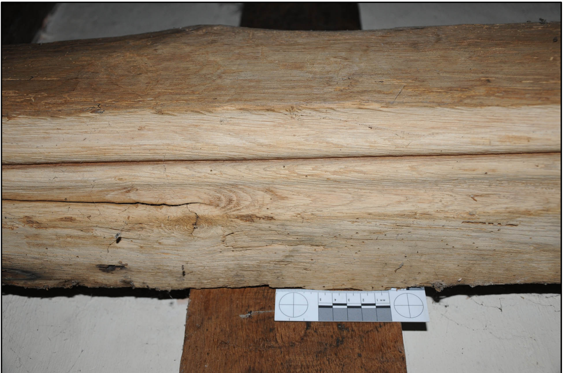
Appendix 5.142: Detail of re-used purlin in southeast roof section in F13 (5cm scale) (Photo 160)
