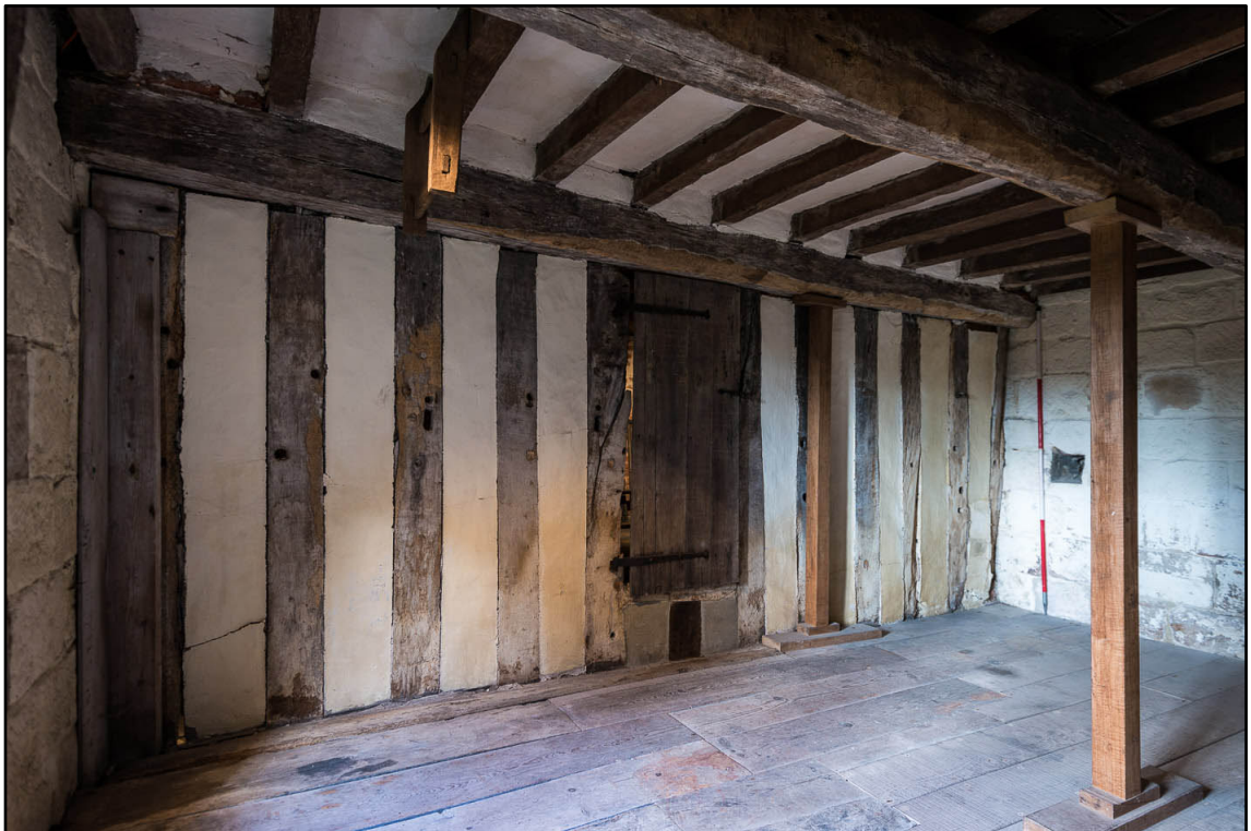
Appendix 5.103: View of studwork partition in G10, looking northeast (2m scale) (Photo 83)
