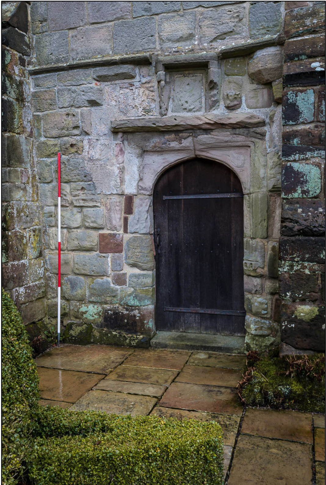
Appendix 5.80: Detail of west doorway into B2 of Building 2 (2m scale) (Photo 23)
