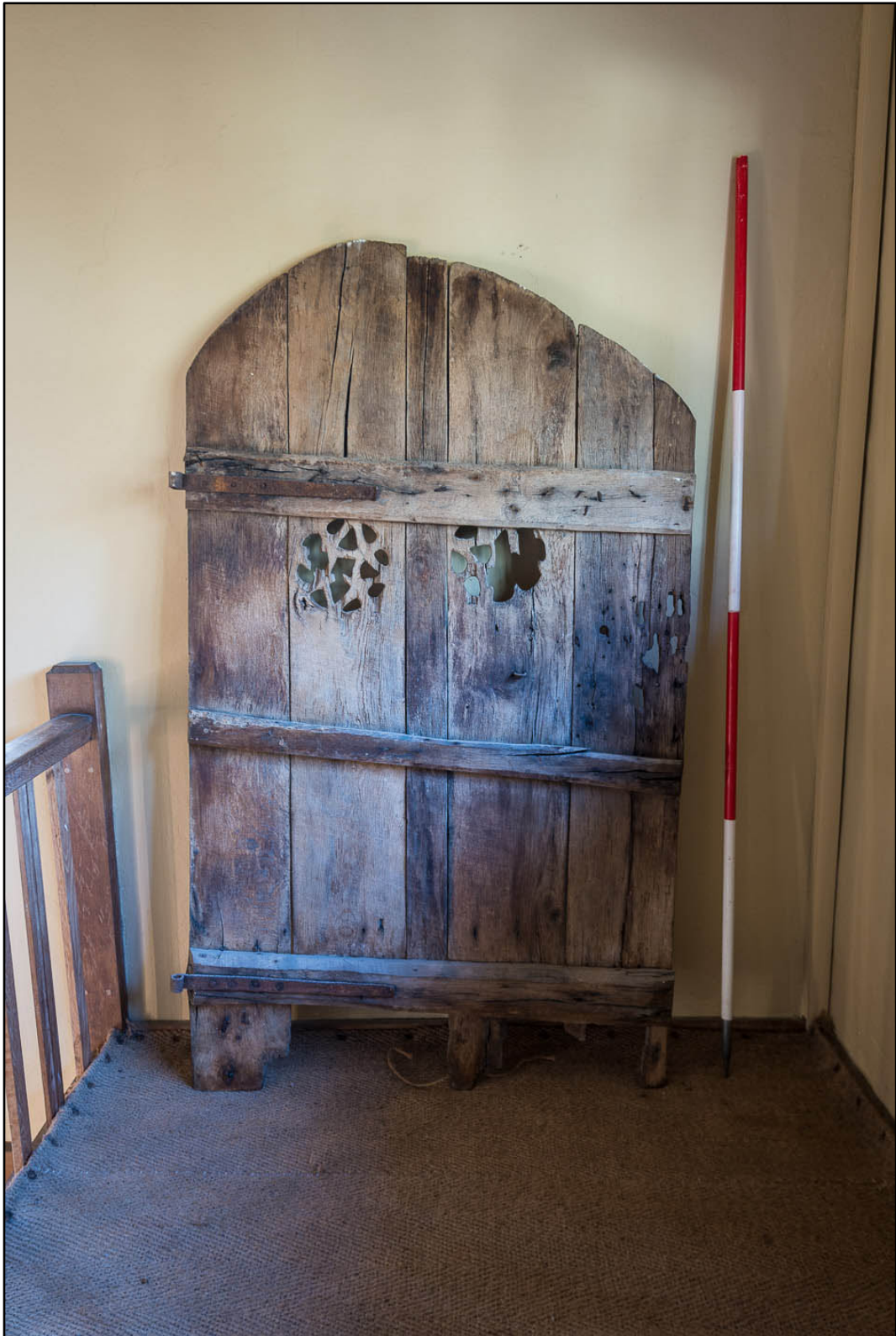
Appendix 5.123: Detail of former door (rear) used in F13 (2m scale) (Photo 55)
