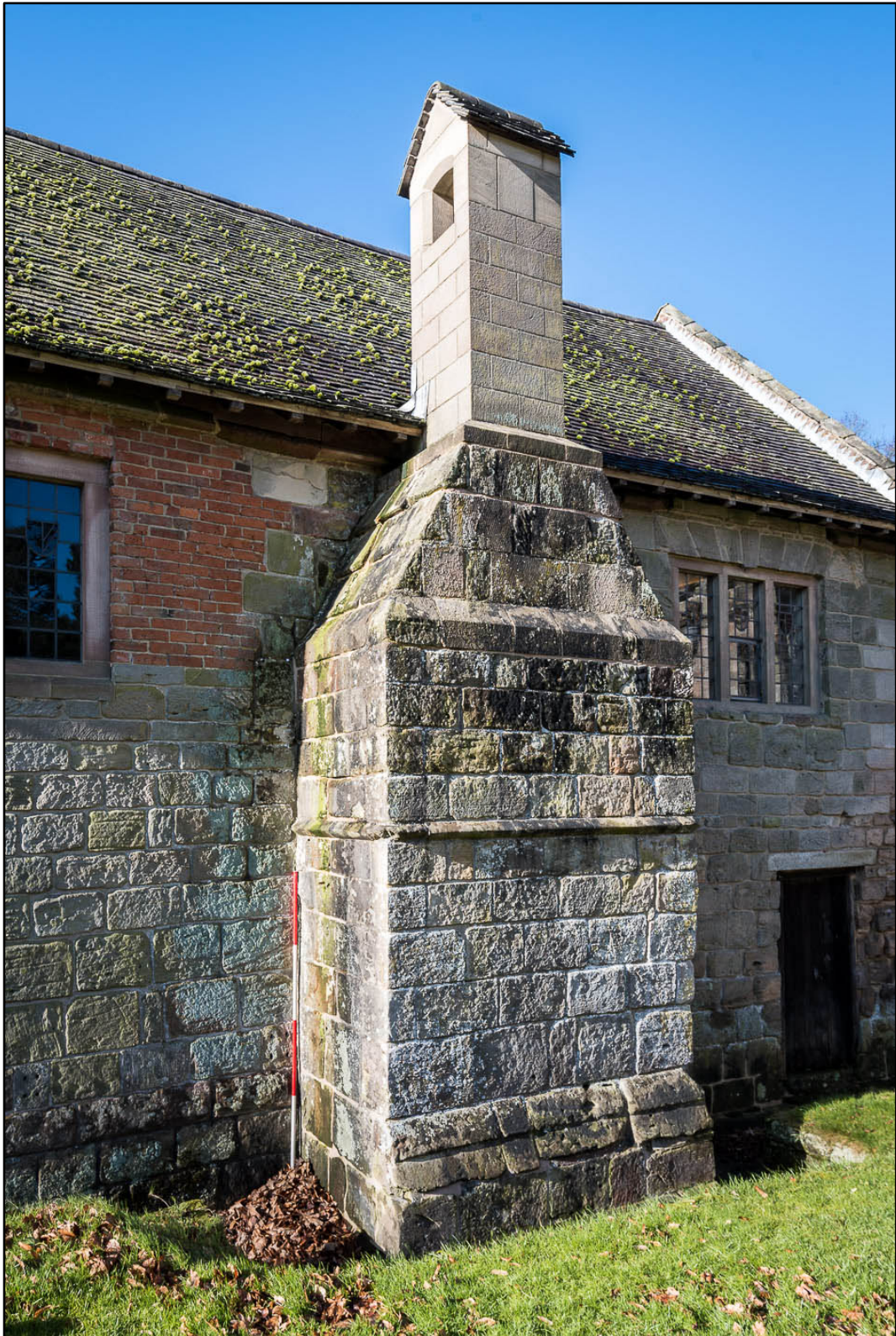
Appendix 5.85: External chimney stack on east elevation of Building 2 (2m scale) (Photo 50)
