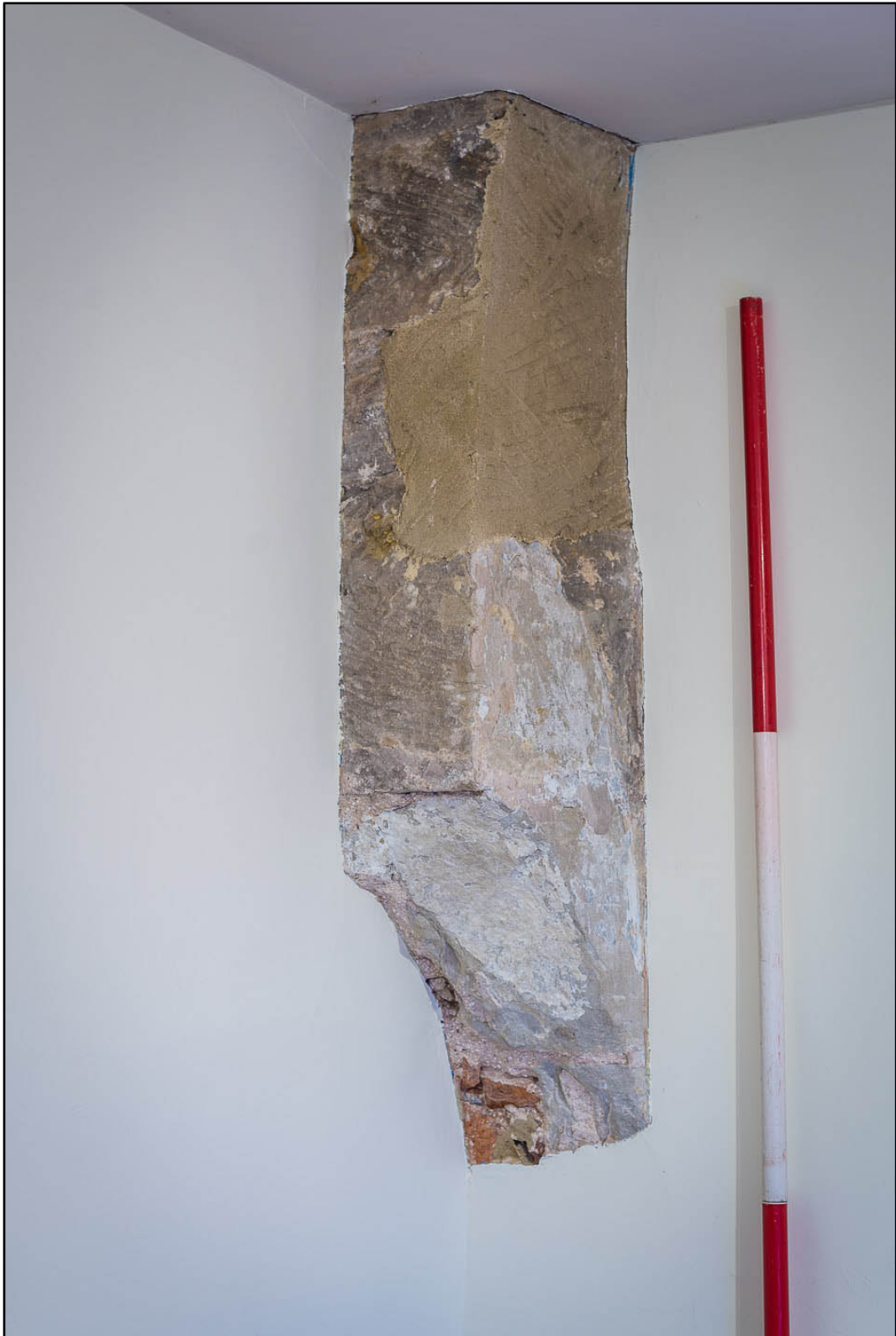
Appendix 5.30: Detail of exposed masonry in southwest corner of kitchen G5 (Photo 149)
