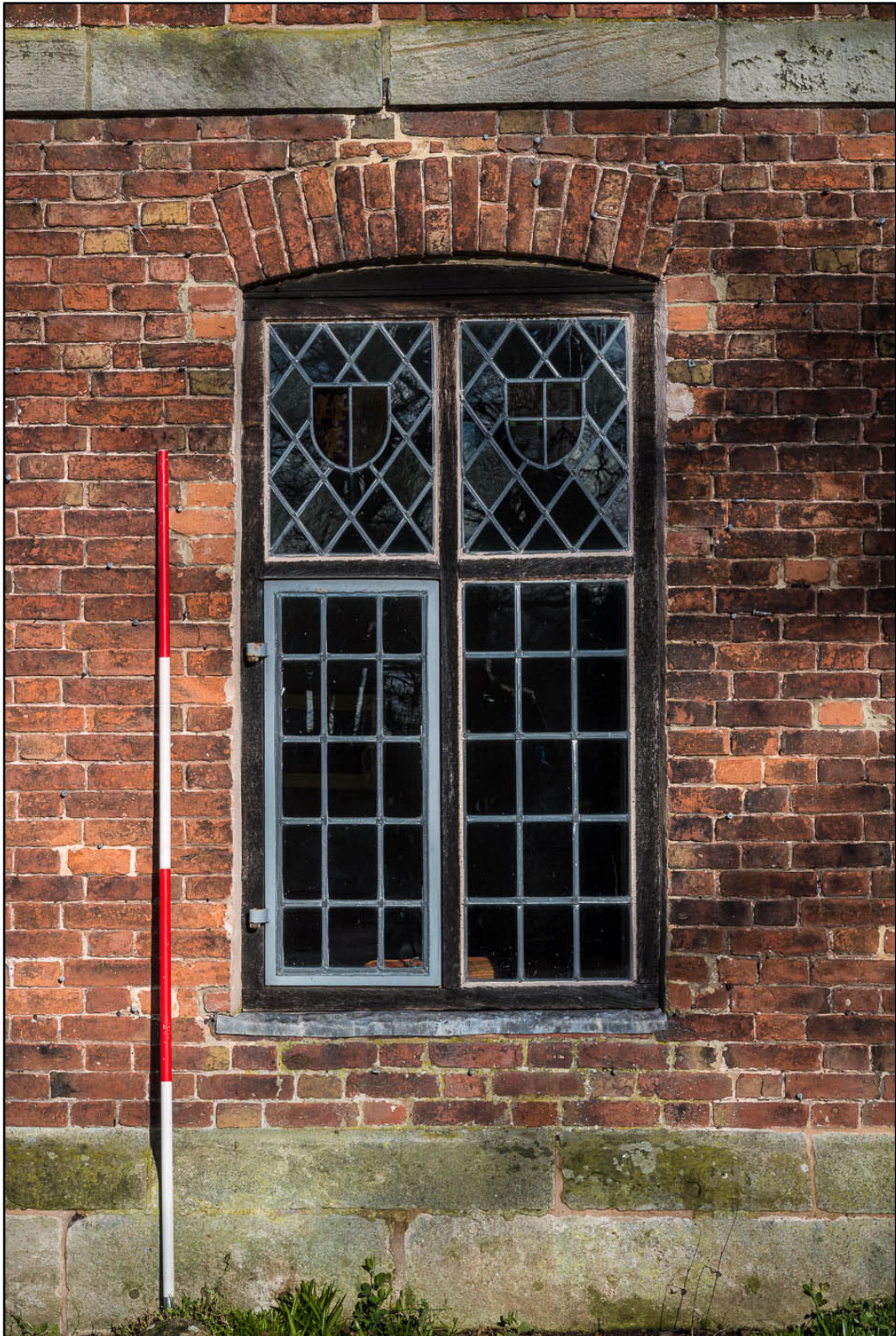
Appendix 5.18: Detail of restored window in façade of Building 1 (2m scale) (Photo 31)
