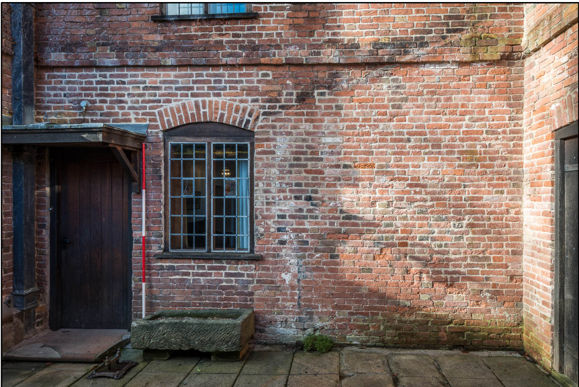
Appendix 5.24: Detail of east elevation of Building 1; note roof scar (2m scale) (Photo 36)
