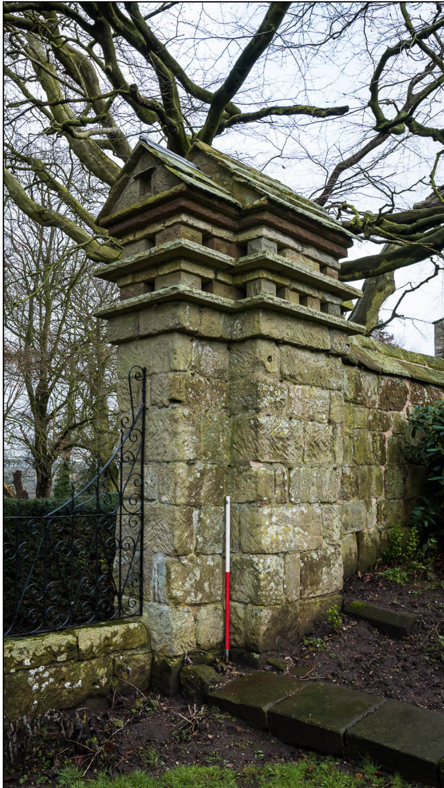
Appendix 5.13: Detail of dovecote in northwest end of garden wall (1m scale) (Photo 15)
