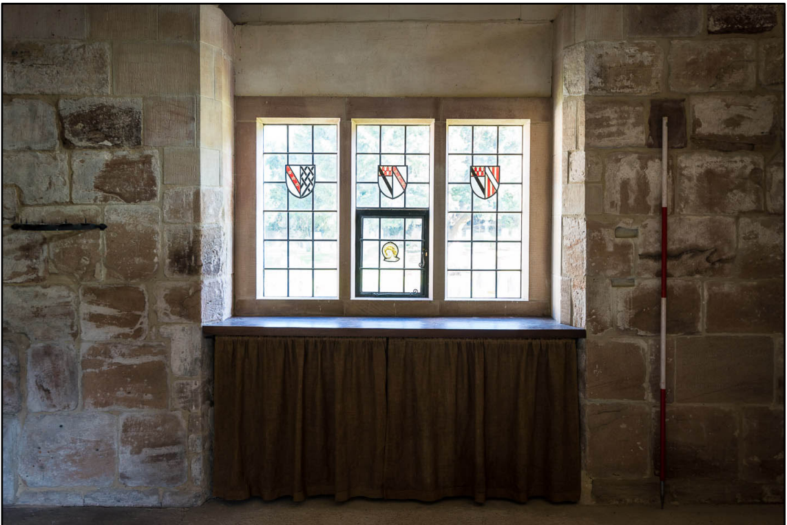
Appendix 5.133: Detail of inserted window in southeast wall of F13 (2m scale) (Photo 62)
