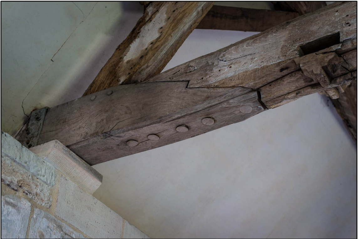
Appendix 5.126: Detail of scarf repair on tie beam of roof truss of F13 (Photo 64)
