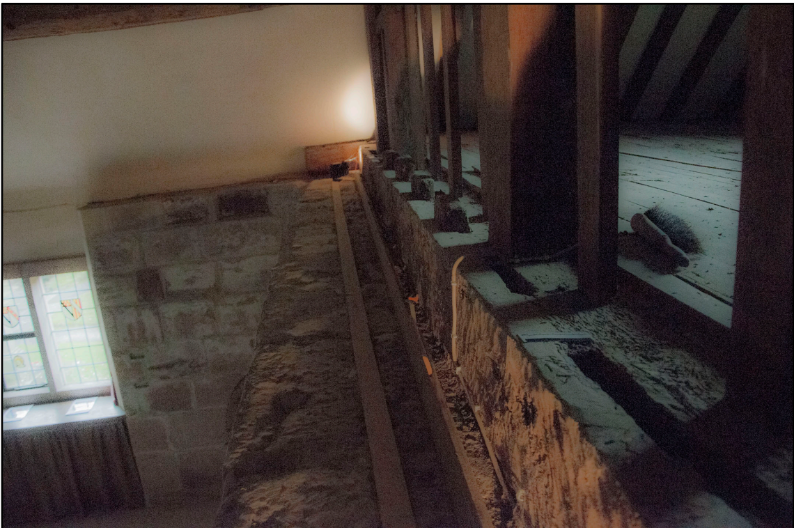
Appendix 5.136: Detail along wallplate at south end of F13 (10cm scale) looking east (Photo 161)
