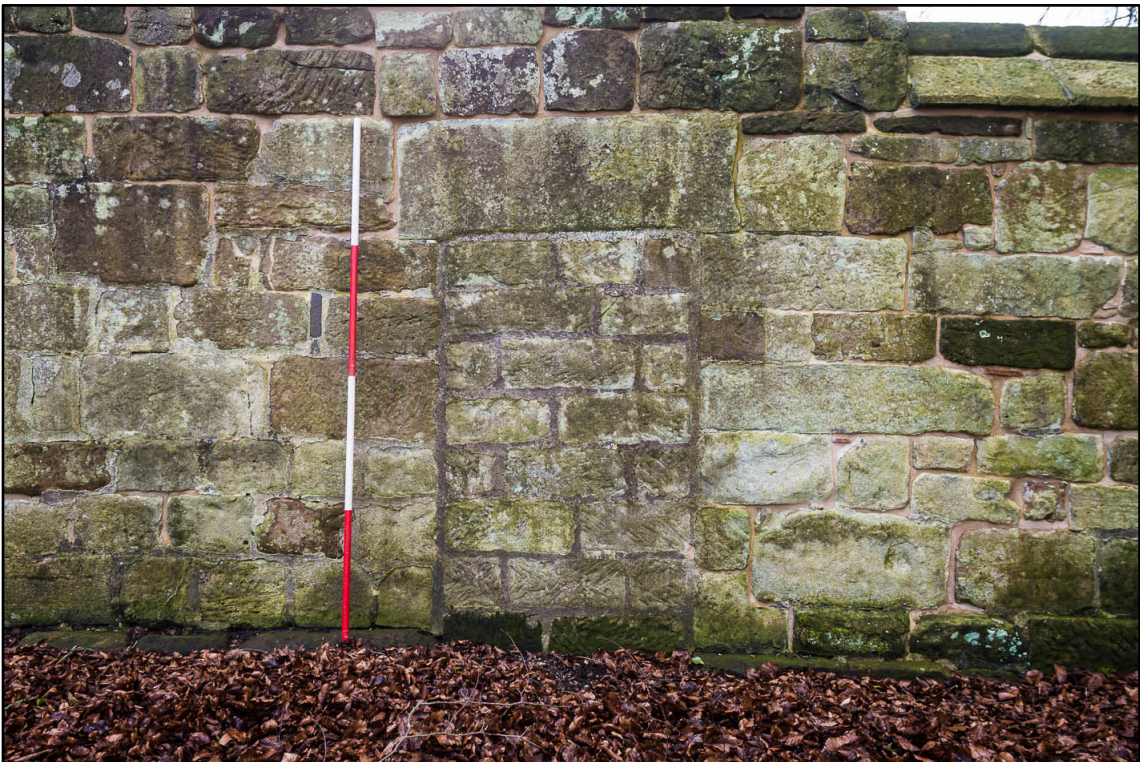
Appendix 5.12: Detail of blocked doorway in garden wall, looking south (1m scale) (Photo 43)
