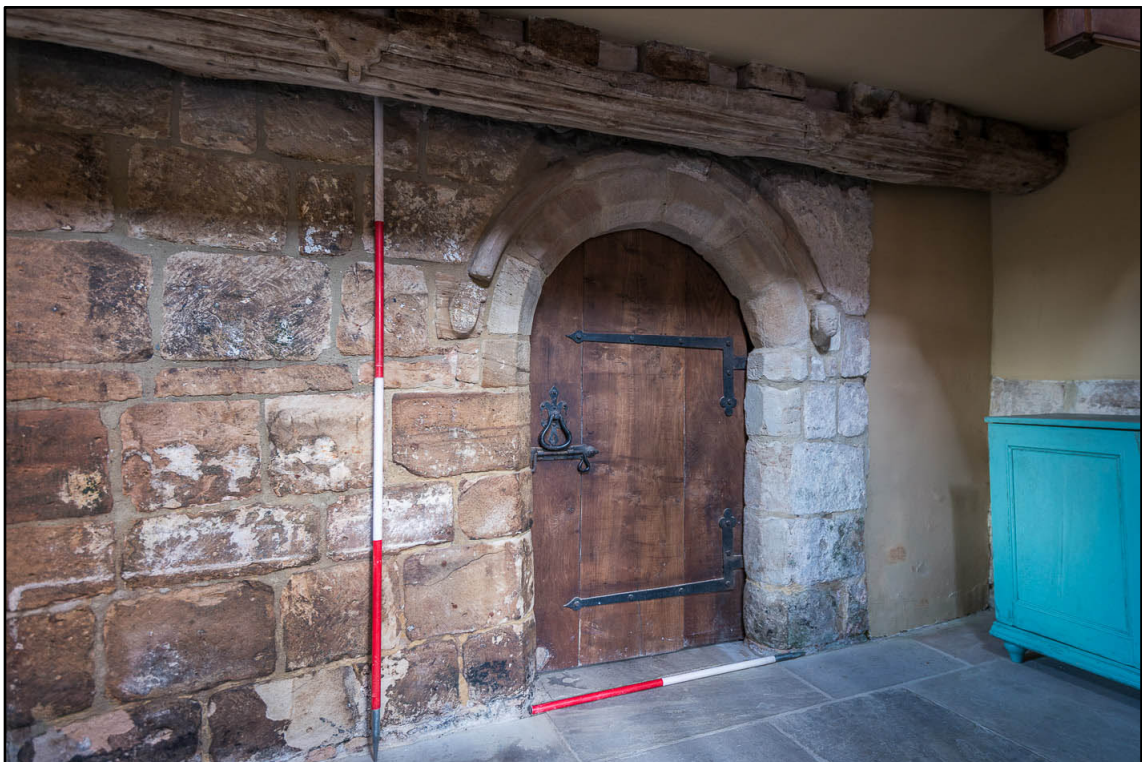
Appendix 5.95: Detail of doorway in north wall of G9 (south wall of 12-13 th century section of Building 2; 1m/2m scale) (Photo 74)
