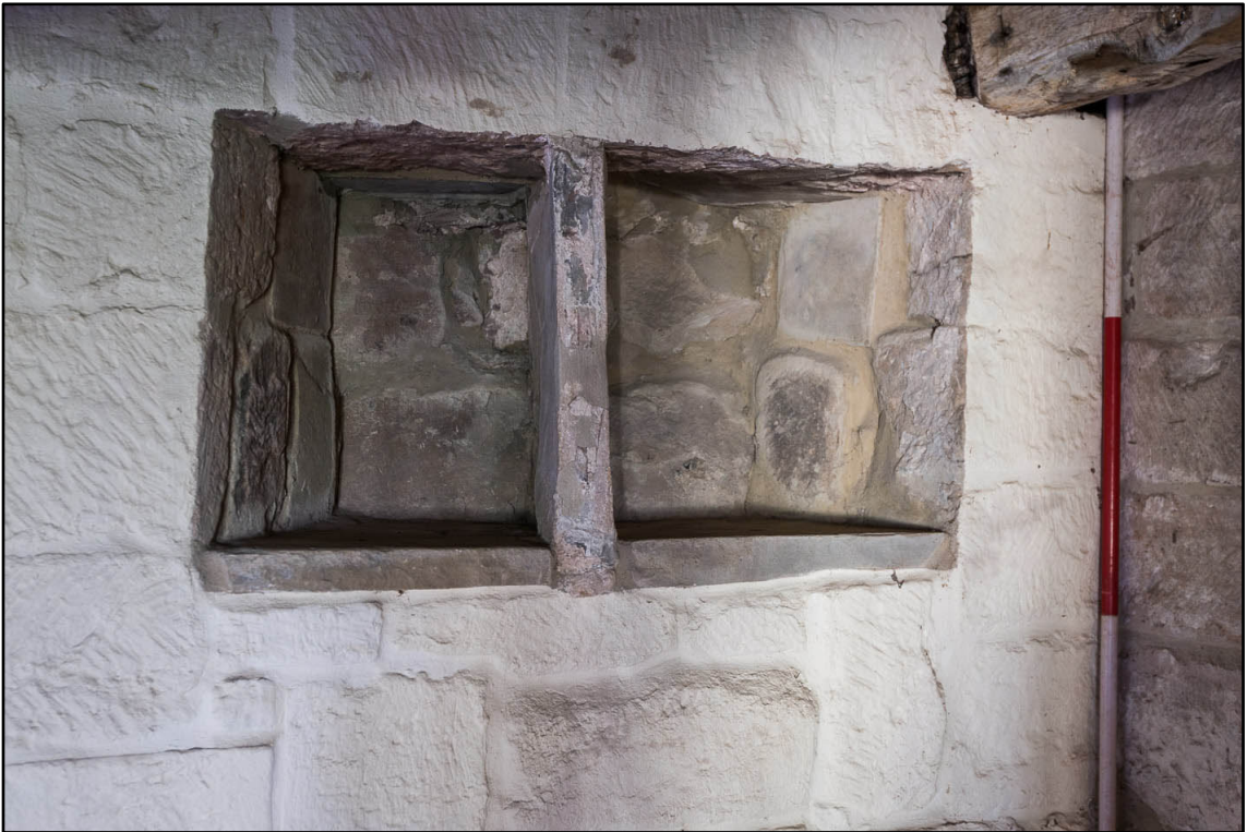
Appendix 5.106: Detail of blocked window (?) in east wall of G10 (2m scale) (Photo 76)
