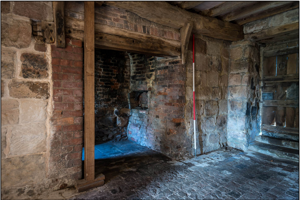
Appendix 5.116: Detail of inserted fireplace in north wall of G12 (2m scale) (Photo 99)
