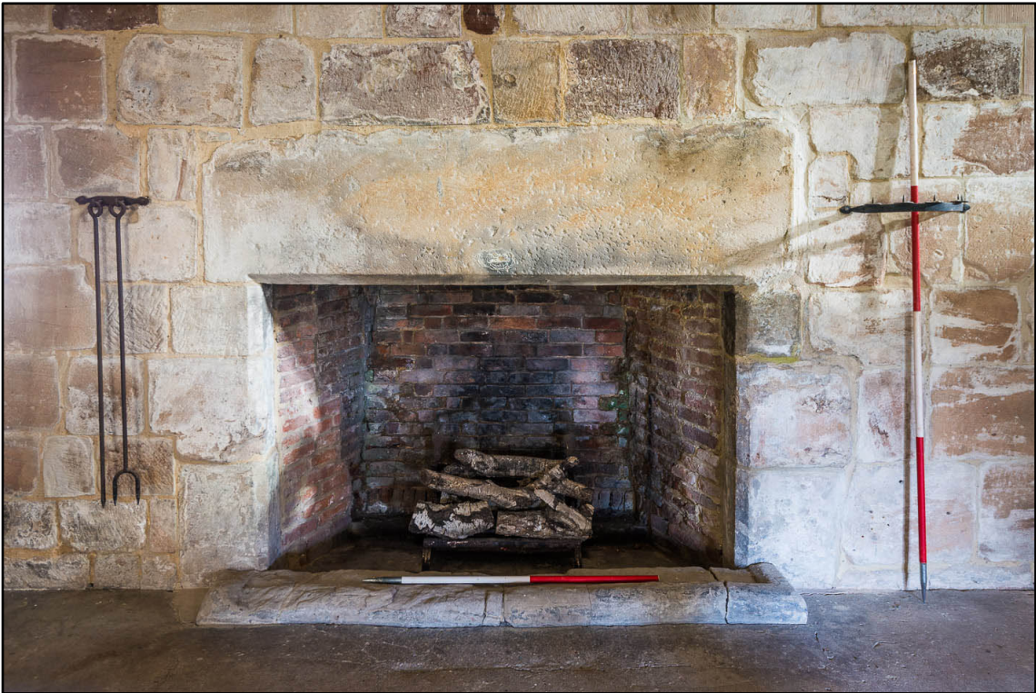
Appendix 5.135: Detail of fireplace in east wall of F13 (2m scale) (Photo 66)
