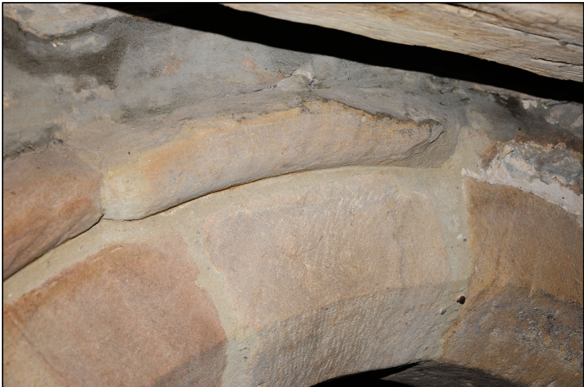
Appendix 5.98: Detail of hood moulding above doorway in north wall of G9 (Photo 175)
