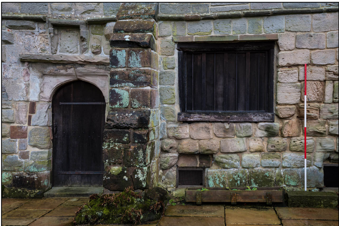
Appendix 5.78: Detail of ground floor of west elevation of Building 2 showing d22 and I18 (2m scale) (Photo 24)
