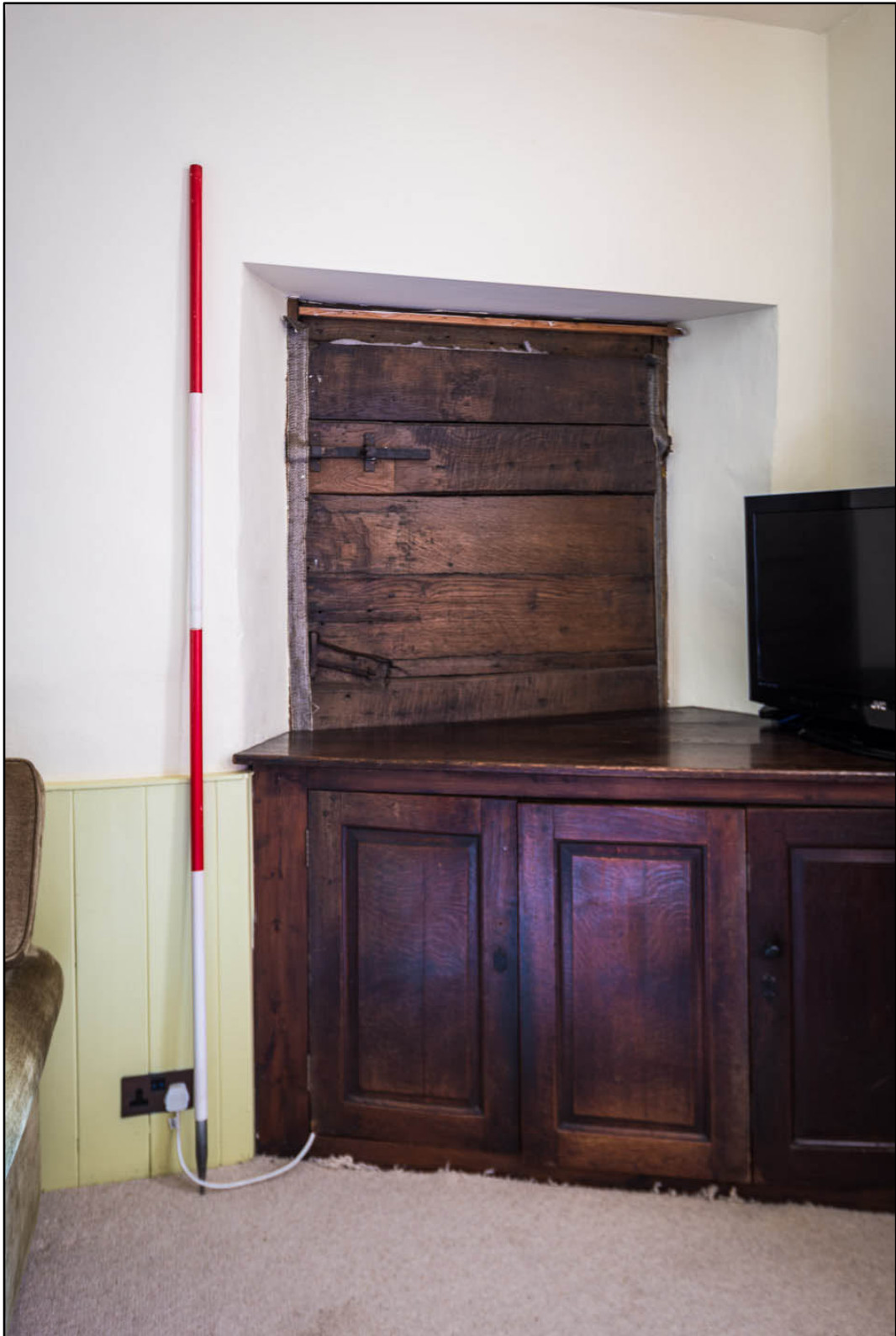
Appendix 5.45: Blocked internal doorway into southeast corner of G2 (2m scale) (Photo 143)
