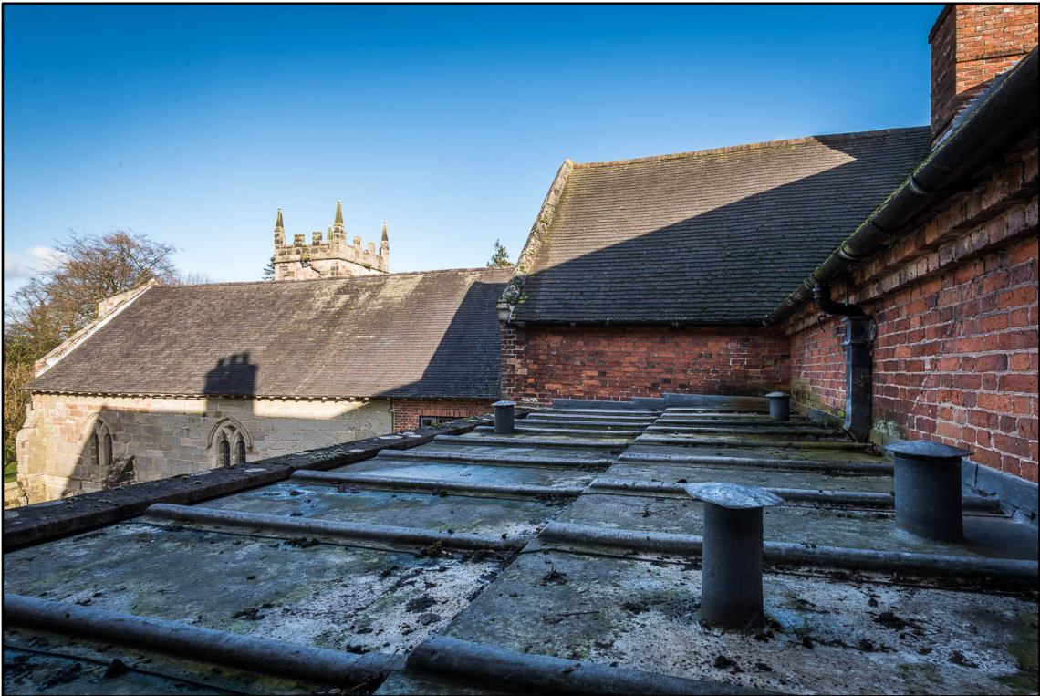
Appendix 5.23: Detail of rear flat roof above Building 1; note gable scars (Photo 107)
