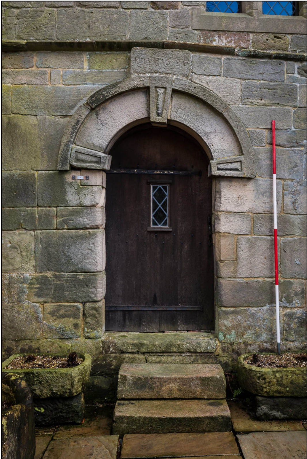
Appendix 5.79: Detail of west doorway into G12 of Building 2 (2m scale) (Photo 21)
