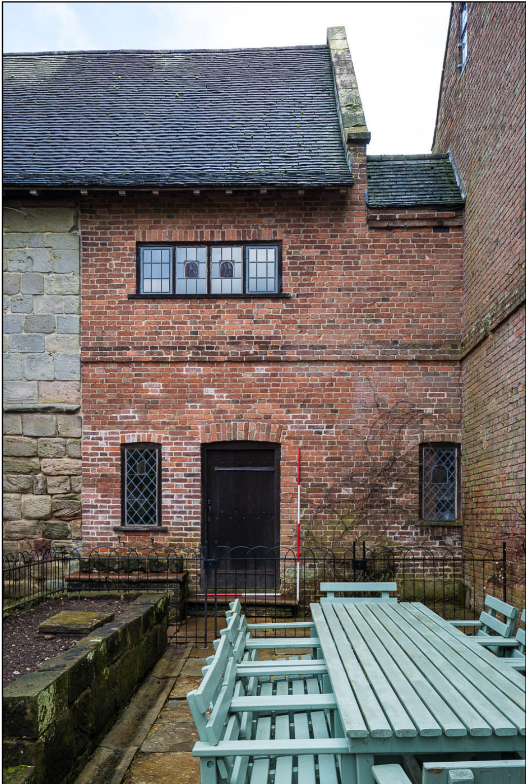
Appendix 5.81: Detail of west doorway into G9 of Building 2 (2m scale) (Photo 30)
