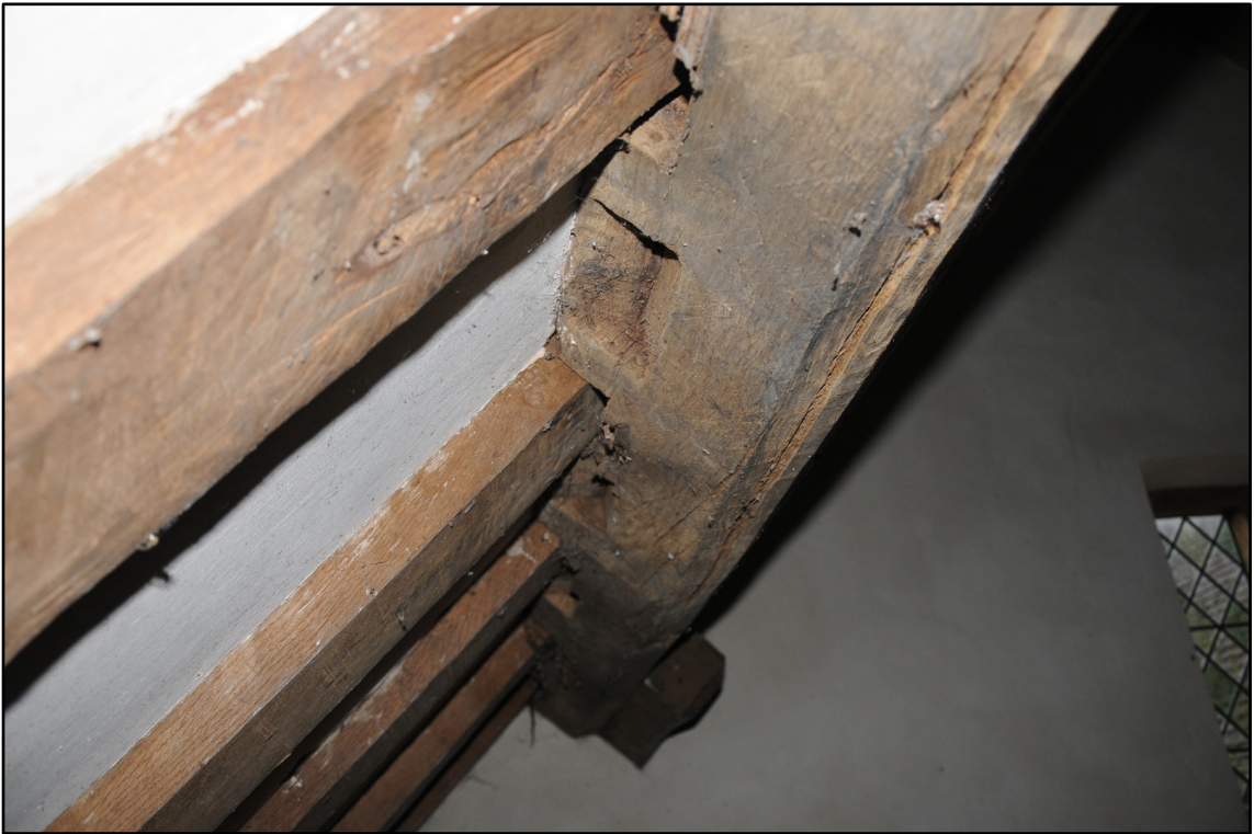
Appendix 5.141: Detail of re-used purlin in southeast roof section in F13 (Photo 159)
