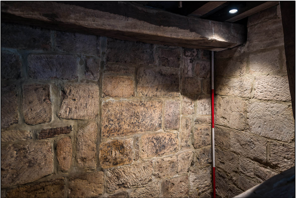
Appendix 5.104: Detail of blocked window in southwest corner of G10 (2m scale) (Photo 80)
