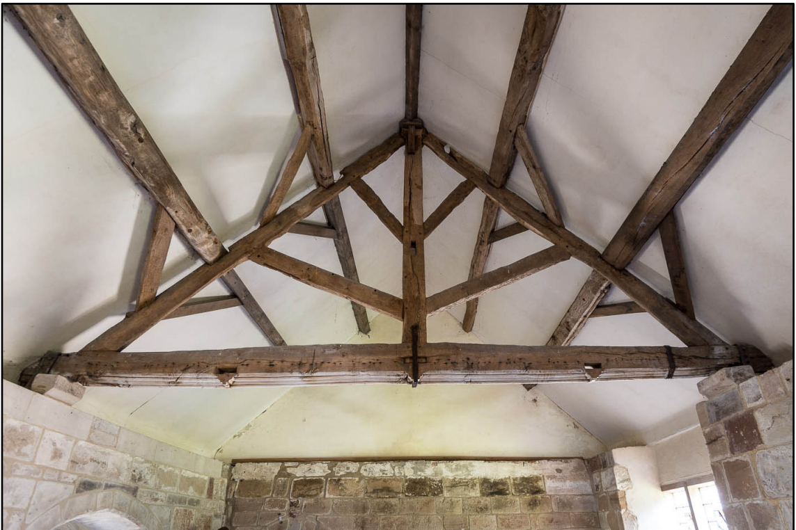
Appendix 5.127: General view of roof truss at north end of F13, looking north (Photo 65)
