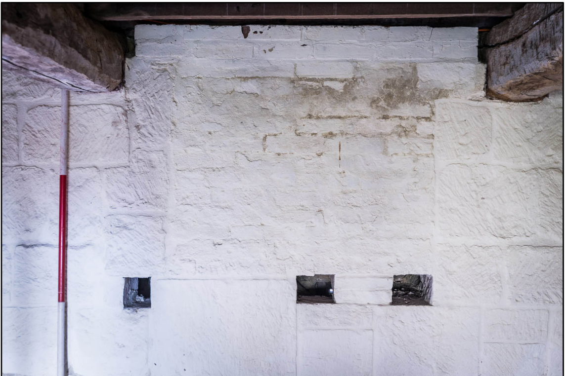
Appendix 5.107: Detail of blocked window (?) in east wall of G10 (2m scale) (Photo 77)
