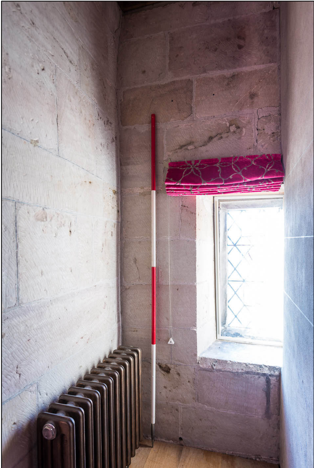
Appendix 5.62: Detail of reveal behind fireplace in F7, looking west (2m scale) (Photo 128)
