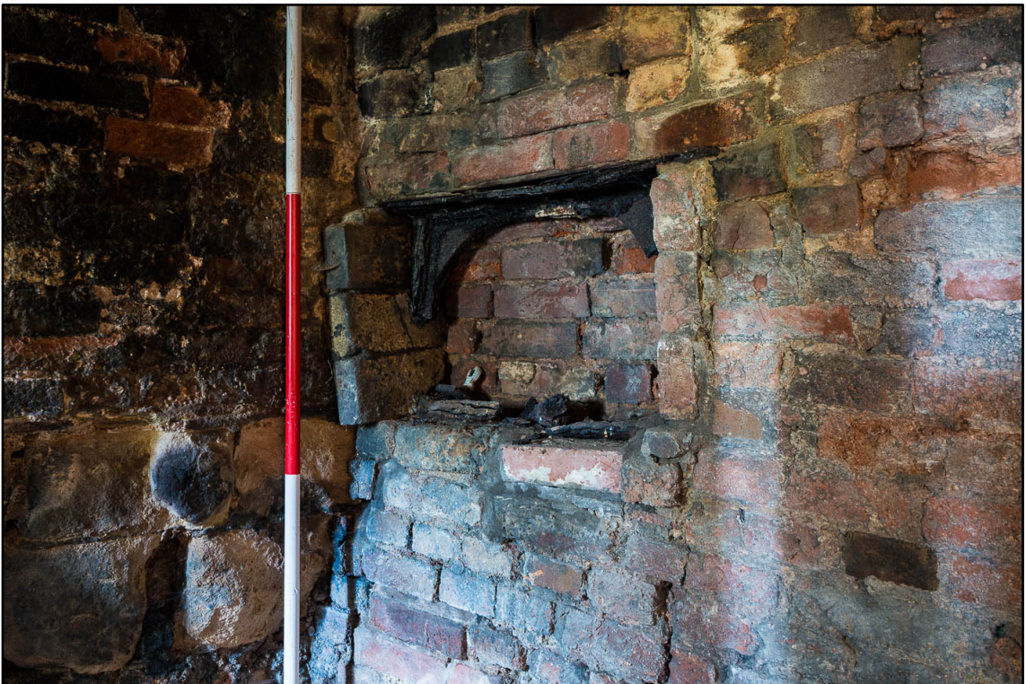
Appendix 5.117: Blocked bread oven in northeast corner of chimney reveal in G12 (Photo 100)
