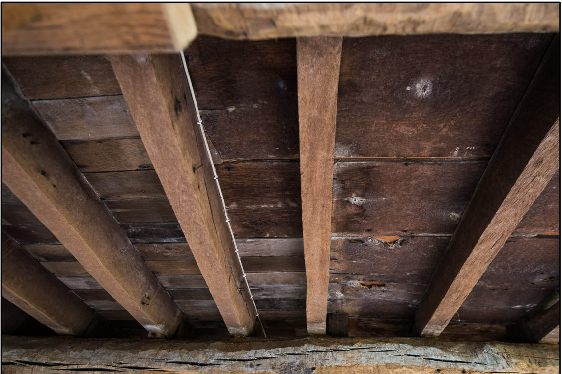
Appendix 5.109: Detail of change in ceiling boards in G10 (Photo 79)
