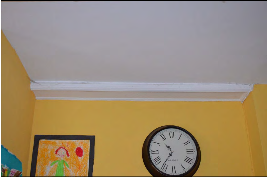
Appendix 2.7: Detail of moulded beam above doorway between G7 and G8, looking south
