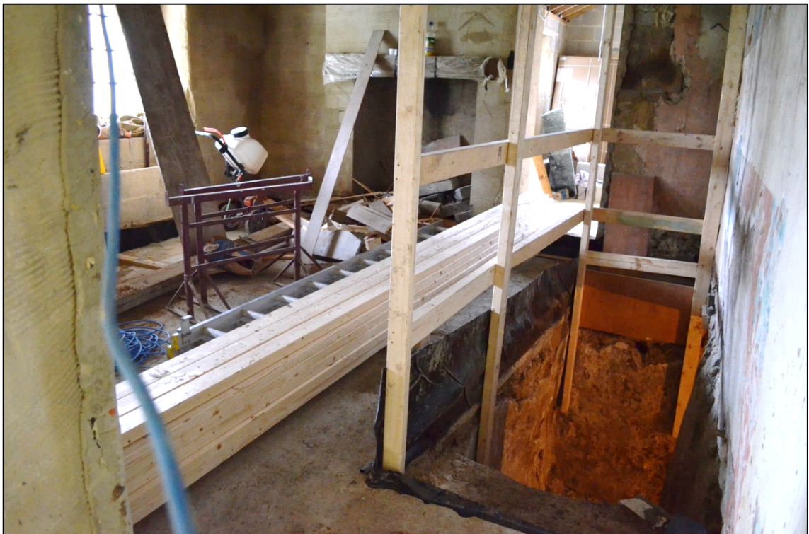
Appendix 2.2: View showing access to cellar within Holy Bush Farmhouse, looking east
