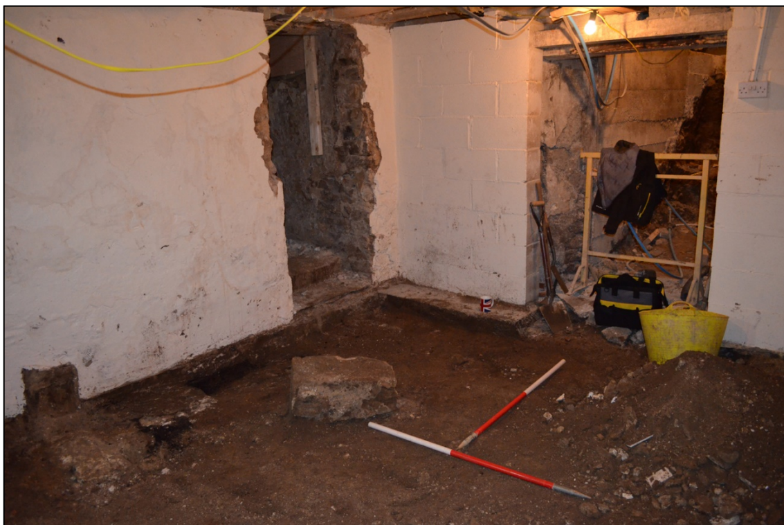
Appendix 2.3: View of cellar following removal of flagstones, looking south-west (scale 1m)
