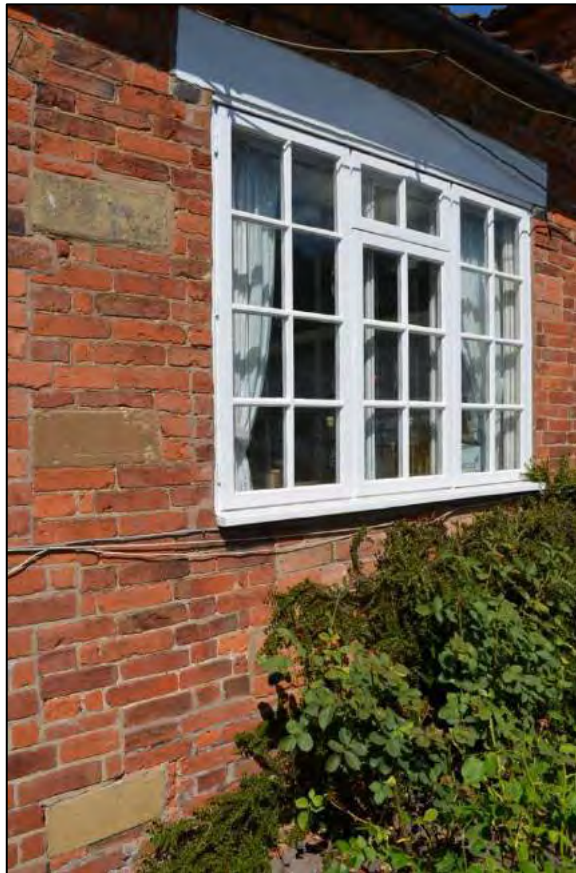
Appendix 2.26: Detail of window in west elevation of Building 3, noting scar of blocked door below sill
