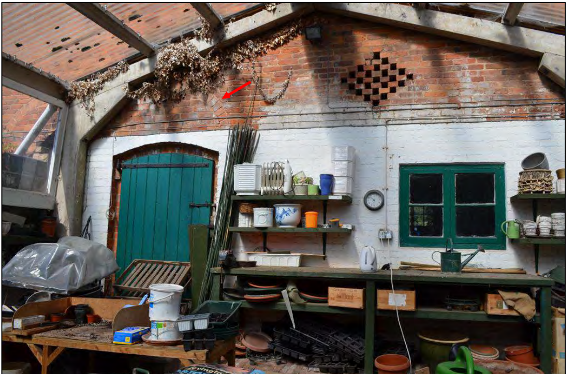
Appendix 2.32: Detail of east elevation of Building 4 from modern portal frame structure, noting blocked arched entrance (indicated)
