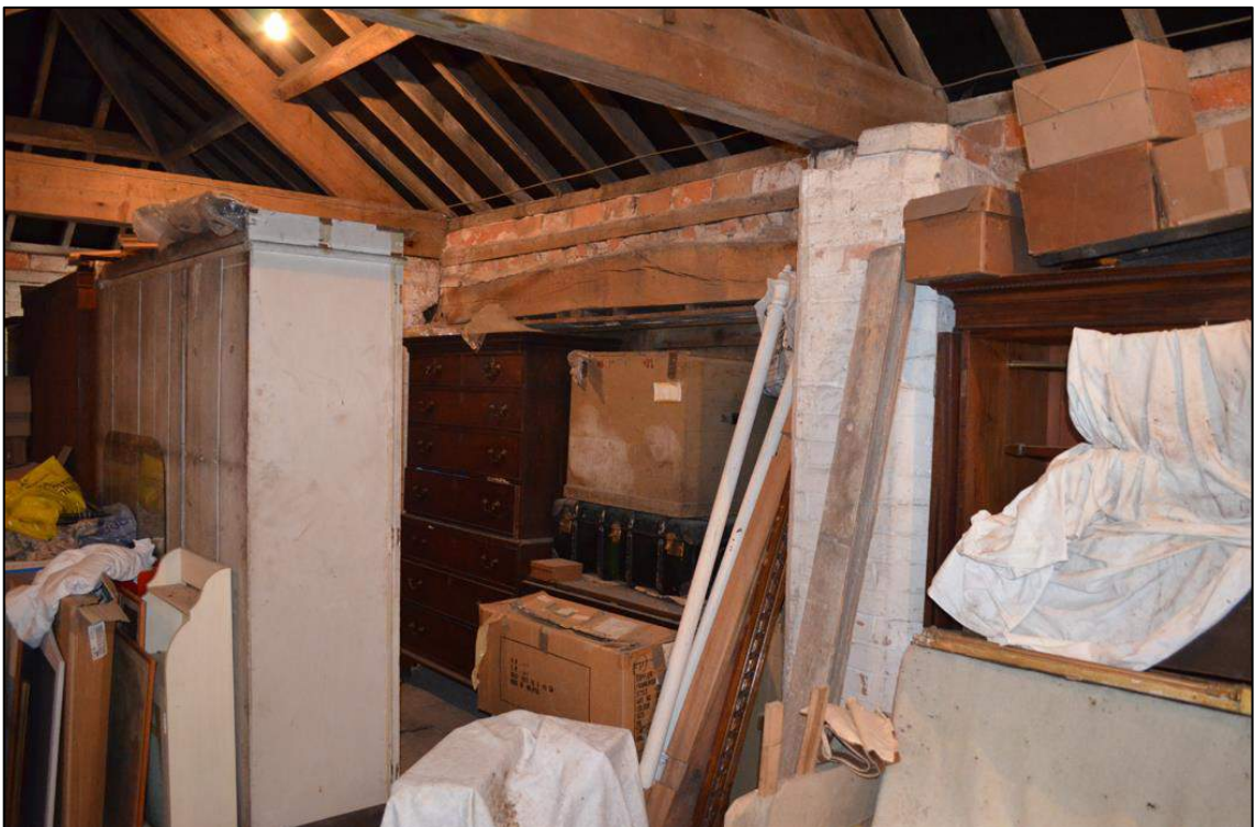
Appendix 2.36: Detail view of interior of F8 in Building 4, looking southeast, noting timber lintel of former doorway
