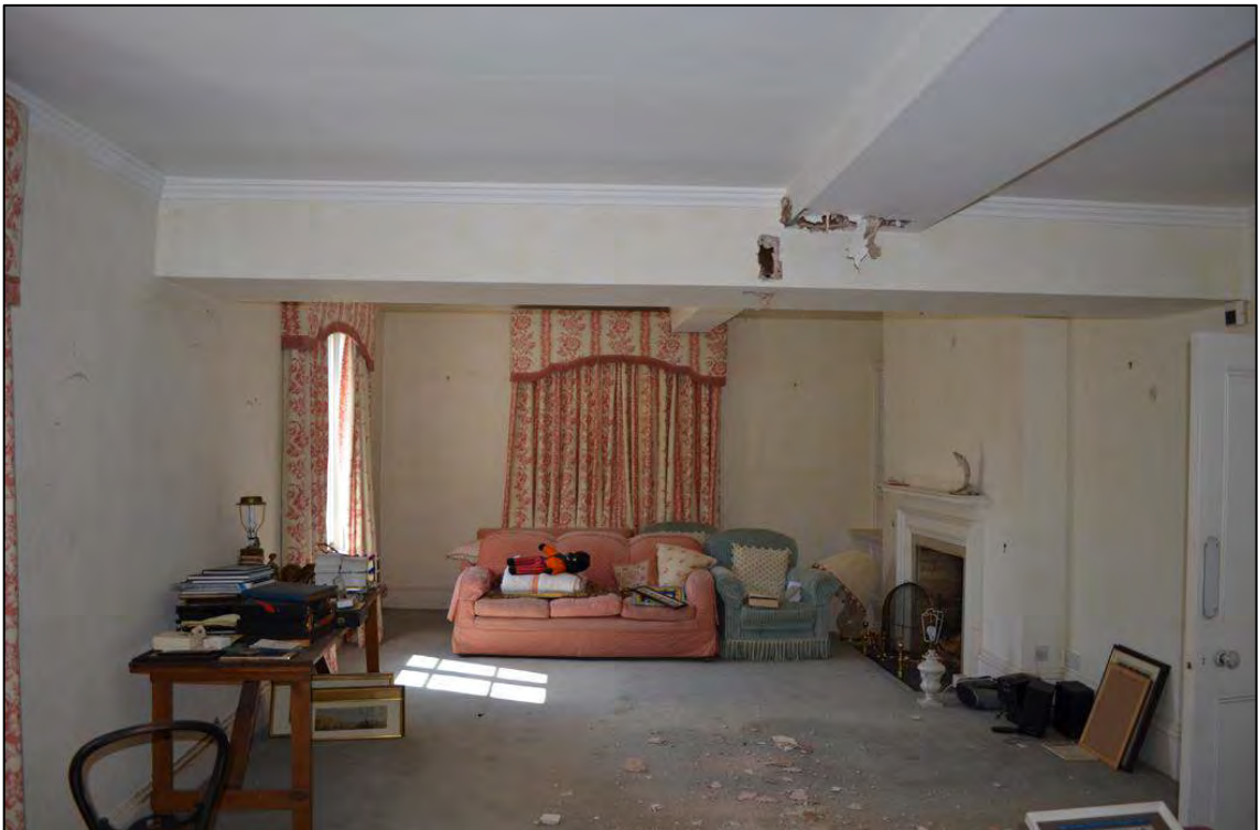
Appendix 2.12: General view of G5 in Building I, looking south, noting boxed in RSJs
