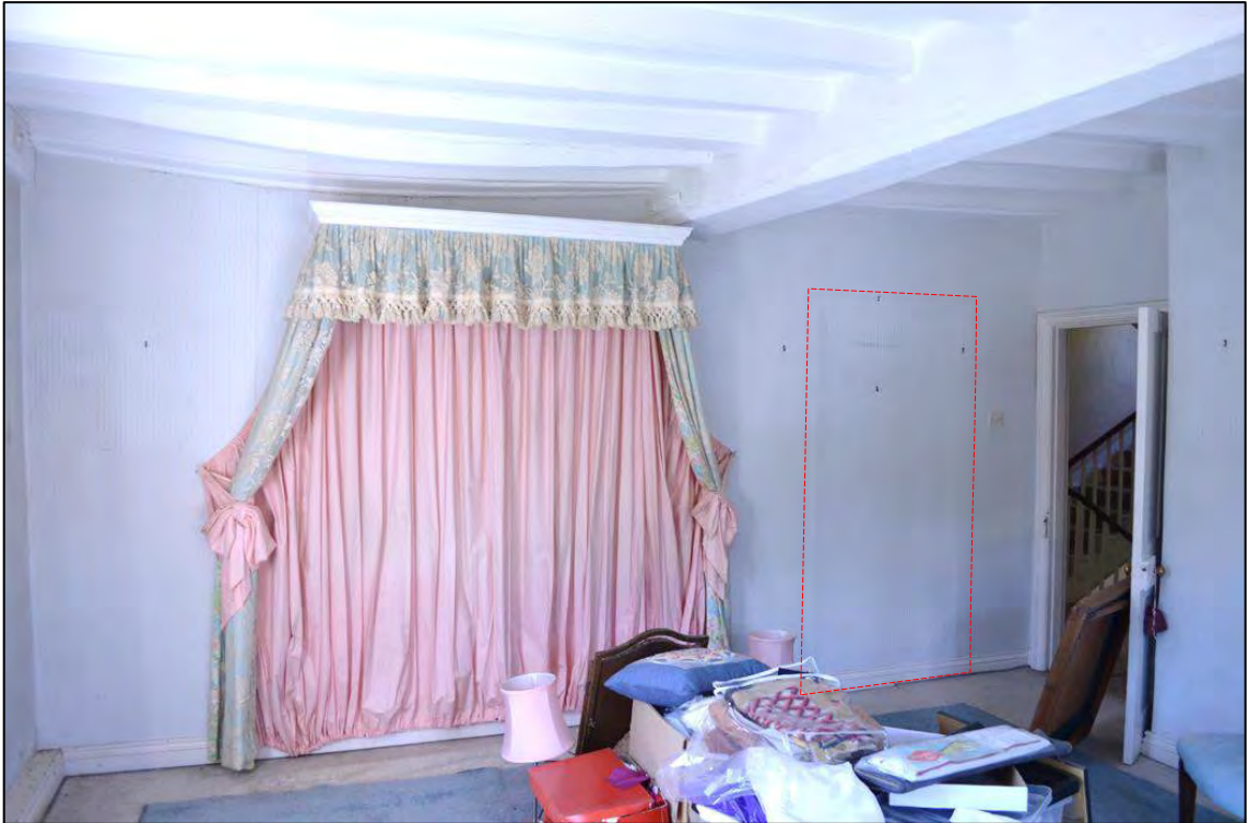
Appendix 2.17: General view of F3 in Building I, looking south, noting shadow of blocked door (indicated)
