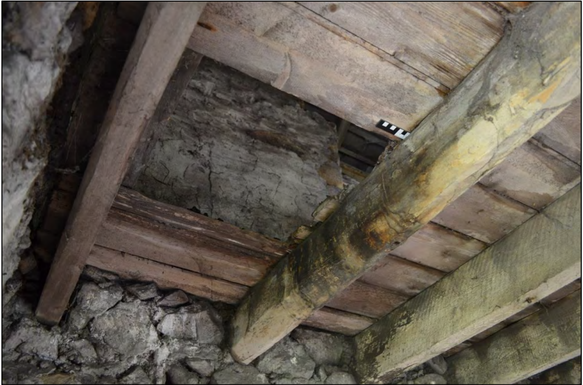
Appendix 2.9: Detail of worn joist and hole in ceiling in southwest corner of GI (scale: 1cm intervals)
