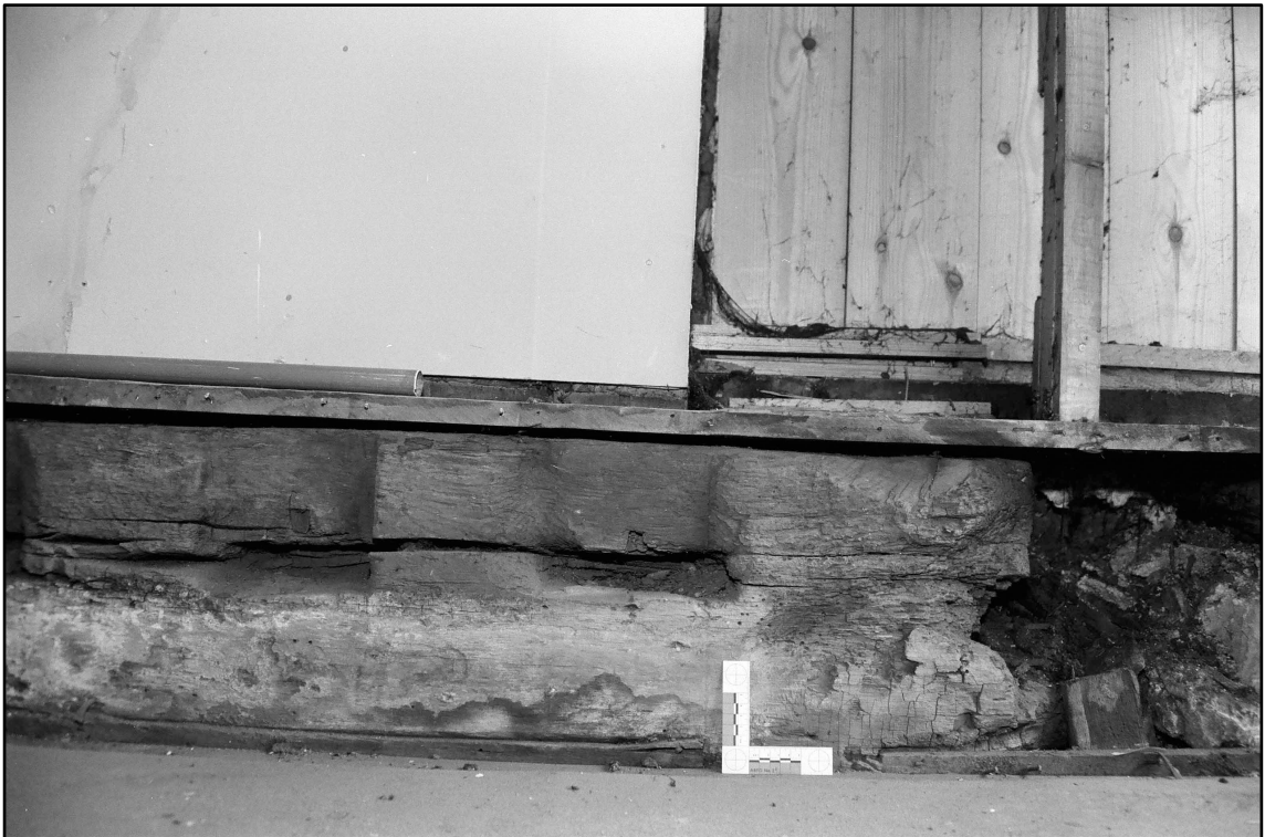
Appendix 2.22: Detail of mortice in re-used beam in GI , looking west (5cm scale; Film 2.12)
