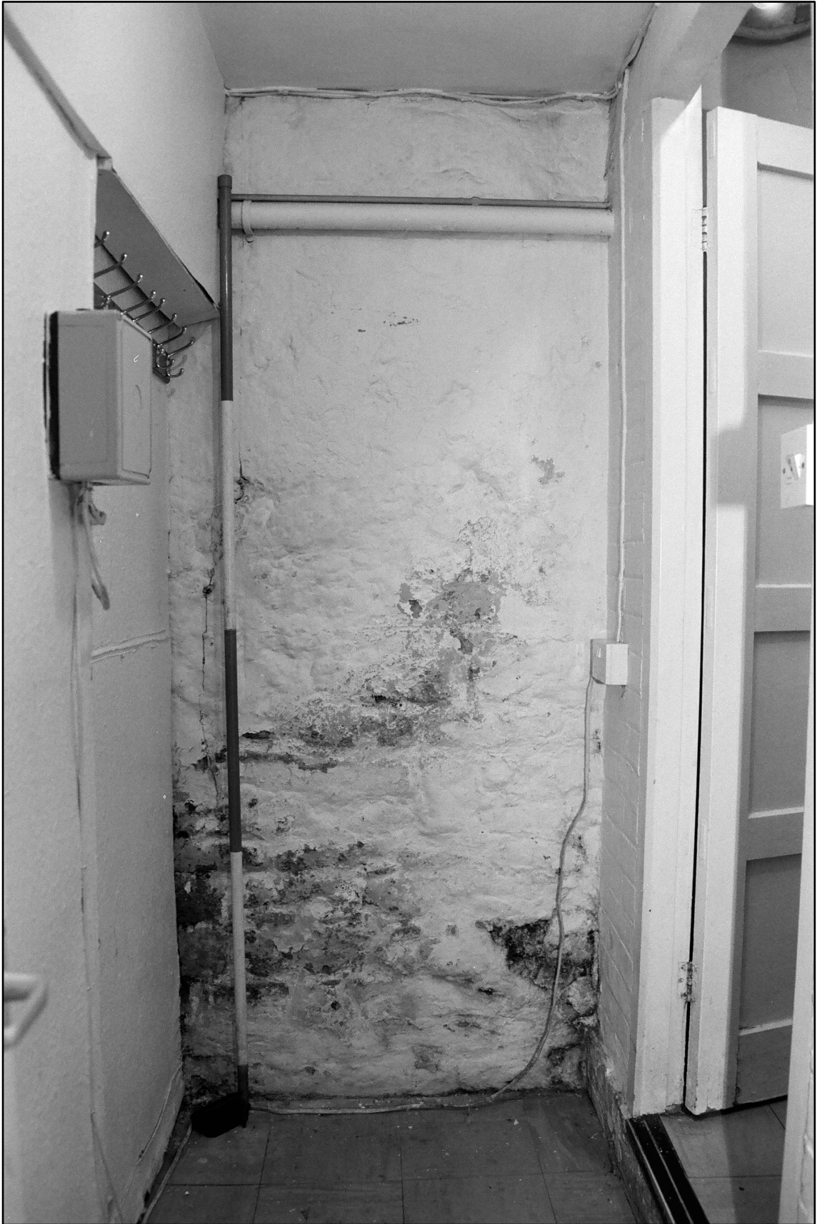
Appendix 2.12: General view of masonry wall in C4 , looking south (2m scale; Film 1.30)
