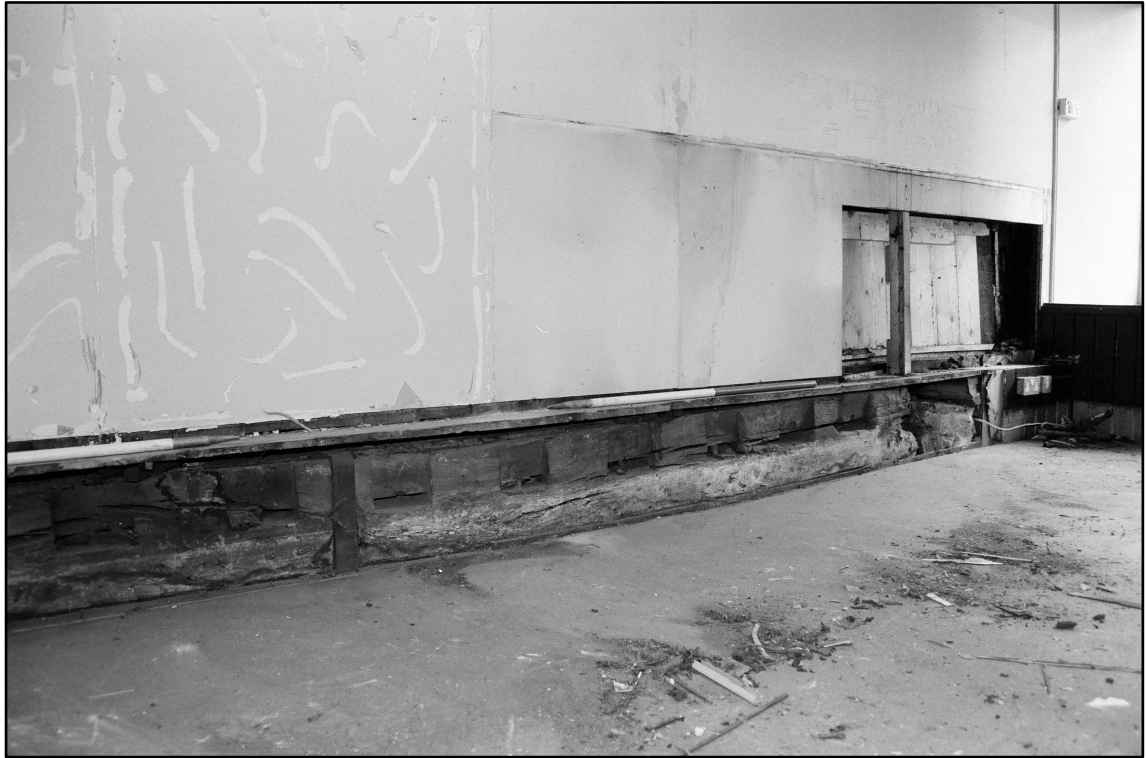
Appendix 2.25: General view looking along re-used beam in GI (1m scale; Film 2.17)
