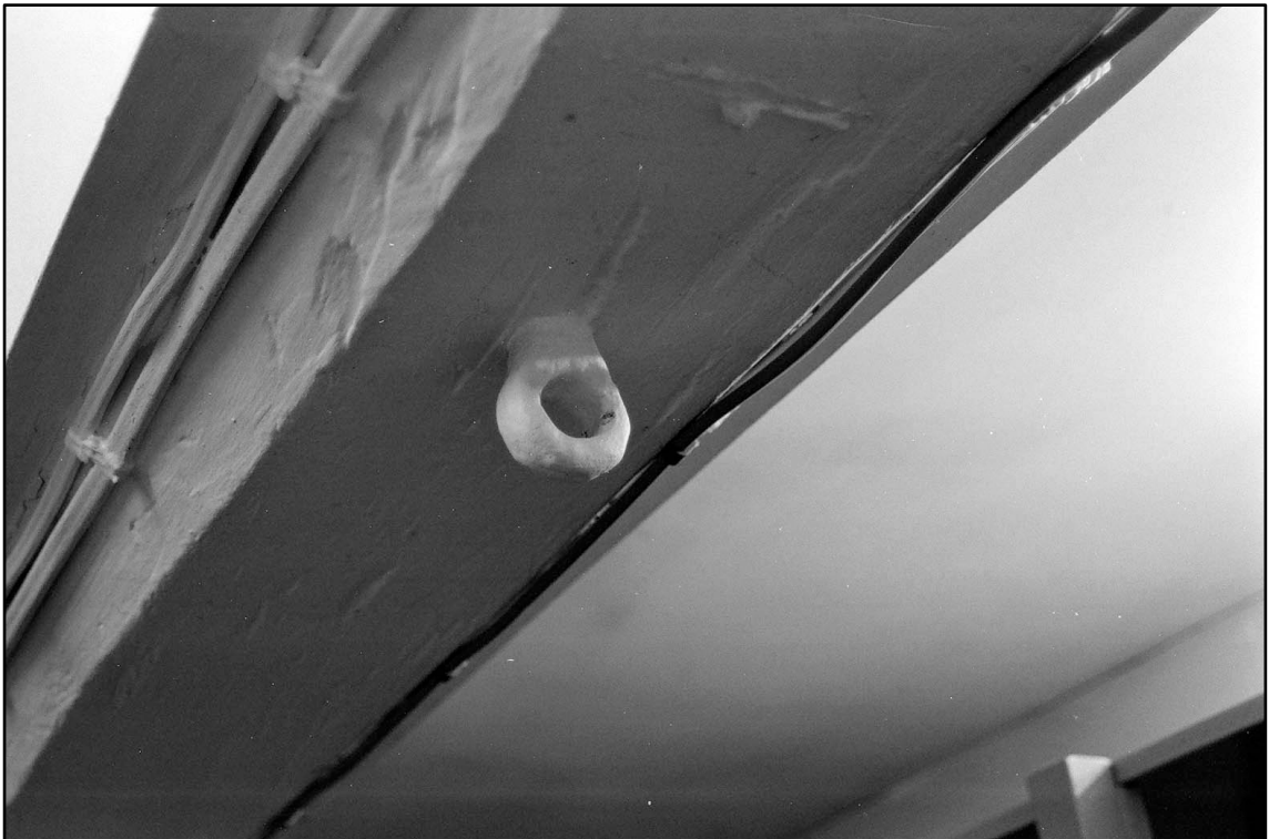
Appendix 2.16: Detail of ceiling loop on beam in CI, looking south (Film 1.36)
