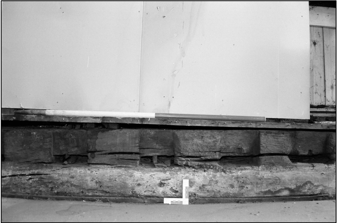
Appendix 2.21: Detail of mortices in re-used beam in GI , looking west (5cm/1m scale; Film 2.10)
