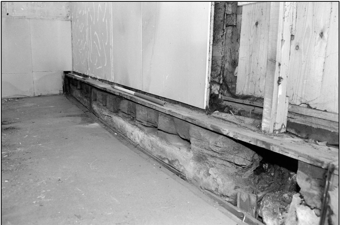
Appendix 2.24: General view looking along re-used beam in G1 (1m scale; Film 2.14)
