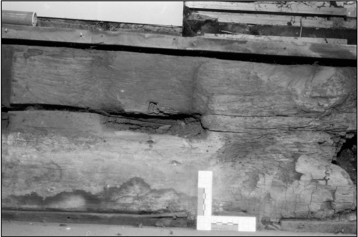
Appendix 2.23: Detail of white paint on re-used beam in G1 , looking west (Film 2.13)
