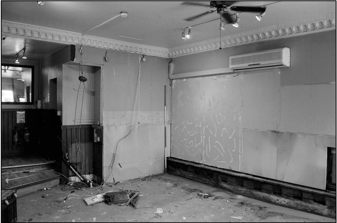
Appendix 2.4: General view of interior of G1 following soft strip; note beam (2m scale; Film 1.12)
