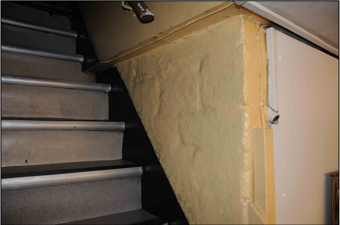
Appendix I.8: Detail of exposed section of medieval masonry in cellar, room CI
