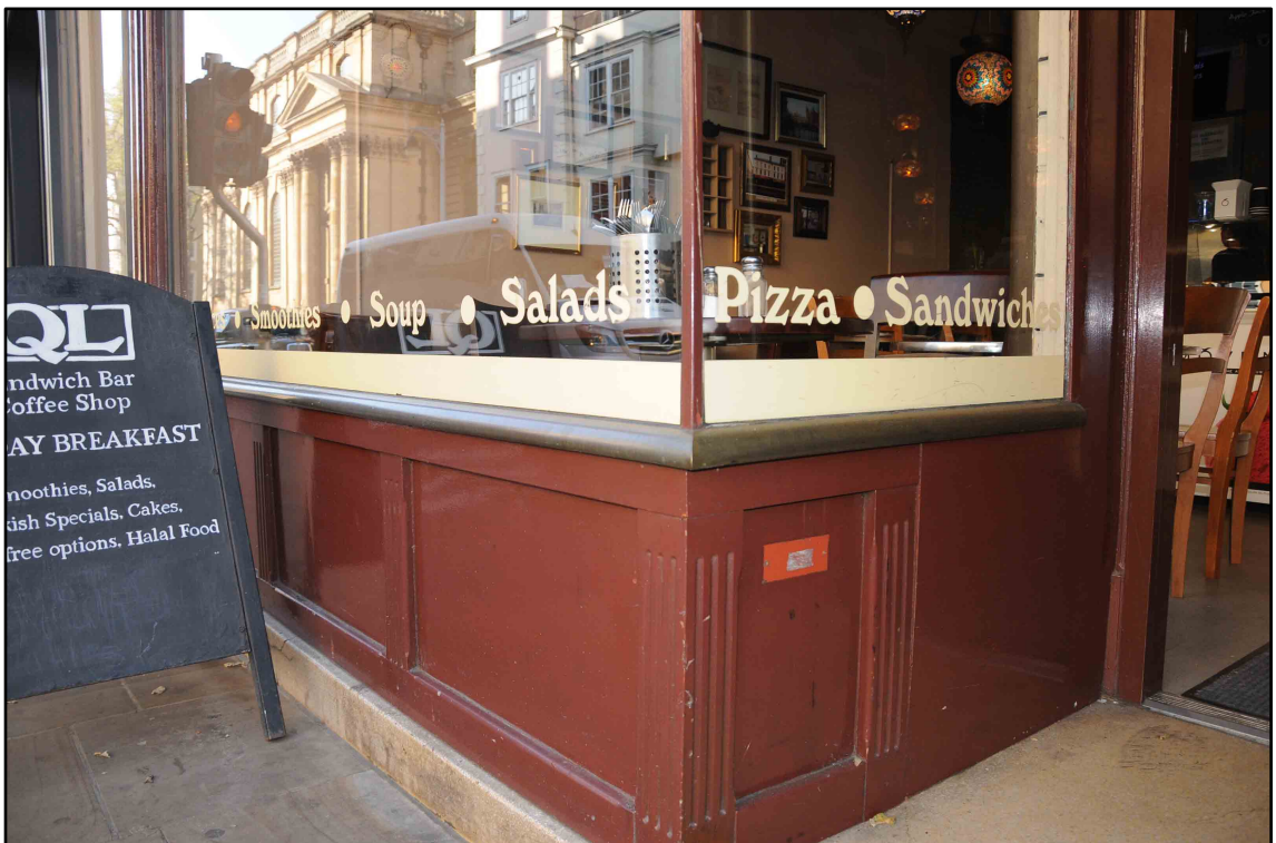
Appendix I.7: Detail of modern stall risers and (reused?) bronze edging strip
