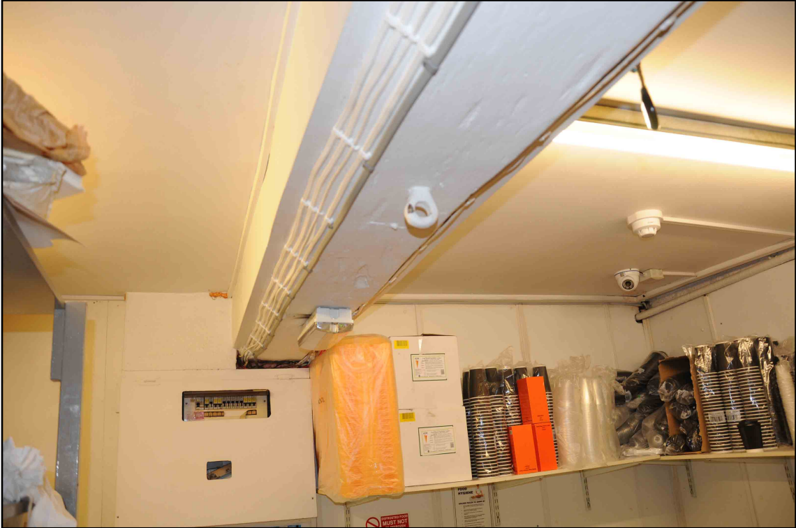
Appendix I.10: Detail view along ceiling beam in CI. Note metal lifting eye
