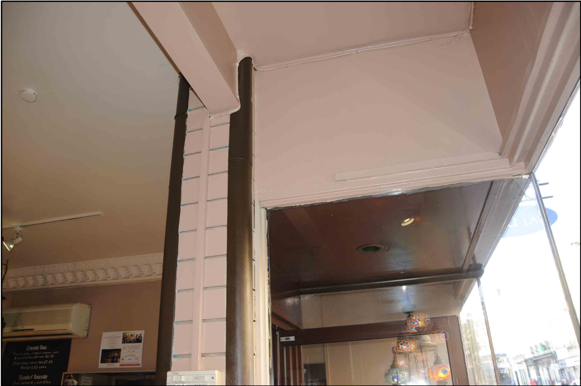
Appendix I.18: Detail of ceiling of window bay in GI; note modern surface finishes
