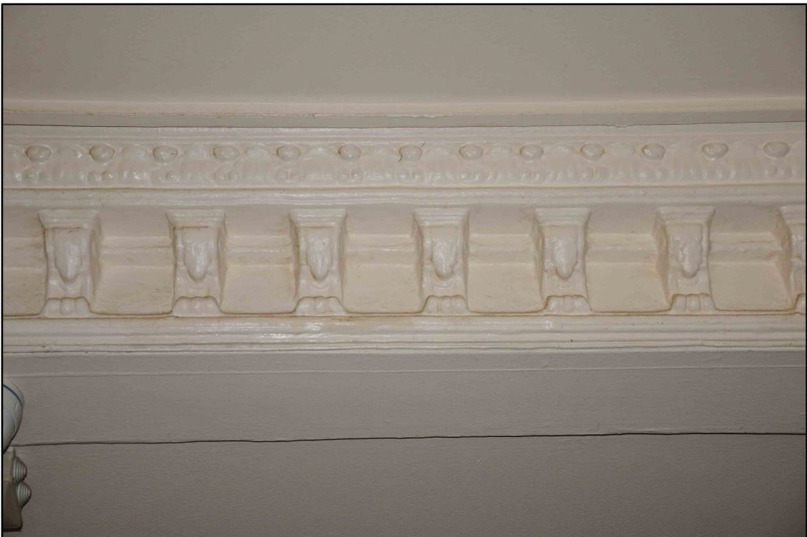
Appendix I.19: Detail of plaster cornice in GI, c.18 th century in date
