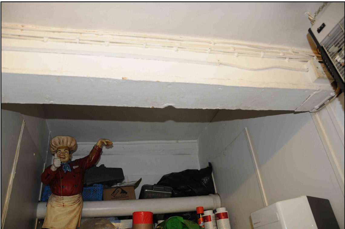
Appendix I.13: Detail of chamfered ceiling beam along western wall of rooms C2, C3, C4
