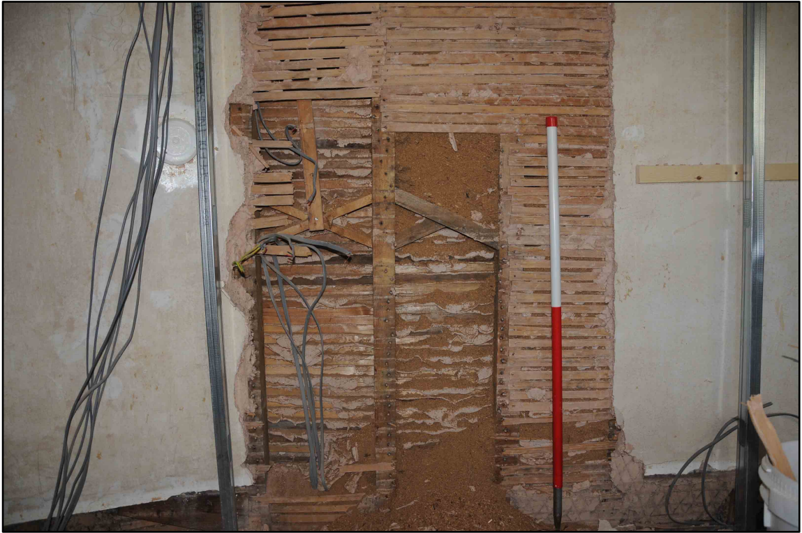
Appendix 2.14: West wall of Bedroom 4 during of laths; note sawdust (1m scale; b/w Film I.28)
