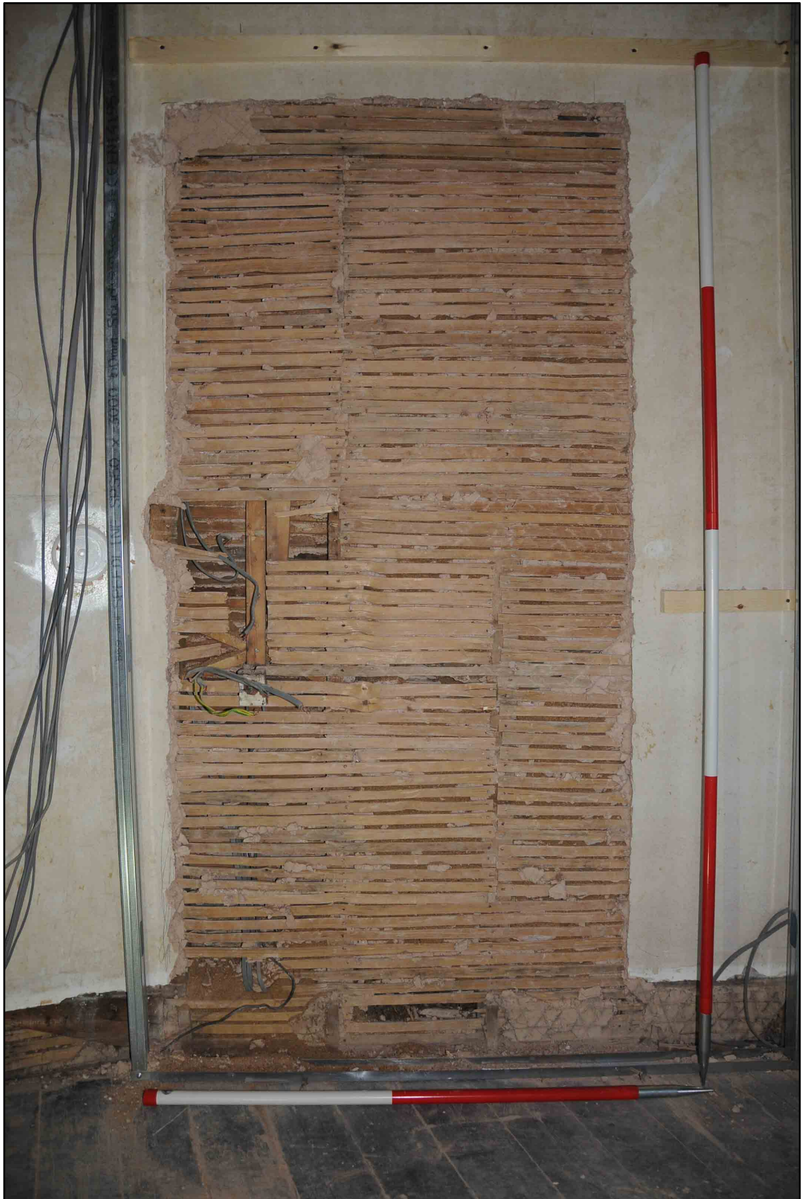
Appendix 2.9: West wall of Bedroom 4 following plaster removal (1m/2m scale; b/w Film 1.24)
