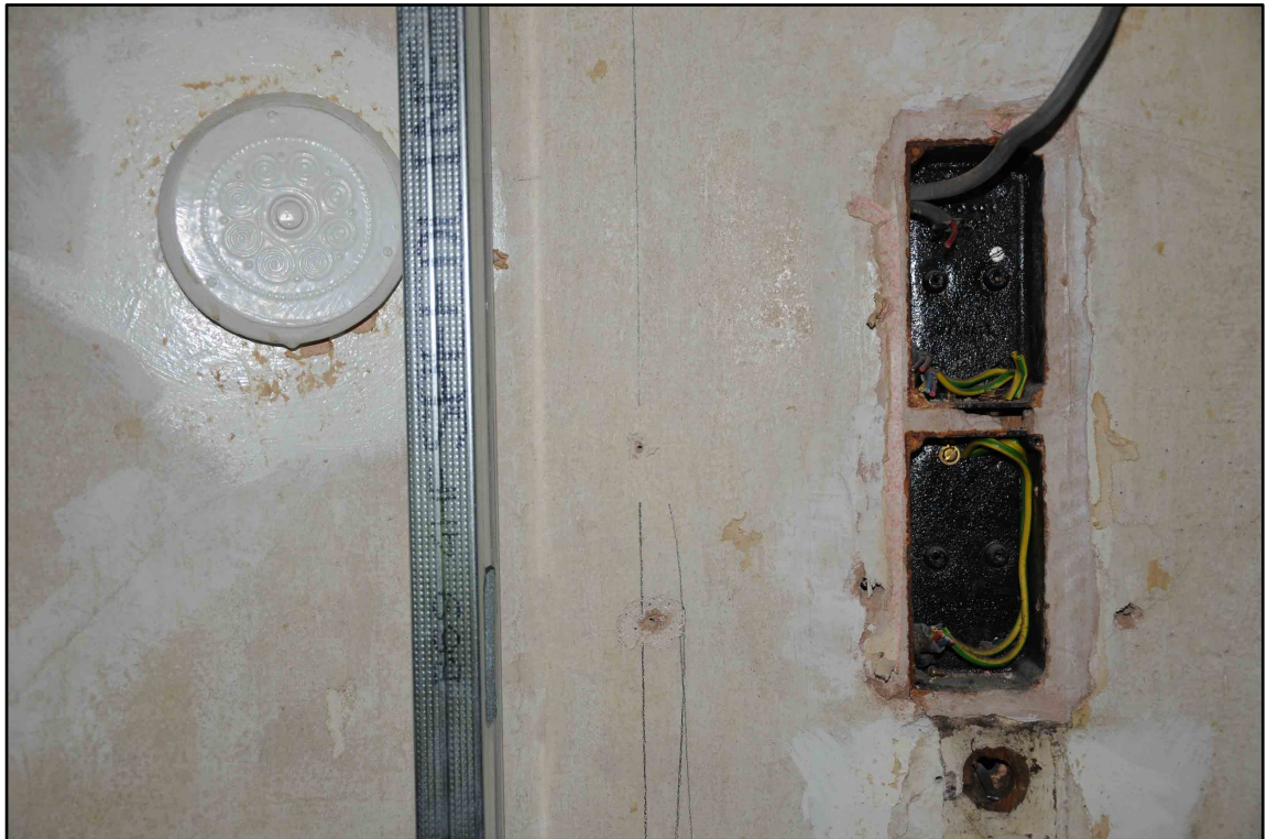
Appendix 2.7: Detail of push switch and housing in Bedroom 4 prior to works (b/w Film I.12)
