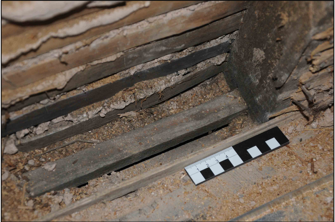
Appendix 2.18: Detail of notch at base of wall studs in Bedroom 4 (10cm scale; b/w Film 1.34)
