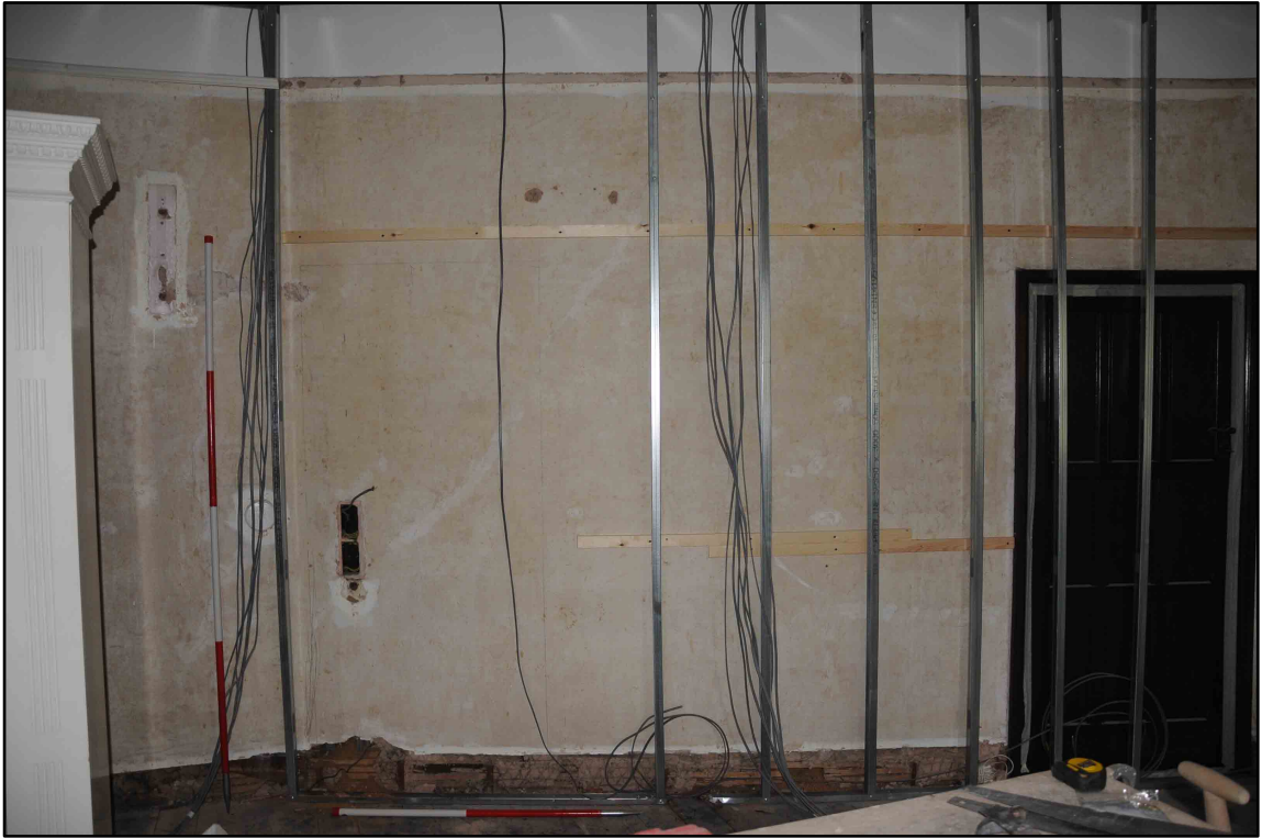
Appendix 2.5: Detail of west wall of Bedroom 4 prior to works (1m/2m scale; b/w Film I.6)
