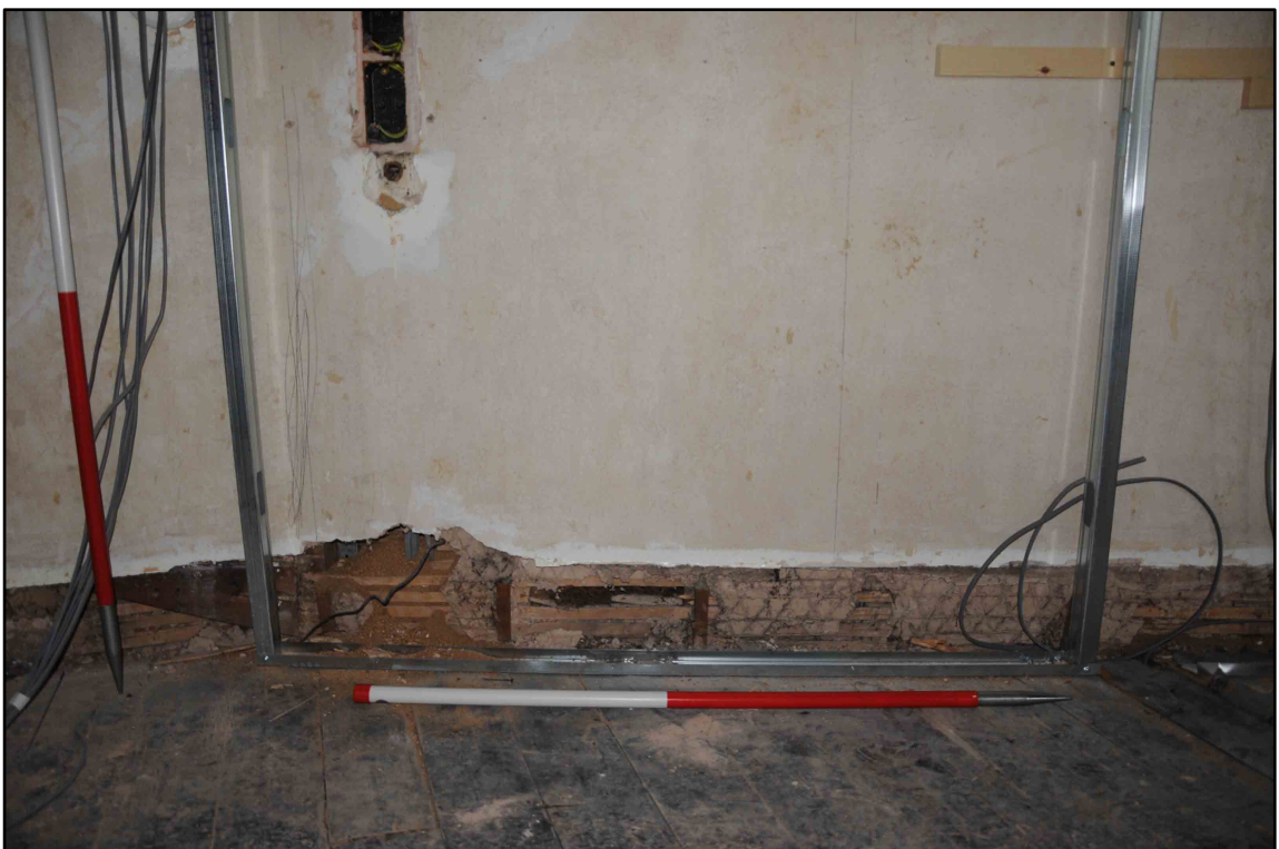
Appendix 2.6: Detail behind skirting in Bedroom 4 prior to works (1m scale; b/w Film I.10)
