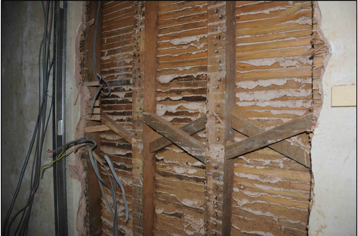
Appendix 2.15: Detail of timber noggins in Bedroom 4 following removal of laths (b/w Film I.32)
