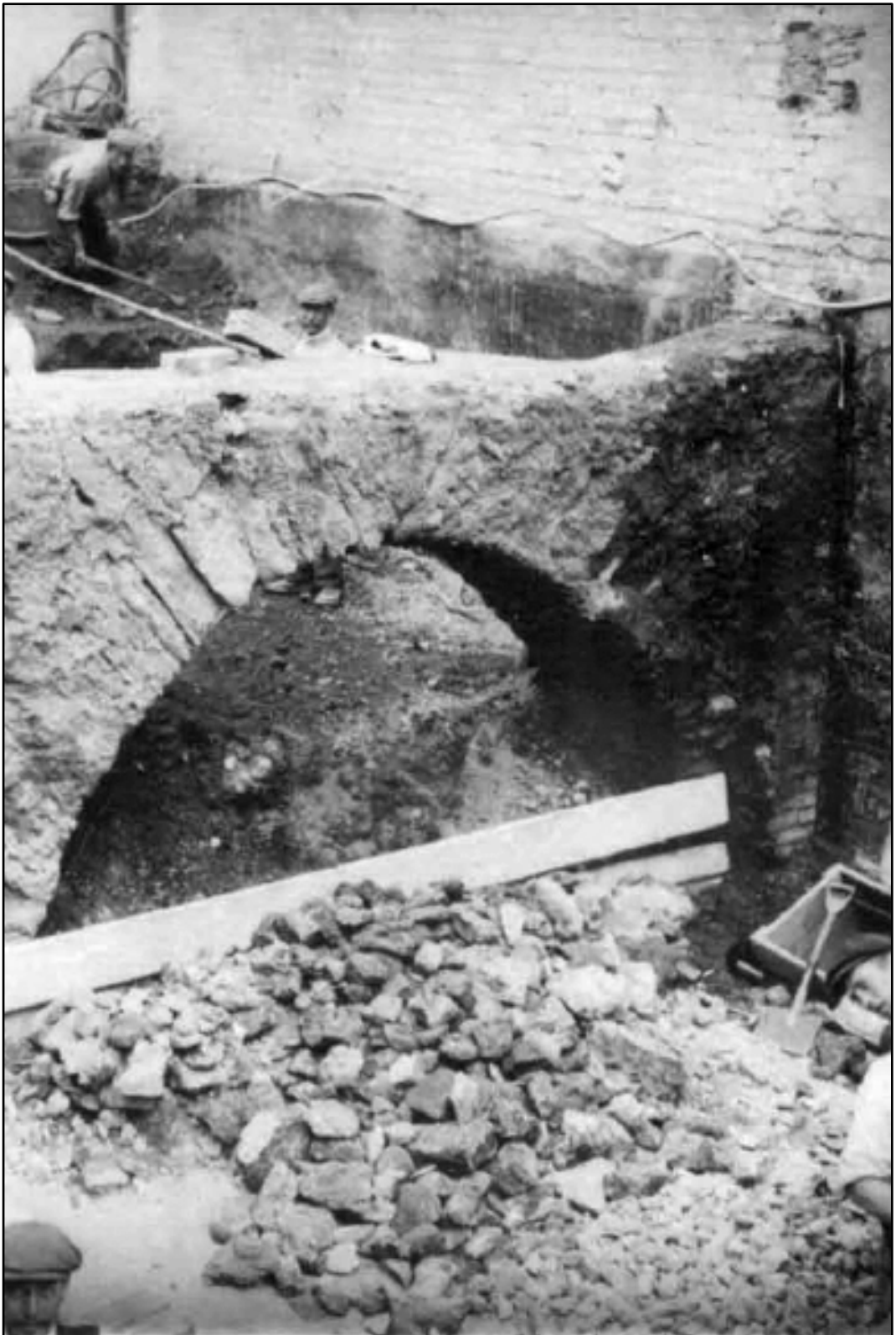
Appendix I.3: Detail of foundation relieving arch during demolition works of adjacent north range in 1911 (after Munby 1992, Figure 19; Minns archive Bodleian)
