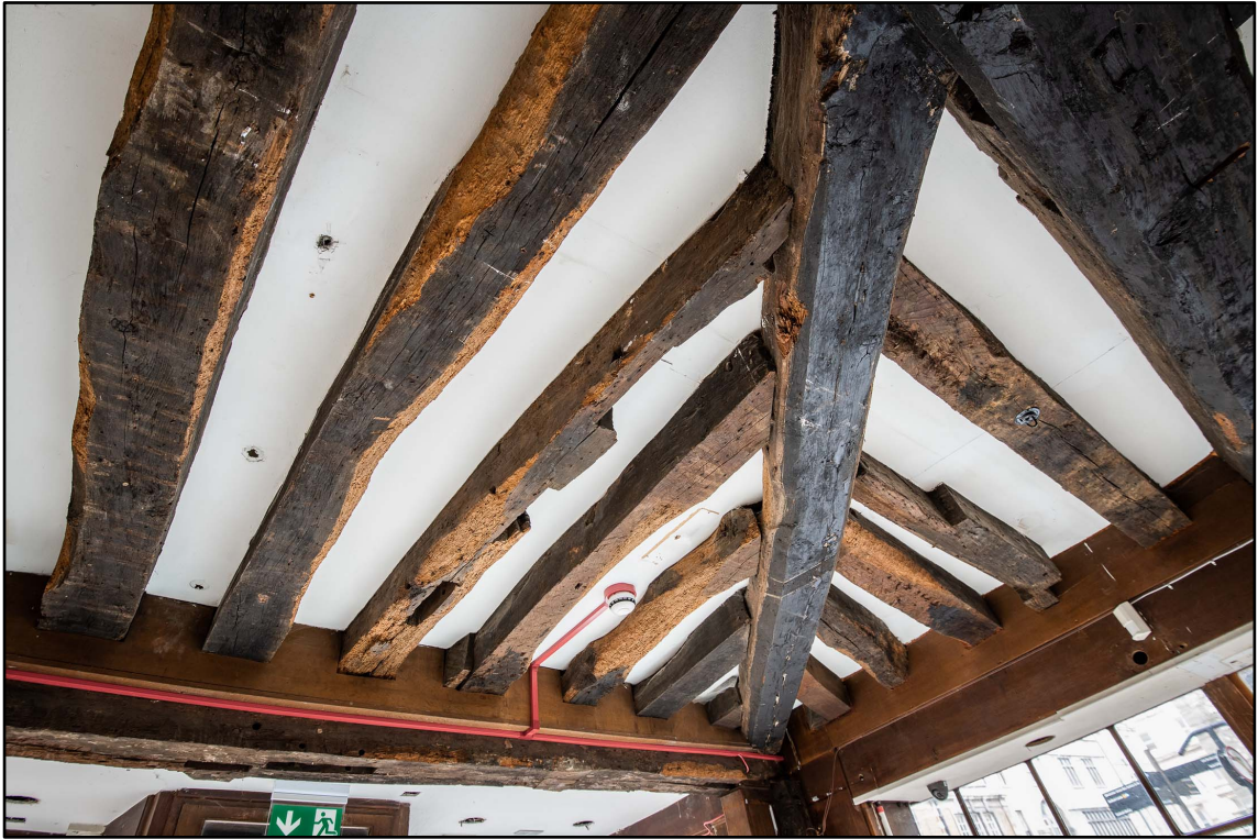
Appendix 3.18: Detail of ceiling beams in GI; note replaced timbers (b/w *Film 2.7)
