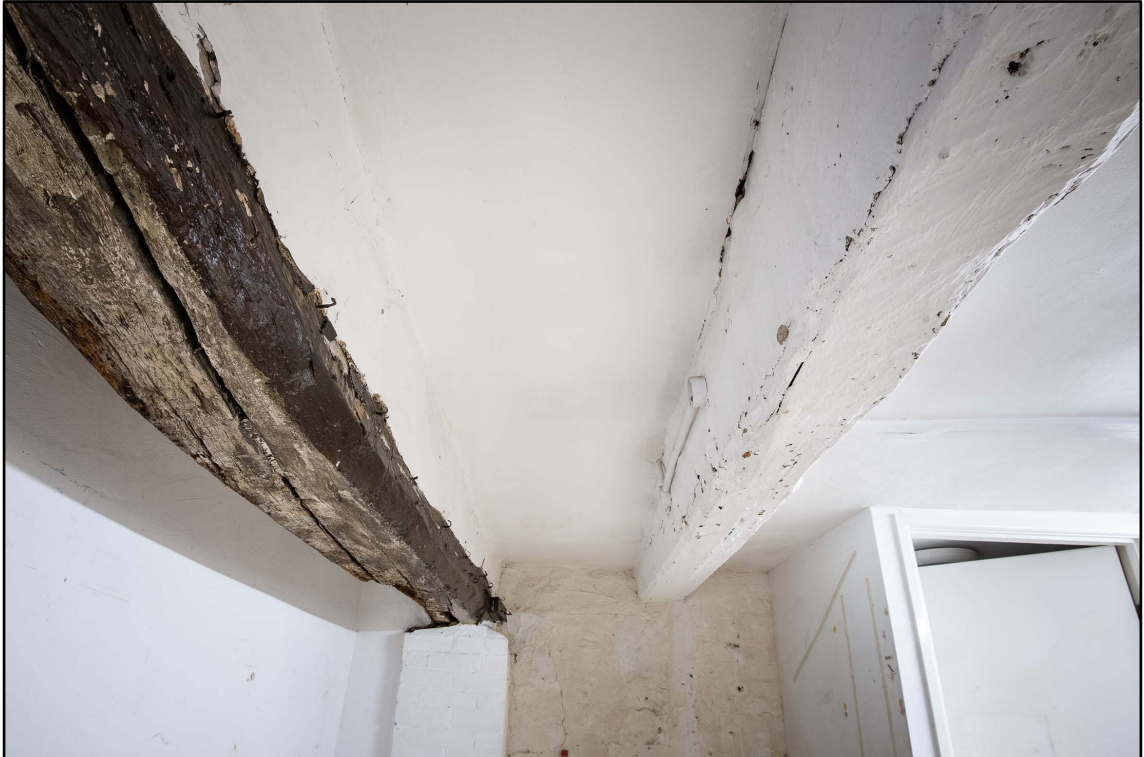
Appendix 3.13: Detail of ceiling beams in CI; note chamfered edges (b/w *Film 3.4)
