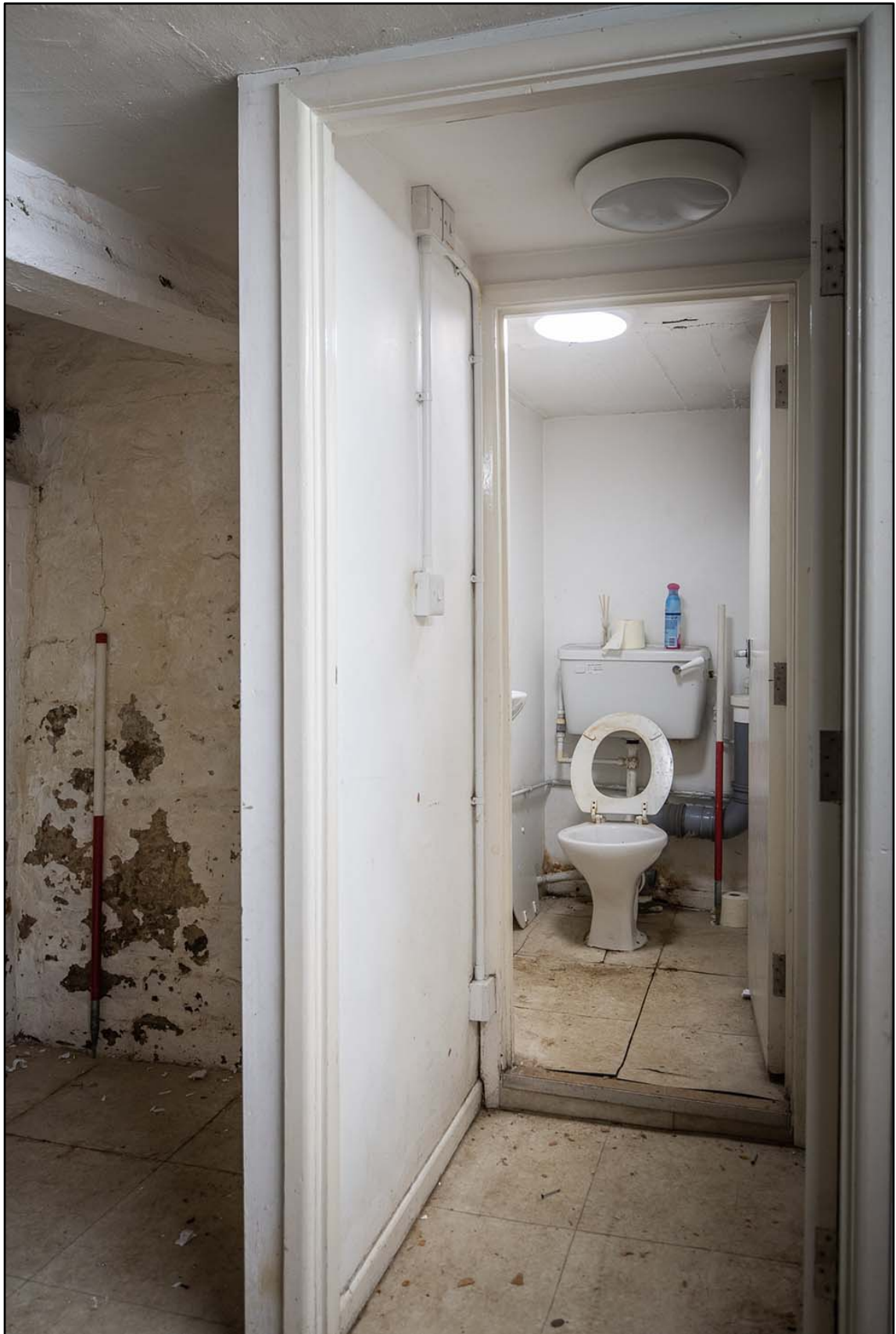
Appendix 3.14: General view of modern toilet in C2 (1m scale; b/w *Film 3.10)
