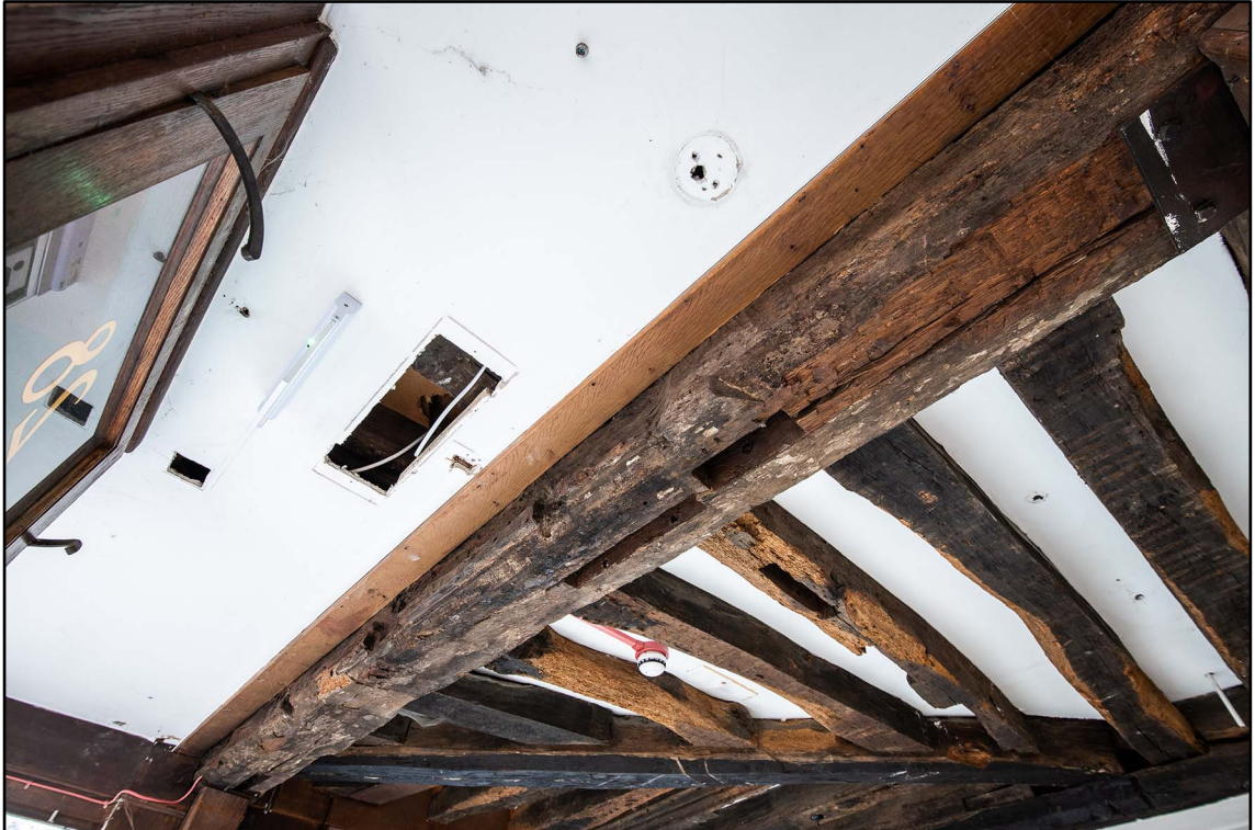
Appendix 3.19: Detail of ceiling beam in shop window of GI, note mortices (b/w *Film 2.9)
