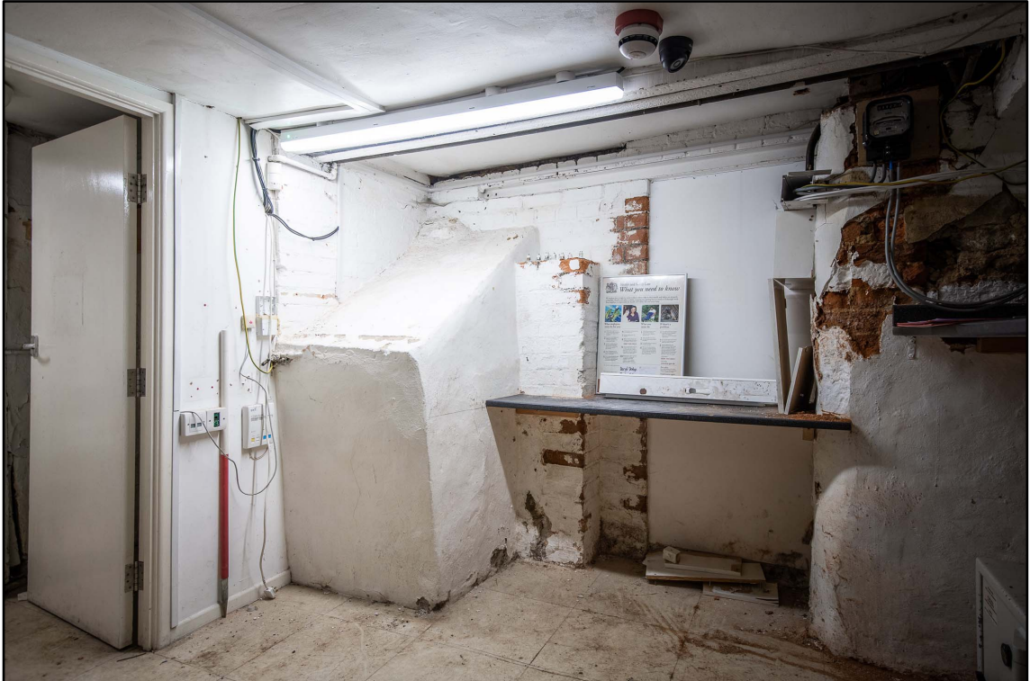
Appendix 3.11: View of CI looking north; note angled buttress (1m scale; b/w *Film 3.8)
