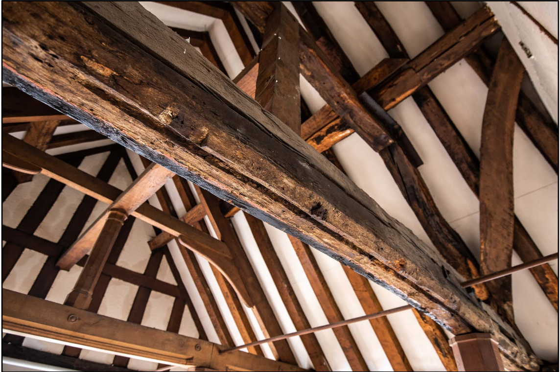
Appendix 3.36: Detail of underside of tie beam in SI; note groove for partition (b/w *Film 1.24)
