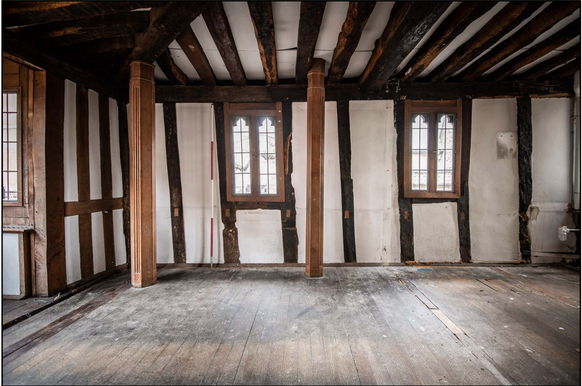
Appendix 3.24: General view of F1, looking north; note 195 l columns (2m scale; b/w *Film 4.6)
