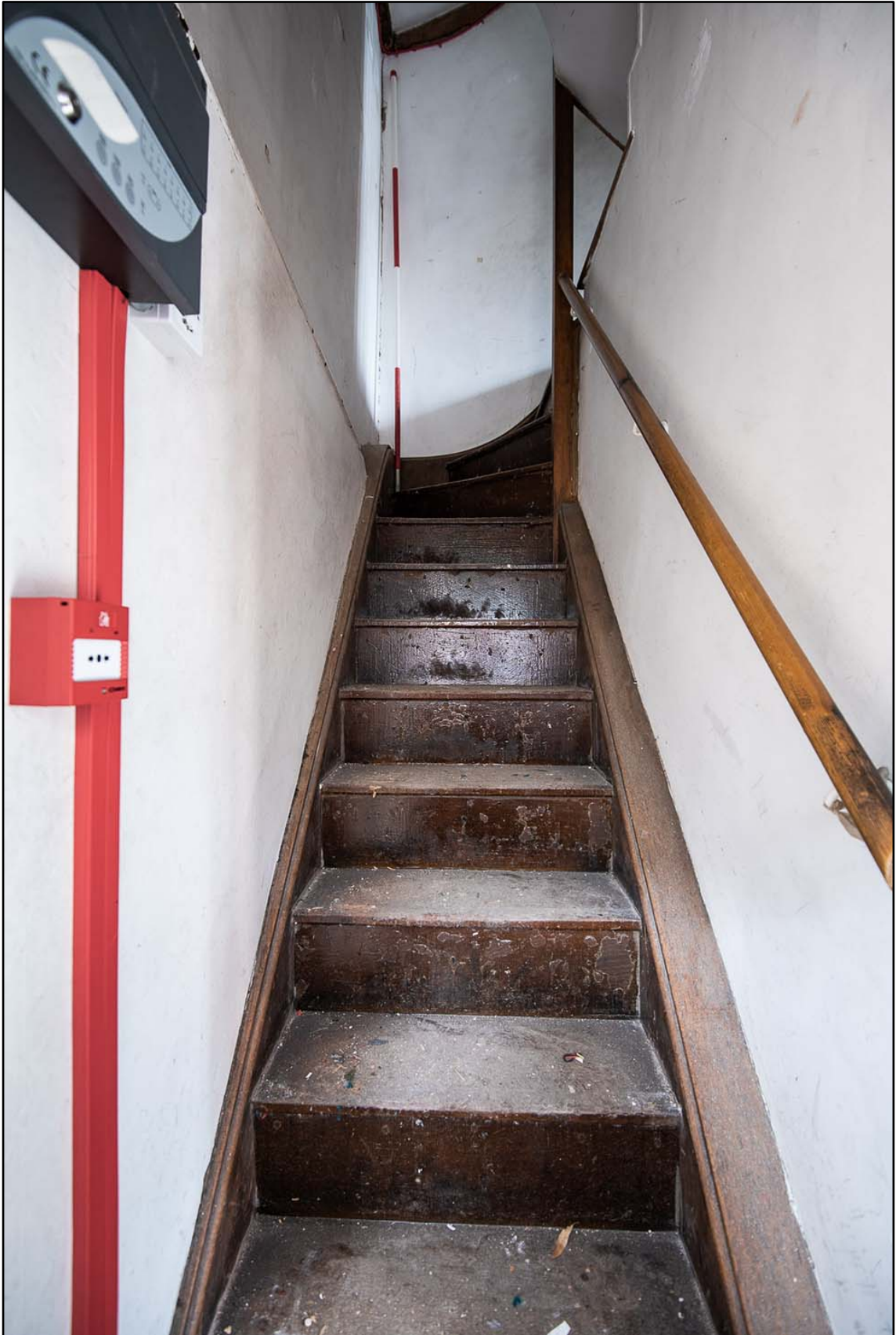
Appendix 3.20: General view of staircase in G2 to first floor (2m scale; b/w *Film 2.11)
