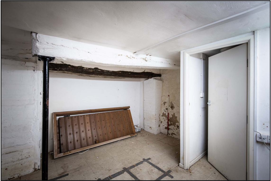
Appendix 3.12: General view of CI looking south; note beams (1m scale; b/w *Film 3.2)
