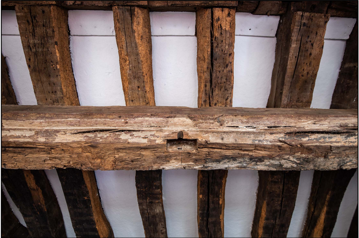
Appendix 3.26: Detail of ceiling beam with mortice for former mullion in F1 (b/w *Film 4.8)
