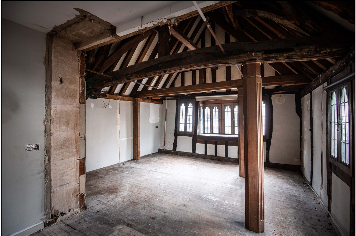
Appendix 3.33: General view of SI, looking south; note 1951 column (2m scale; b/w *Film 5.7)
