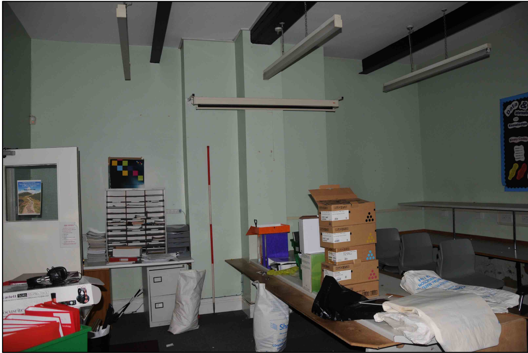
Appendix 2.15: General view of G7 looking south-west; note former chimney breast (2m scale)
