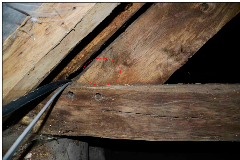
Appendix 2.30: Detail of pegged construction and assembly marks on truss in FI
